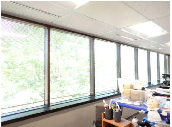
The majority of the interiors of the office suites appeared to be in fair condition at the time of the inspection.
