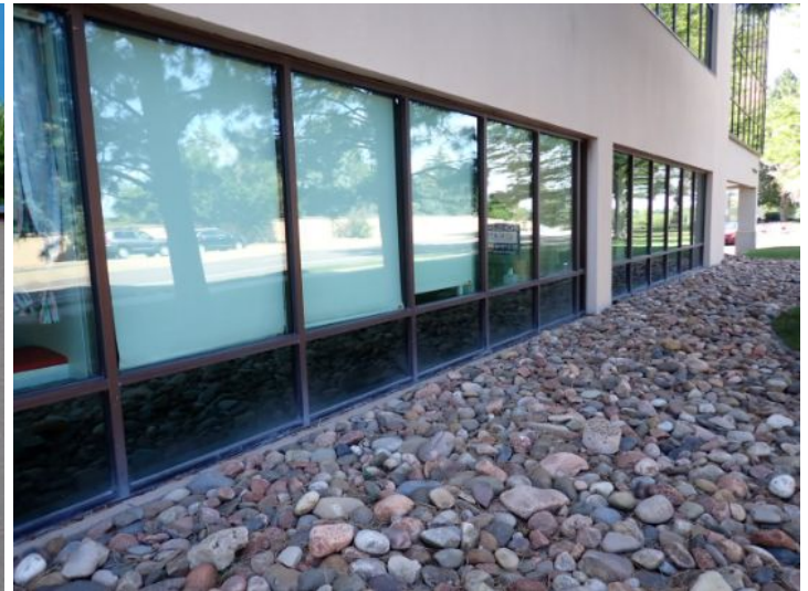
The majority of the exterior envelope of the structure appeared to be in fair condition at the time of the inspection.
