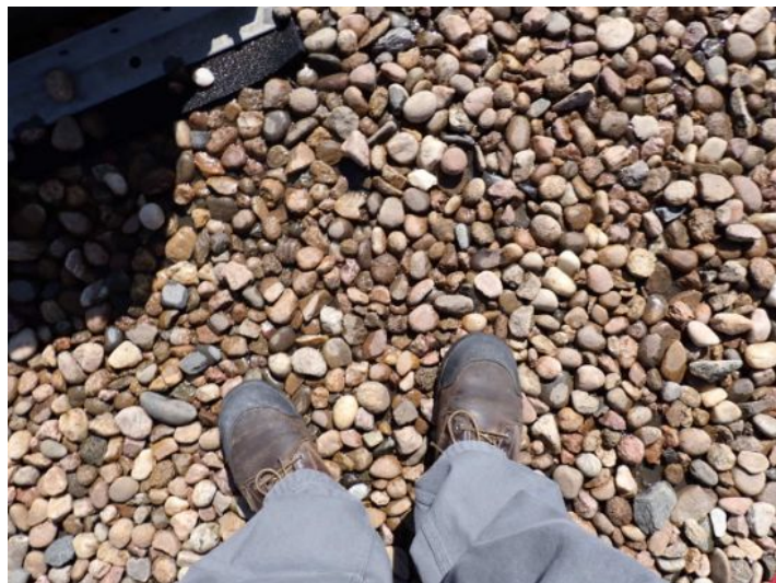
Minor ponding noted in areas. Recommend monitoring for future repairs.
