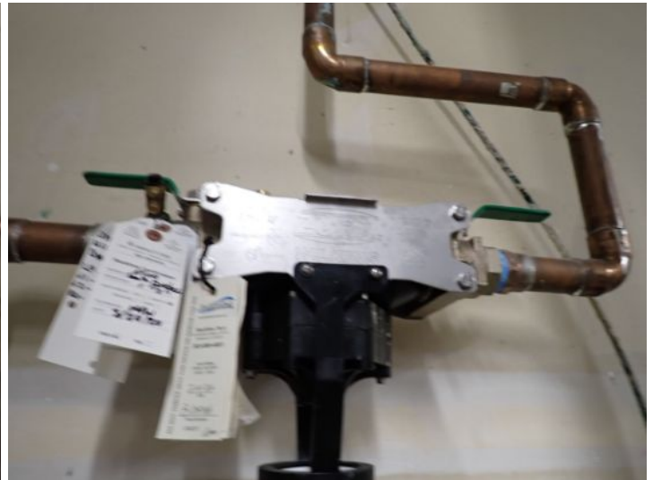
A backflow preventer was installed on the main water supply line at the time of the inspection.
