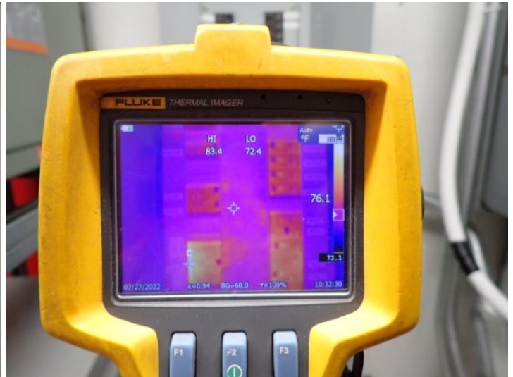
The main electrical panels were scanned with a thermal camera and no abnormalities were noted at the time of the inspection.
