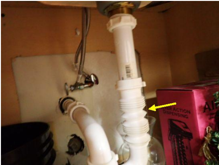
Conference Room (3rd Floor): No GFCI protection noted next to sink. Sub standard plumbing noted below sink. Recommend repairs.
