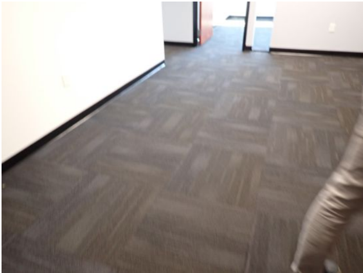
The majority of the interiors of the office suites appeared to be in fair condition at the time of the inspection.
