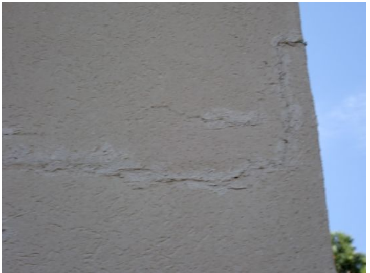
EIFS damage/cracking and past patching noted in areas around the structure. Recommend repairs as needed by a licensed contractor.
