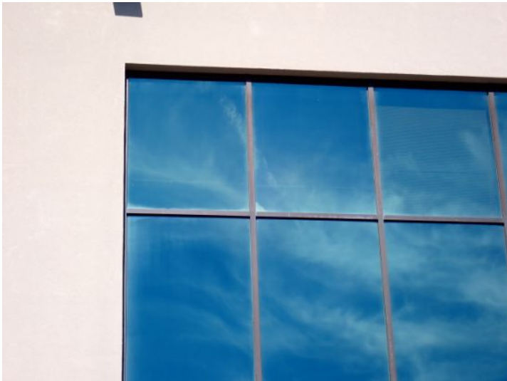
Failed seals noted in one or more insulated window panels at the time of the inspection. Recommend repairs by a licensed contractor.
