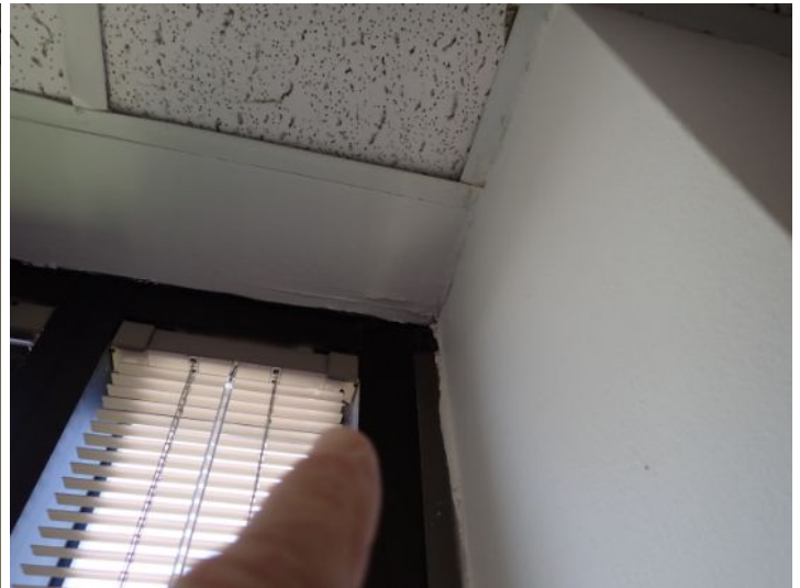
Active moisture intrusion noted in areas of the structure on the outside walls. Recommend having a licensed contractor properly weather proof all of the window systems prior to taking possession of the property.
