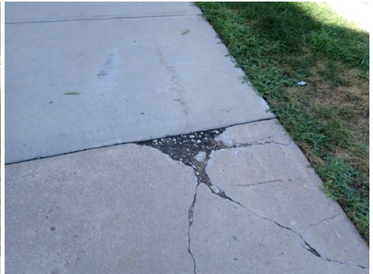
Significant cracking and deterioration noted in areas of the public/city sidewalk system at the time of the inspection. Many municipalities are requiring property owners to maintain the city sidewalks around their property. Recommend repairs as needed by a licensed contractor.
