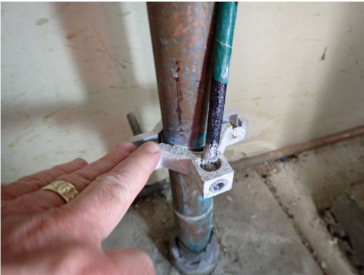
The cold water ground was in place and appeared functional at the time of the inspection.
