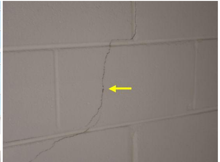
Minor mortar and block cracking noted in the stairwell area at the time of the inspection. Recommend repairs by a licensed contractor.
