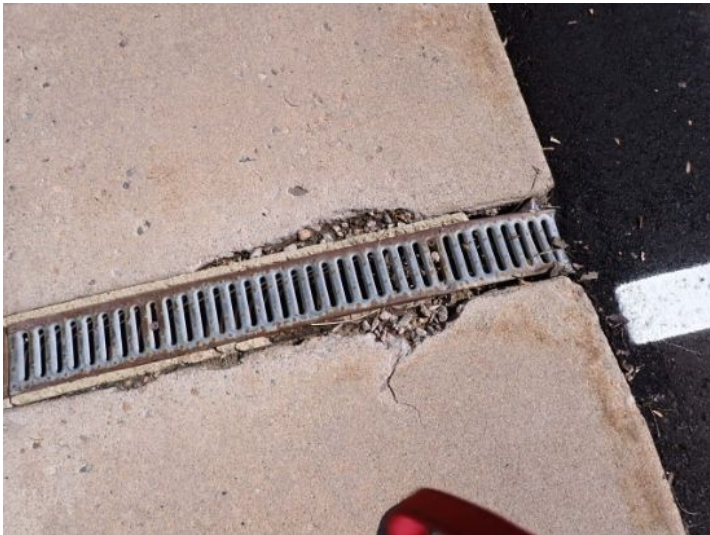
Significant cracking and deterioration noted in areas of the public/city sidewalk system at the time of the inspection. Many municipalities are requiring property owners to maintain the city sidewalks around their property. Recommend repairs as needed by a licensed contractor.
