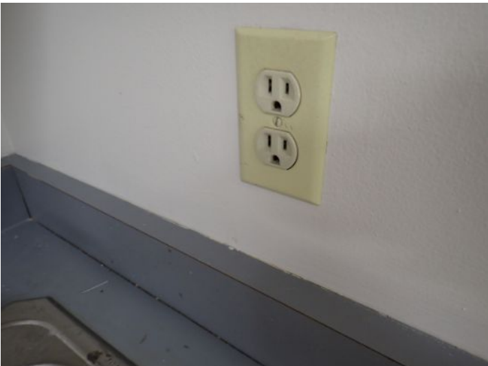
Suite 330: Significant moisture damage noted in the cabinet floor below break area sink. No GFCI protection noted near sink. VCT flooring damage noted. Recommend repairs.
