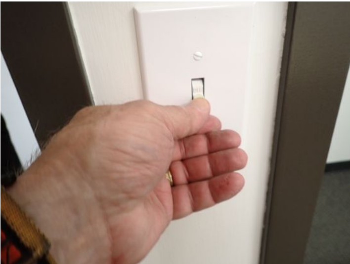
One or more light switches did not appear to operate anything at the time of the inspection. Recommend repairs as needed by a licensed contractor.
