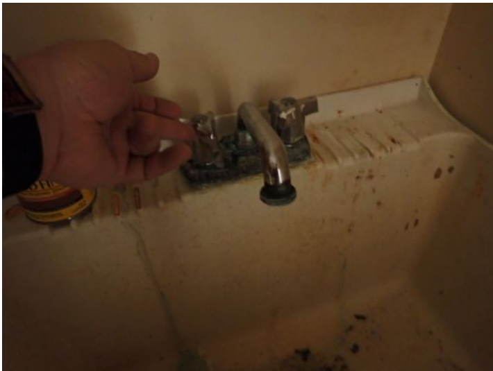
Suite 100: Drywall cracking noted in areas. Sink did not have hot water at the time of the inspection. Recommend repairs.
