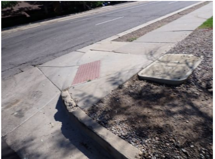
Curbing damage noted in areas. Recommend repairs.
