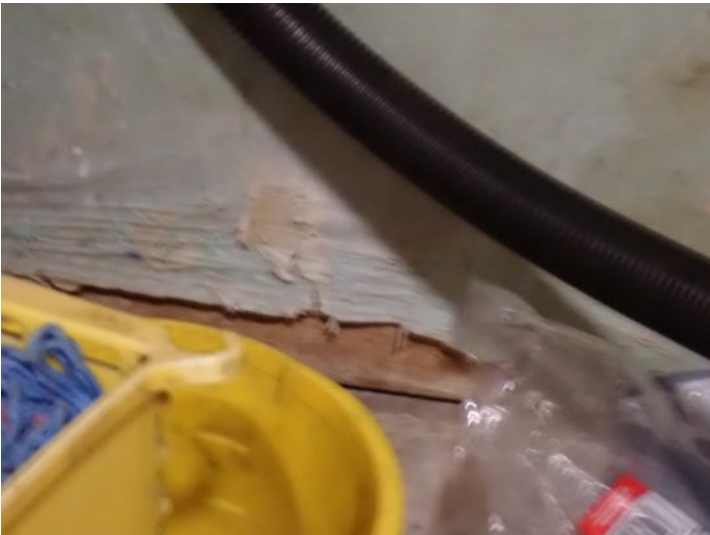
Drywall moisture damage noted in the mop closet on the main level. Recommend repairs by a licensed contractor.
