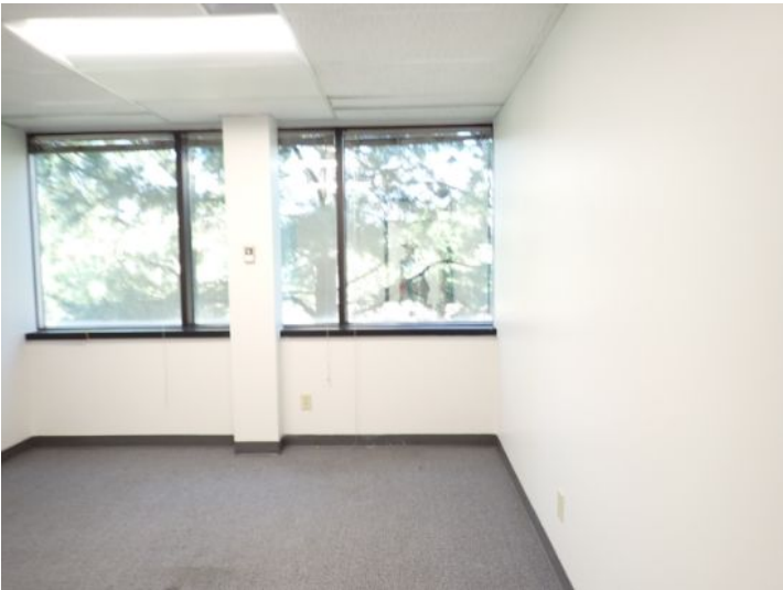
The majority of the interiors of the office suites appeared to be in fair condition at the time of the inspection.
