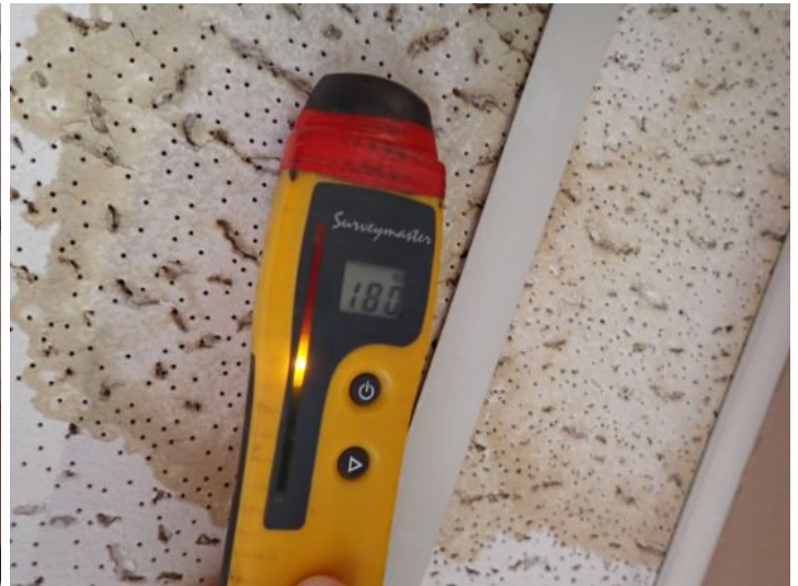
Active moisture intrusion noted in areas of one or more of the suites along the outside walls. Recommend having a licensed contractor properly weather proof all of the window systems prior to taking possession of the property.
