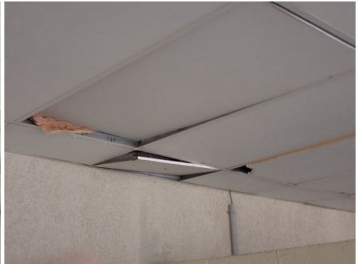
Loose/damaged/missing suspended ceiling tiles noted in areas of the covered parking at the time of the inspection. Recommend repairs.
