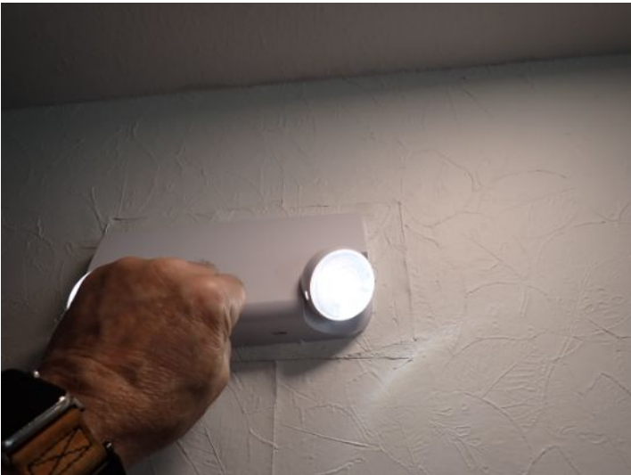
The emergency lighting was tested and functional at the time of the inspection.
