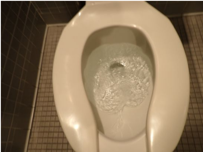
The common restrooms were tested and functional at the time of the inspection.
