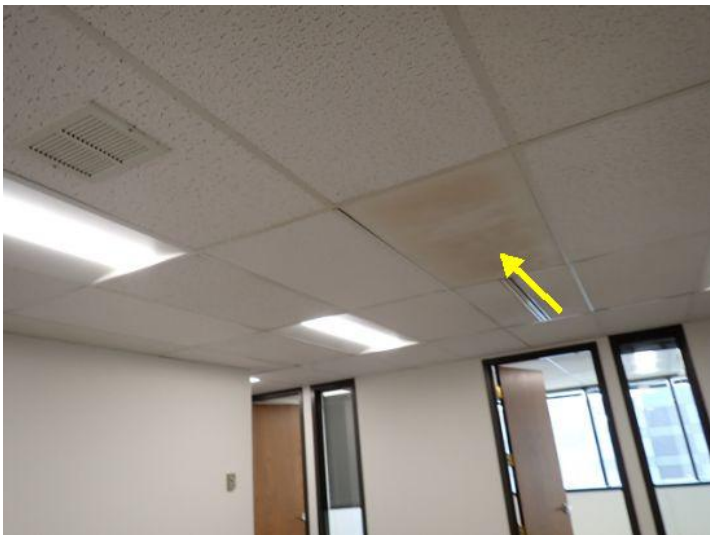
Several of the ceiling mounted radiant heating panels were showing signs of age/wear at the time of the inspection. Recommend repair/replacement as needed by a licensed contractor.
