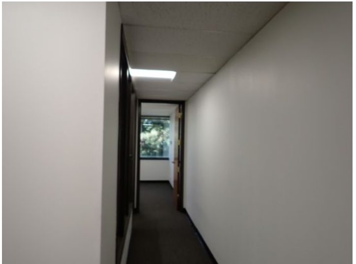
The majority of the interiors of the office suites appeared to be in fair condition at the time of the inspection.
