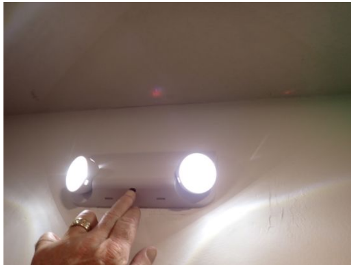
The emergency lighting was tested and functional at the time of the inspection.
