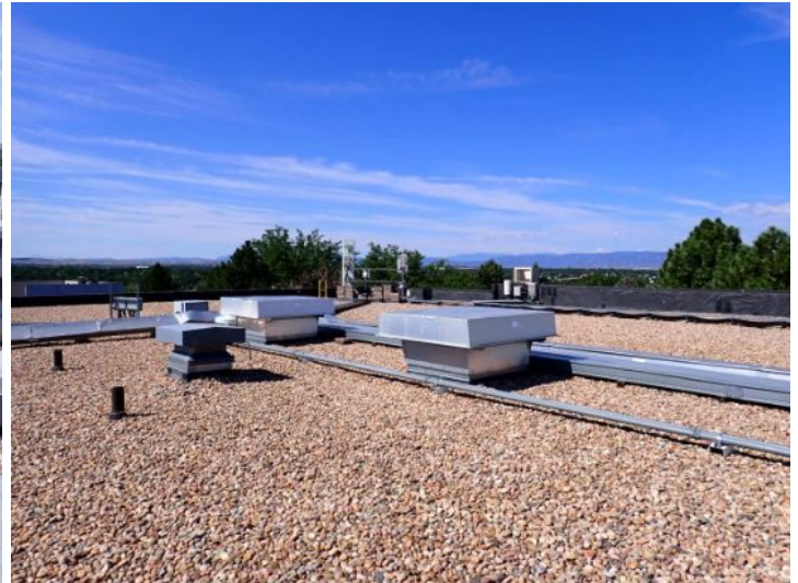
The roofing membrane was last replaced in 2001. The nominal serviceable life expectancy of an EPDM membrane, with proper slope, is 20 years which would be slightly extended with the use of gravel ballast.
