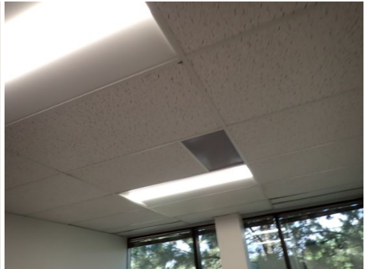
The majority of the interiors of the office suites appeared to be in fair condition at the time of the inspection.
