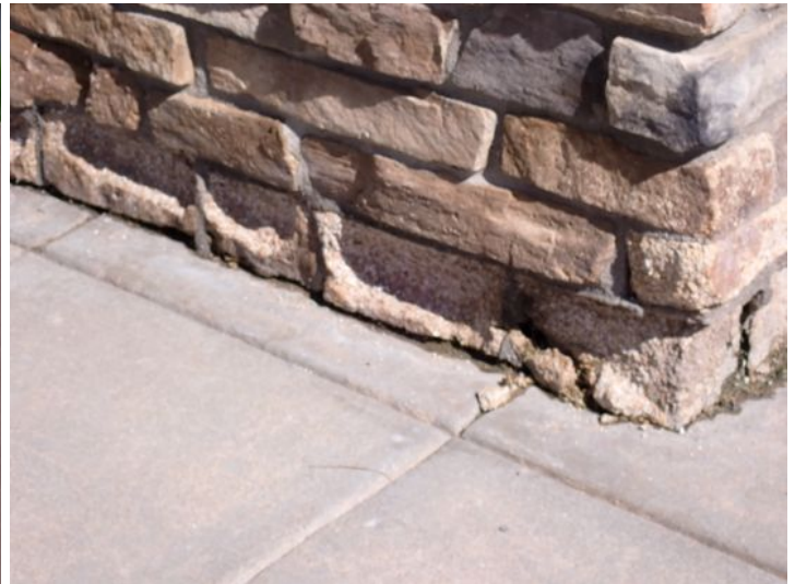
Damaged/deteriorated stone noted around the planting beds at the time of the inspection. Recommend repairs by a licensed contractor.
