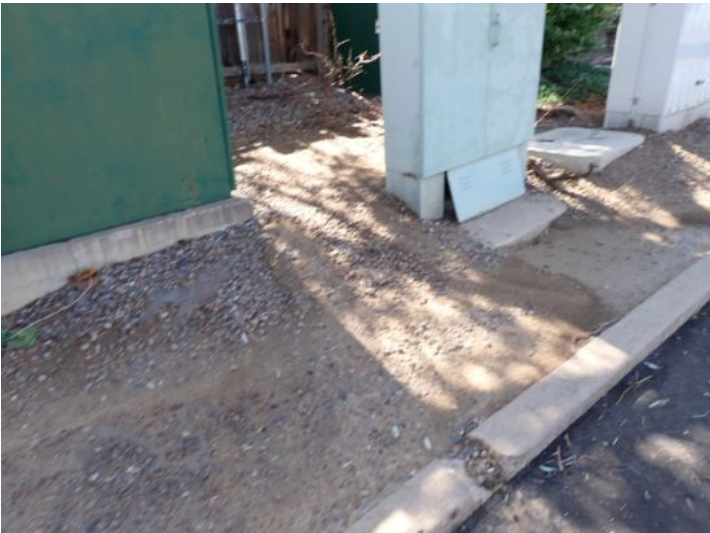
Curbing damage noted in areas. Recommend repairs.
