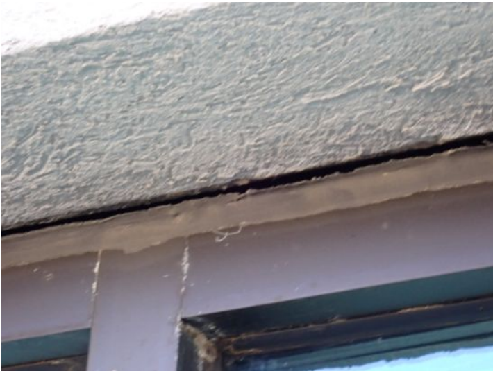
Due to failure of the concrete beam on the west side of the structure the storefront material is settling and pulling away from the structure at the top. Recommend repairs as needed by a licensed contractor.
