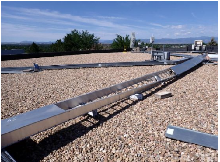
Multiple damaged cable tray systems noted on the roof top at the time of the inspection. Recommend repairs by the cellular contractors to aid in preventing possible membrane damage.
