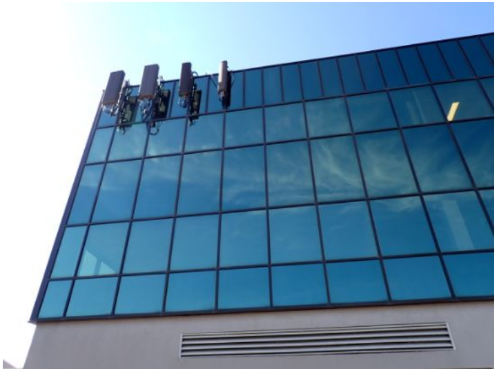
The majority of the exterior envelope of the structure appeared to be in fair condition at the time of the inspection.
