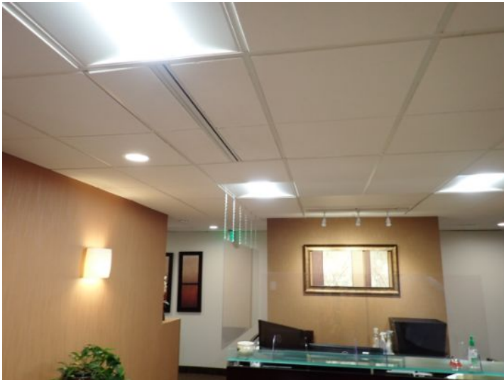
The majority of the interiors of the office suites appeared to be in fair condition at the time of the inspection.
