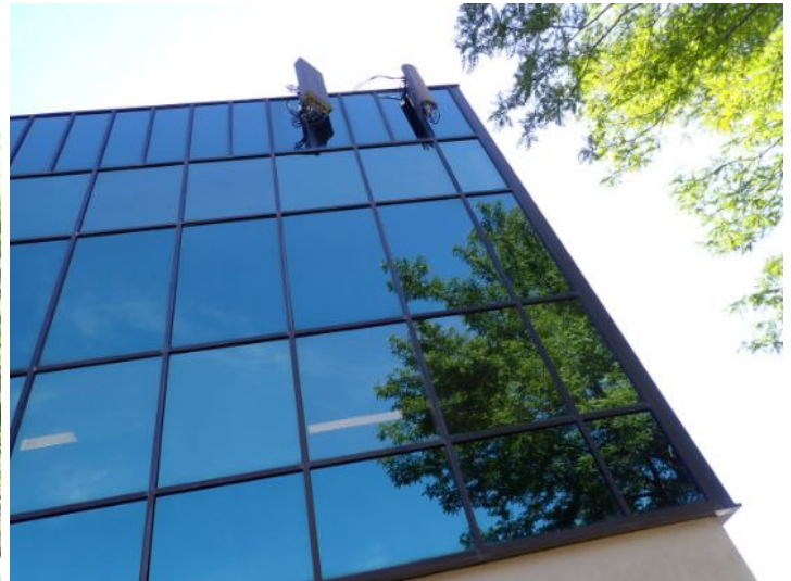
The majority of the exterior envelope of the structure appeared to be in fair condition at the time of the inspection.
