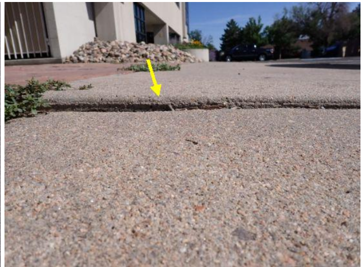
Trip hazards noted. Recommend repairs.
