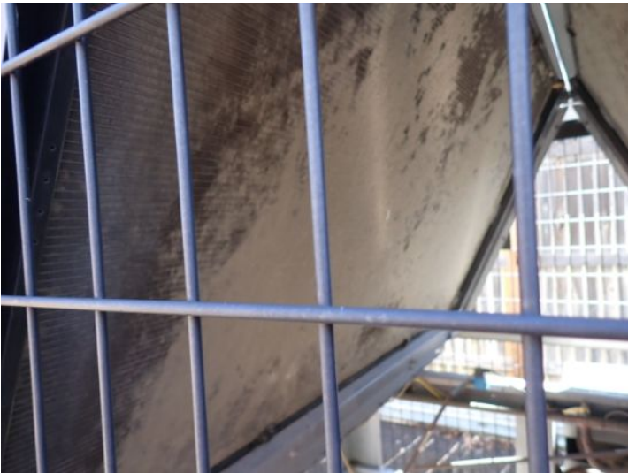
Recommend cleaning/servicing of the a/c chiller system.
