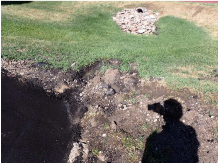
The landscaping requires attention in areas.
