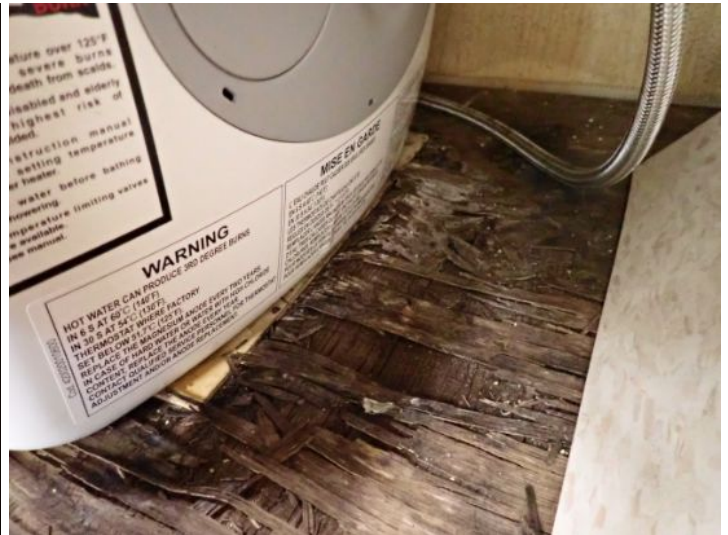
Suite 330: Significant moisture damage noted in the cabinet floor below break area sink. No GFCI protection noted near sink. VCT flooring damage noted. Recommend repairs.
