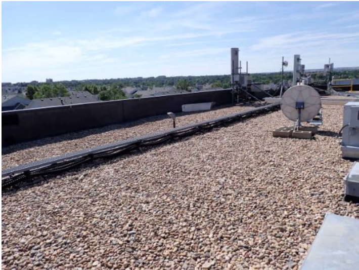
The majority of the roofing system appeared to be in fair condition at the time of the inspection.
