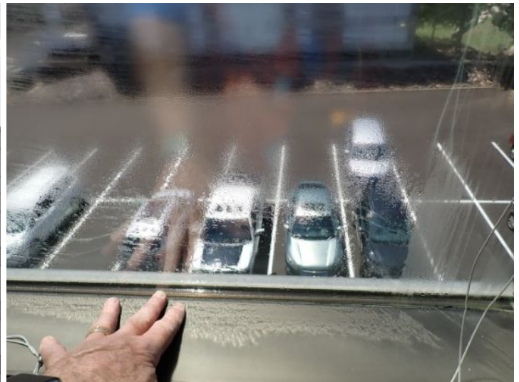
Failed seals noted in one or more insulated window panels at the time of the inspection. Recommend repairs by a licensed contractor.
