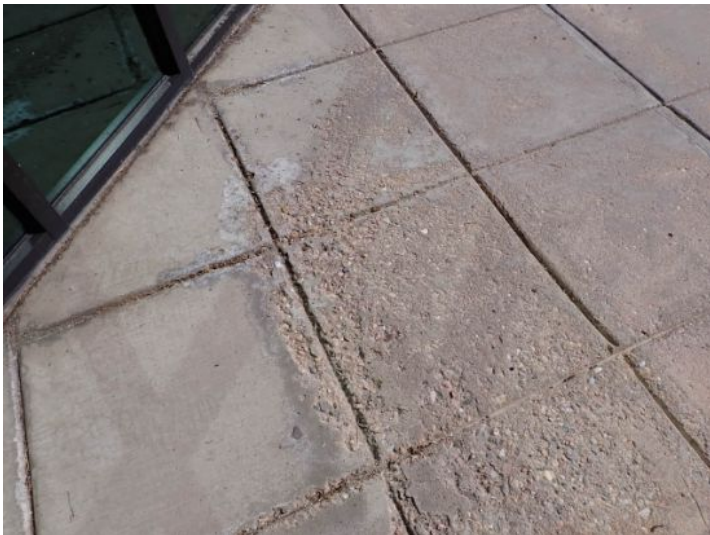
Significant spalling noted on the flatwork on the east side of the structure at the time of the inspection. Recommend repairs by a licensed contractor.
