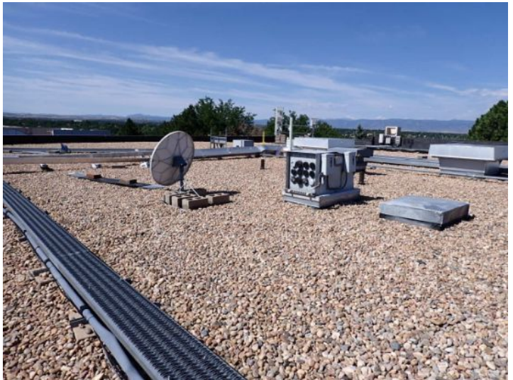
The majority of the roofing system appeared to be in fair condition at the time of the inspection.
