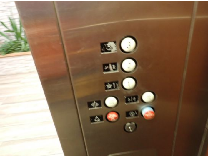
The elevator system was tested and appeared to function properly at the time of the inspection.
