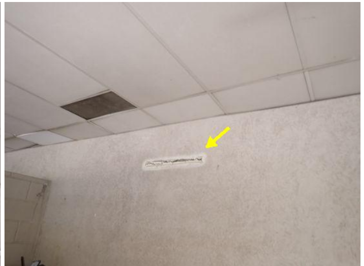
EIFS damage/cracking and past patching noted in areas around the structure. Recommend repairs as needed by a licensed contractor.
