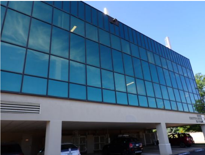
The majority of the exterior envelope of the structure appeared to be in fair condition at the time of the inspection.
