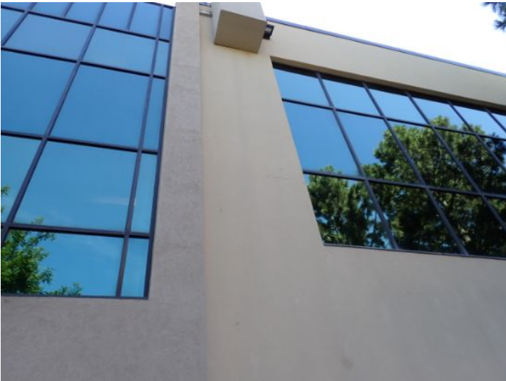
The majority of the exterior envelope of the structure appeared to be in fair condition at the time of the inspection.
