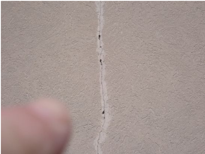
EIFS damage/cracking and past patching noted in areas around the structure. Recommend repairs as needed by a licensed contractor.
