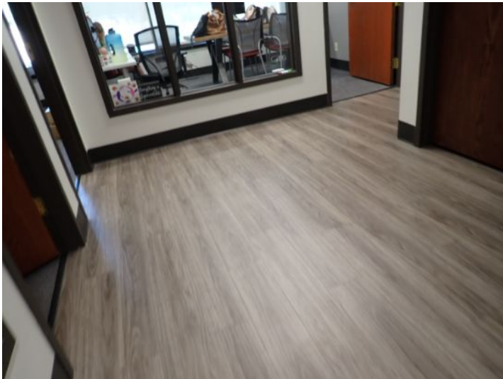
The majority of the interiors of the office suites appeared to be in fair condition at the time of the inspection.
