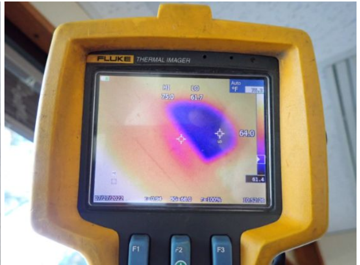
Active moisture intrusion noted in areas of one or more of the suites along the outside walls. Recommend having a licensed contractor properly weather proof all of the window systems prior to taking possession of the property.
