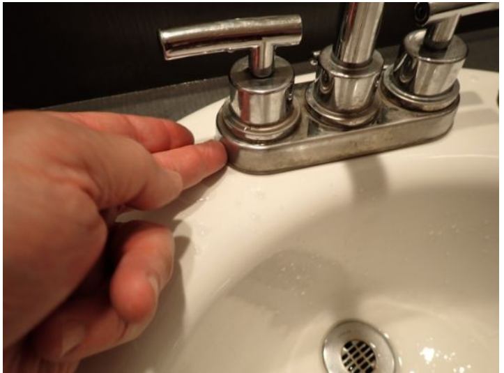
Loose sink faucet noted in the first floors lady's restroom. Recommend repairs.
