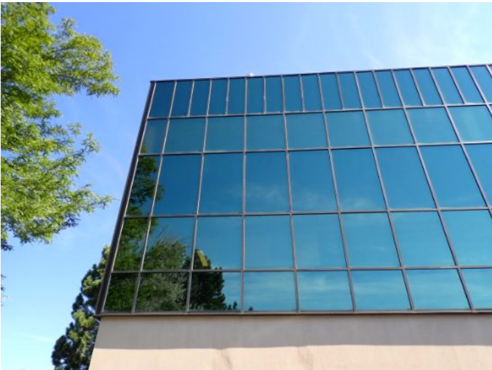
The majority of the exterior envelope of the structure appeared to be in fair condition at the time of the inspection.
