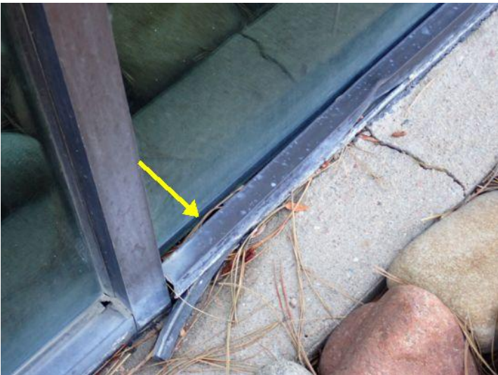
Damaged glass stop noted on the west side bottom of the storefront system at the time of the inspection. Recommend repairs by a licensed contractor.
