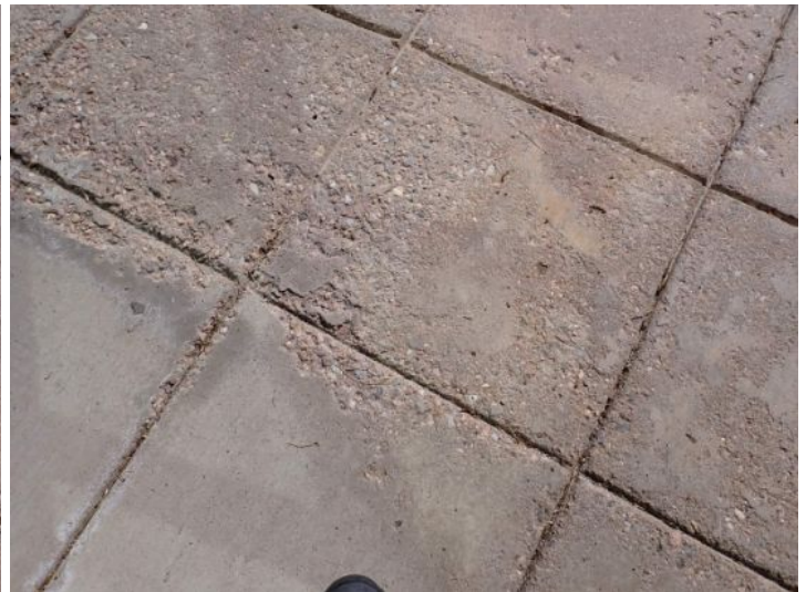
Significant spalling noted on the flatwork on the east side of the structure at the time of the inspection. Recommend repairs by a licensed contractor.
