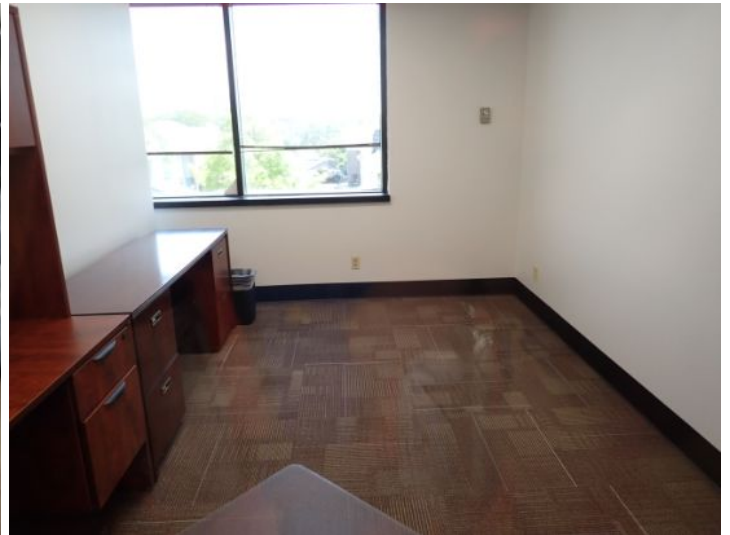
The majority of the interiors of the office suites appeared to be in fair condition at the time of the inspection.
