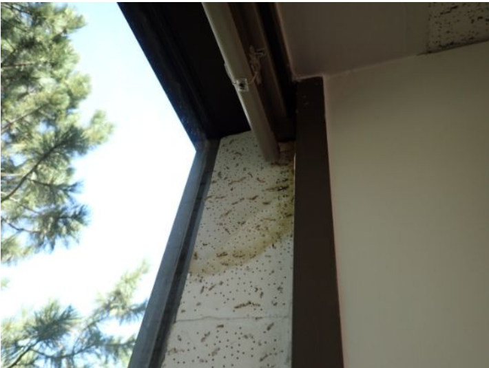
Active moisture intrusion noted in areas of the structure on the outside walls. Recommend having a licensed contractor properly weather proof all of the window systems prior to taking possession of the property.
