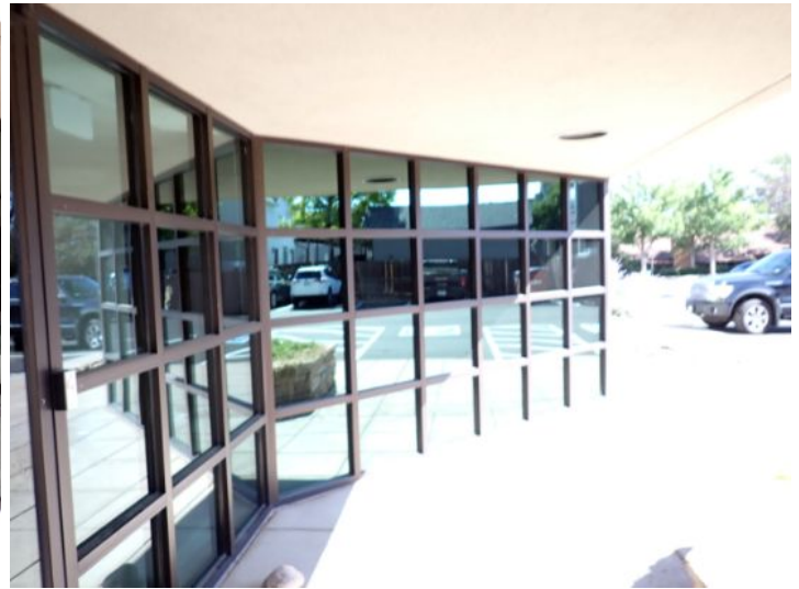
The majority of the exterior envelope of the structure appeared to be in fair condition at the time of the inspection.
