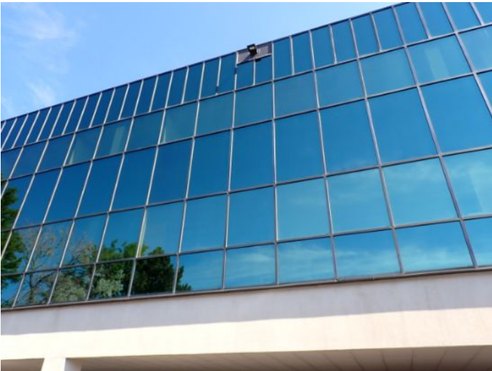
The majority of the exterior envelope of the structure appeared to be in fair condition at the time of the inspection.
