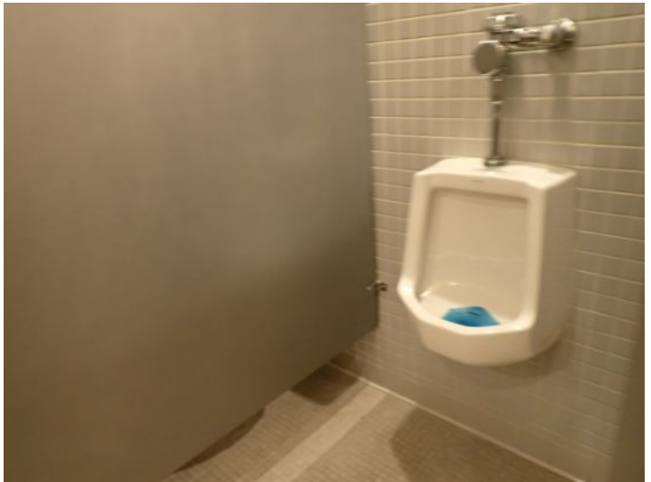
The common restrooms were tested and functional at the time of the inspection.
