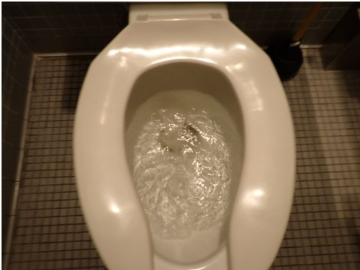
The common restrooms were tested and functional at the time of the inspection.
