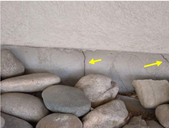
Minor cracking noted in the slab perimeter on the south side of the structure at the time of the inspection. Recommend monitoring for future repairs.
