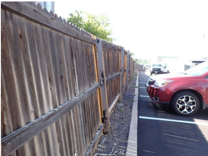
Fencing damage noted on the side of the property at the time of the inspection. Recommend repairs.
