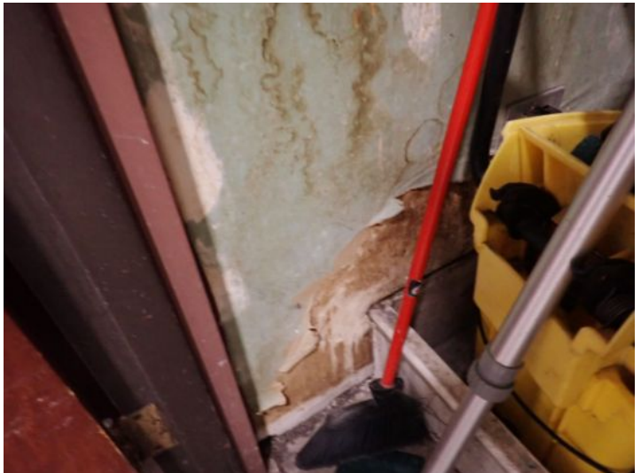
Drywall moisture damage noted in the mop closet on the main level. Recommend repairs by a licensed contractor.
