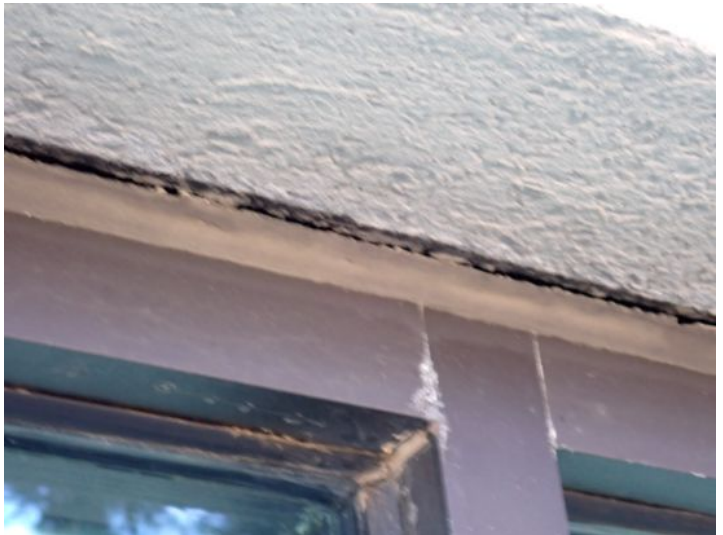
Due to failure of the concrete beam on the west side of the structure the storefront material is settling and pulling away from the structure at the top. Recommend repairs as needed by a licensed contractor.
