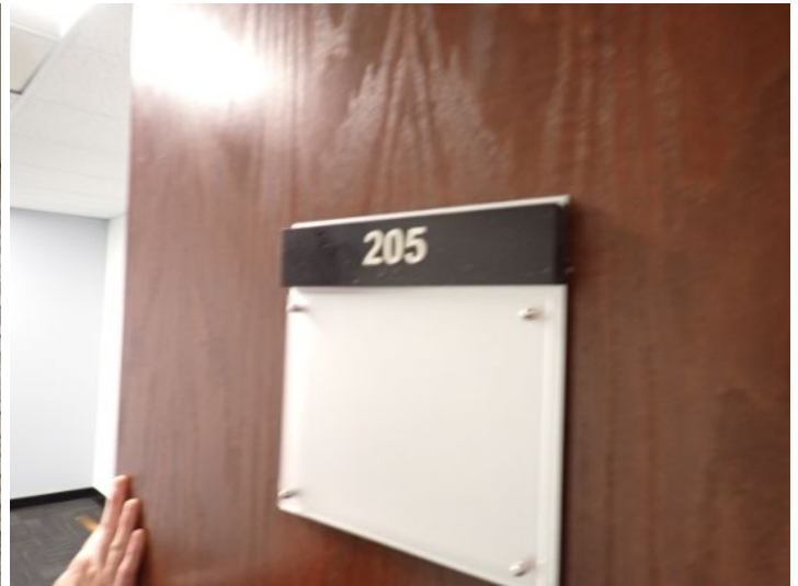
The majority of the interiors of the office suites appeared to be in fair condition at the time of the inspection.
