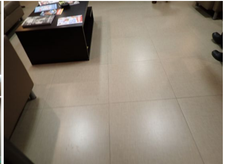
The majority of the interiors of the office suites appeared to be in fair condition at the time of the inspection.
