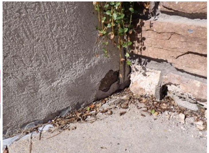
Damaged stucco coating noted on planting beds. Recommend repairs by a licensed contractor.
