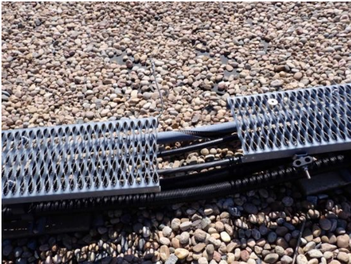
Multiple damaged cable tray systems noted on the roof top at the time of the inspection. Recommend repairs by the cellular contractors to aid in preventing possible membrane damage.
