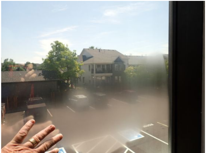
Failed seals noted in one or more insulated window panels at the time of the inspection. Recommend repairs by a licensed contractor.
