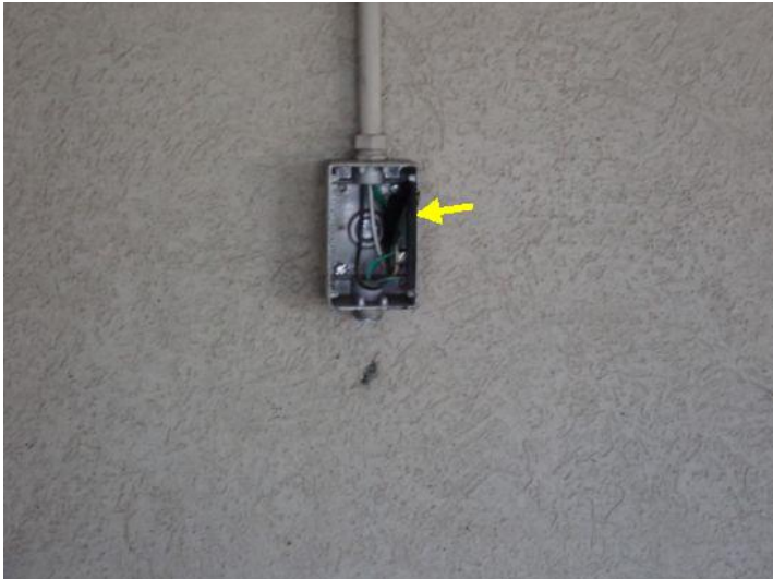
Missing cover and exposed wiring noted on the exterior north side of the structure at the time of the inspection. Recommend repairs.
