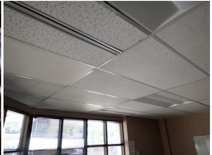
The majority of the interiors of the office suites appeared to be in fair condition at the time of the inspection.
