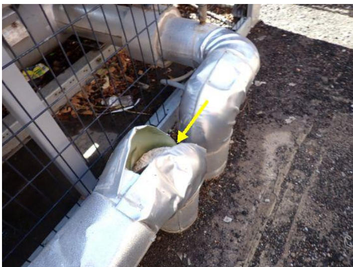
Damaged insulation noted on the cooling lines at the chiller system. Recommend repairs by a licensed contractor.
