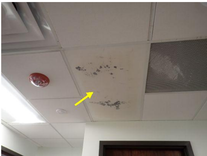
Several of the ceiling mounted radiant heating panels were showing signs of age/wear at the time of the inspection. Recommend repair/replacement as needed by a licensed contractor.
