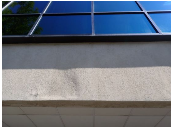
EIFS damage/cracking and past patching noted in areas around the structure. Recommend repairs as needed by a licensed contractor.
