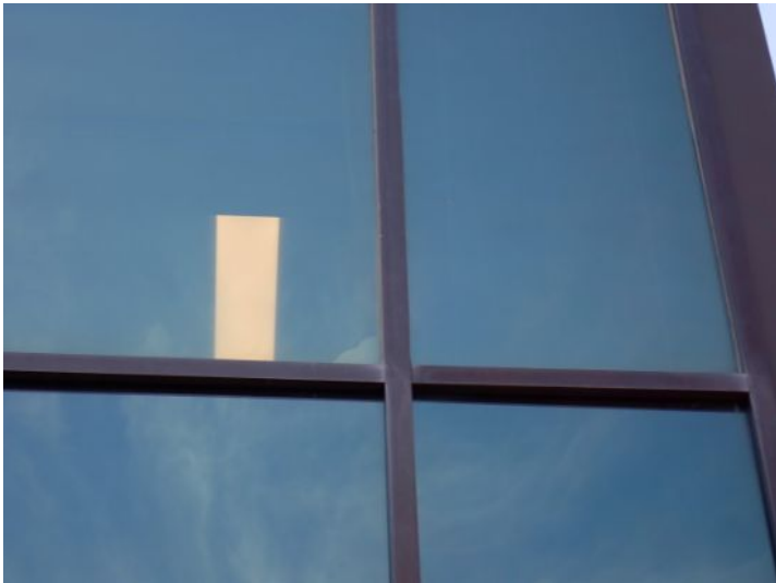
Failed seals noted in one or more insulated window panels at the time of the inspection. Recommend repairs by a licensed contractor.
