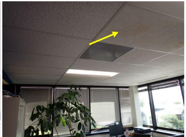
Several of the ceiling mounted radiant heating panels were showing signs of age/wear at the time of the inspection. Recommend repair/replacement as needed by a licensed contractor.
