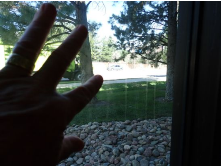
Failed seals noted in one or more insulated window panels at the time of the inspection. Recommend repairs by a licensed contractor.
