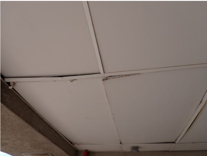
Loose/damaged/missing suspended ceiling tiles noted in areas of the covered parking at the time of the inspection. Recommend repairs.
