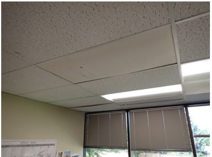
The majority of the interiors of the office suites appeared to be in fair condition at the time of the inspection.
