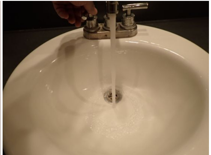
The common restrooms were tested and functional at the time of the inspection.
