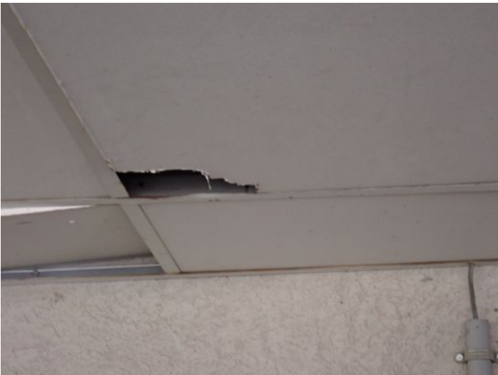
Loose/damaged/missing suspended ceiling tiles noted in areas of the covered parking at the time of the inspection. Recommend repairs.
