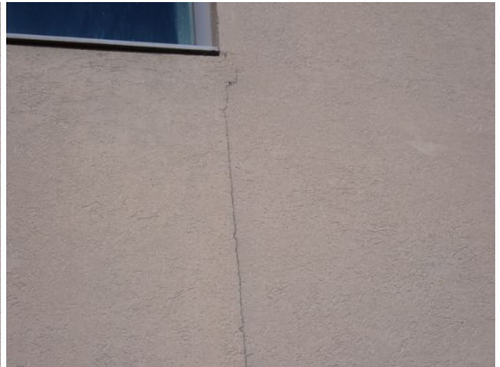
EIFS damage/cracking and past patching noted in areas around the structure. Recommend repairs as needed by a licensed contractor.
