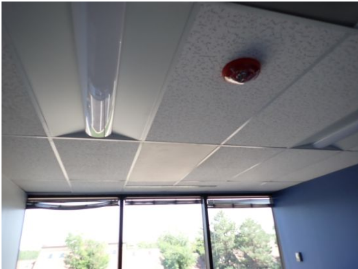
The majority of the interiors of the office suites appeared to be in fair condition at the time of the inspection.
