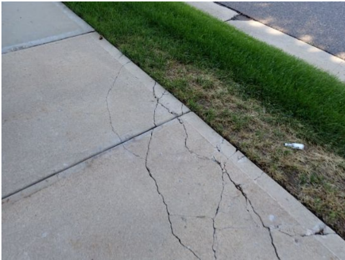
Significant cracking and deterioration noted in areas of the public/city sidewalk system at the time of the inspection. Many municipalities are requiring property owners to maintain the city sidewalks around their property. Recommend repairs as needed by a licensed contractor.
