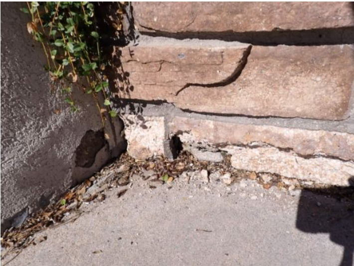
Damaged/deteriorated stone noted around the planting beds at the time of the inspection. Recommend repairs by a licensed contractor.
