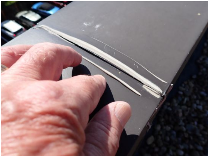
Recommend sealant repairs on parapet wall cap seams. Recommend repairs by a licensed contractor.
