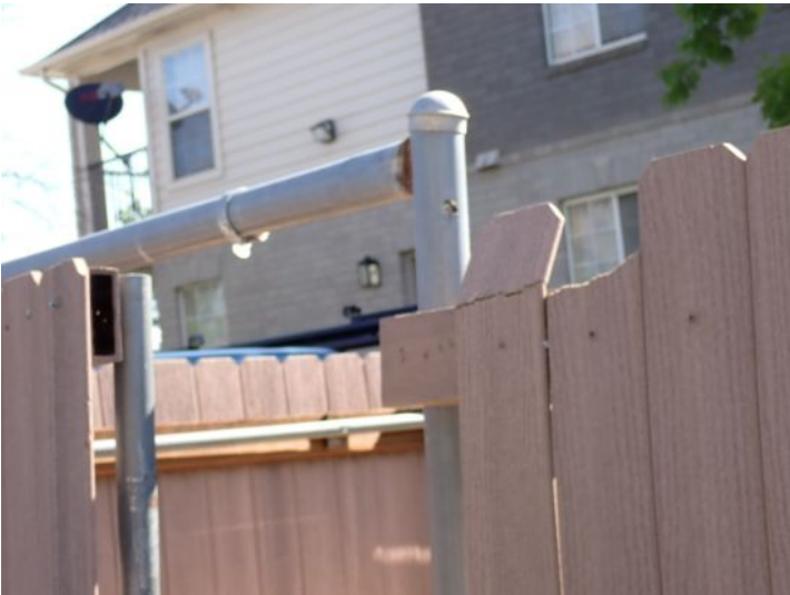
The fencing enclosure for the chiller system was in poor condition at the time of the inspection. Recommend repairs
