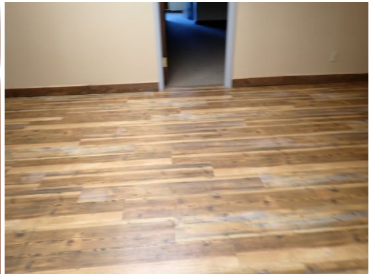
The majority of the interiors of the office suites appeared to be in fair condition at the time of the inspection.
