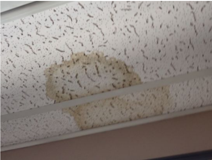
Active moisture intrusion noted in areas of one or more of the suites along the outside walls. Recommend having a licensed contractor properly weather proof all of the window systems prior to taking possession of the property.
