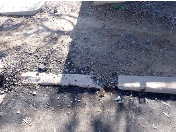
Curbing damage noted in areas. Recommend repairs.
