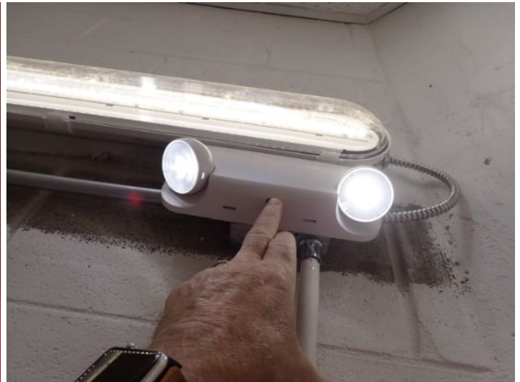
The emergency lighting was tested and functional at the time of the inspection.
