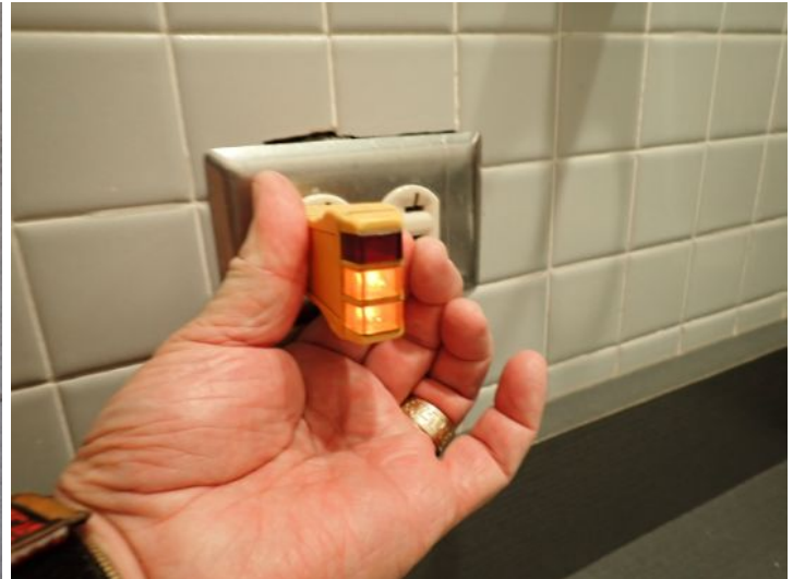
No GFCI protection for the restroom(s) at the time of the inspection. Recommend repairs by a licensed electrician.
