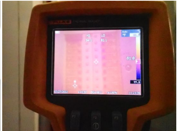
The main electrical panels were scanned with a thermal camera and no abnormalities were noted at the time of the inspection.
