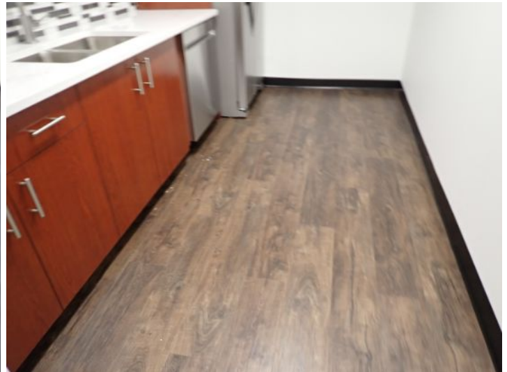
The majority of the interiors of the office suites appeared to be in fair condition at the time of the inspection.
