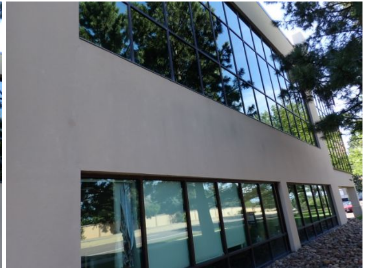
The majority of the exterior envelope of the structure appeared to be in fair condition at the time of the inspection.
