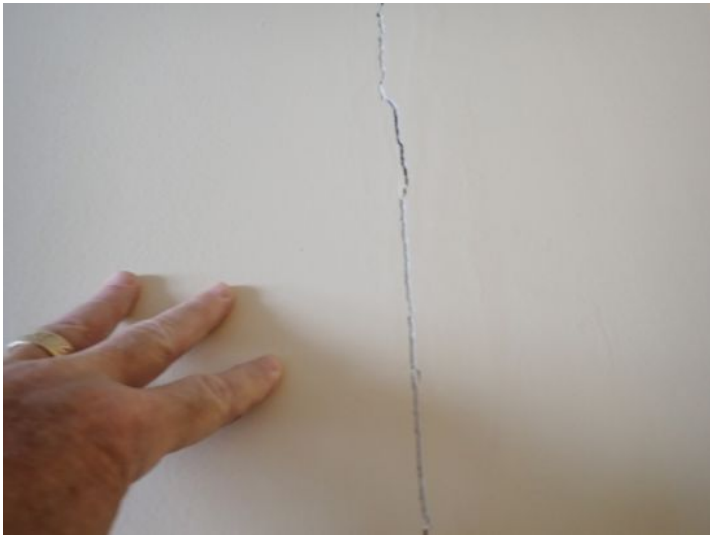
Suite 100: Drywall cracking noted in areas. Sink did not have hot water at the time of the inspection. Recommend repairs.
