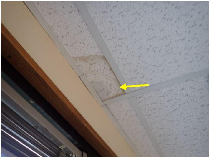
Active moisture intrusion noted in areas of one or more of the suites along the outside walls. Recommend having a licensed contractor properly weather proof all of the window systems prior to taking possession of the property.
