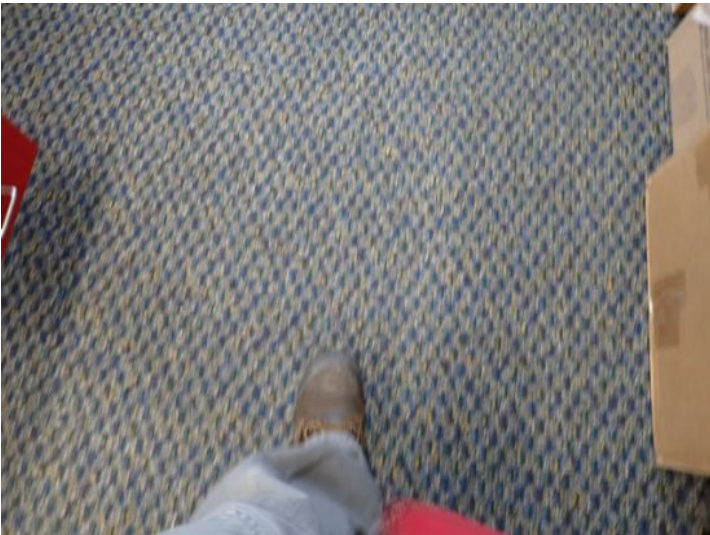
Flooring deflection noted under foot in areas. Recommend monitoring for future repairs.
