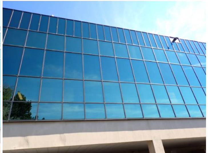
The majority of the exterior envelope of the structure appeared to be in fair condition at the time of the inspection.
