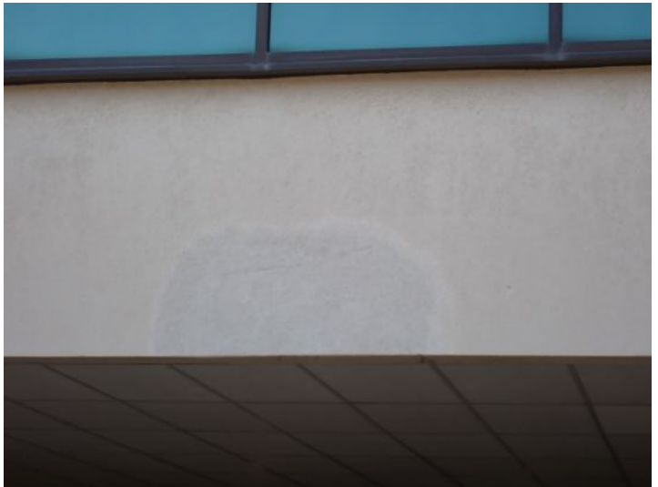
EIFS damage/cracking and past patching noted in areas around the structure. Recommend repairs as needed by a licensed contractor.
