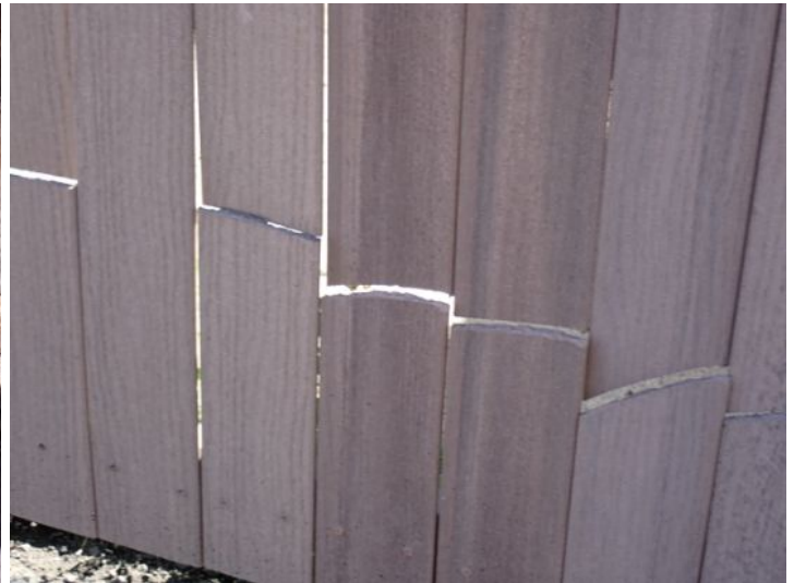
The fencing enclosure for the chiller system was in poor condition at the time of the inspection. Recommend repairs
