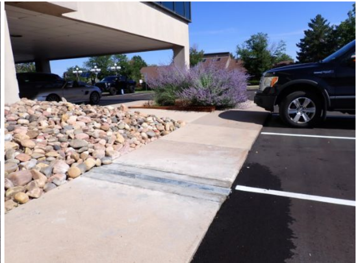
Missing ADA ramps noted where the ADA parking was designated and the main entrance to the building was located. Recommend repairs by a licensed contractor.
