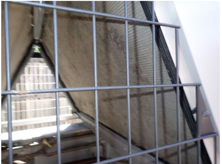
Recommend cleaning/servicing of the a/c chiller system.
