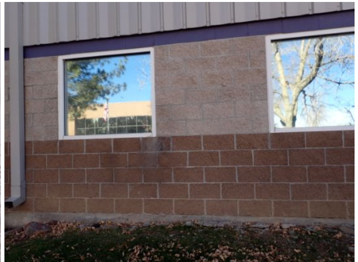
The majority of the exterior envelope of the structure appeared to be in fair condition with no significant movement noted at the time of the inspection.
