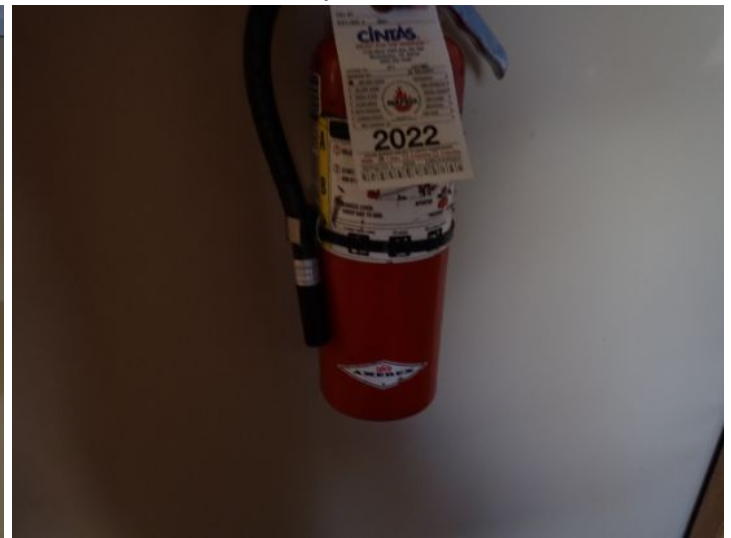
Last date of inspection/certification for the fire extinguishers was 7/22.
