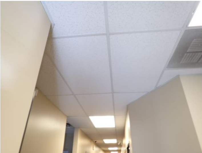
The majority of the interior of the office area appeared to be in fair condition at the time of the inspection.
