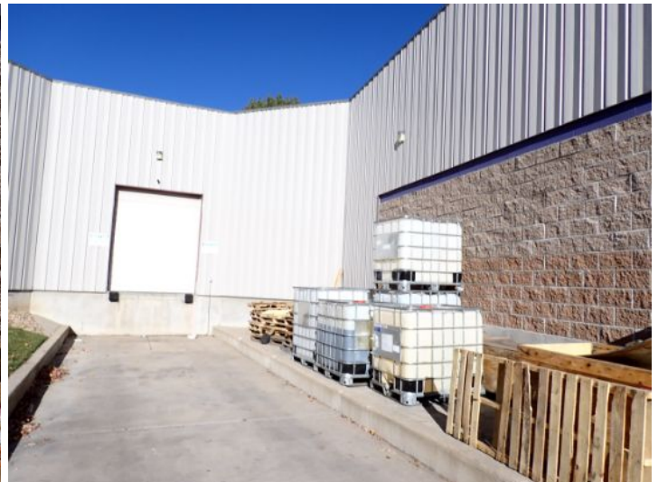
The majority of the exterior envelope of the structure appeared to be in fair condition with no significant movement noted at the time of the inspection.
