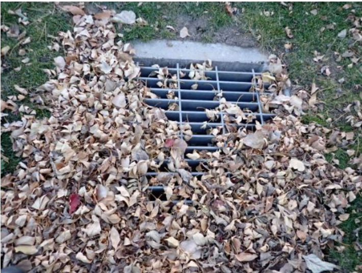
There were storm water catch basins located on the property at the time of the inspection.
