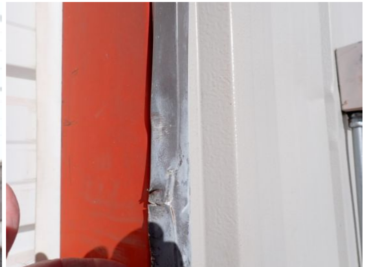
Minor steel trim damage noted around one or more of the overhead doors at the time of the inspection. Recommend repairs by a licensed contractor.
