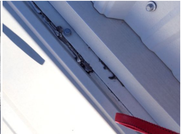
Sealant/repairs noted in areas along the parapet walls of the roofing system. At the time of the inspection the sealant appeared to have reached or be nearing its serviceable life expectancy. Recommend repairs as needed by a licensed contractor.
