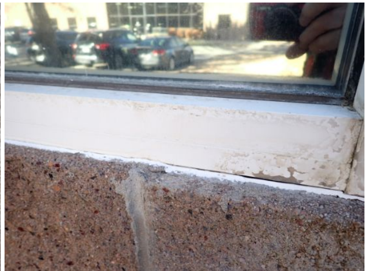
Recommend assuring that any area where two separate substrates meet be properly caulked/sealed. Recommend repairs by a licensed contractor.
