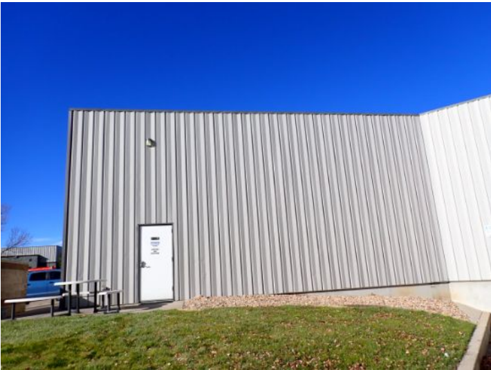
The majority of the exterior envelope of the structure appeared to be in fair condition with no significant movement noted at the time of the inspection.
