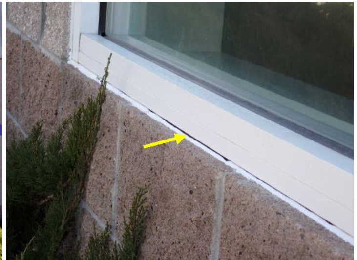
Recommend assuring that any area where two separate substrates meet be properly caulked/sealed. Recommend repairs by a licensed contractor.
