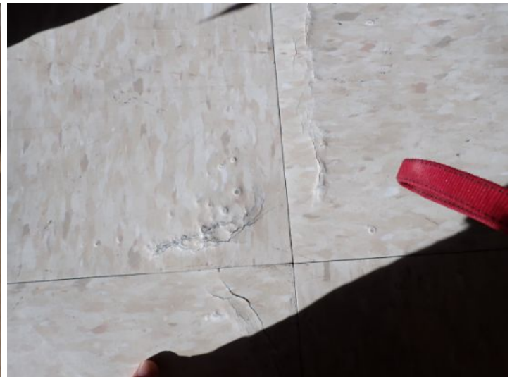
VCT flooring damage noted in the main entry area. Recommend repairs as needed by a licensed contractor.
