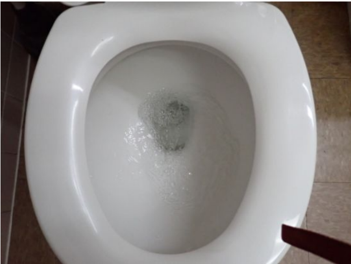
The restroom facilities were tested and functional at the time of the inspection.
