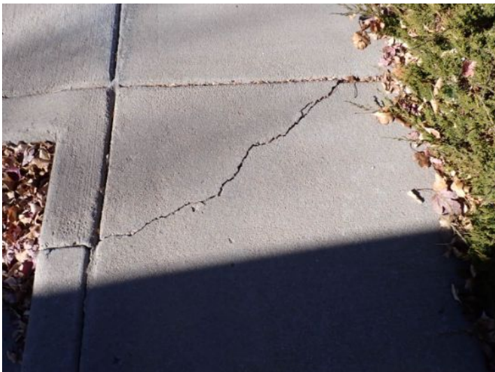
Minor cracking. Recommend monitoring for future repairs.
