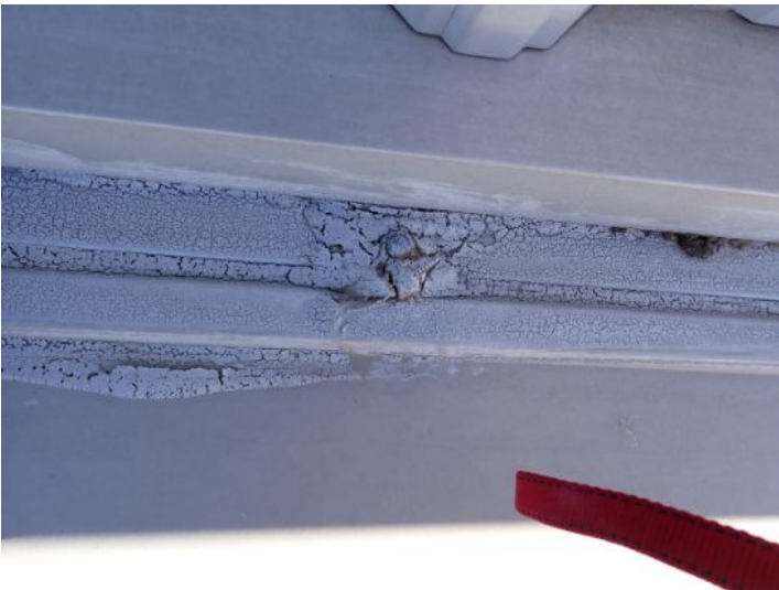
Sealant/repairs noted in areas along the parapet walls of the roofing system. At the time of the inspection the sealant appeared to have reached or be nearing its serviceable life expectancy. Recommend repairs as needed by a licensed contractor.
