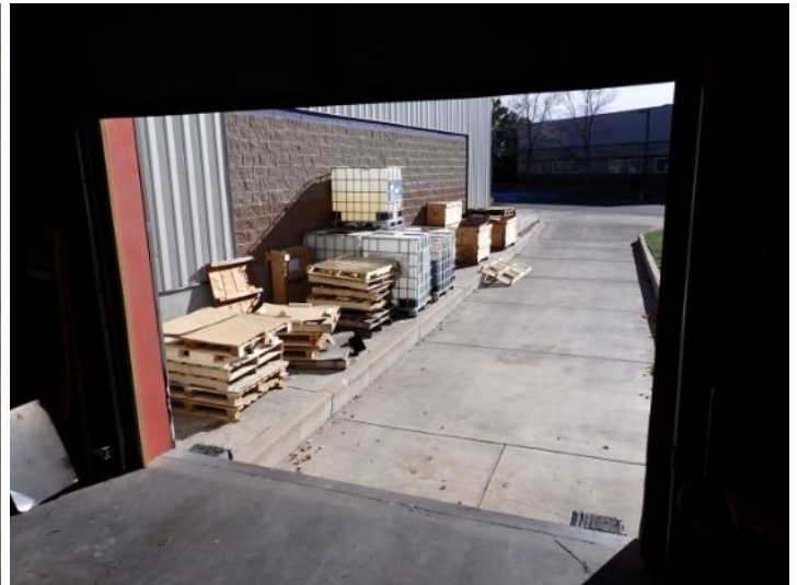
The overhead doors and personnel doors were tested and functional at the time of the inspection.
