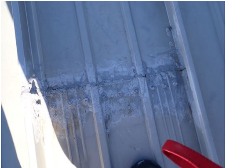
Past repairs/sealant noted in areas of the roofing system. At the time of the inspection the sealant appeared to be nearing failure. Recommend repairs as needed by a licensed contractor.
