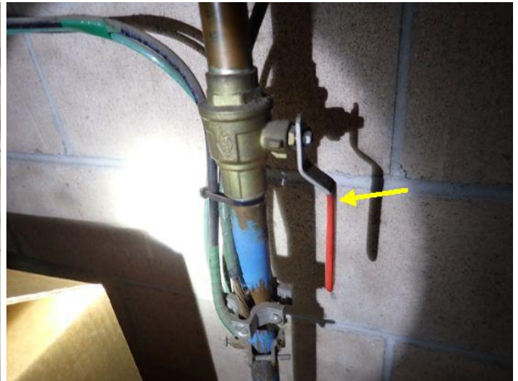
The main water shut off valve was functional at the time of the inspection.
