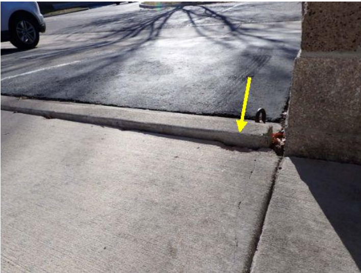
Trip hazards noted. Recommend repairs.
