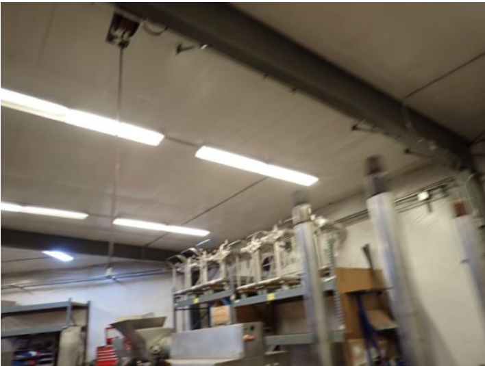
The majority of the interior of the warehouse area appeared to be in fair condition at the time of the inspection.
