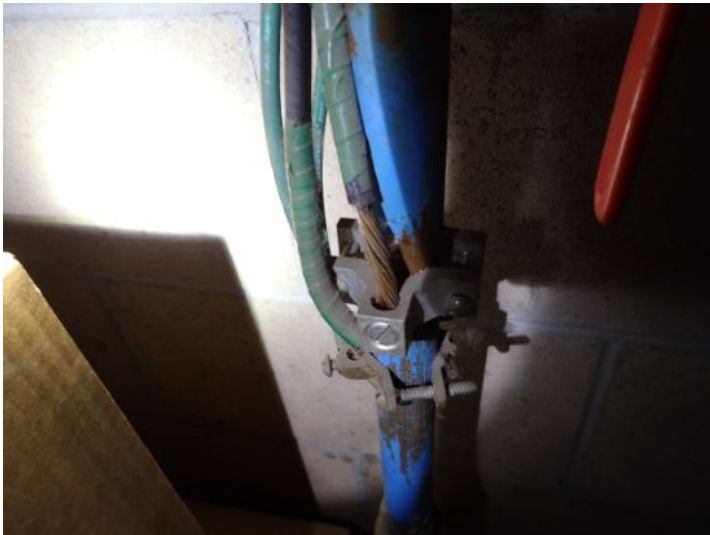
The cold water ground was in place and appeared functional at the time of the inspection.
