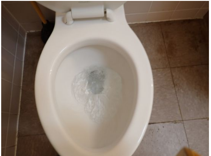
The restroom facilities were tested and functional at the time of the inspection.
