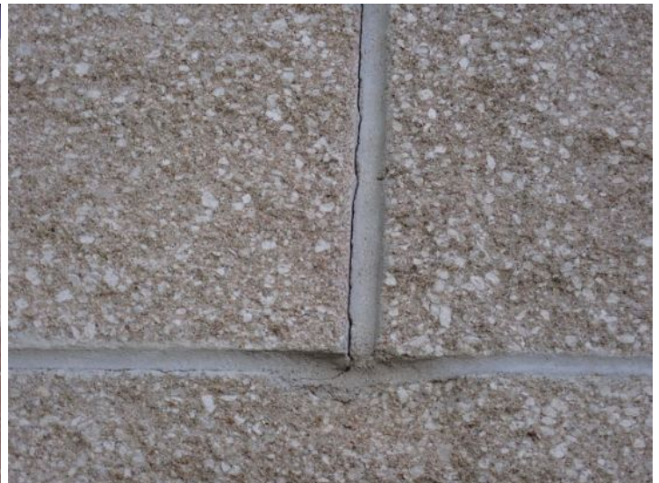
Minor stair stepping noted in the mortar on the rear of the structure at the time of the inspection. Recommend monitoring for future repairs.
