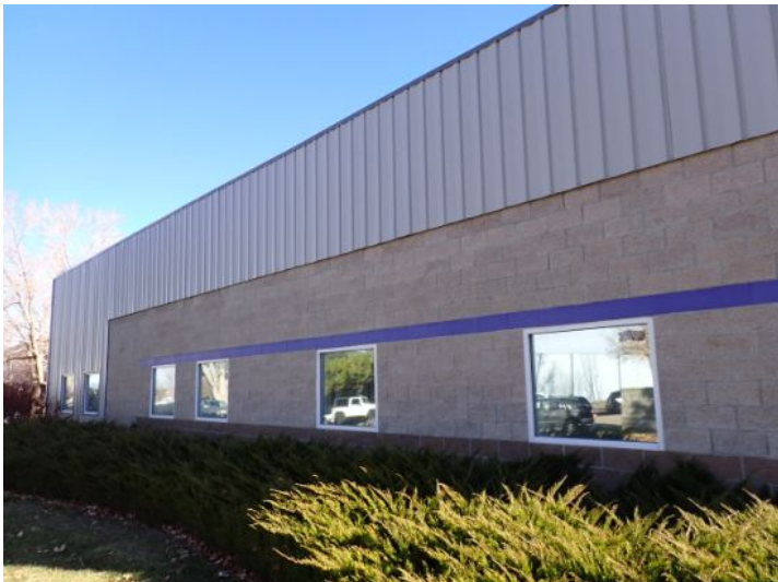
The majority of the exterior envelope of the structure appeared to be in fair condition with no significant movement noted at the time of the inspection.
