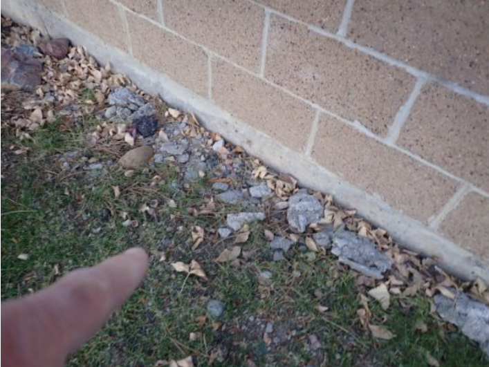
Signs of poor drainage noted along the rear of the structure at the time of the inspection. Recommend repairs by a licensed contractor.
