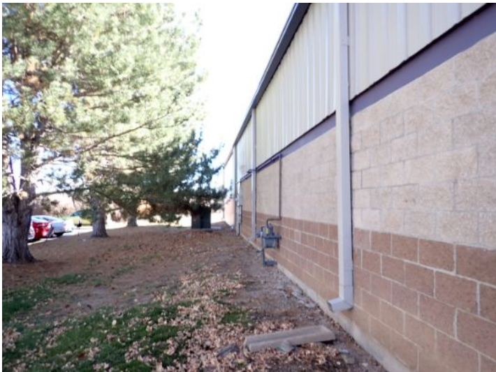
The majority of the exterior envelope of the structure appeared to be in fair condition with no significant movement noted at the time of the inspection.
