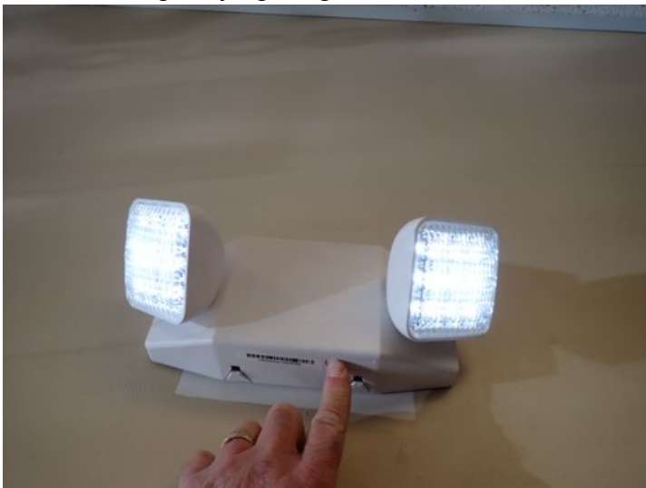
The emergency lighting was tested and functional at the time of the inspection.
