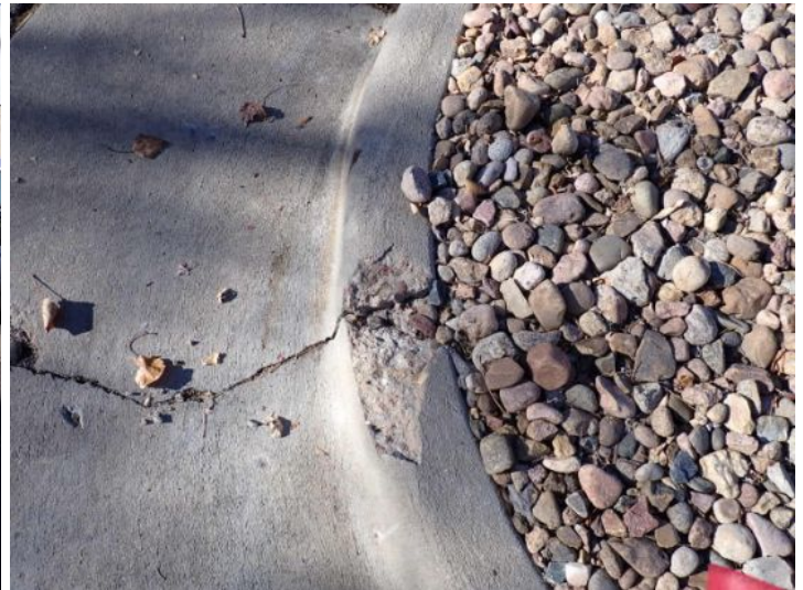
Minor curbing damage noted in areas. Recommend repairs.
