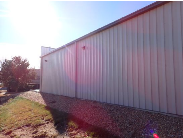
The majority of the exterior envelope of the structure appeared to be in fair condition with no significant movement noted at the time of the inspection.
