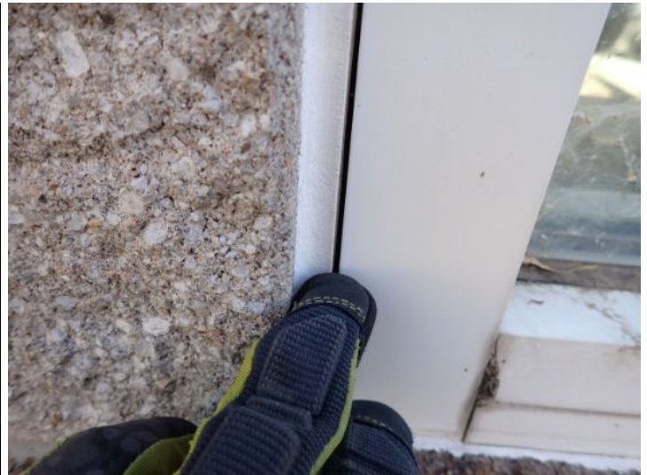
Recommend assuring that any area where two separate substrates meet be properly caulked/sealed. Recommend repairs by a licensed contractor.
