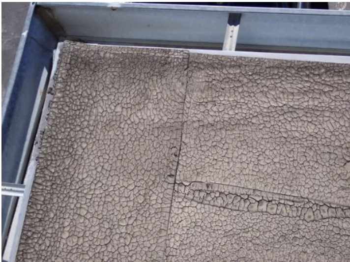
The roofing system located above the front entry was in poor condition and requires complete replacement. Recommend replacement by a licensed contractor.
