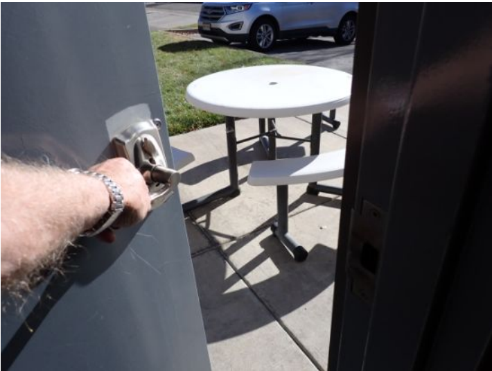
The overhead doors and personnel doors were tested and functional at the time of the inspection.
