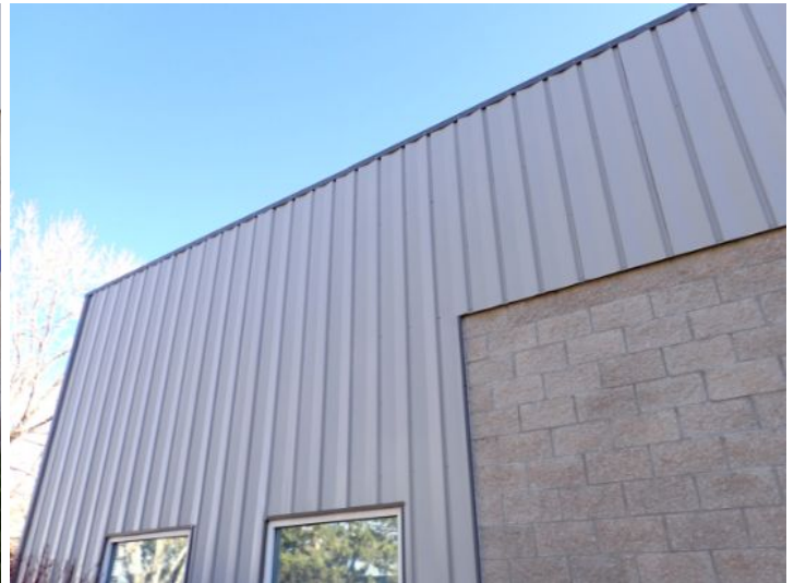
The majority of the exterior envelope of the structure appeared to be in fair condition with no significant movement noted at the time of the inspection.
