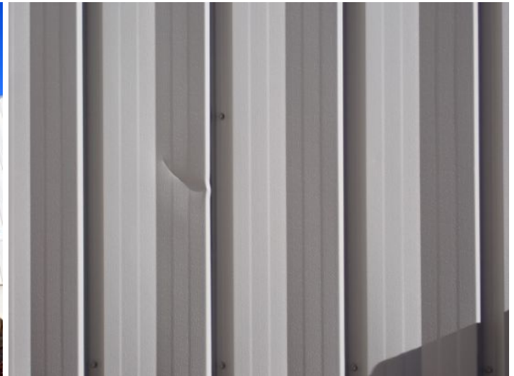
Minor steel siding damage noted in areas. Recommend repairs by a licensed contractor.
