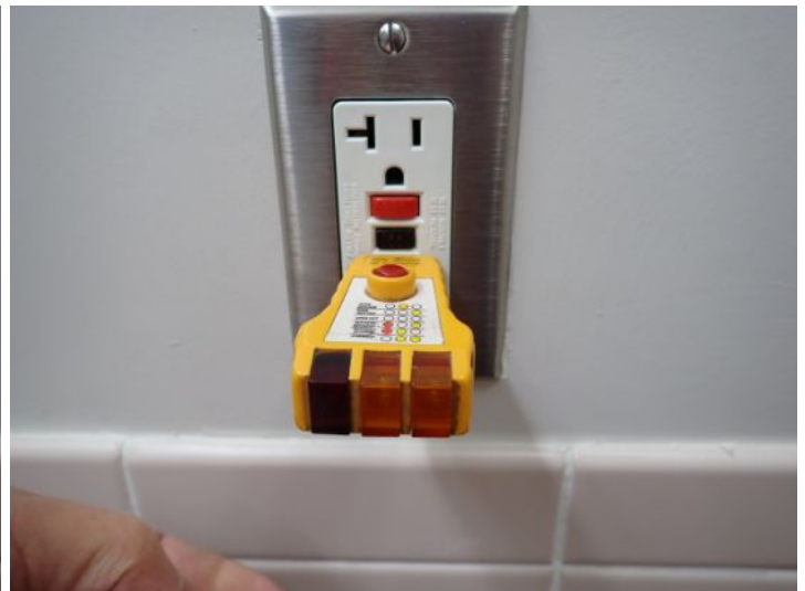
GFCI outlets were tested and operated correctly at the time of the inspection.
