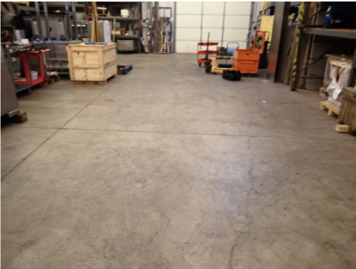
The majority of the interior of the warehouse area appeared to be in fair condition at the time of the inspection.
