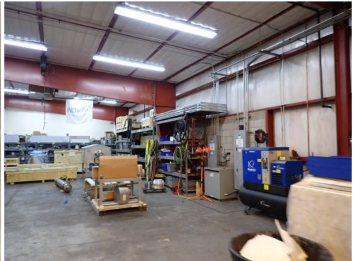
The majority of the interior of the warehouse area appeared to be in fair condition at the time of the inspection.
