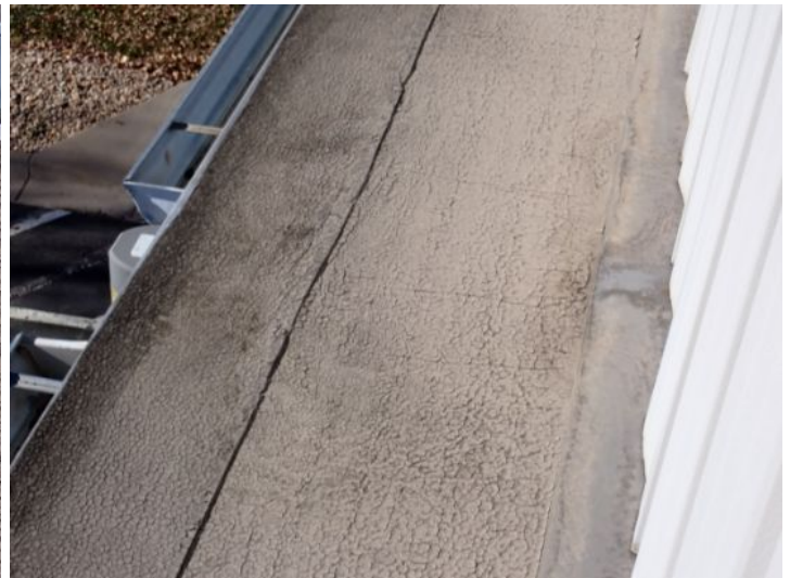
The roofing system located above the front entry was in poor condition and requires complete replacement. Recommend replacement by a licensed contractor.
