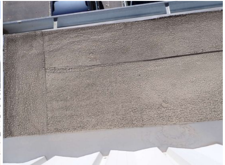
The roofing system located above the front entry was in poor condition and requires complete replacement. Recommend replacement by a licensed contractor.
