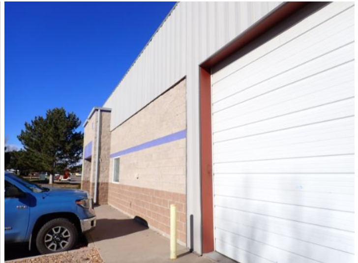
The majority of the exterior envelope of the structure appeared to be in fair condition with no significant movement noted at the time of the inspection.
