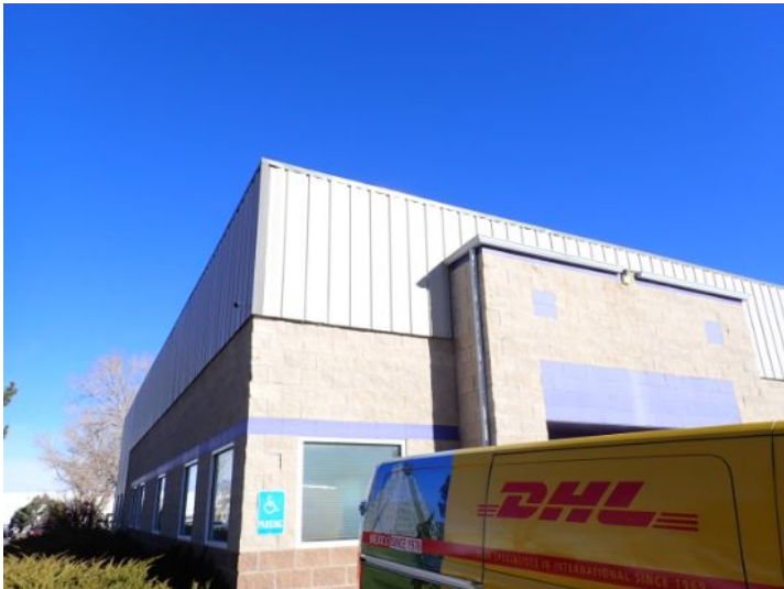
The majority of the exterior envelope of the structure appeared to be in fair condition with no significant movement noted at the time of the inspection.
