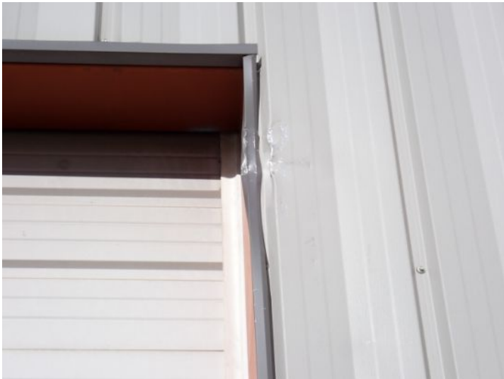
Minor steel trim damage noted around one or more of the overhead doors at the time of the inspection. Recommend repairs by a licensed contractor.
