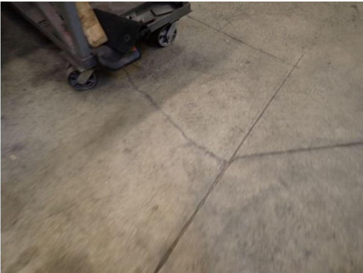
Minor slab cracking noted within the structure at the time of the inspection. Recommend monitoring for future movement/repairs.
