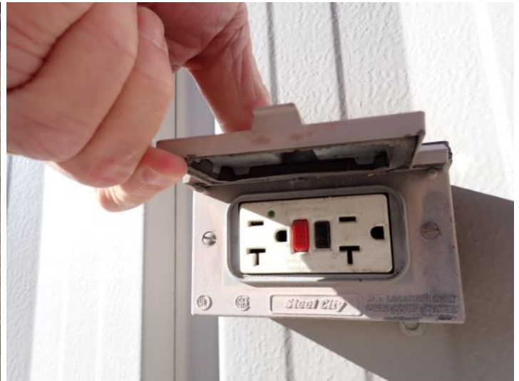
GFCI outlets were tested and operated correctly at the time of the inspection.
