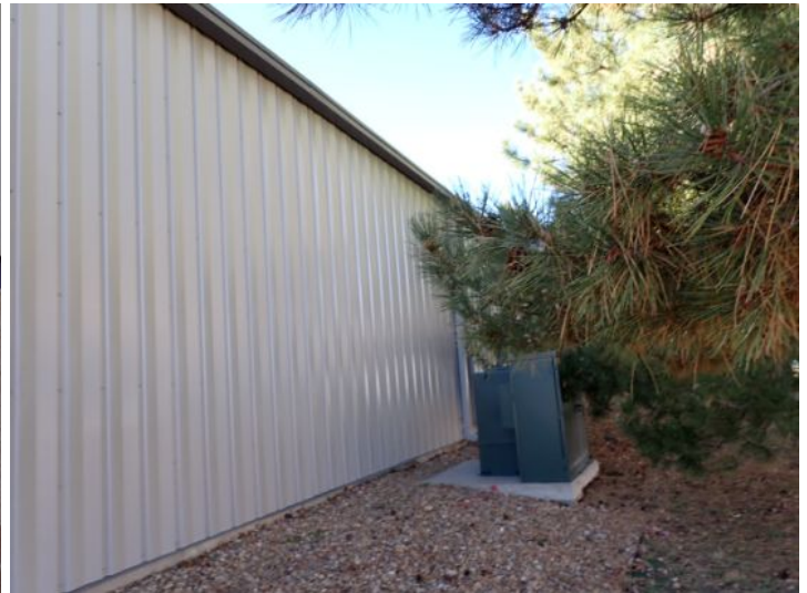
The majority of the exterior envelope of the structure appeared to be in fair condition with no significant movement noted at the time of the inspection.
