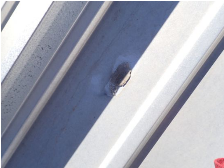
Past repairs/sealant noted in areas of the roofing system. At the time of the inspection the sealant appeared to be nearing failure. Recommend repairs as needed by a licensed contractor.
