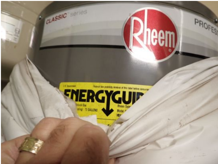
Age of water heater could not be determined as the unit was wrapped in an insulating blanket at the time of the inspection.
