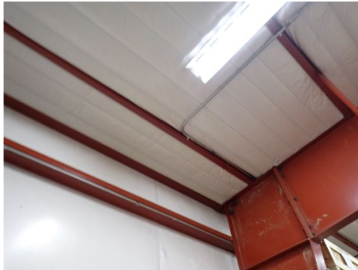
The majority of the interior of the warehouse area appeared to be in fair condition at the time of the inspection.
