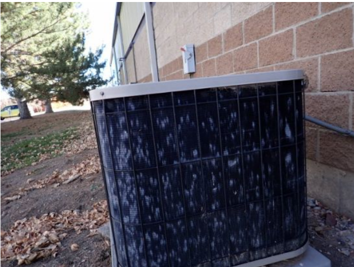
Hail damage noted on the external cooling fins of CU 1 at the time of the inspection.
