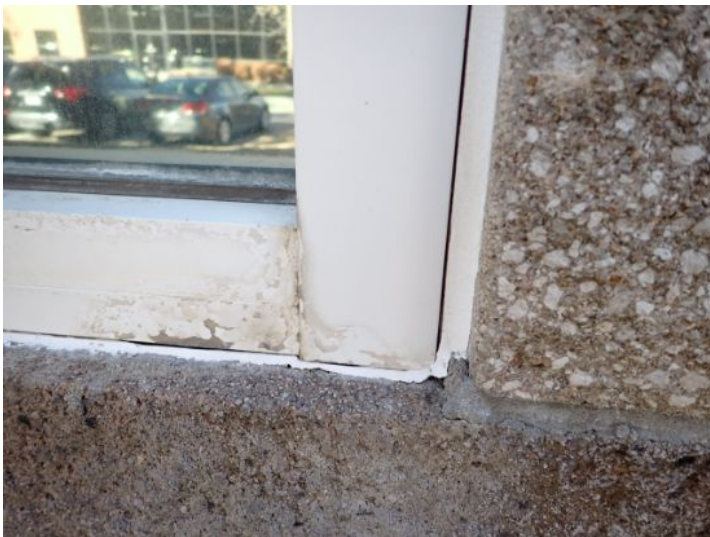
Recommend assuring that any area where two separate substrates meet be properly caulked/sealed. Recommend repairs by a licensed contractor.
