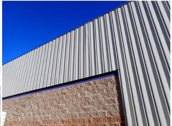
The majority of the exterior envelope of the structure appeared to be in fair condition with no significant movement noted at the time of the inspection.
