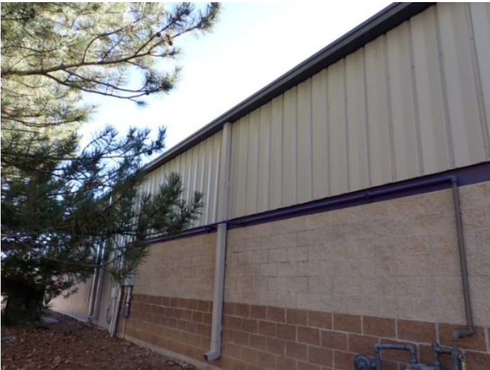
The majority of the exterior envelope of the structure appeared to be in fair condition with no significant movement noted at the time of the inspection.
