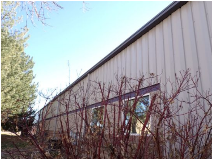
The majority of the exterior envelope of the structure appeared to be in fair condition with no significant movement noted at the time of the inspection.
