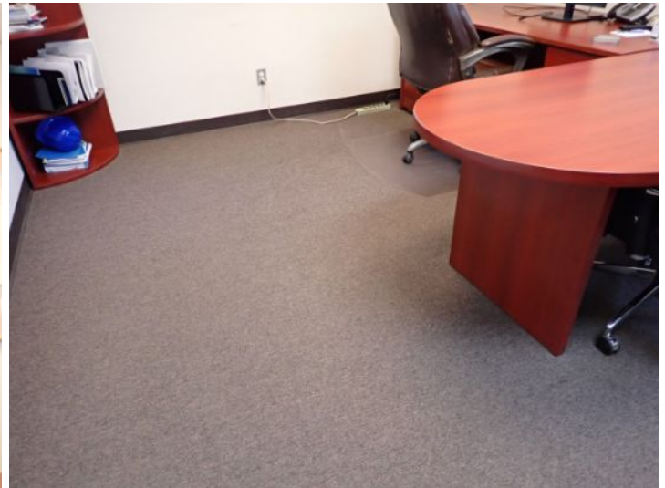
The majority of the interior of the office area appeared to be in fair condition at the time of the inspection.
