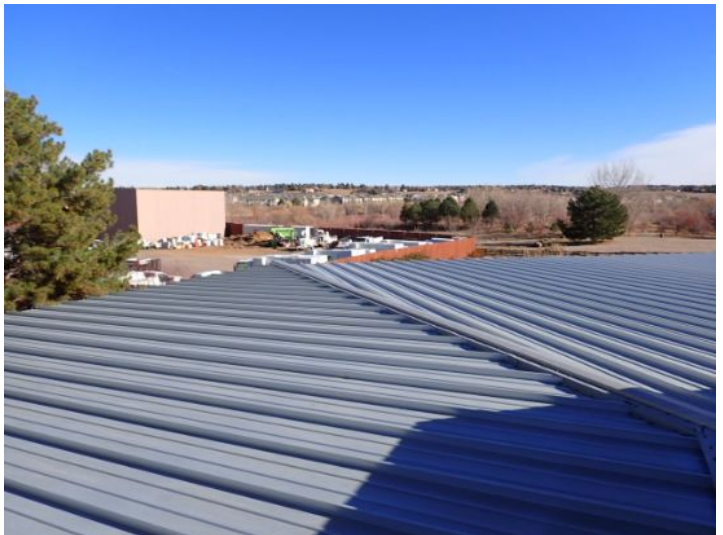
The majority of the standing seam metal roofing system appeared to be in fair condition at the time of the inspection.
