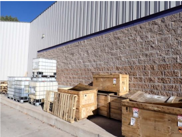
The majority of the exterior envelope of the structure appeared to be in fair condition with no significant movement noted at the time of the inspection.
