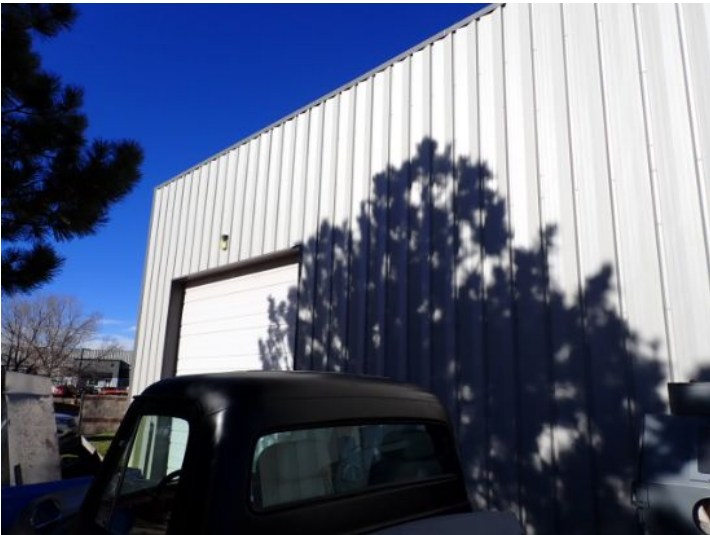
The majority of the exterior envelope of the structure appeared to be in fair condition with no significant movement noted at the time of the inspection.
