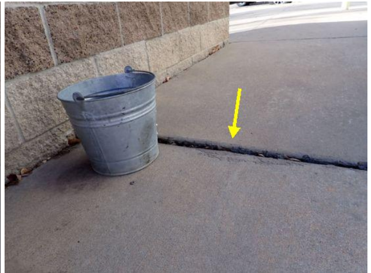
Trip hazards noted. Recommend repairs.
