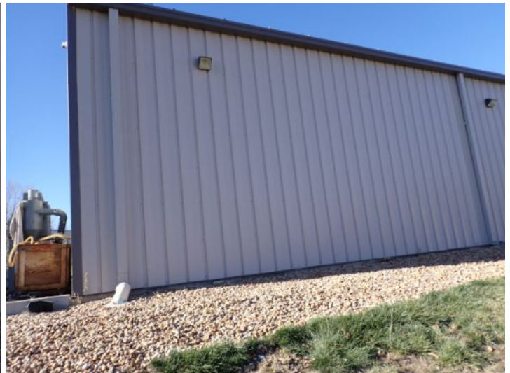
The majority of the exterior envelope of the structure appeared to be in fair condition with no significant movement noted at the time of the inspection.
