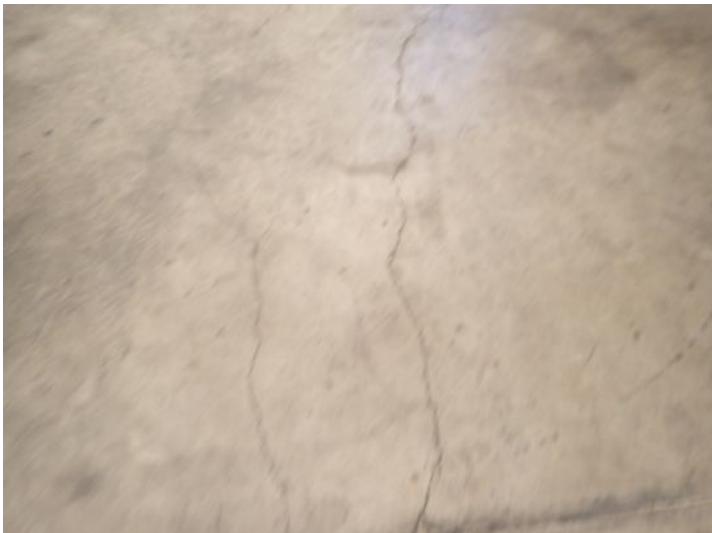
Minor slab cracking noted within the structure at the time of the inspection. Recommend monitoring for future movement/repairs.
