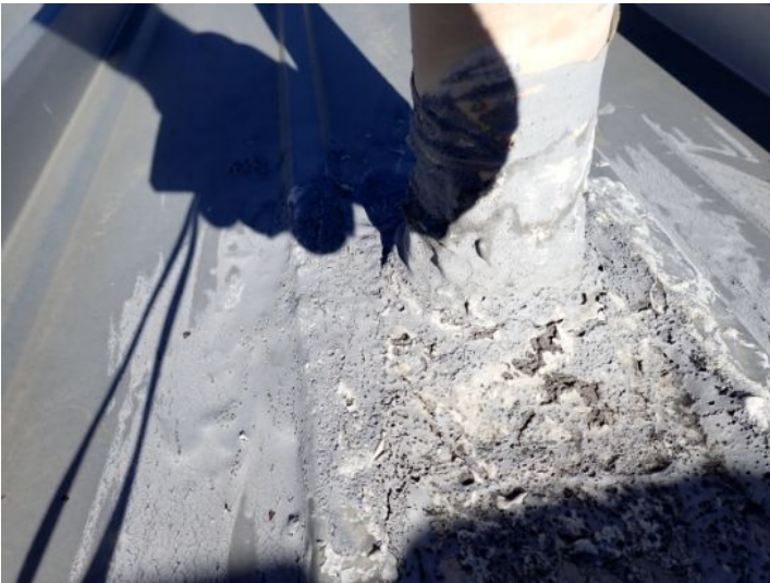
The sealant around the roof penetrations appeared to have reached its serviceable life expectancy and may begin leaking soon. Recommend repairs as needed by a licensed contractor.
