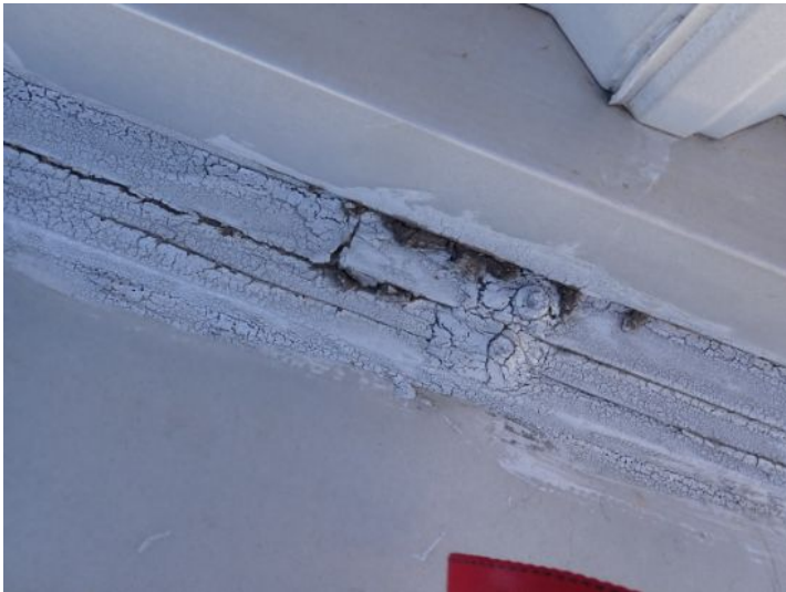
Sealant/repairs noted in areas along the parapet walls of the roofing system. At the time of the inspection the sealant appeared to have reached or be nearing its serviceable life expectancy. Recommend repairs as needed by a licensed contractor.
