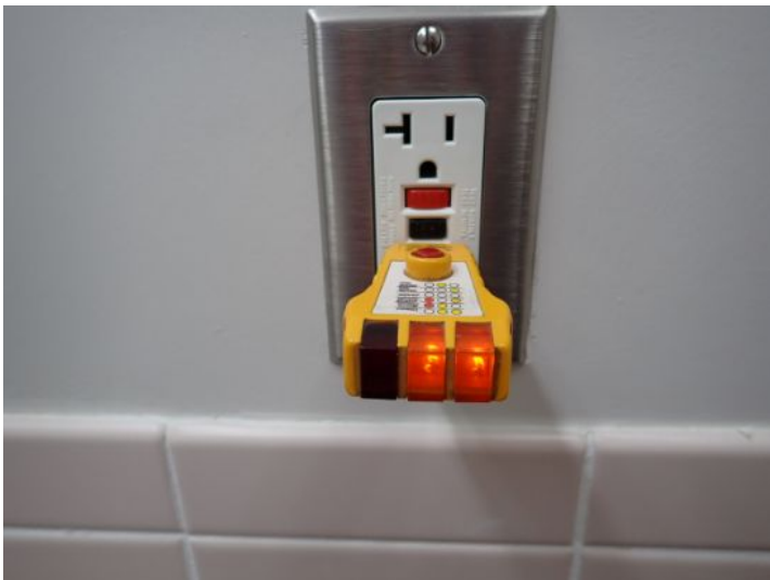
GFCI outlets were tested and operated correctly at the time of the inspection.
