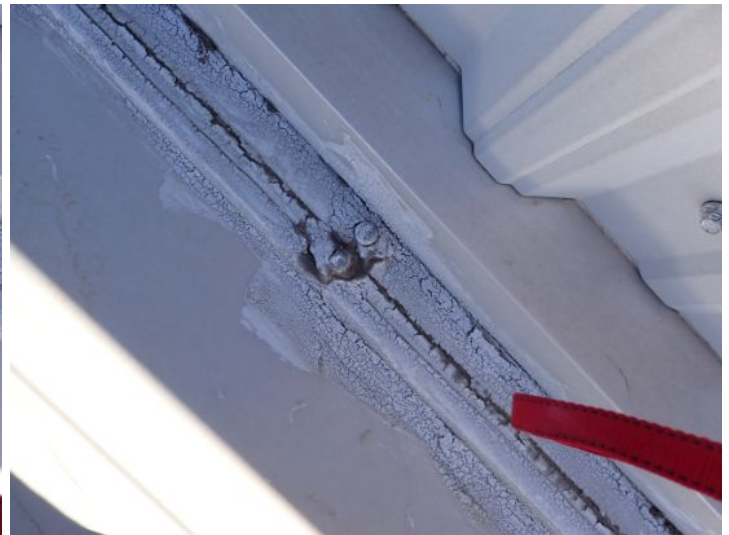
Sealant/repairs noted in areas along the parapet walls of the roofing system. At the time of the inspection the sealant appeared to have reached or be nearing its serviceable life expectancy. Recommend repairs as needed by a licensed contractor.
