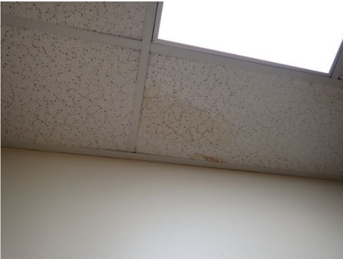
Minor past moisture staining noted in one or more of the acoustical ceiling tiles but no moisture present at the time of the inspection. Recommend repairs and monitoring for any future issues.
