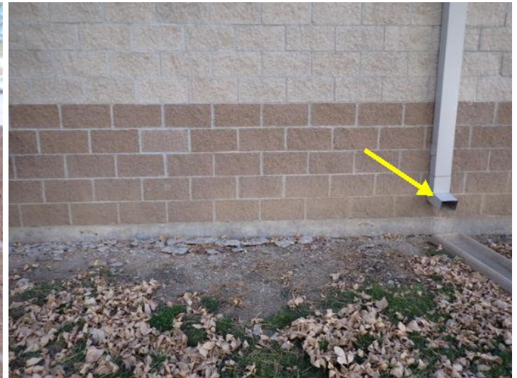
Gutters down spouts missing extensions to direct storm water away from the foundation of the structure. Recommend repairs.
