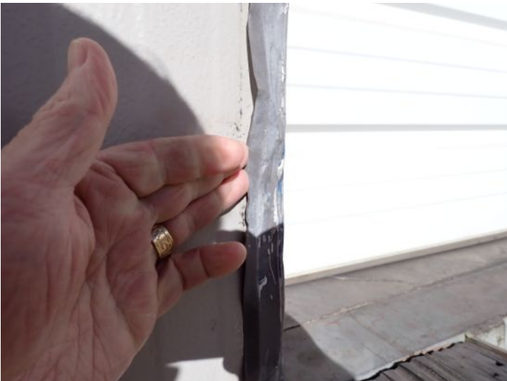
Minor steel trim damage noted around one or more of the overhead doors at the time of the inspection. Recommend repairs by a licensed contractor.
