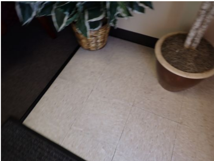
VCT flooring damage noted in the main entry area. Recommend repairs as needed by a licensed contractor.
