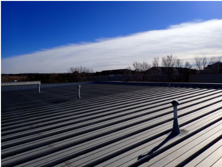
The majority of the standing seam metal roofing system appeared to be in fair condition at the time of the inspection.
