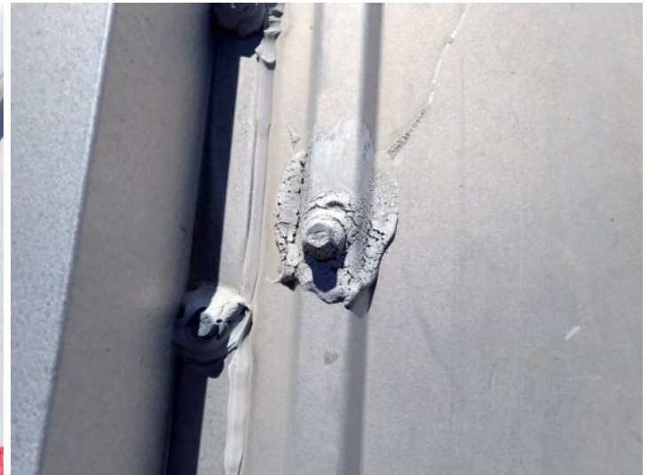
Past repairs/sealant noted in areas of the roofing system. At the time of the inspection the sealant appeared to be nearing failure. Recommend repairs as needed by a licensed contractor.
