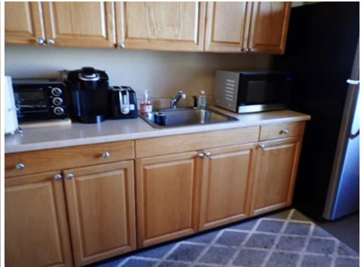
The majority of the interior of the office area appeared to be in fair condition at the time of the inspection.
