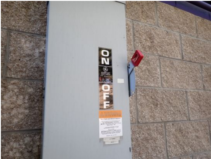
The main electrical disconnect appeared functional at the time of the inspection.
