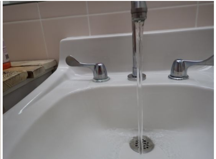
The restroom facilities were tested and functional at the time of the inspection.
