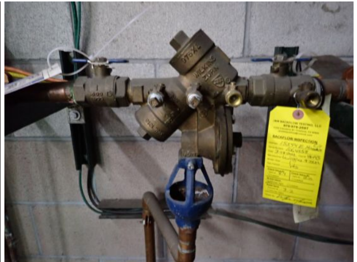
A backflow preventer was installed on the main water supply line at the time of the inspection.
