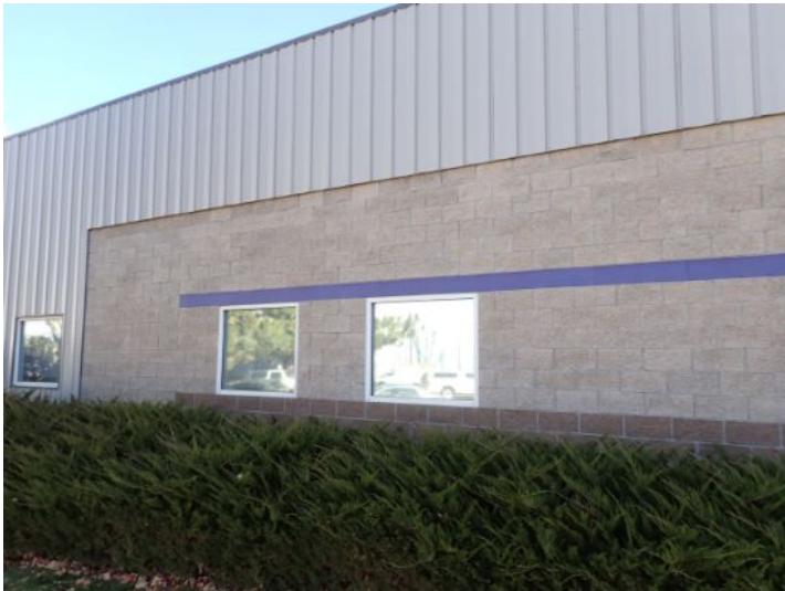
The majority of the exterior envelope of the structure appeared to be in fair condition with no significant movement noted at the time of the inspection.
