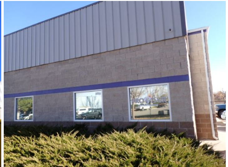
The majority of the exterior envelope of the structure appeared to be in fair condition with no significant movement noted at the time of the inspection.
