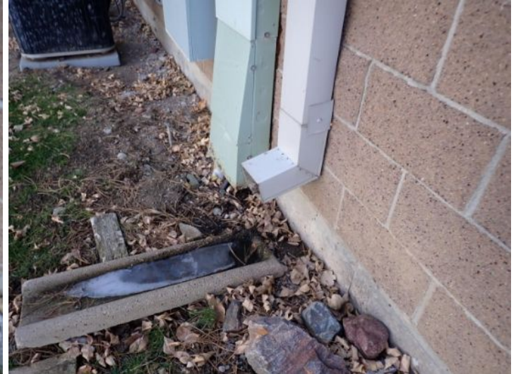
Signs of poor drainage noted along the rear of the structure at the time of the inspection. Recommend repairs by a licensed contractor.
