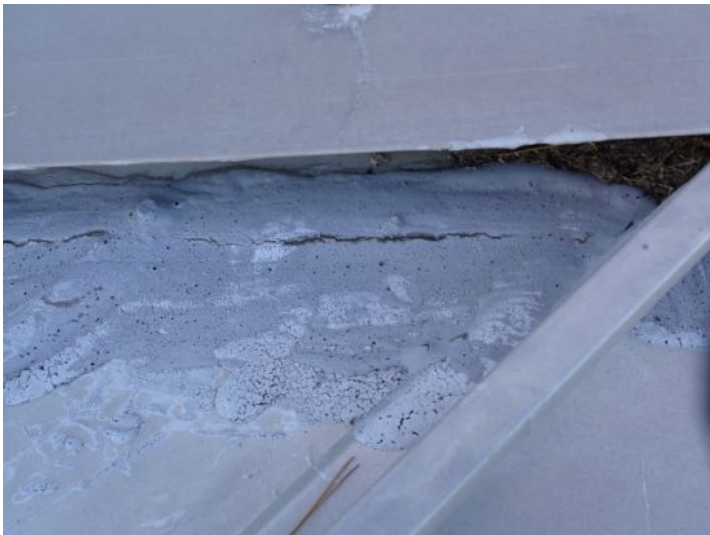
Past repairs/sealant noted in areas of the roofing system. At the time of the inspection the sealant appeared to be nearing failure. Recommend repairs as needed by a licensed contractor.
