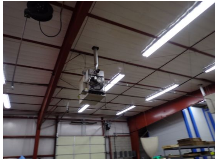
The majority of the interior of the warehouse area appeared to be in fair condition at the time of the inspection.
