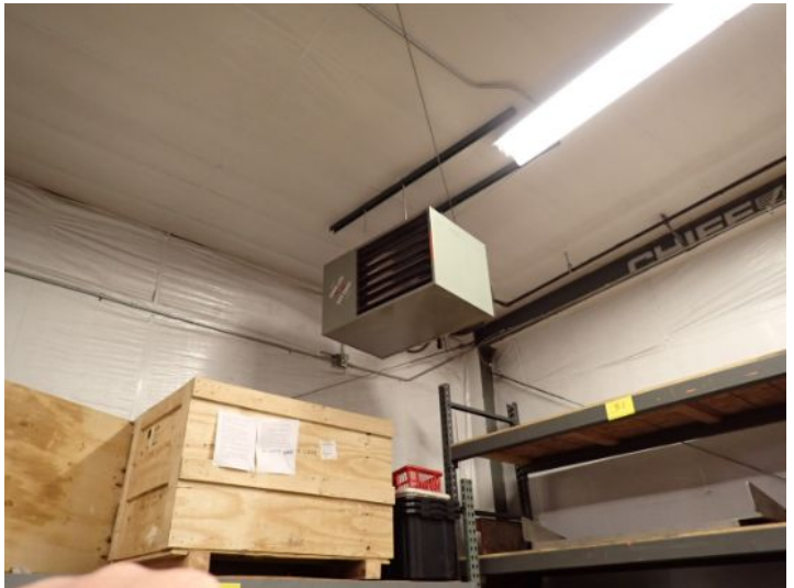
The shop heaters located in the east side of the warehouse were not functional at the time of the inspection. Recommend repairs as needed by a licensed contractor.
