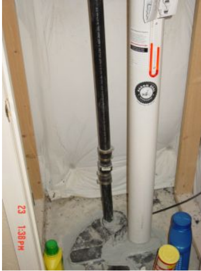
Radon Mitigation System
