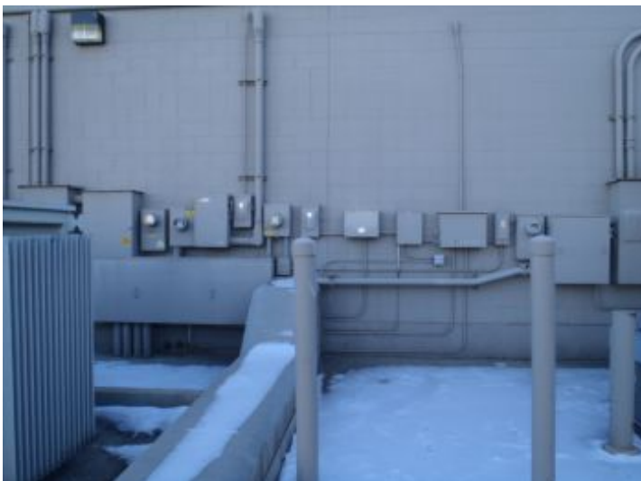
Current Electrical is located on the outside of the building. New electrical will be placed in an electrical room.
