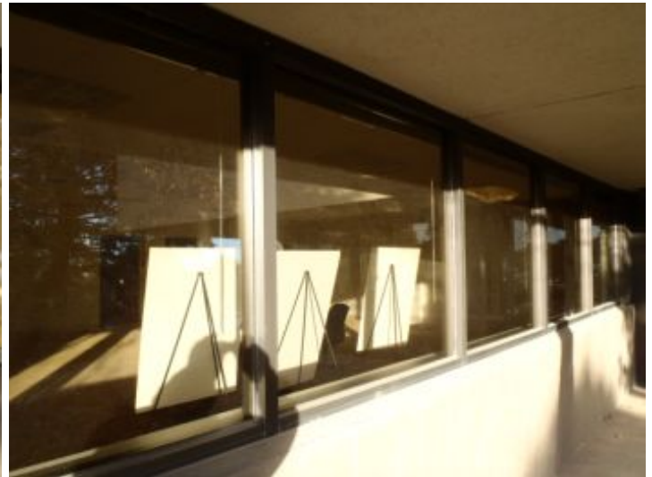
The front of the condo consists of concrete masonry partial walls with insulated glass storefront above that running to the ceiling.
