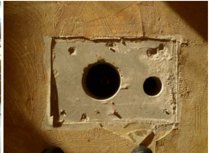
There is evidence of previous movement of the buildings slab. The slab was mud jacked to repair it. At the time of the inspection the slab appeared to be in good condition, and was relatively level throughout. There is a noticeable crack near the wall to the next to the condo south with a slight rise in the floor. When interviewing Bill Woodward he informed inspector that the association is responsible for the buildings slab. There is a whole in the slab from an old water line. The line has been decommissioned and the holes will be filled.
