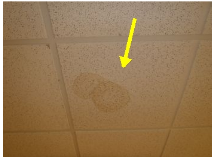
Observed leakage: When viewing the roof from the underside, by lifting interior suspended roof tiles, there were no leaks observed at the time of the inspection. There is a moisture stain in one of the ceiling tiles, but there was not moisture present at the time of the inspection.
