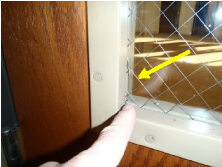
The secondary entrance door, that is equipped with the wire safety glass, has a crack in the glass. Recommend repair/replacement.
