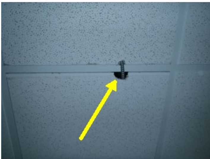
In the back office there is a section of flexible electrical conduit running through two ceiling tiles and around a suspended ceiling support. Recommend repair/replacement when electrical contractor is running new electrical in the building.
