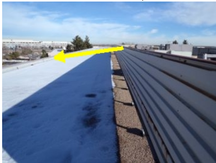
Drainage: The roof is sloped to the back of the building to aid in drainage. The gutter drainage appeared clear. There were additional roof drains located strategically throughout the roofs surface.
