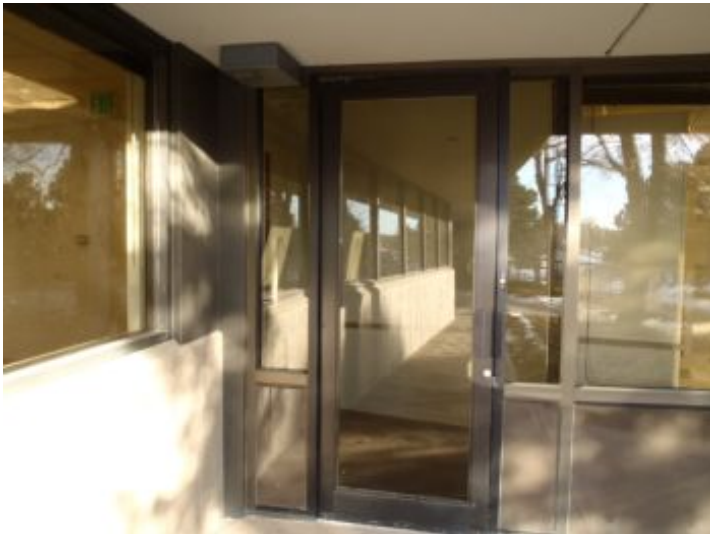
The current entrance door to the unit would not be considered ADA compliant as it requires too much force to open and closes too quickly. Upon interviewing Bill Woodward concerning the remodel that is taking place in the unit inspector was informed that the new entrance door will be ADA compliant.
