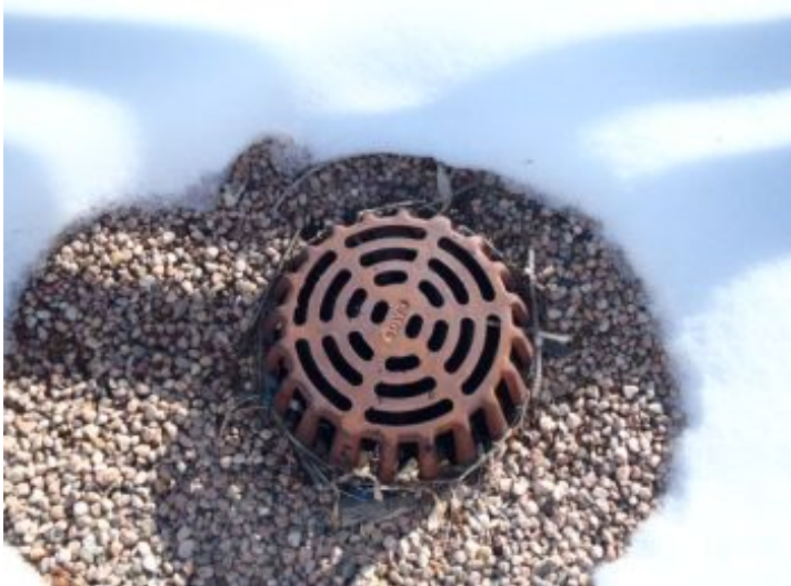
Drainage: The roof is sloped to the back of the building to aid in drainage. The gutter drainage appeared clear. There were additional roof drains located strategically throughout the roofs surface.
