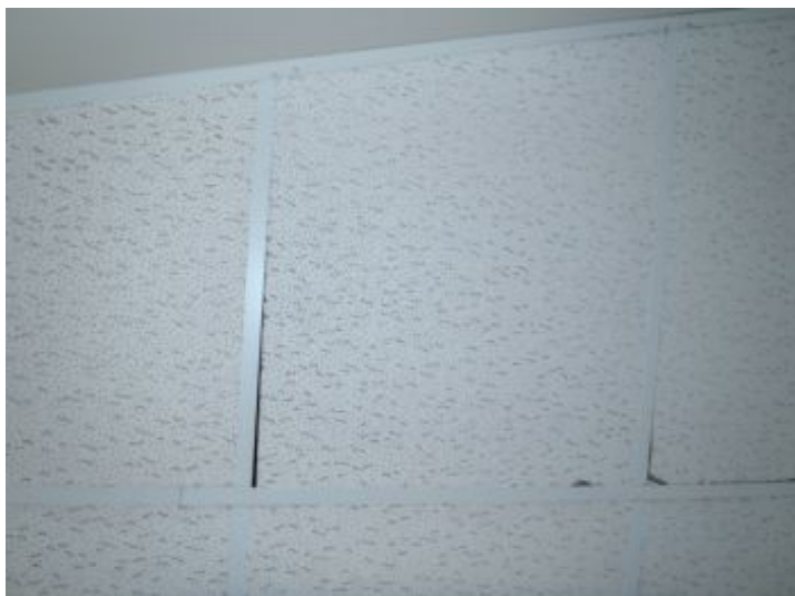
There are several damaged, or dirty, ceiling tiles. Recommend replacement after the remodel/build out.
