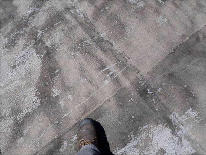
The narrow or small rolled torch down roofing system located approximately the center of the West Wing was an extremely poor condition of time inspection and requires completely recommend a licensed roofing contractor
