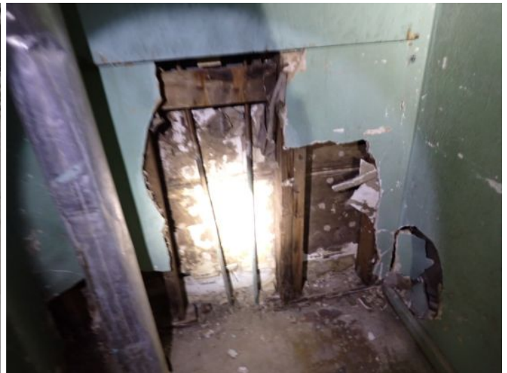
Unit 108-107: Vacant: Unit will require significant renovations prior to installing tenant. Active moisture noted in interior wall with possible microbial growth. Significant drywall damage noted in ceiling in loading dock area. Basement area in poor condition. Basement bathrooms in poor condition. Electrical not working at the time of the inspection. Moisture intrusion/damage noted in basement walls. Recommend repairs as needed by a licensed contractor.
