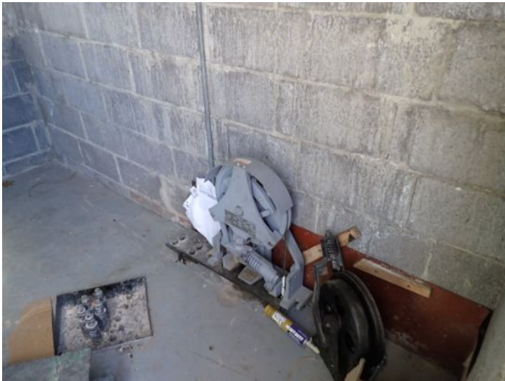
There was an old elevator room located on the roof above the mall area at time the inspection that no longer appear to be in use.
