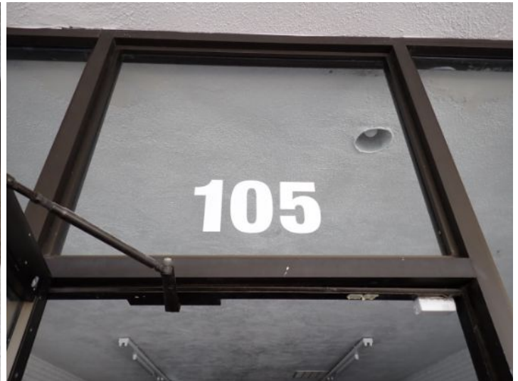
Unit 105: Vacant Unit: No significant findings noted at the time of the inspection
