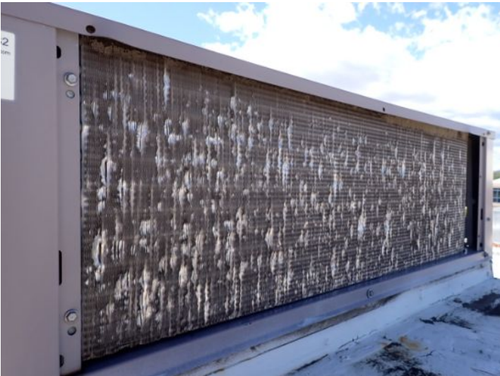
Significant hail damage noted on RTU 32 at the time of the inspection. Due to the age and condition of the unit we recommend a complete replacement by a licensed hvac contractor.
