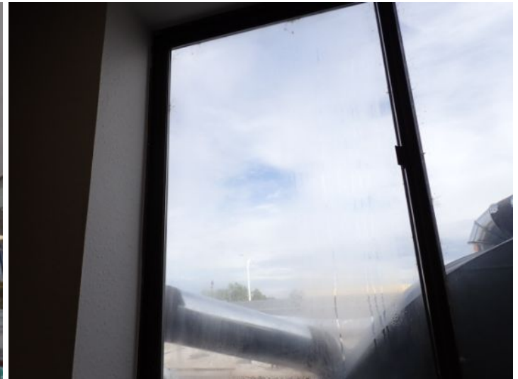
Failed seals noted in multiple insulated window units at the time of the inspection. Recommend repairs by a licensed contractor.
