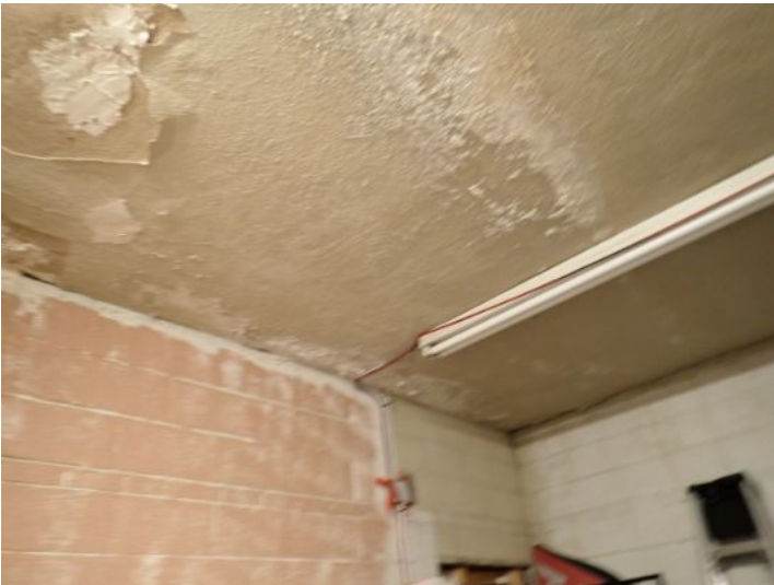
Unit 103: VCT flooring damage noted. Moisture staining noted in ceiling tiles. Moisture damage noted in rear ceiling. Recommend repairs.
