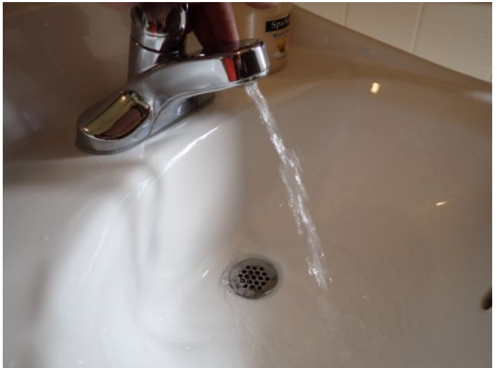
The common area restrooms in the office building and mall areas were tested and functional at the time of the inspection.
