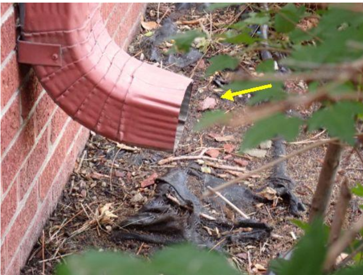
Gutters down spouts missing extensions to direct storm water away from the foundation of the structure. Recommend repairs.
