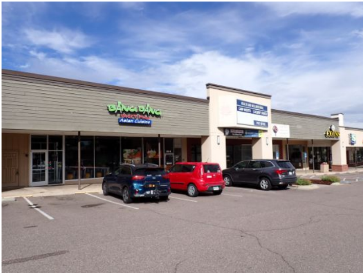
The majority of the exterior envelope of the structure appeared to be in fair condition with no significant structural movement noted at the time of the inspection.
