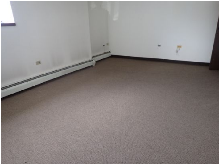
The majority of the interior offices, that were accessible at the time of the inspection, appeared to be in fair condition at the time of the inspection.
