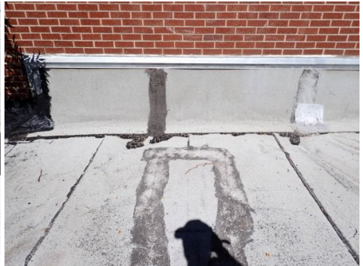
The rolled asphalt composition roof and system located above the awning between the two wings was in extremely poor condition why is it a plate replacement. Recommend repair by a licensed contractor.
