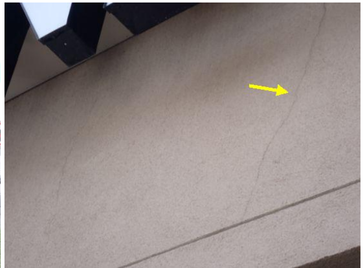
Stucco cracking noted in areas around the structure at the time of the inspection. Recommend repairs by a licensed contractor.
