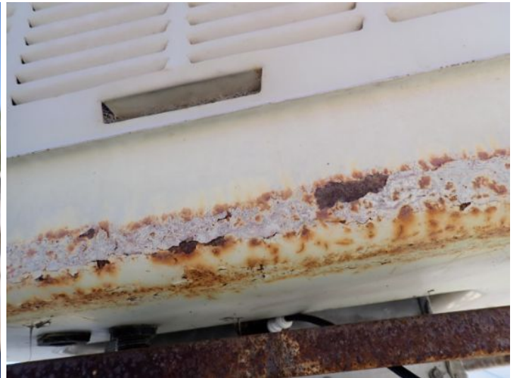
The small swamp cooler located on the upper level roof on the east end of the property was in poor condition at time of the inspection requires complete replacement. Recommend replacement by a licensed contractor.
