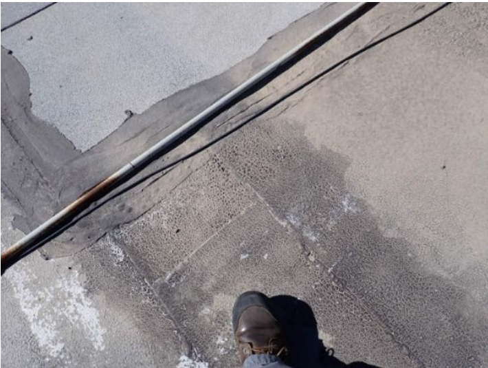
The rolled torch down roofing system above what used to be the old theater it is now currently being used as the office area appeared to be original to the structure and was showing signs of hail damage excessive ponding where and patching. Recommend replacement by licensed contractor.
