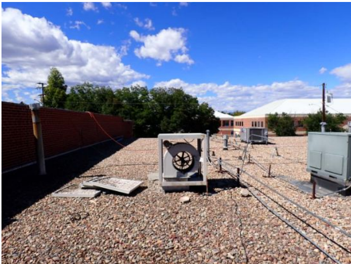
The swamp coolers located on the top of the gravel coated EPDM roofing system located on the north end of the west wing or poor condition in that social time of the inspection. These units are no longer in service we recommend removal.
