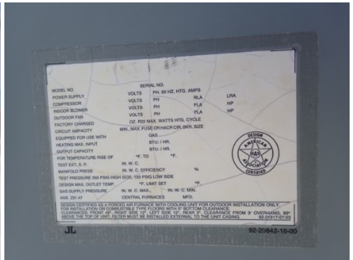
RTU 25: RUUD: M/N? S/N ? Manufacture year ?
