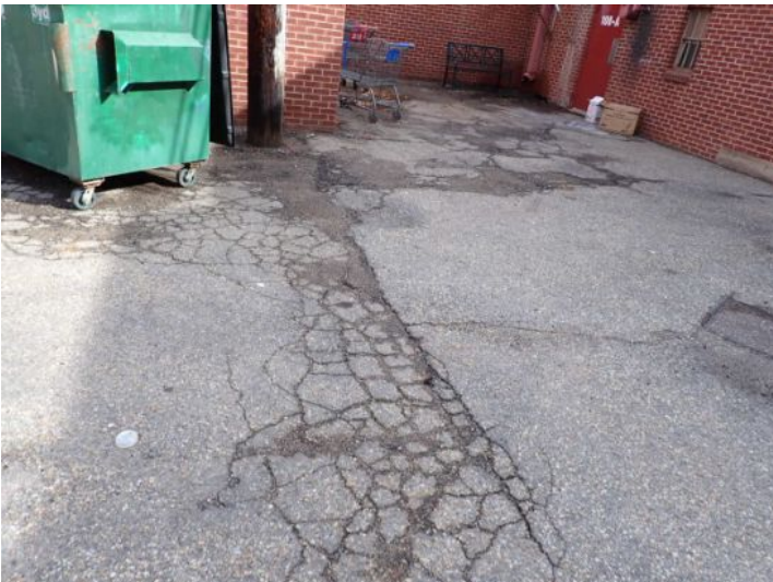
The asphalt running along the rear west side of the structure was in poor condition at the time of the inspection. Recommend resurfacing by a licensed contractor.
