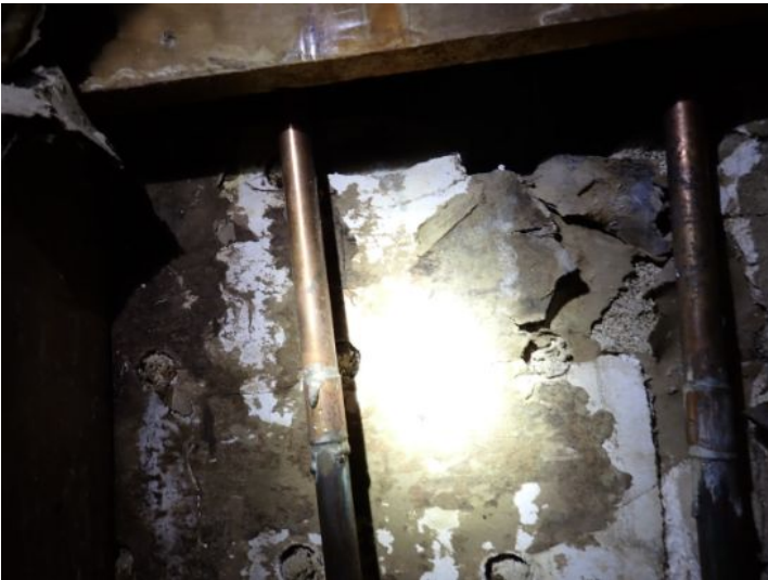
Unit 108-107: Vacant: Unit will require significant renovations prior to installing tenant. Active moisture noted in interior wall with possible microbial growth. Significant drywall damage noted in ceiling and walls in loading dock area. Basement area in poor condition. Basement bathrooms in poor condition. Electrical not working at the time of the inspection. Moisture intrusion/damage noted in basement walls. Recommend repairs as needed by a licensed contractor.
