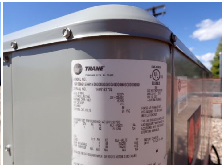
RTU 22: Trane: M/N YSC060E1EHA1N00000 S/N 144912273L. Manufacture year 2014.
