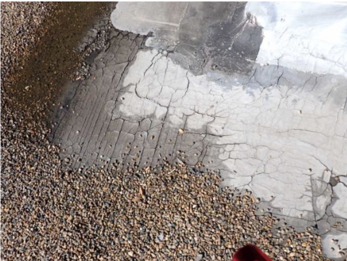
The rolled torch down roofing system above what used to be the old theater it is now currently being used as the office area appeared to be original to the structure and was showing signs of hail damage excessive ponding where and patching. Recommend replacement by licensed contractor.
