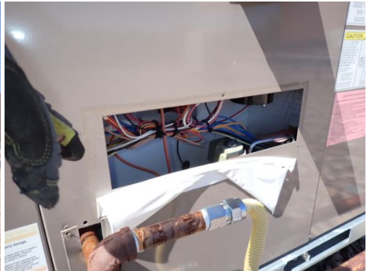
Missing side cover plate noted on RTU 29. Recommend repairs by a licensed contractor.
