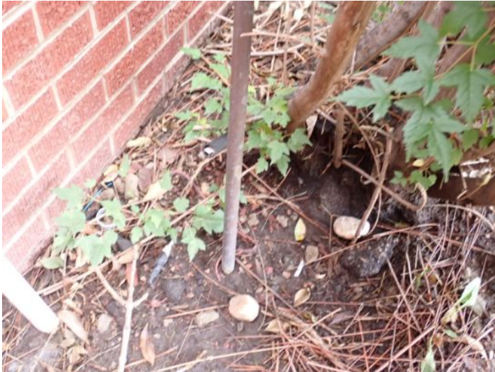
The topography of the property requires attention to assure that the grade directs ground/storm water away from the foundation of the structure.
