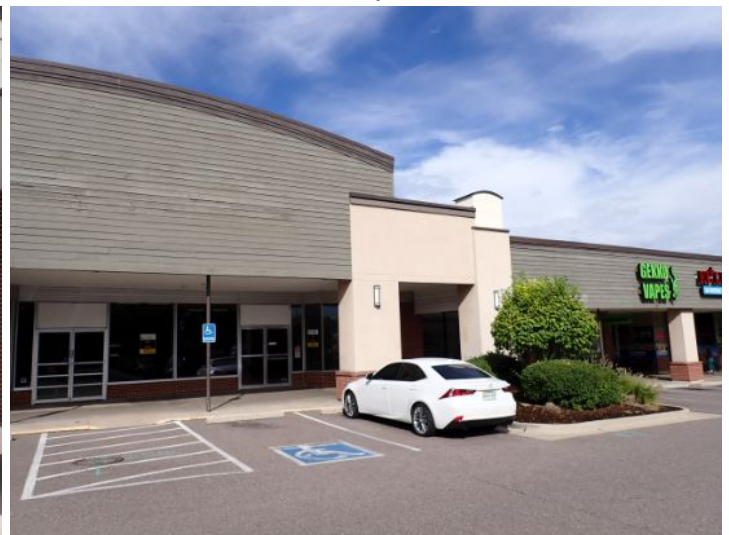
The majority of the exterior envelope of the structure appeared to be in fair condition with no significant structural movement noted at the time of the inspection.
