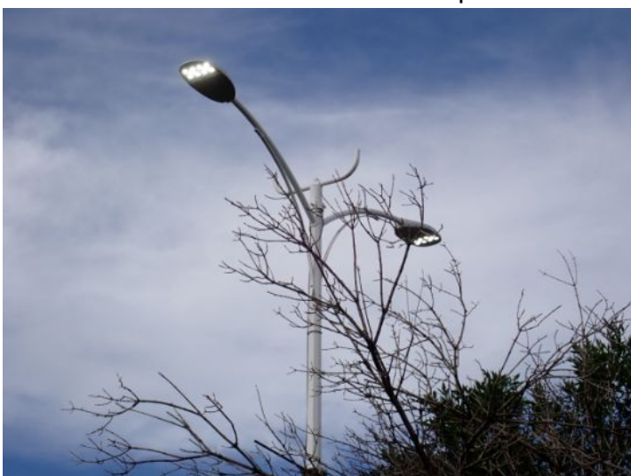
Parking lot lighting system appeared functional at the time of the inspection.
