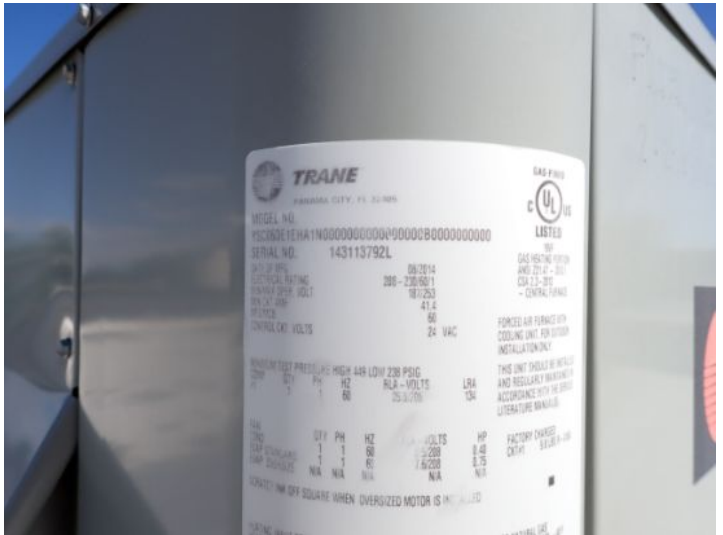
RTU 30: Trane: M/N YSC060E1EHA1N00000 S/N 143113792L. Manufacture year 2014.
