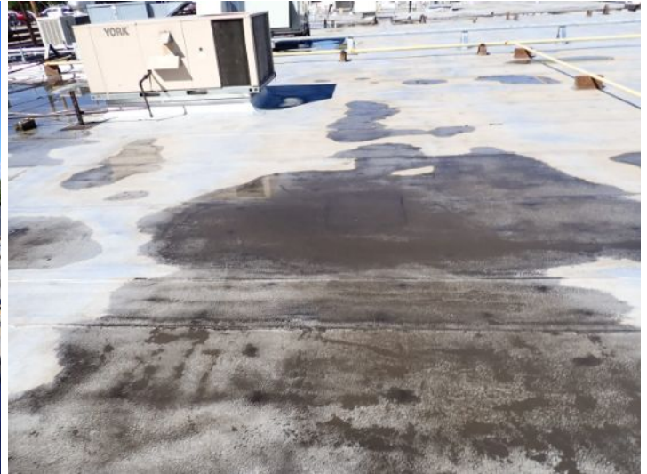
The rolled torch down roofing system located on the lower level south wing of the structure showing signs of excessive deferred maintenance, excessive ponding, possible hail damage and age. Recommend complete replacement by licensed contractor.
