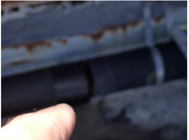
There was what appeared to be a 4 inch wet Vent piping located on the narrow roof above the center of the west wing that was not strapped properly and it becomes separated overtime. This could cause odor issues inside the building. Recommend repairs by licensed contractor.
