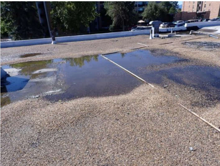
The BUR roofing system located on the east end of the south wing of the building is showing signs of excessive wear excessive ponding it was an extremely poor condition at the time of the inspection. Recommend replacement by a licensed contractor.
