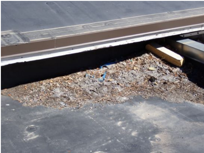
The EPDM roofing membrane located on the lower level of the south wing appeared to be in fair condition at the time of the inspection but was showing signs of excessive ponding and minor seam issues in areas. Recommend repairs as required by a licensed contractor.
