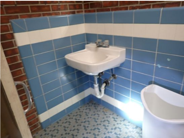
Unit 132: Unit was in poor condition and will require complete renovations prior to installing a new tenant.
