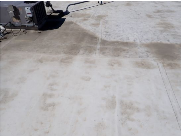
TPO roofing membrane located above the mall area of the property while appearing to be in fair condition was showing signs of excessive deferred maintenance and ponding at the time of the inspection. Recommend repairs by licensed contractor.
