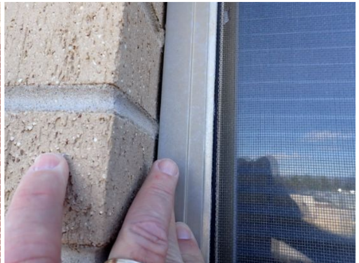
Any area where two separate substrates meet should be properly caulked and sealed. Recommend repairs as needed by a licensed contractor.
