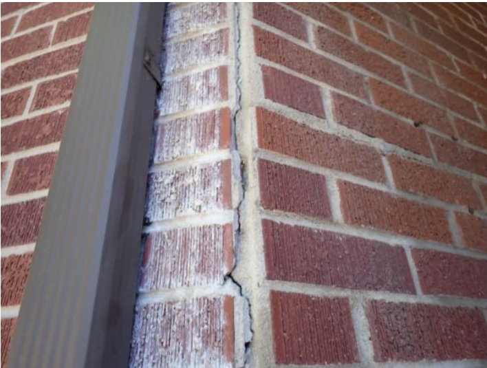
Minor brick damaged and movement noted in the brick siding material at the awning area between the structures. Recommend repairs by a licensed contractor.
