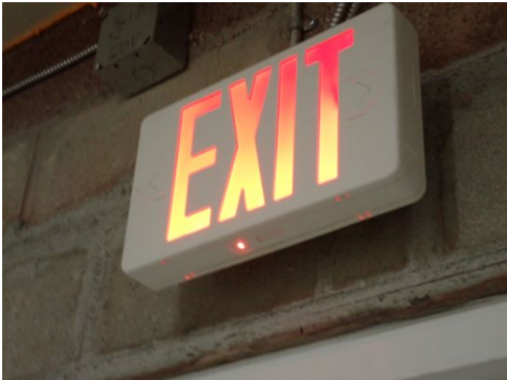
Multiple lighted EXIT signs still have the old red lenses. Many municipalities are now requiring the lenses to be green for better viewing during a fire. Recommend budgeting for replacement of any required units.
