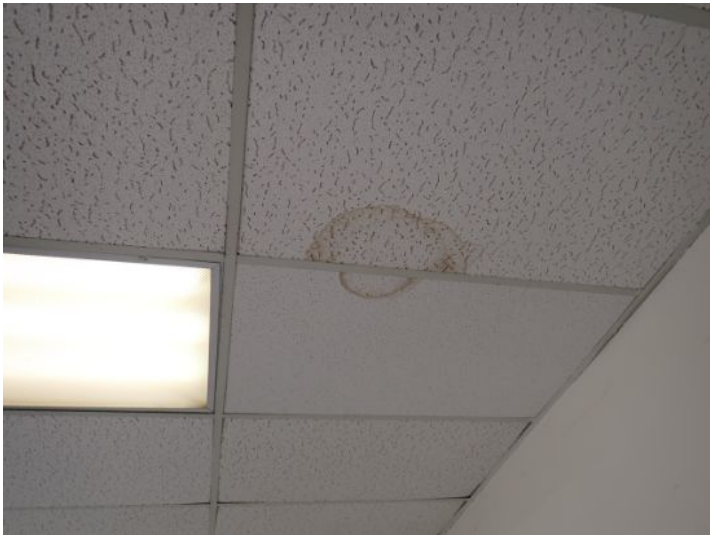
Moisture staining noted in areas of the acoustical tile ceilings throughout the building at the time of the inspection. Recommend repairs and monitoring
