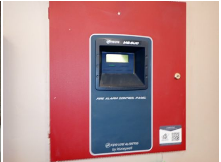
There was a fire alarm and fire suppression system for the basement units located below the mall area. There was also an old fire suppression system located in the basement below the large vacant unit. The remainder of the property did NOT have a fire alarm or fire suppression system located within it at the time of the inspection.
