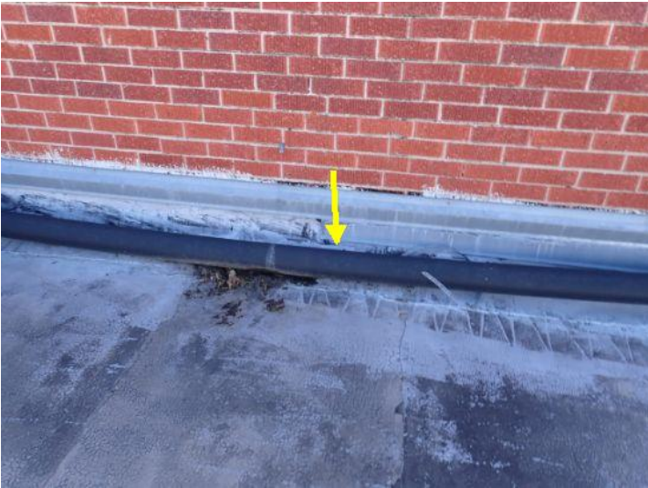
There was what appeared to be a 4 inch wet Vent piping located on the narrow roof above the center of the west wing that was not strapped properly and it becomes separated overtime. This could cause odor issues inside the building. Recommend repairs by licensed contractor.
