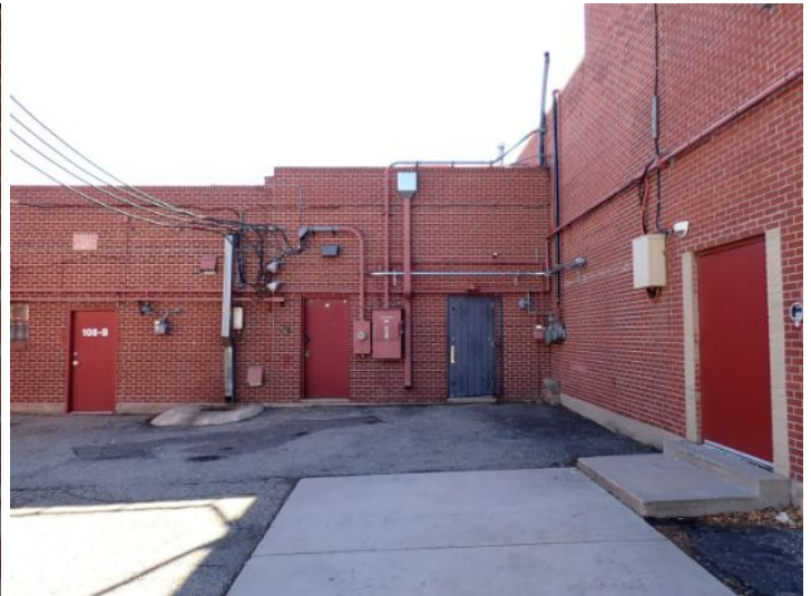
The majority of the exterior envelope of the structure appeared to be in fair condition with no significant structural movement noted at the time of the inspection.
