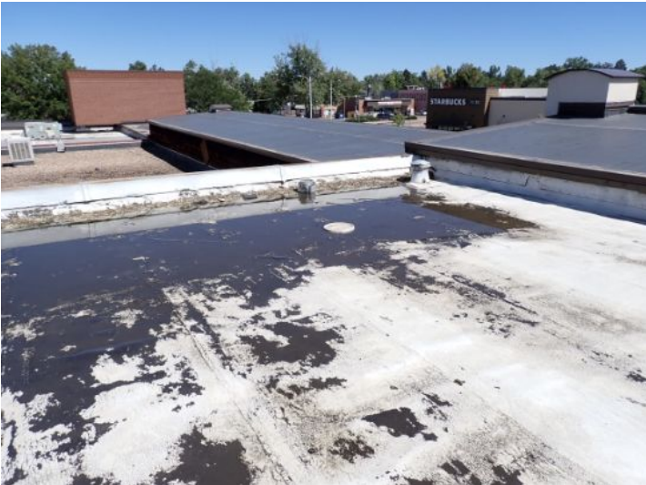
The rolled torch down roofing system above what appeared to be the old family dollar store and the vacant unit was an extremely poor condition excessive ponding feeling coding possible hail damage and excessive wear noted at the time of the inspection. Recommend complete replacement by licensed contractor.
