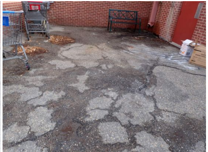
The asphalt running along the rear west side of the structure was in poor condition at the time of the inspection. Recommend resurfacing by a licensed contractor.
