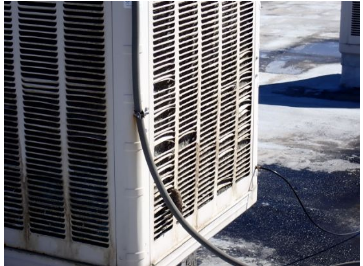
The swamp coolers located above the old theater area that is now being used as office or in fair to poor condition and require servicing and filter repairs by a licensed contractor. Recommend repairs prior to taking possession of the property.
