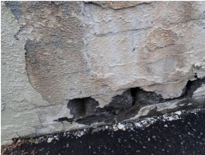
The block retaining wall for the neighboring parking garage was showing signs of significant moisture damage and deterioration in areas. Recommend monitoring to aid in possibly preventing wall failure onto your property.
