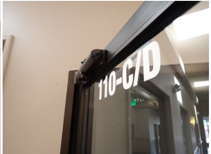
Unit 110C&D: Unit was vacant. Floor settling/deflection noted. Recommend repairs as needed by a licensed contractor.
