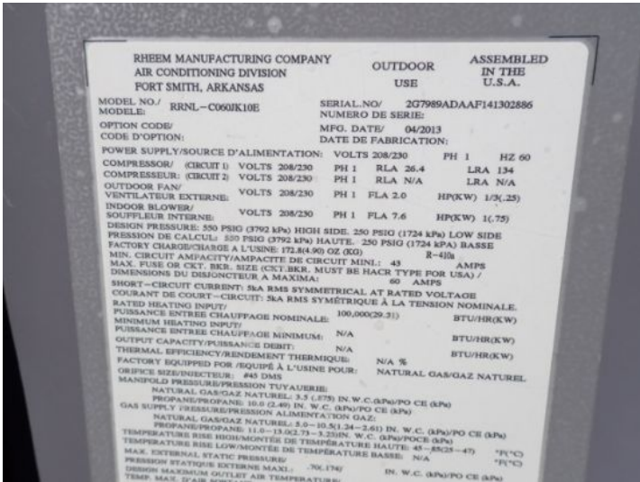
RTU 6: Rheem: M/N RRNL-C060JK10E S/N 2G7989ADAAF141302886. Manufacture year 2013.
