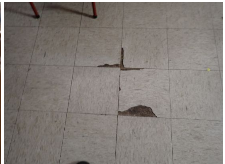
Unit 121: VCT flooring damage noted. Recommend repairs.
