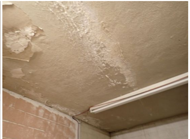
Unit 103: VCT flooring damage noted. Moisture staining noted in ceiling tiles. Moisture damage noted in rear ceiling. Recommend repairs.
