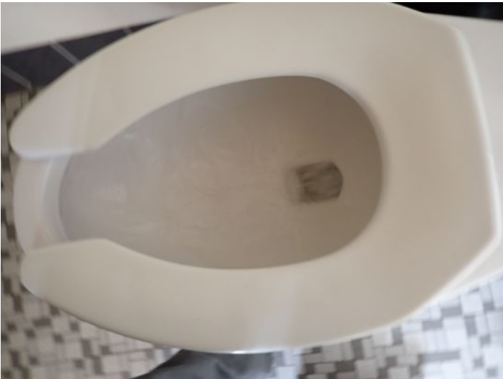
The common area restrooms in the office building and mall areas were tested and functional at the time of the inspection.
