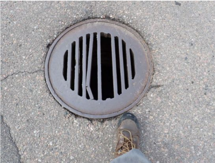
Damaged drainage vent cover noted in the front parking lot area that could be considered a safety hazard. Recommend repairs by a licensed contractor.
