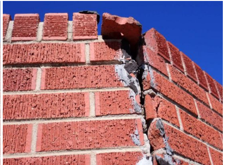
Minor brick damaged and movement noted in the brick siding material at the awning area between the structures. Recommend repairs by a licensed contractor.
