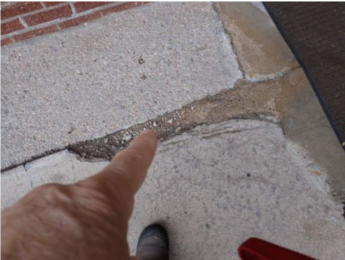
Damage/heaving noted on the flatwork at the ADA ramp for unit 100 (restaurant) at the time of the inspection. Recommend repairs by a licensed contractor.
