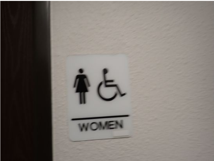
The common area restrooms in the office building and mall areas were tested and functional at the time of the inspection.
