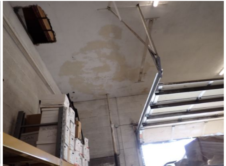
Unit 111-112: Moisture staining noted in ceiling tiles. Moisture damage noted in warehouse ceiling. Water heater not functional. Drywall ceiling damage noted. Recommend repairs.
