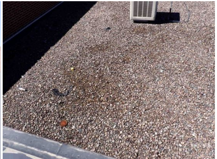
The gravel coated EPDM roofing membrane located towards the north end of the west structure was showing signs of significant ponding and deferred maintenance at the time of the inspection. Recommend repair by licensed contractor.
