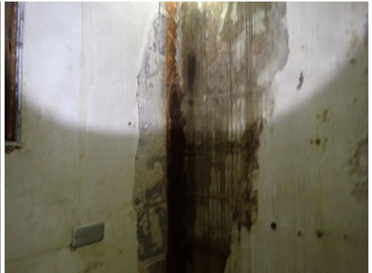
Unit 108-107: Vacant: Unit will require significant renovations prior to installing tenant. Active moisture noted in interior wall with possible microbial growth. Significant drywall damage noted in ceiling and walls in loading dock area. Basement area in poor condition. Basement bathrooms in poor condition. Electrical not working at the time of the inspection. Moisture intrusion/damage noted in basement walls. Recommend repairs as needed by a licensed contractor.
