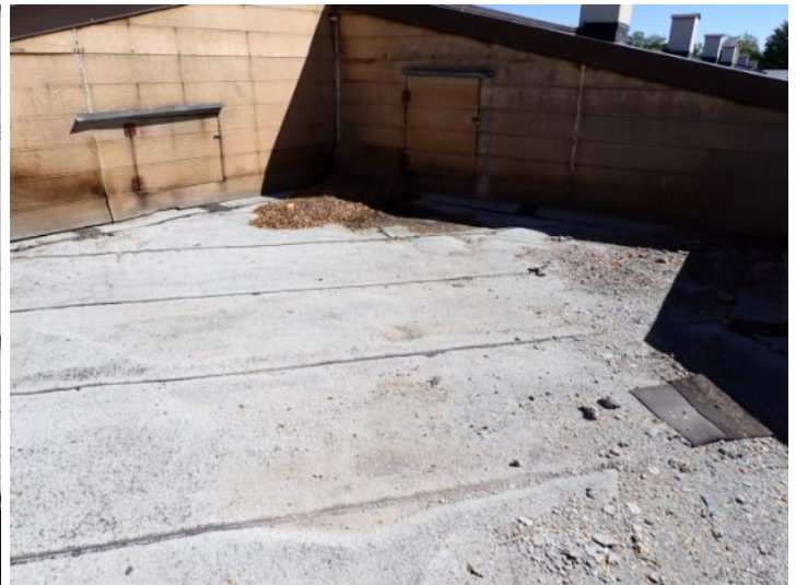
The rolled asphalt composition roof and system located above the awning between the two wings was in extremely poor condition why is it a plate replacement. Recommend repair by a licensed contractor.
