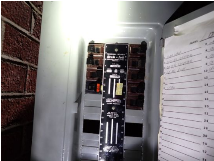
Old Federal Pacific Stab Lock breaker systems noted in some of the units at the time of the inspection. These systems have been proven to be safety/fire issues. Recommend replacement of all FPE panels and stab lock breaker systems by a licensed contractor prior to taking possession of the property.
