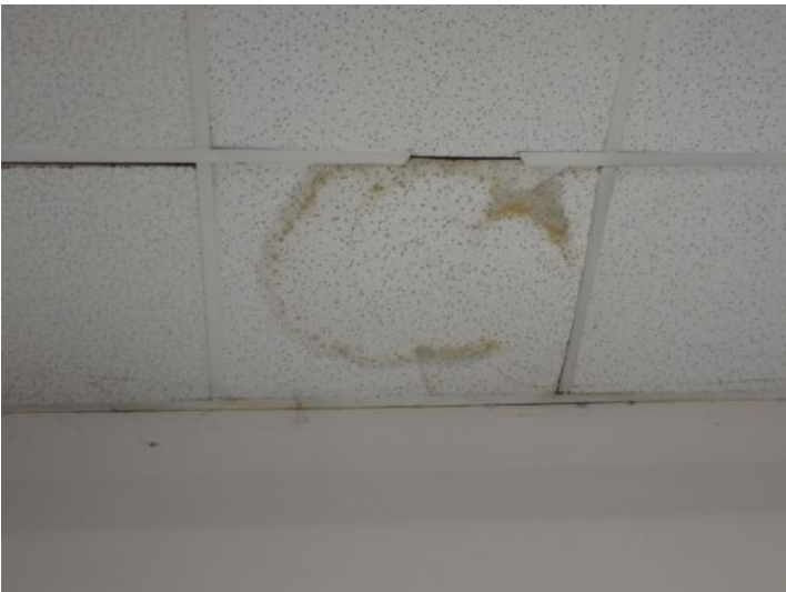
Unit 111-112: Moisture staining noted in ceiling tiles. Moisture damage noted in warehouse ceiling. Water heater not functional. Drywall ceiling damage noted. Recommend repairs.
