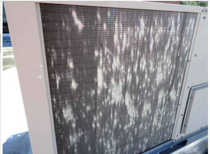
Significant hail damage noted on the cooling fins on RTU 8 at the time of the inspection. Recommend repairs by a licensed contractor.
