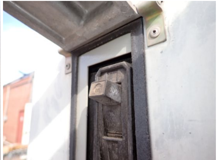
The main electrical disconnects appeared functional at the time of the inspection.
