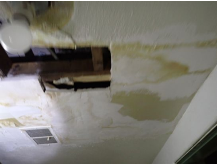
Unit 108-107: Vacant: Unit will require significant renovations prior to installing tenant. Active moisture noted in interior wall with possible microbial growth. Significant drywall damage noted in ceiling and walls in loading dock area. Basement area in poor condition. Basement bathrooms in poor condition. Electrical not working at the time of the inspection. Moisture intrusion/damage noted in basement walls. Recommend repairs as needed by a licensed contractor.
