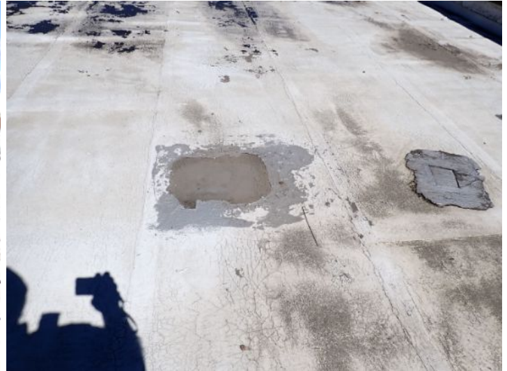
The rolled torch down roofing system above what appeared to be the old family dollar store and the vacant unit was an extremely poor condition excessive ponding feeling coding possible hail damage and excessive wear noted at the time of the inspection. Recommend complete replacement by licensed contractor.
