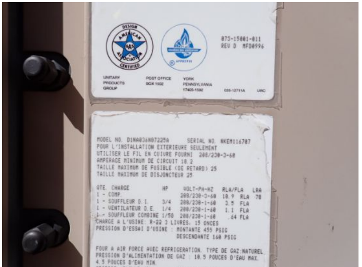
The nominal serviceable life expectancy of an RTU is 15 years. Based on the age of one or more of the RTU's they have neared or surpassed their serviceable life expectancy. Recommend replacement or budgeting for replacement of these units in the near future.
