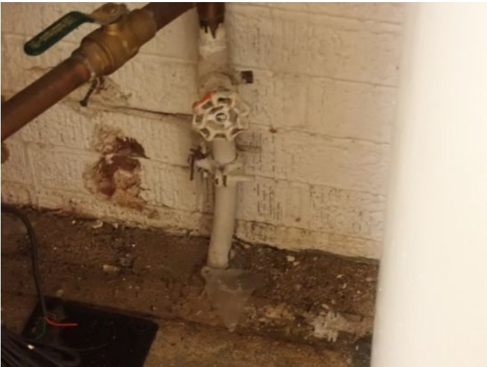
Several shutoff valves were noted in tenant units that did not have backflow preventers installed on them but appeared to be metered. Recommend repairs as needed by a licensed contractor.
