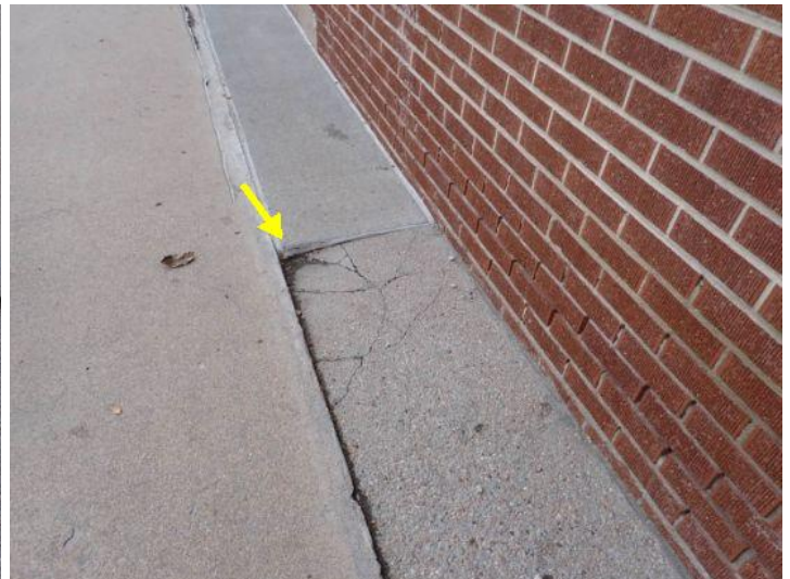
Trip hazards noted. Recommend repairs.
