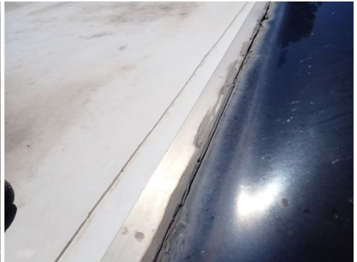
Skylight systems require sealant repairs. Recommend repairs by a licensed contractor.
