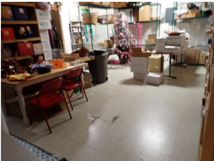
Unit 121: VCT flooring damage noted. Recommend repairs.
