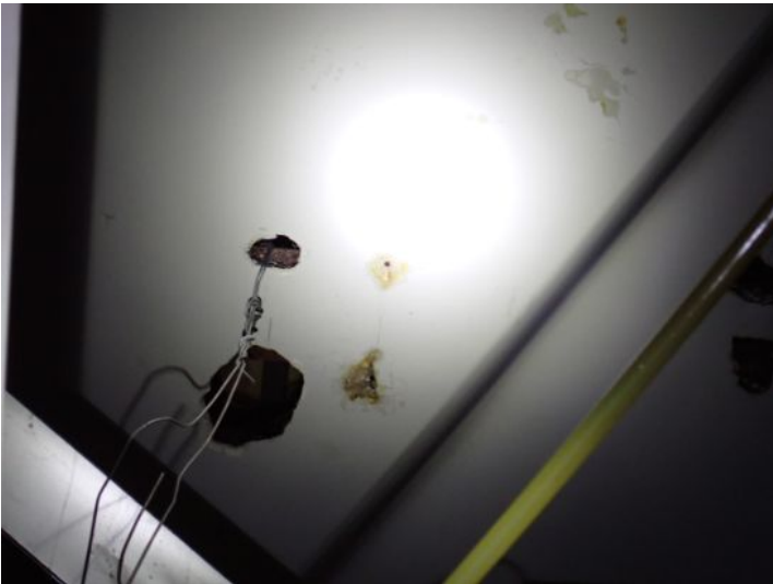
Unit 110A: Moisture staining noted in ceilings. Recommend repairs.
