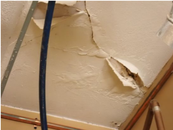
Unit 118: Moisture staining noted in ceiling. Moisture damage noted in drywall ceiling. Recommend repairs and monitoring.
