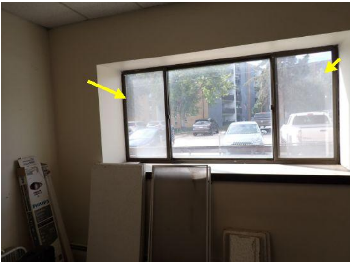
Failed seals noted in multiple insulated window units at the time of the inspection. Recommend repairs by a licensed contractor.
