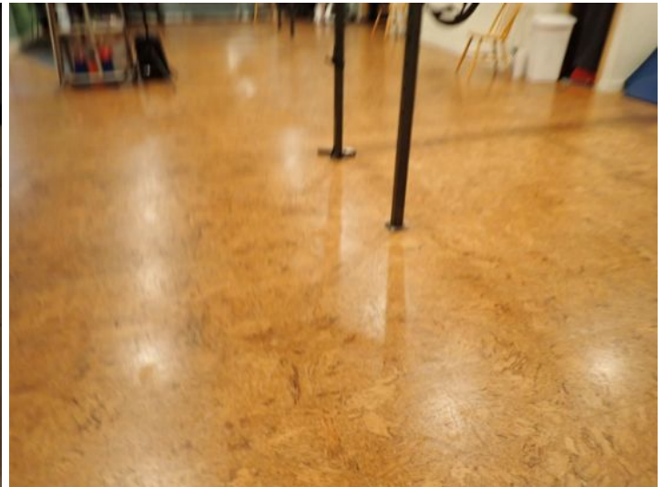
Unit 110B: No significant findings noted at the time of the inspection
