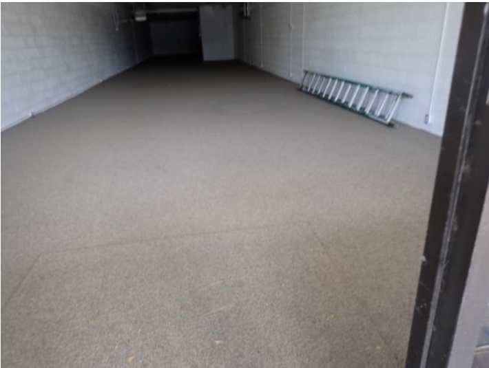
Unit 105: Vacant Unit: No significant findings noted at the time of the inspection
