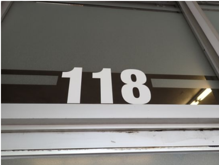
Unit 118: Moisture staining noted in ceiling. Moisture damage noted in drywall ceiling. Recommend repairs and monitoring.
