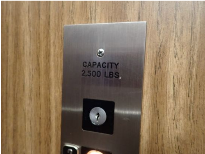
The elevator system in the office building was tested and functional at the time of the inspection.
