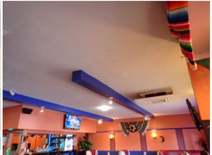
Unit 120: Old Santa Fe Restaurant: No significant findings noted at the time of the inspection
