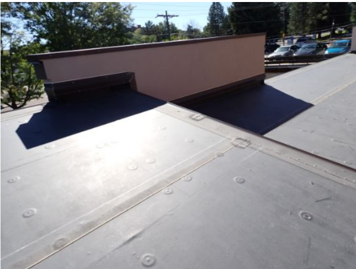
The EPDM membrane on the low slope front sections of each wing appeared be in fair condition at time of inspection. There were areas where it appeared that debris below the membrane was attempting to push through the membrane but had not penetrated at the time of the inspection. Recommend monitoring for future repairs.
