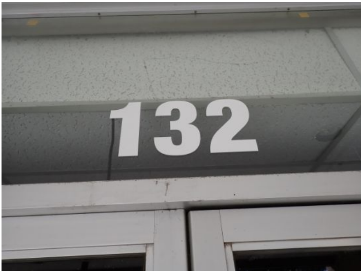
Unit 132: Unit was in poor condition and will require complete renovations prior to installing a new tenant.
