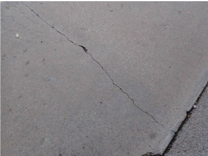
Minor cracking. Recommend monitoring for future repairs.
