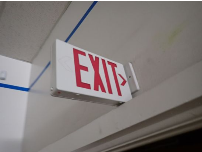
Multiple lighted EXIT signs still have the old red lenses. Many municipalities are now requiring the lenses to be green for better viewing during a fire. Recommend budgeting for replacement of any required units.
