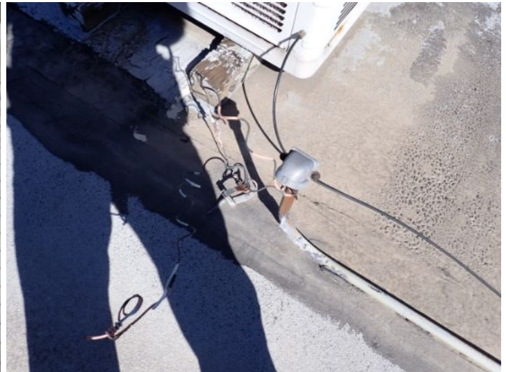
Exposed electrical wiring noted in areas around the exterior and on the roof of the structure at the time of the inspection. Recommend proper repairs by a licensed electrician.
