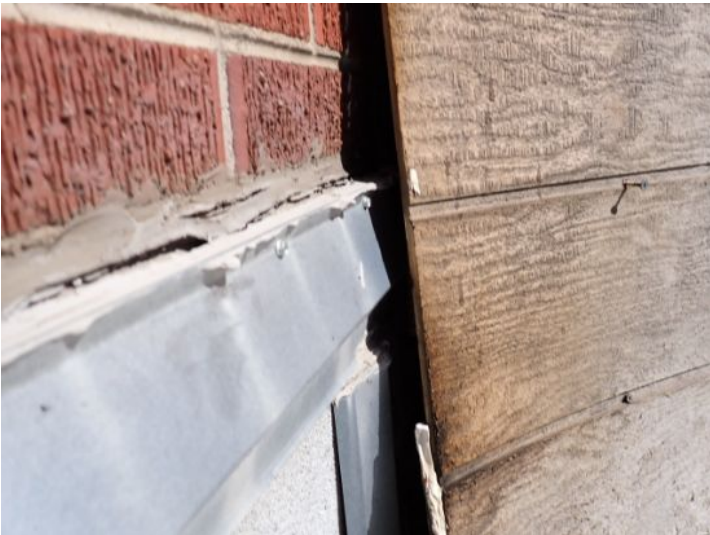
The wood siding material located above the corner awning roof on the ends of the pitched roof sections were in poor condition at the time of the inspection. Recommend repairs by a licensed contractor.
