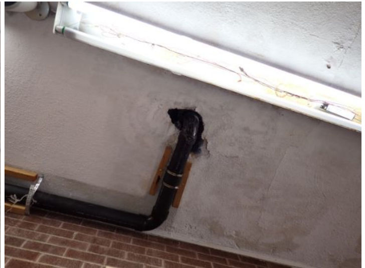
Unit 101: Active leak noted coming from roof drain. Restroom in poor condition. Recommend repairs.
