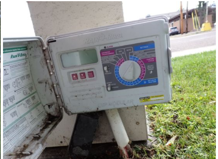
The property had an irrigation system at the time of the inspection.
