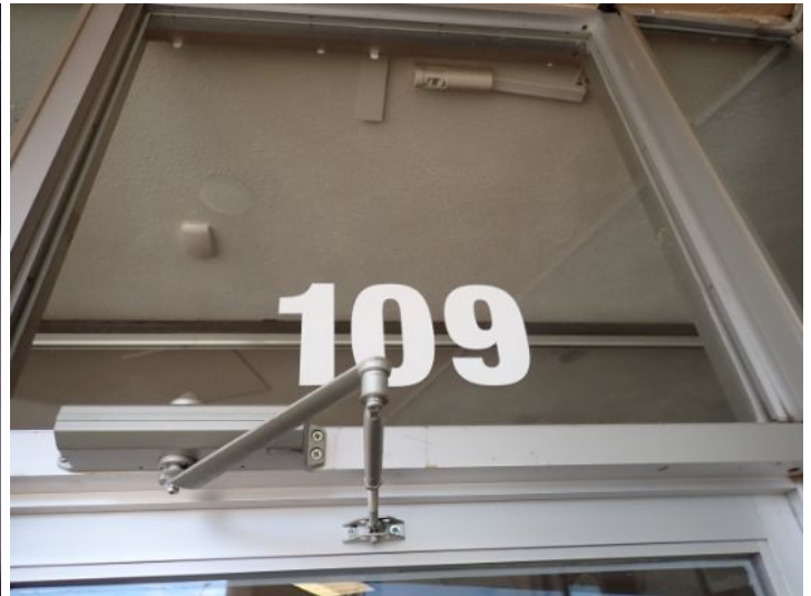
Unit 109: Past moisture staining noted in ceiling tiles. Recommend repairs.
