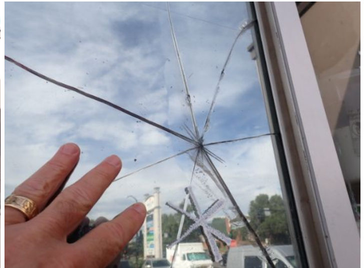
Cracked/broken window glass noted on the front of unit 100 (restaurant) at the time of the inspection. Recommend repairs by a licensed contractor.
