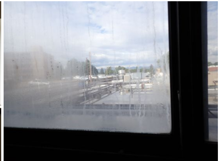
Failed seals noted in multiple insulated window units at the time of the inspection. Recommend repairs by a licensed contractor.
