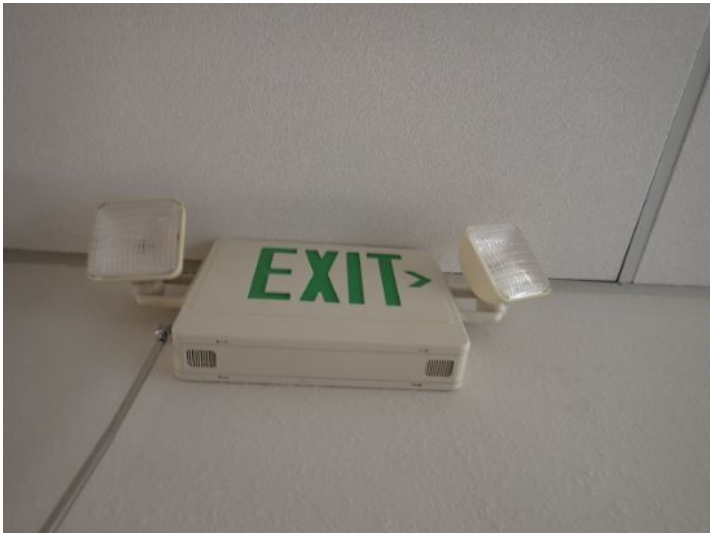
Multiple emergency lighting systems failed when tested at the time of the inspection. Recommend repairs as needed by a licensed contractor.
