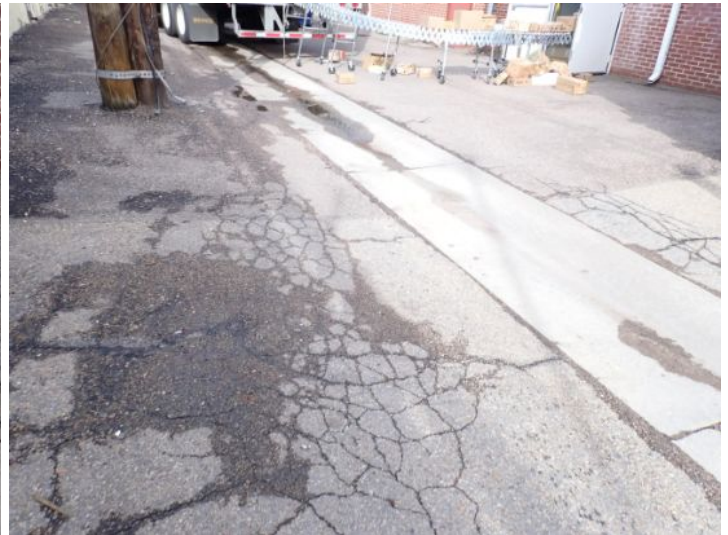
The asphalt running along the rear south side of the structure was in poor condition at the time of the inspection. Recommend resurfacing by a licensed contractor.
