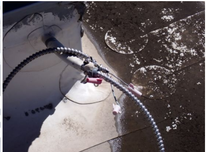
Exposed electrical wiring noted in areas around the exterior and on the roof of the structure at the time of the inspection. Recommend proper repairs by a licensed electrician.
