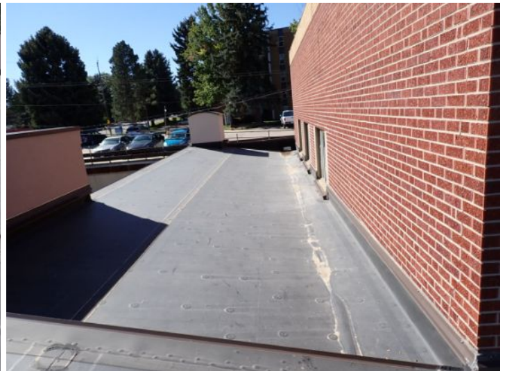
The EPDM membrane on the low slope front sections of each wing appeared be in fair condition at time of inspection. There were areas where it appeared that debris below the membrane was attempting to push through the membrane but had not penetrated at the time of the inspection. Recommend monitoring for future repairs.
