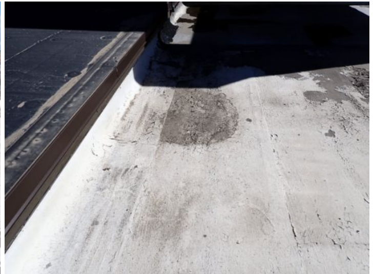
The rolled torch down roofing membrane located above the fitness center on the north end of the west wing was an extremely poor condition and has reached the end of the service for life expectancy. Recommend complete replacement by licensed roofing contractor.
