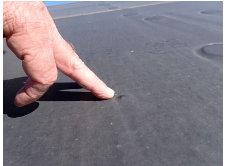
The EPDM membrane on the low slope front sections of each wing appeared be in fair condition at time of inspection. There were areas where it appeared that debris below the membrane was attempting to push through the membrane but had not penetrated at the time of the inspection. Recommend monitoring for future repairs.
