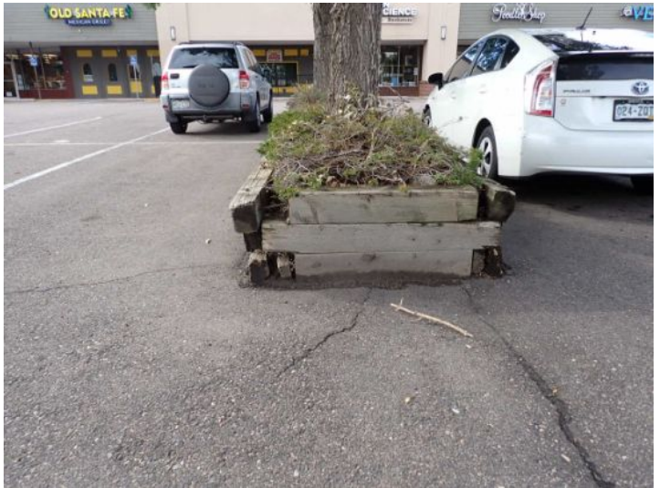
The timber retaining walls located around the planning beds in the parking lot were in poor condition at the time of the inspection. Recommend repairs by a licensed contractor.
