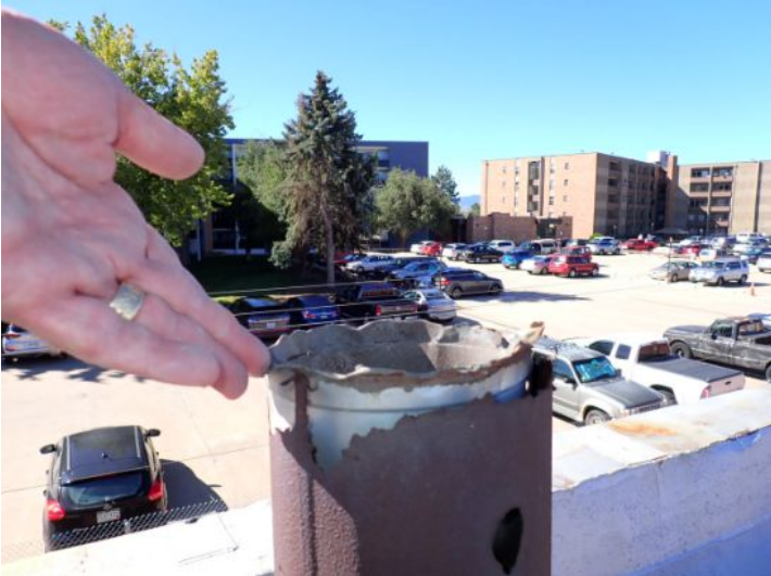
Missing boiler vent stack cover noted on the upper level of the building of time and inspection. Recommend repair by licensed contractor.
