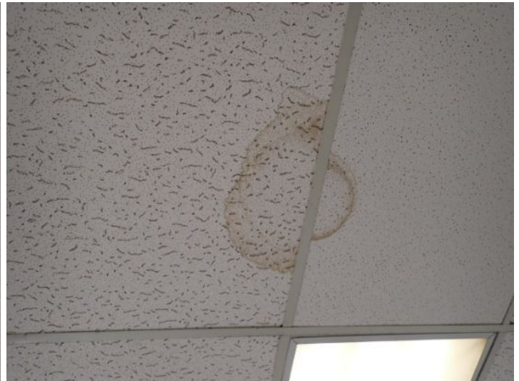
Moisture staining noted in areas of the acoustical tile ceilings throughout the building at the time of the inspection. Recommend repairs and monitoring
