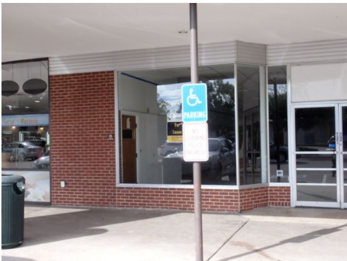
Missing safety stamps noted on some of the required safety glass panels. This is typical of structures of this age. Today's standards require that any glass located within 18" of grade level next to a walkway, in an operable door, with a leaking edge within 24" of an operable door or with a total of 9 sq. ft. or larger be glazed with safety glass and be labeled as such. Recommend repairs as needed by a certified glazing contractor.
