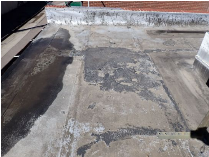
The rolled torch down roofing system located on the lower level south wing of the structure showing signs of excessive deferred maintenance, excessive ponding, possible hail damage and age. Recommend complete replacement by licensed contractor.
