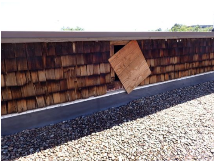
Bird and possible rodent nesting noted in the low slope front area above the unit next to the lifetime fitness center at time of inspection. Loose access panel noted at that time. Recommend bird and rodent removal cleaning of the interior of the area and repairs to the access panel by licensed contractor.
