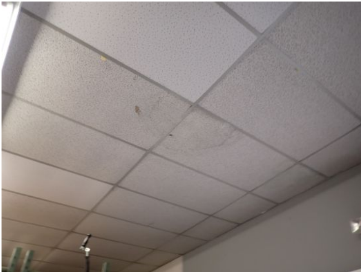
Unit 111-112: Moisture staining noted in ceiling tiles. Moisture damage noted in warehouse ceiling. Water heater not functional. Drywall ceiling damage noted. Recommend repairs.
