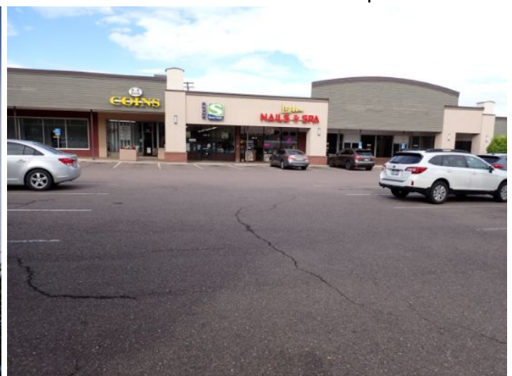
The majority of the parking lot surface was in fair condition at the time of the inspection.
