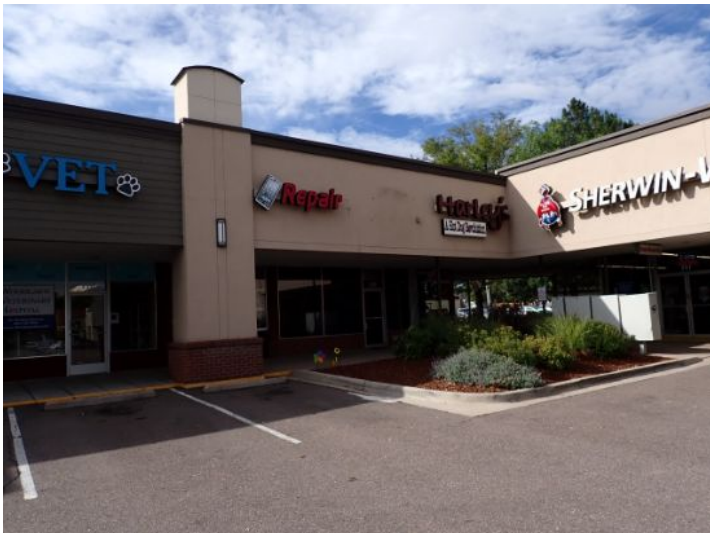
The majority of the exterior envelope of the structure appeared to be in fair condition with no significant structural movement noted at the time of the inspection.
