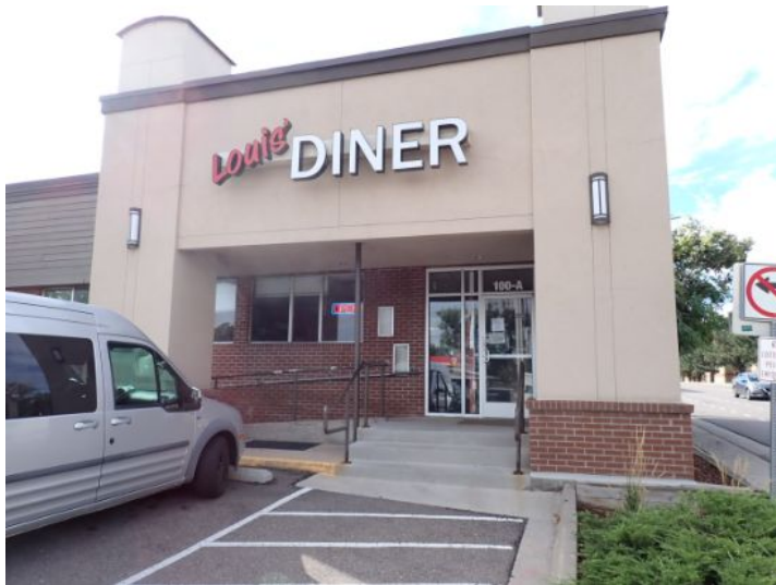
The majority of the exterior envelope of the structure appeared to be in fair condition with no significant structural movement noted at the time of the inspection.
