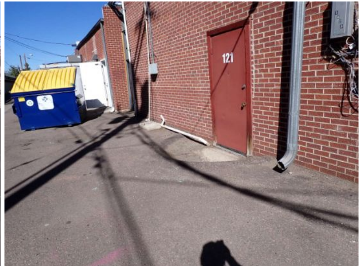
The majority of the exterior envelope of the structure appeared to be in fair condition with no significant structural movement noted at the time of the inspection.
