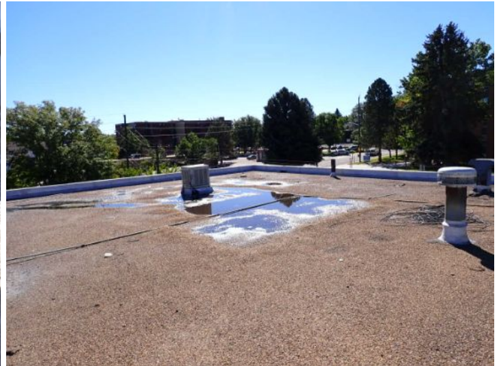
The BUR roofing system located on the east end of the south wing of the building is showing signs of excessive wear excessive ponding it was an extremely poor condition at the time of the inspection. Recommend replacement by a licensed contractor.
