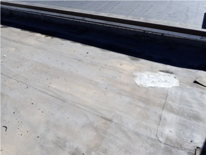
The rolled torch down roofing system located above the east end of the south wing appear did reach the end of its serviceable life expectancy with areas of significant ponding and cracking noted. Recommend repairs/replacement by licensed contractor.
