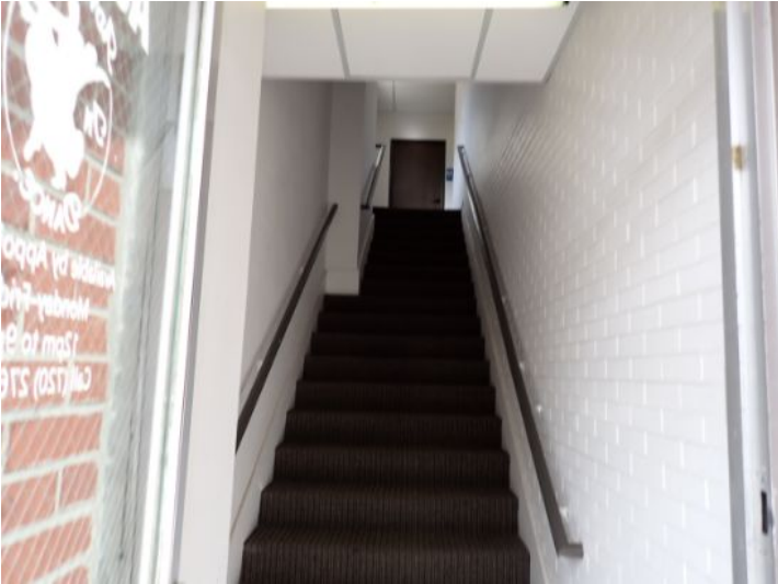
The majority of the interior common areas of the structure appeared to be in fair condition at the time of the inspection.
