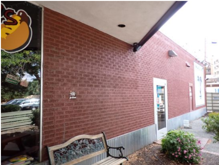
The majority of the exterior envelope of the structure appeared to be in fair condition with no significant structural movement noted at the time of the inspection.
