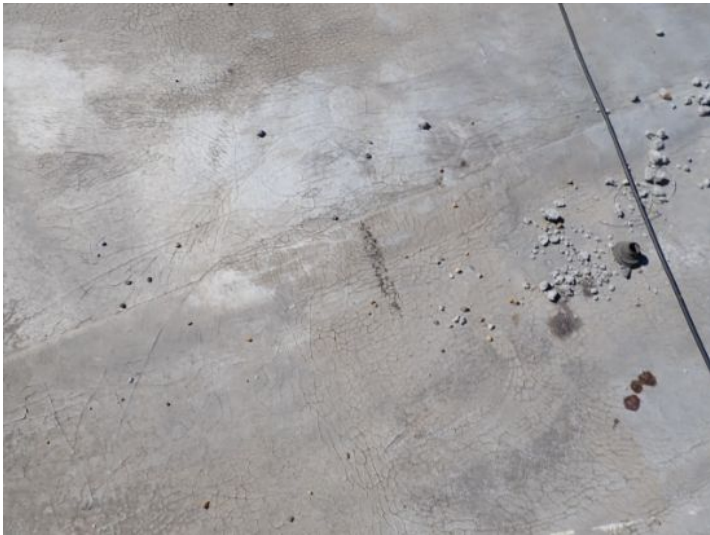
The rolled torch down roofing system located on the lower level south wing of the structure showing signs of excessive deferred maintenance, excessive ponding, possible hail damage and age. Recommend complete replacement by licensed contractor.
