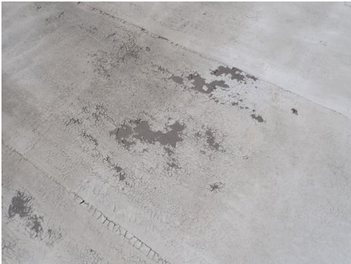
The rolled torch down roofing system above what appeared to be the old family dollar store and the vacant unit was an extremely poor condition excessive ponding feeling coding possible hail damage and excessive wear noted at the time of the inspection. Recommend complete replacement by licensed contractor.
