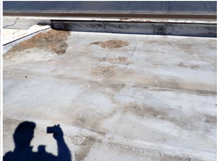
The rolled torch down roofing system located on the lower level south wing of the structure showing signs of excessive deferred maintenance, excessive ponding, possible hail damage and age. Recommend complete replacement by licensed contractor.
