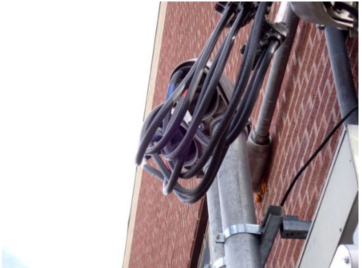
The main electrical system was a 3 phase 4 wire system
