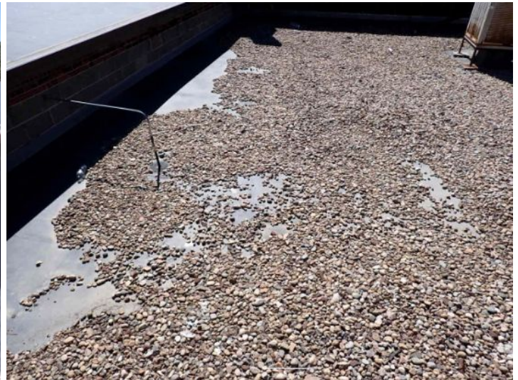
The gravel coated EPDM roofing membrane located towards the north end of the west structure was showing signs of significant ponding and deferred maintenance at the time of the inspection. Recommend repair by licensed contractor.
