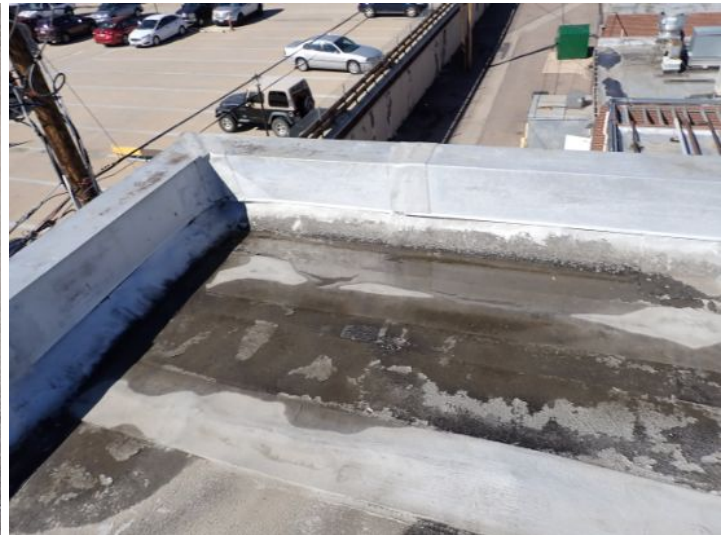
The rolled torch down roofing system above what used to be the old theater it is now currently being used as the office area appeared to be original to the structure and was showing signs of hail damage excessive ponding where and patching. Recommend replacement by licensed contractor.
