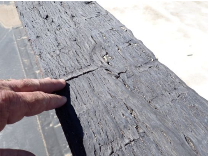
Recommend capping of all brick/block parapet walls with metal capping material. Recommend repairs by a licensed contractor.
