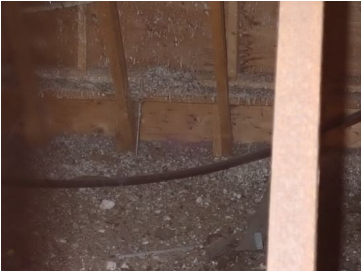
Bird and possible rodent nesting noted in the low slope front area above the unit next to the lifetime fitness center at time of inspection. Loose access panel noted at that time. Recommend bird and rodent removal cleaning of the interior of the area and repairs to the access panel by licensed contractor.
