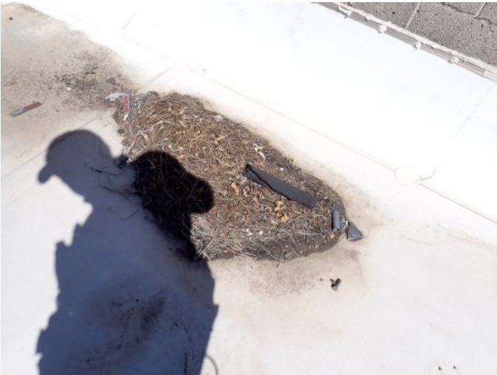
TPO roofing membrane located above the mall area of the property while appearing to be in fair condition was showing signs of excessive deferred maintenance and ponding at the time of the inspection. Recommend repairs by licensed contractor.
