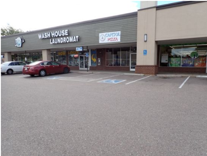
The majority of the parking lot surface was in fair condition at the time of the inspection.
