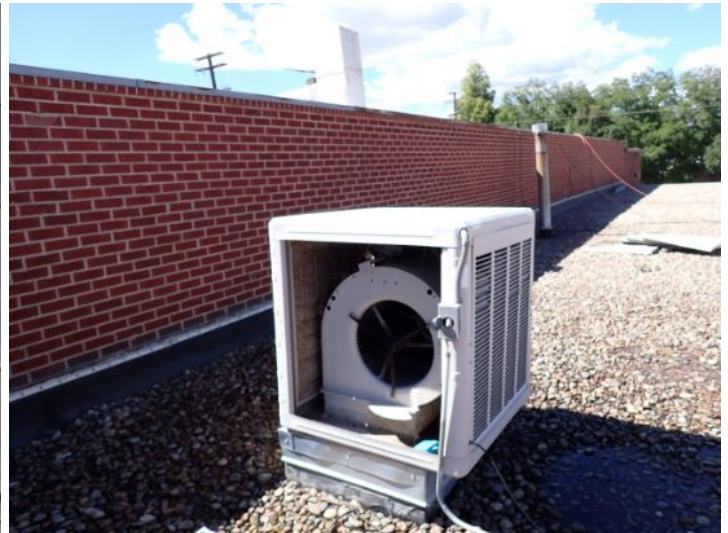
The swamp coolers located on the top of the gravel coated EPDM roofing system located on the north end of the west wing or poor condition in that social time of the inspection. These units are no longer in service we recommend removal.
