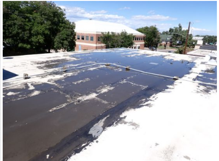
The rolled torch down roofing system above what appeared to be the old family dollar store and the vacant unit was an extremely poor condition excessive ponding feeling coding possible hail damage and excessive wear noted at the time of the inspection. Recommend complete replacement by licensed contractor.
