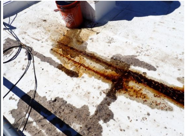
One or more kitchen roof top vent systems were showing signs of significant deferred maintenance. Recommend repairs by a licensed contractor.
