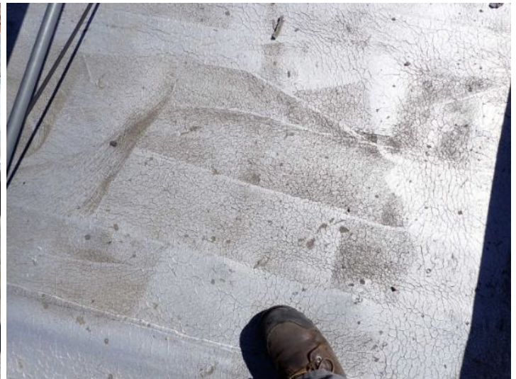
The rolled torch down roofing system located on the lower level south wing of the structure showing signs of excessive deferred maintenance, excessive ponding, possible hail damage and age. Recommend complete replacement by licensed contractor.
