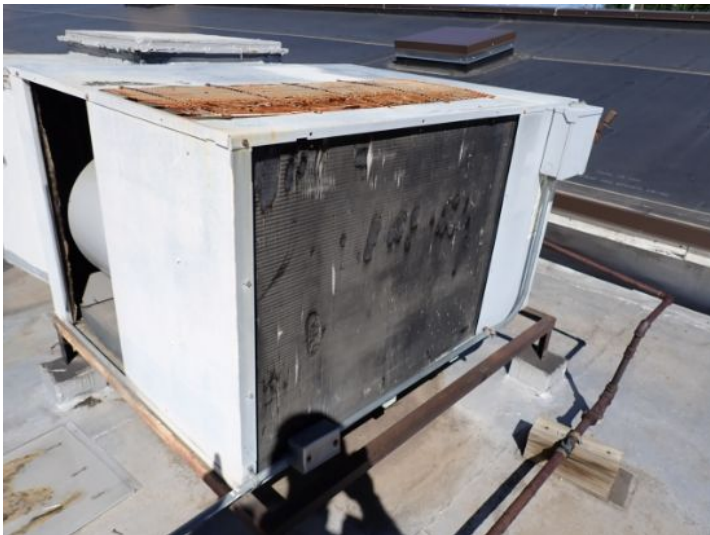
RTU 10 was in extremely poor condition and requires replacement. Recommend replacement by a licensed contractor.
