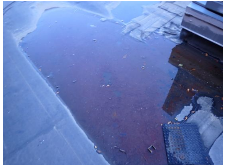
The EPDM roofing membrane located on the lower level of the south wing appeared to be in fair condition at the time of the inspection but was showing signs of excessive ponding and minor seam issues in areas. Recommend repairs as required by a licensed contractor.
