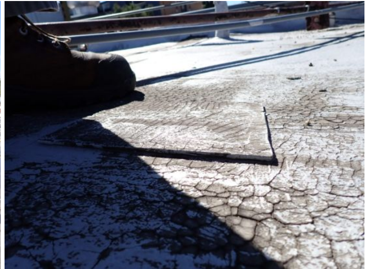
The rolled torch down roofing system located on the lower level south wing of the structure showing signs of excessive deferred maintenance, excessive ponding, possible hail damage and age. Recommend complete replacement by licensed contractor.
