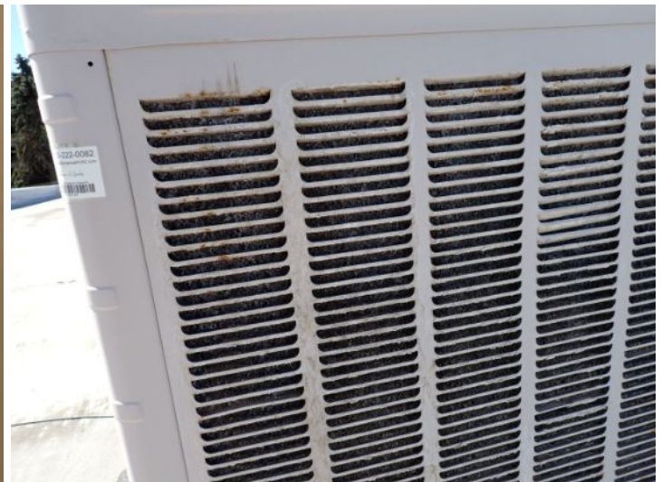
The swamp coolers located above the old theater area that is now being used as office or in fair to poor condition and require servicing and filter repairs by a licensed contractor. Recommend repairs prior to taking possession of the property.
