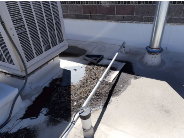
TPO roofing membrane located above the mall area of the property while appearing to be in fair condition was showing signs of excessive deferred maintenance and ponding at the time of the inspection. Recommend repairs by licensed contractor.
