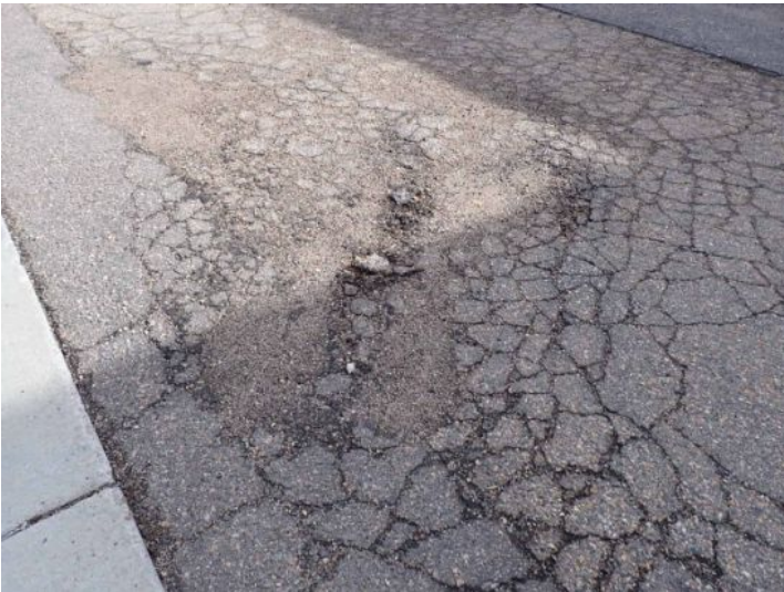
The asphalt running along the rear west side of the structure was in poor condition at the time of the inspection. Recommend resurfacing by a licensed contractor.
