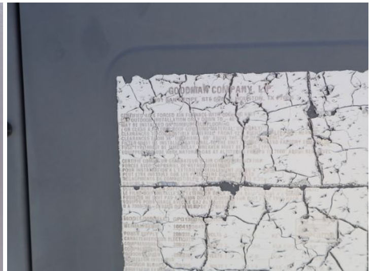
RTU 19: Goodman: M/N GPG13601? S/N 1004123649. Manufacture year 2010.
