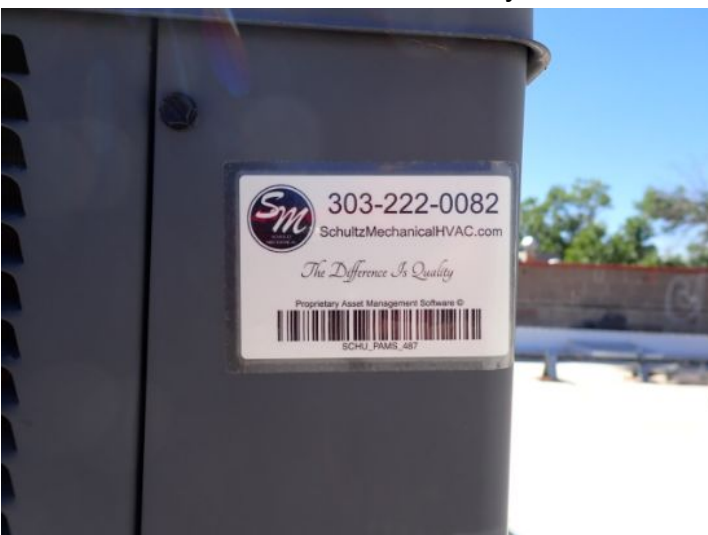
The hvac systems appeared to be being serviced by Shultz Mechanical 303-222-0082.
