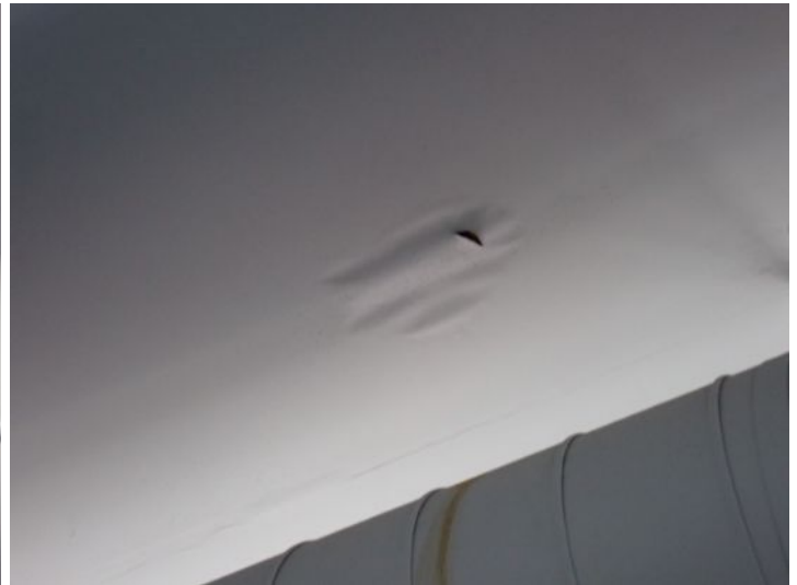
Unit 100: Active moisture damage and roof leaking noted. Recommend repairs.
