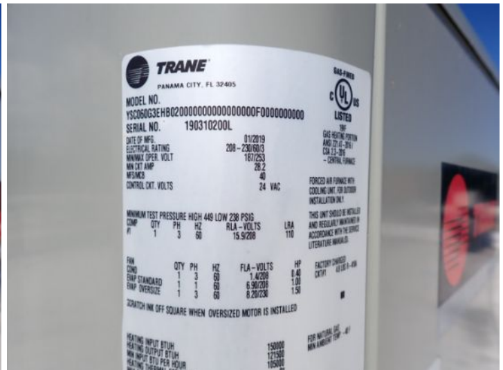
RTU 24: Trane: M/N YSC060G3EHB0200000 S/N 190310200L. Manufacture year 2019.
