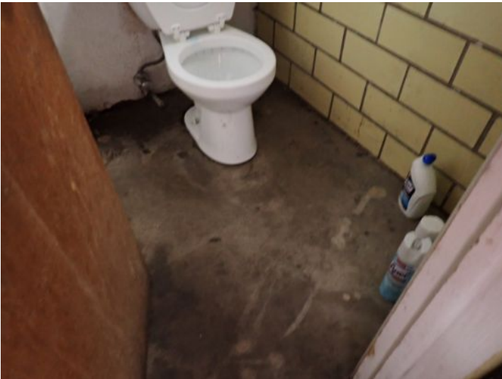
Unit 101: Active leak noted coming from roof drain. Restroom in poor condition. Recommend repairs.
