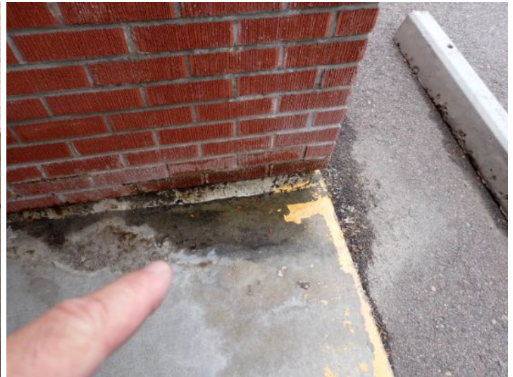
Due to flashing issues storm water was getting into one of the stucco awning support pillars and running down the inside of the system. Recommend repairs as needed by a licensed contractor.
