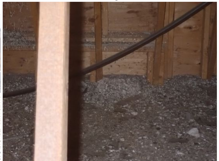
Bird and possible rodent nesting noted in the low slope front area above the unit next to the lifetime fitness center at time of inspection. Loose access panel noted at that time. Recommend bird and rodent removal cleaning of the interior of the area and repairs to the access panel by licensed contractor.
