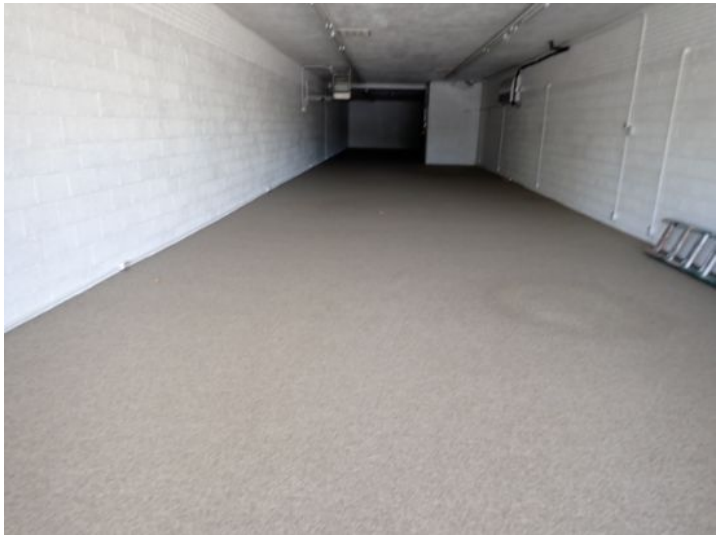
Unit 105: Vacant Unit: No significant findings noted at the time of the inspection
