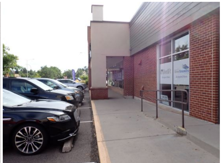
The majority of the exterior envelope of the structure appeared to be in fair condition with no significant structural movement noted at the time of the inspection.
