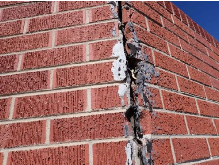
Minor brick damaged and movement noted in the brick siding material at the awning area between the structures. Recommend repairs by a licensed contractor.
