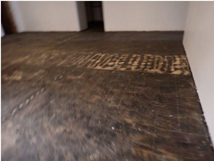
Unit 110C&D: Unit was vacant. Floor settling/deflection noted. Recommend repairs as needed by a licensed contractor.
