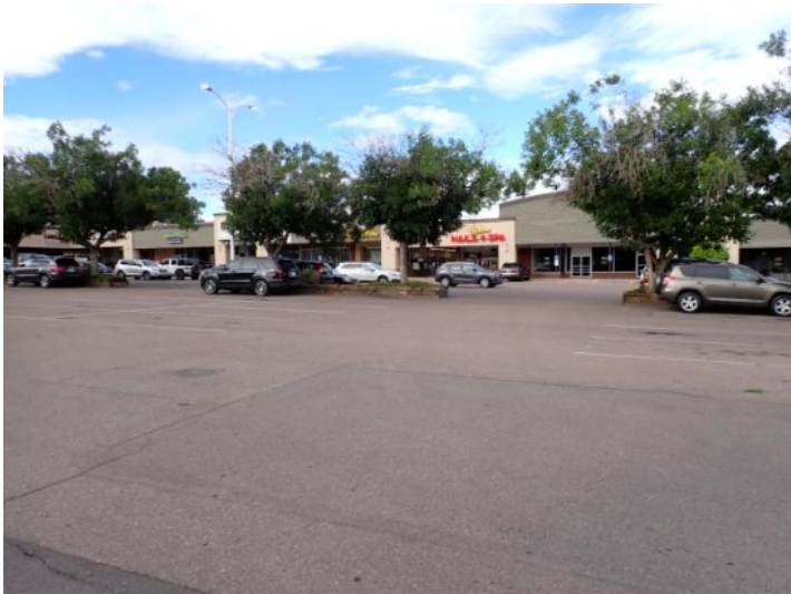
The majority of the parking lot surface was in fair condition at the time of the inspection.
