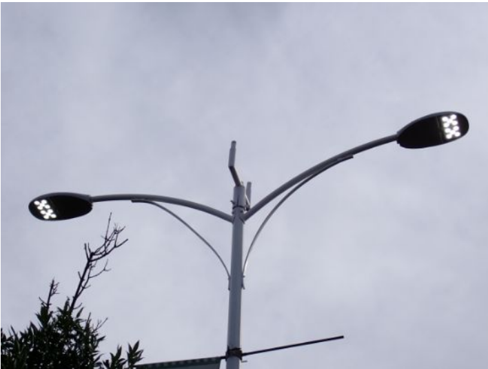
Parking lot lighting system appeared functional at the time of the inspection.
