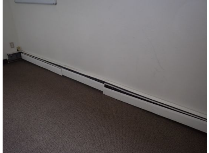
The majority of the interior offices, that were accessible at the time of the inspection, appeared to be in fair condition at the time of the inspection.
