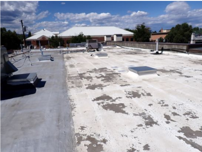
The rolled torch down roofing membrane located above the fitness center on the north end of the west wing was an extremely poor condition and has reached the end of the service for life expectancy. Recommend complete replacement by licensed roofing contractor.
