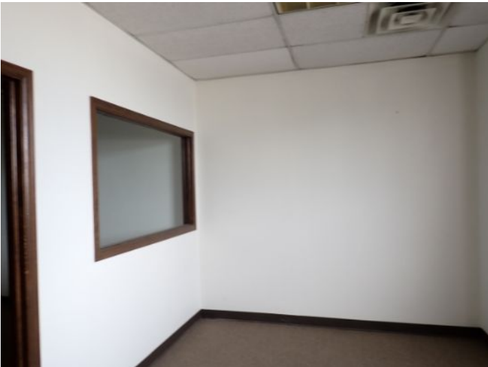
The majority of the interior offices, that were accessible at the time of the inspection, appeared to be in fair condition at the time of the inspection.
