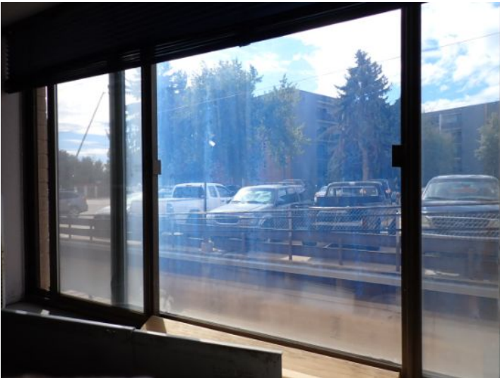
Failed seals noted in multiple insulated window units at the time of the inspection. Recommend repairs by a licensed contractor.
