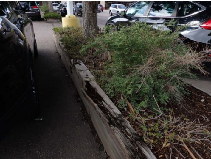
The timber retaining walls located around the planning beds in the parking lot were in poor condition at the time of the inspection. Recommend repairs by a licensed contractor.
