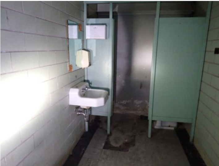
Unit 108-107: Vacant: Unit will require significant renovations prior to installing tenant. Active moisture noted in interior wall with possible microbial growth. Significant drywall damage noted in ceiling and walls in loading dock area. Basement area in poor condition. Basement bathrooms in poor condition. Electrical not working at the time of the inspection. Moisture intrusion/damage noted in basement walls. Recommend repairs as needed by a licensed contractor.
