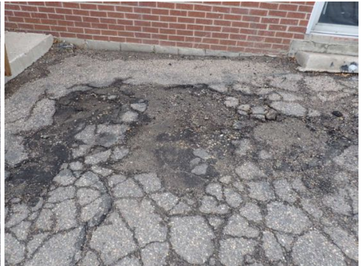
The asphalt running along the rear west side of the structure was in poor condition at the time of the inspection. Recommend resurfacing by a licensed contractor.
