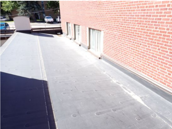
The EPDM membrane on the low slope front sections of each wing appeared be in fair condition at time of inspection. There were areas where it appeared that debris below the membrane was attempting to push through the membrane but had not penetrated at the time of the inspection. Recommend monitoring for future repairs.
