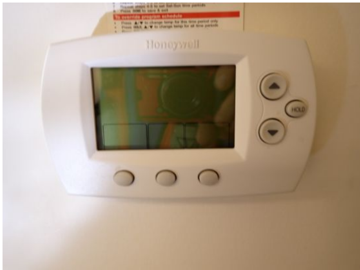
One or more thermostats not responding at the time of the inspection. Recommend repairs by a licensed contractor prior to taking possession of the property.
