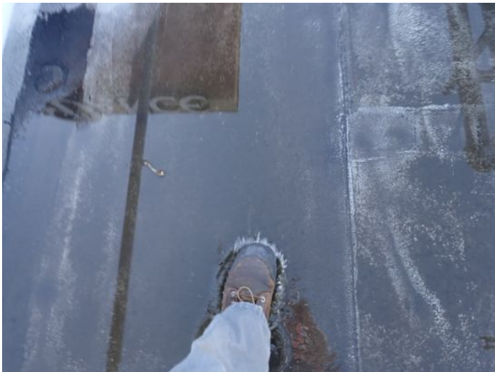
The rolled torch down roofing system located on the lower level south wing of the structure showing signs of excessive deferred maintenance, excessive ponding, possible hail damage and age. Recommend complete replacement by licensed contractor.
