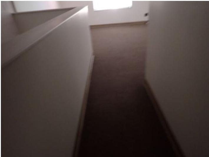
Unit 111B: Emergency egress goes through unit 111 which is locked at night. Recommend repairs by a licensed contractor prior to installing a new tenant.
