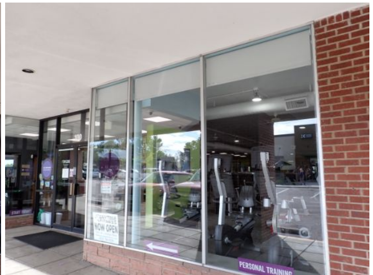
The majority of the exterior envelope of the structure appeared to be in fair condition with no significant structural movement noted at the time of the inspection.
