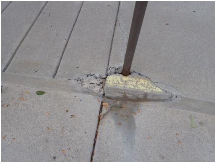
Concrete damage/deterioration noted in areas. Recommend repairs by a licensed contractor.
