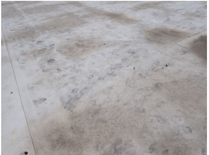
TPO roofing membrane located above the mall area of the property while appearing to be in fair condition was showing signs of excessive deferred maintenance and ponding at the time of the inspection. Recommend repairs by licensed contractor.
