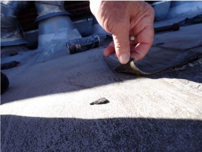
The rolled torch down roofing system located above the east end of the south wing appeared to have reached the end of its serviceable life expectancy with areas of significant ponding and cracking noted. Recommend repairs/replacement by licensed contractor.
