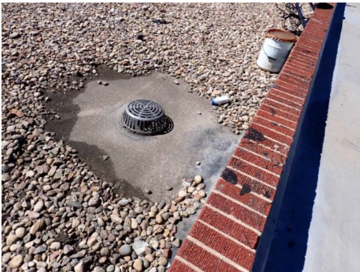
The gravel coated EPDM roofing membrane located towards the north end of the west structure was showing signs of significant ponding and deferred maintenance at the time of the inspection. Recommend repair by licensed contractor.
