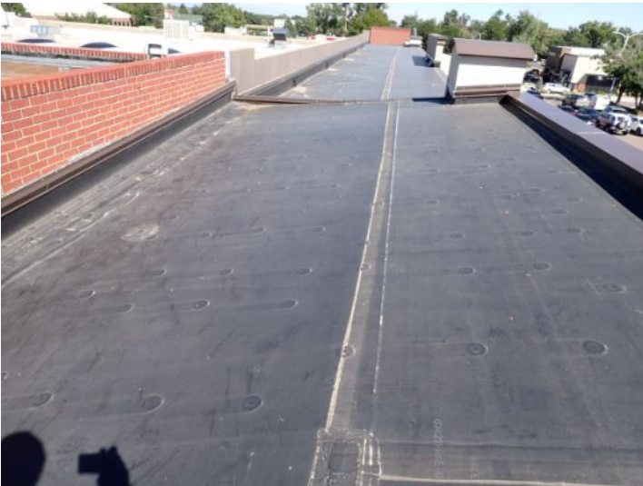
The EPDM membrane on the low slope front sections of each wing appeared to be in fair condition at time of inspection. There were areas where it appeared that debris below the membrane was attempting to push through the membrane but had not penetrated at the time of the inspection. Recommend monitoring for future repairs.
