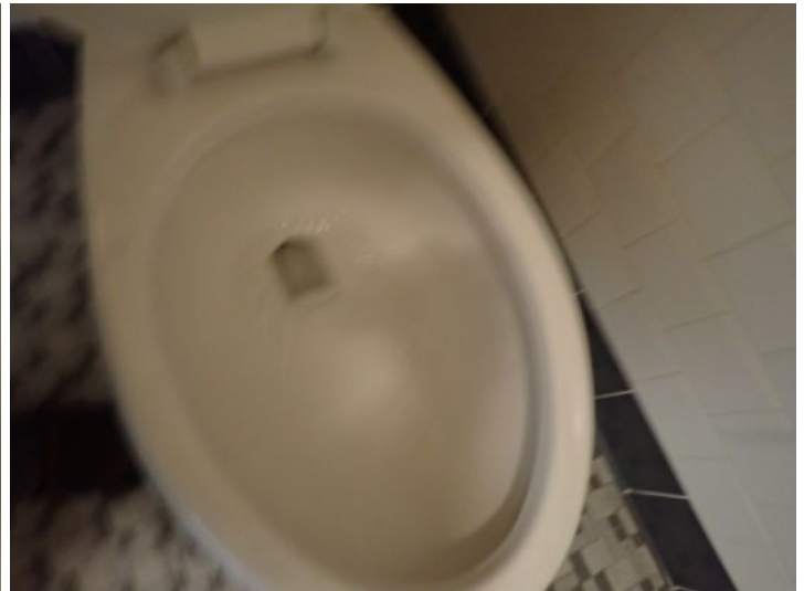
The common area restrooms in the office building and mall areas were tested and functional at the time of the inspection.
