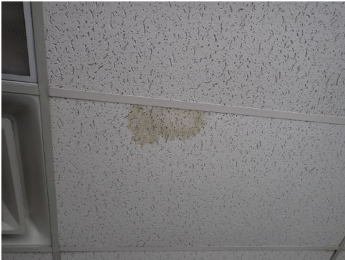
Moisture staining noted in areas of the acoustical tile ceilings throughout the building at the time of the inspection. Recommend repairs and monitoring
