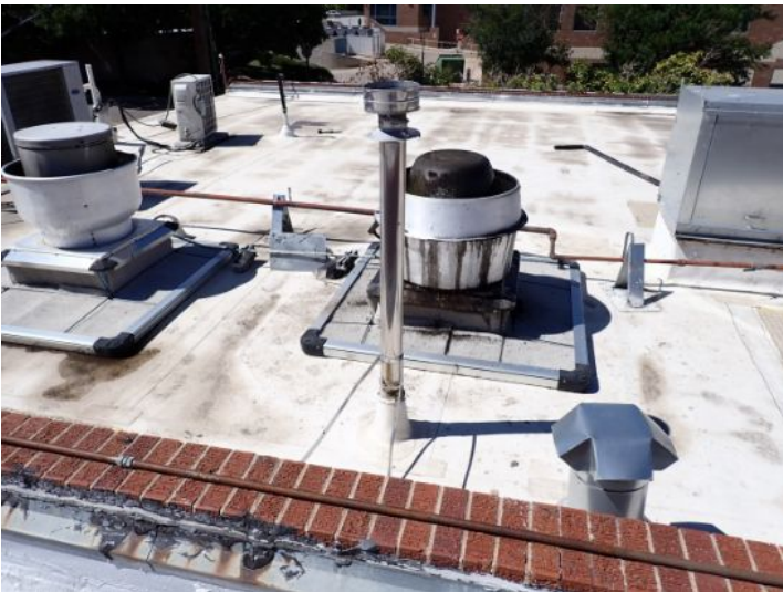
The TPO membrane located above the restaurant on the north end of the West Wing appear to be in fair condition at time of inspection.
