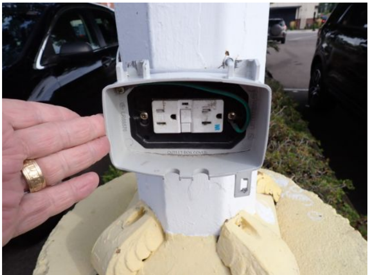
Missing weather cover noted in parking lot area. Recommend repairs by a licensed contractor.
