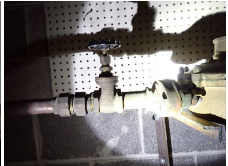
The old fire suppression system located in the basement below the large vacant unit will most likely require updating prior to placing a tenant in the unit. Recommend consulting with the current management company and local fire marshal concerning this matter as updating of fire suppression and alarm systems could be considered a significant capital investment.
