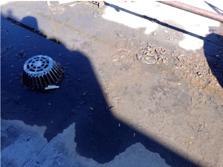
The rolled torch down roofing system located above the east end of the south wing appeared to have reached the end of its serviceable life expectancy with areas of significant ponding and cracking noted. Recommend repairs/replacement by licensed contractor.
