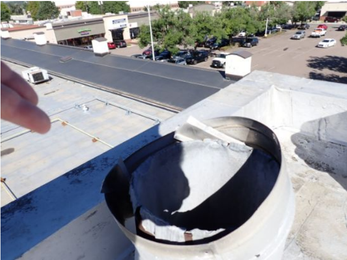
Missing boiler vent stack cover noted on the upper level of the building of time and inspection. Recommend repair by licensed contractor.
