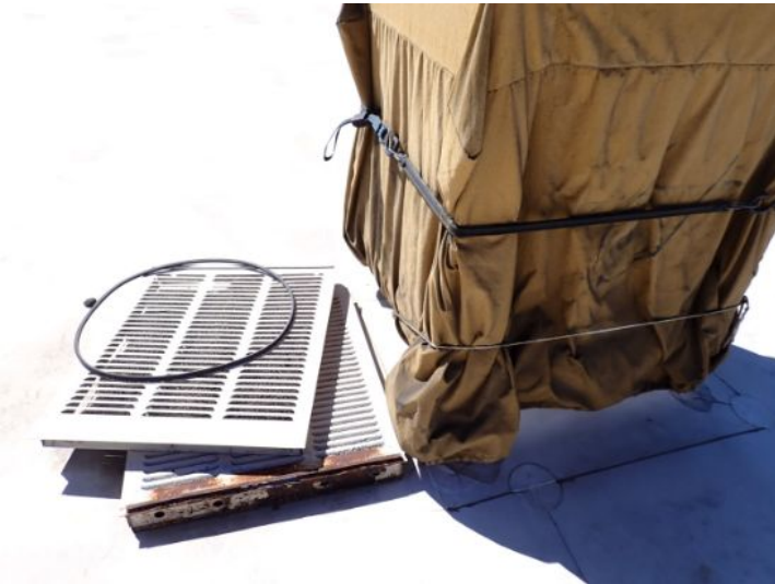
The swamp coolers located on the roofing system above the mall area were in poor condition or not functional at the time of the inspection. If the systems are still in use they require repair or replacement by licensed contractor.
