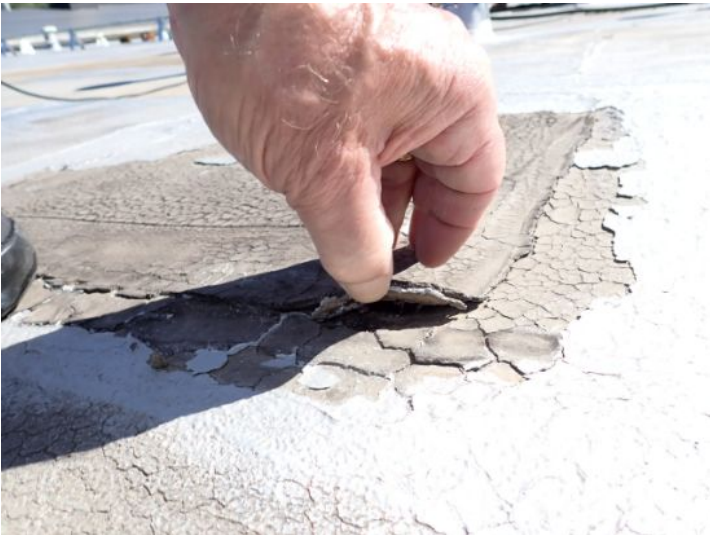
The rolled torch down roofing system located on the lower level south wing of the structure showing signs of excessive deferred maintenance, excessive ponding, possible hail damage and age. Recommend complete replacement by licensed contractor.
