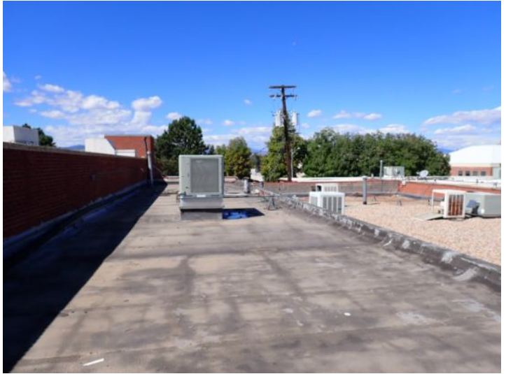
The narrow or small rolled torch down roofing system located approximately the center of the West Wing was an extremely poor condition of time inspection and requires completely recommend a licensed roofing contractor
