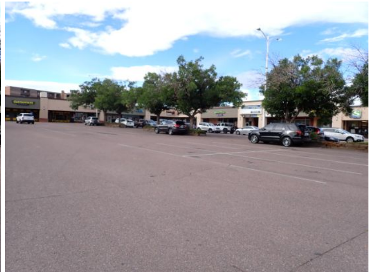
The majority of the parking lot surface was in fair condition at the time of the inspection.
