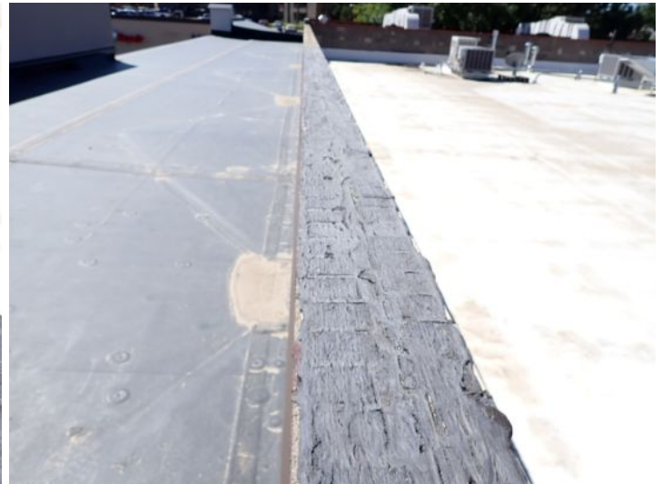
Recommend capping of all brick/block parapet walls with metal capping material. Recommend repairs by a licensed contractor.
