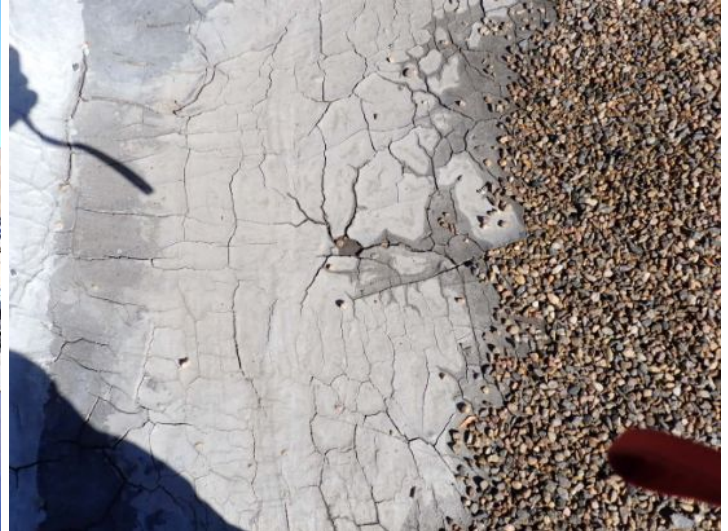
The rolled torch down roofing system above what used to be the old theater it is now currently being used as the office area appeared to be original to the structure and was showing signs of hail damage excessive ponding where and patching. Recommend replacement by licensed contractor.
