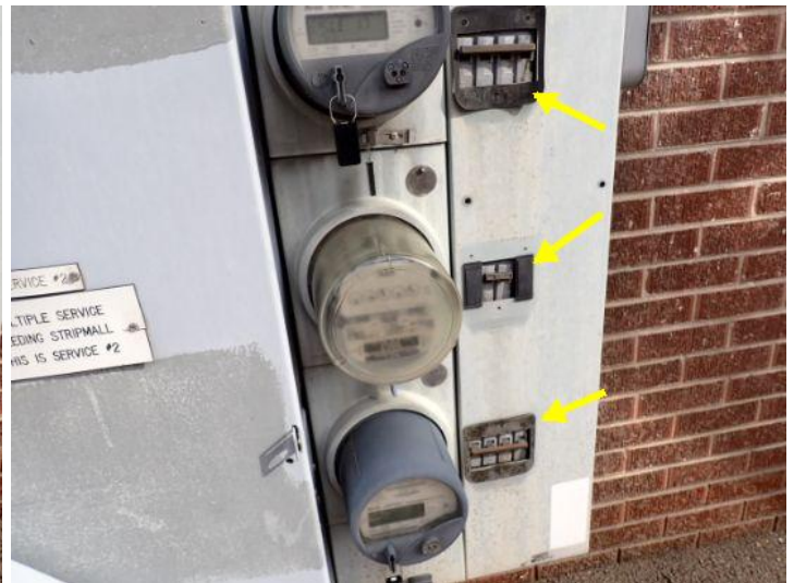
Missing weather covers noted on multiple exterior main breaker systems. Recommend repairs by a licensed contractor.
