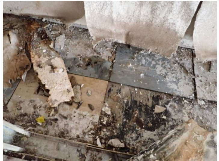
Unit 108-107: Vacant: Unit will require significant renovations prior to installing tenant. Active moisture noted in interior wall with possible microbial growth. Significant drywall damage noted in ceiling in loading dock area. Basement area in poor condition. Basement bathrooms in poor condition. Electrical not working at the time of the inspection. Moisture intrusion/damage noted in basement walls. Recommend repairs as needed by a licensed contractor.
