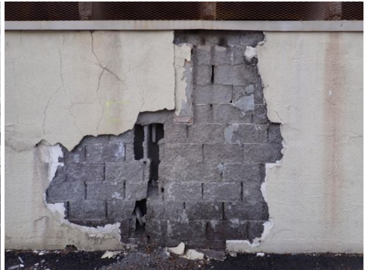
The block retaining wall for the neighboring parking garage was showing signs of significant moisture damage and deterioration in areas. Recommend monitoring to aid in possibly preventing wall failure onto your property.
