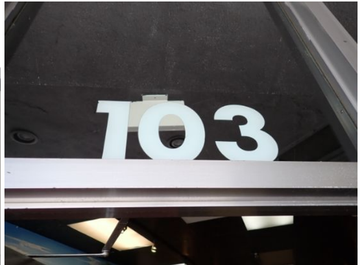
Unit 103: VCT flooring damage noted. Moisture staining noted in ceiling tiles. Moisture damage noted in rear ceiling. Active leak noted coming from roof drain. Restroom in poor condition. Recommend repairs.
