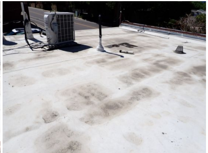
The TPO membrane located above the restaurant on the north end of the West Wing appear to be in fair condition at time of inspection.
