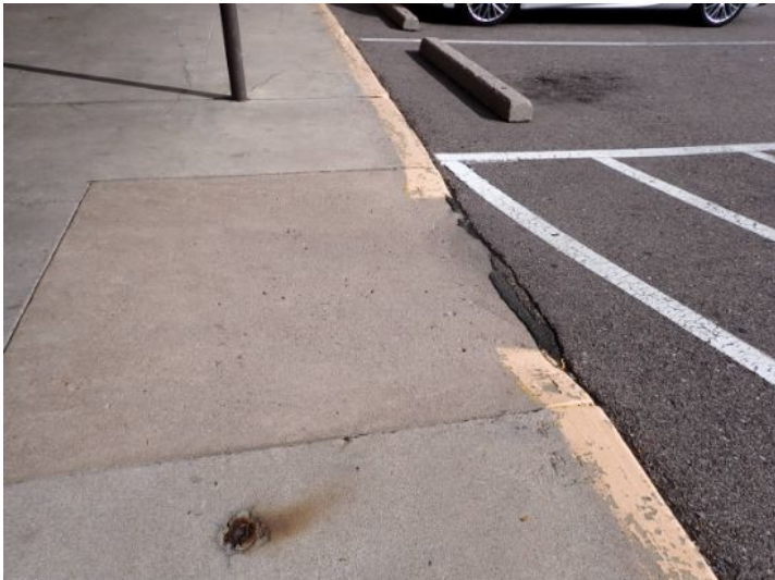
The ADA ramps were checked for proper grade and no significant issues were noted at the time of the inspection.
