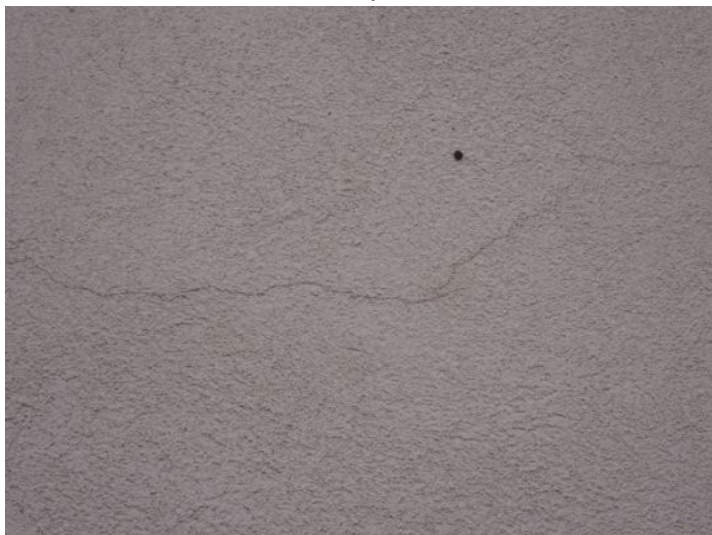
Stucco cracking noted in areas around the structure at the time of the inspection. Recommend repairs by a licensed contractor.
