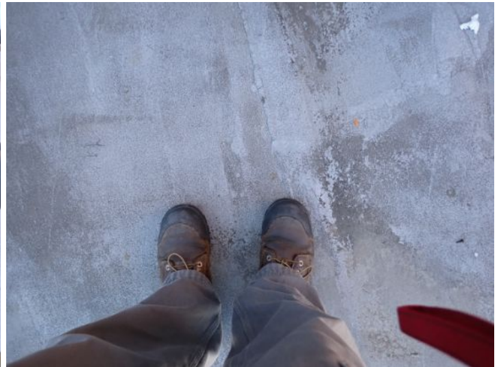
The rolled torch down roofing system located above the east end of the south wing appeared to have reached the end of its serviceable life expectancy with areas of significant ponding and cracking noted. Recommend repairs/replacement by licensed contractor.
