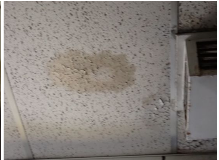
Unit 110E: Unit was vacant and will require renovations prior to placing a tenant. Recommend repairs by a licensed contractor.
