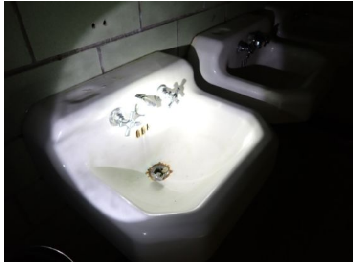
Unit 108-107: Vacant: Unit will require significant renovations prior to installing tenant. Active moisture noted in interior wall with possible microbial growth. Significant drywall damage noted in ceiling and walls in loading dock area. Basement area in poor condition. Basement bathrooms in poor condition. Electrical not working at the time of the inspection. Moisture intrusion/damage noted in basement walls. Recommend repairs as needed by a licensed contractor.
