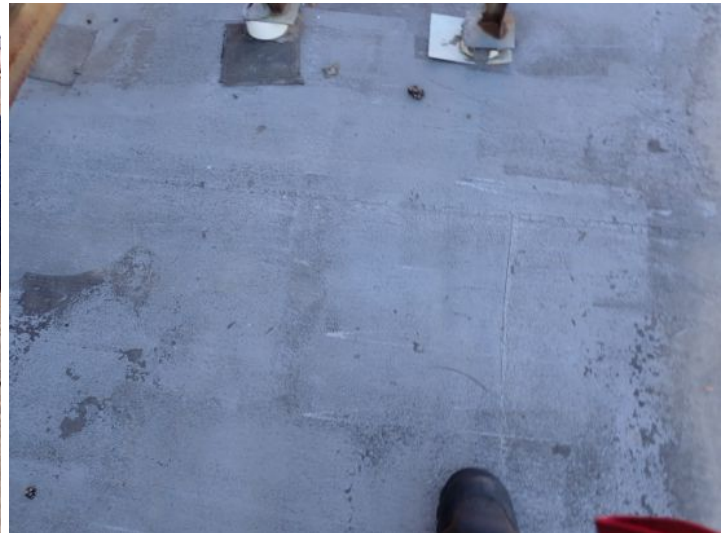
The rolled torch down roofing system located above the east end of the south wing appeared to have reached the end of its serviceable life expectancy with areas of significant ponding and cracking noted. Recommend repairs/replacement by licensed contractor.
