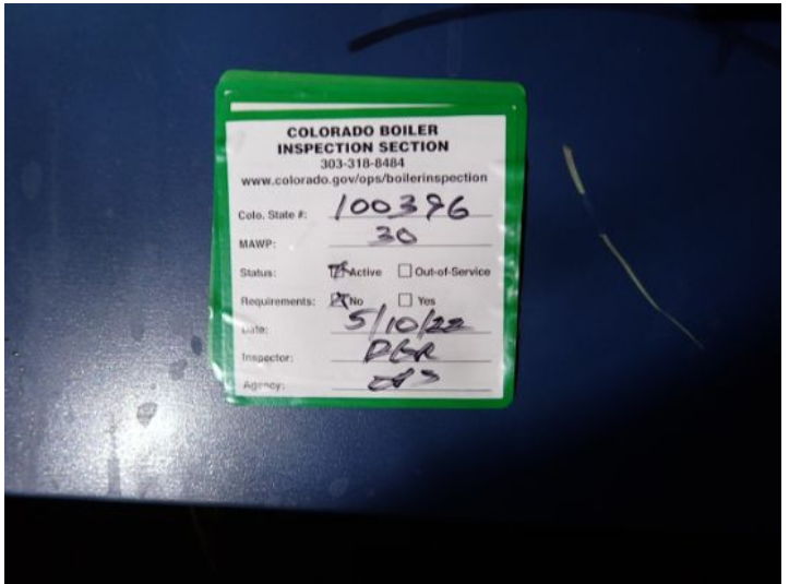
Office Building Boiler: Dunkirk: M/N WPSB-9D-HA5 S/N 331300183. Manufacture year 2013. Colorado Boiler #100396. Last date of state inspection/certification was 5/22.
