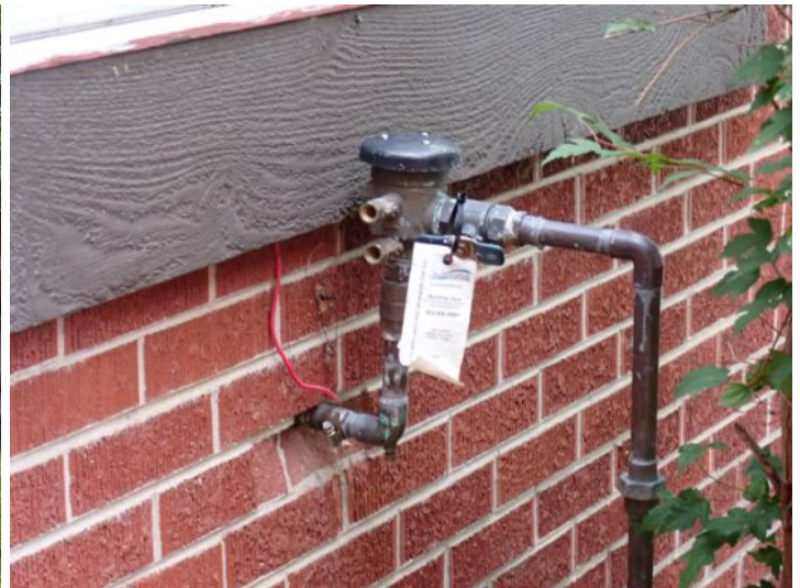
The backflow preventer for the irrigation system appeared to be installed on the roof top above the laundry mat for the east end and in the planting bed behind the paint store for the west end. The backflow preventers appeared functional at the time of the inspection.
