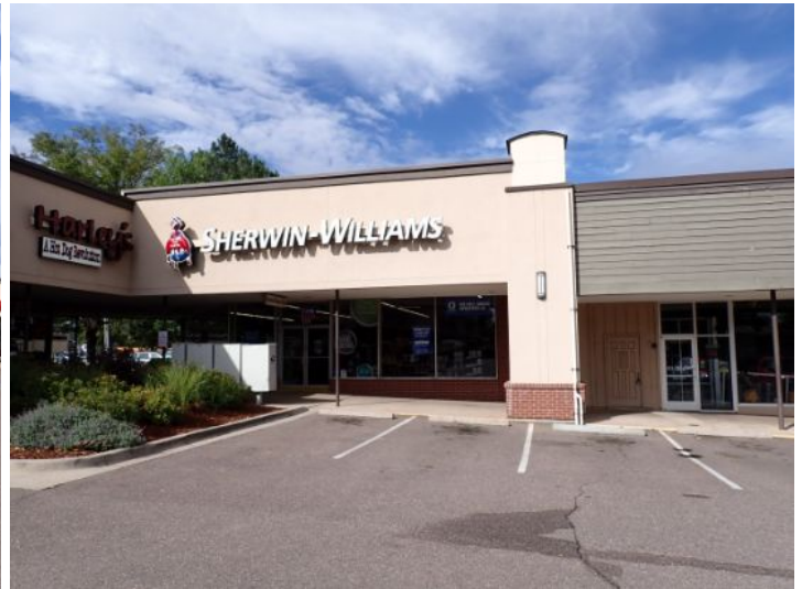
The majority of the exterior envelope of the structure appeared to be in fair condition with no significant structural movement noted at the time of the inspection.
