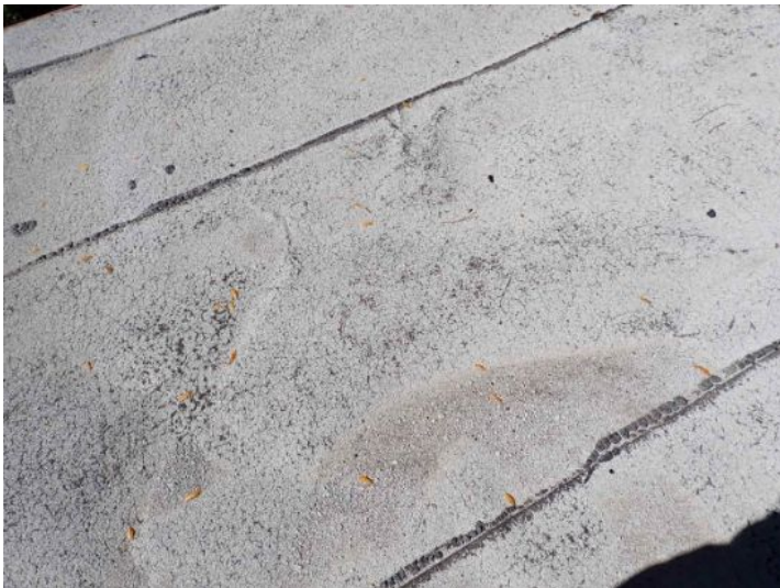
The rolled asphalt composition roof and system located above the awning between the two wings was in extremely poor condition why is it a plate replacement. Recommend repair by a licensed contractor.
