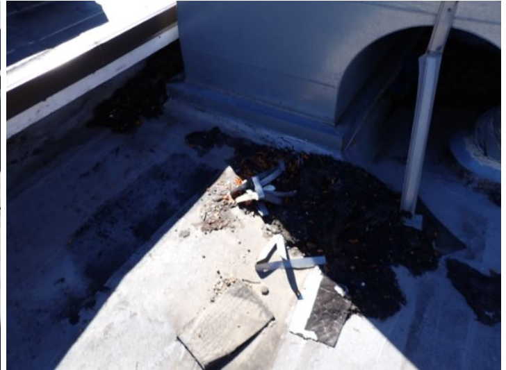
The rolled torch down roofing system located above the east end of the south wing appear did reach the end of its serviceable life expectancy with areas of significant ponding and cracking noted. Recommend repairs/replacement by licensed contractor.
