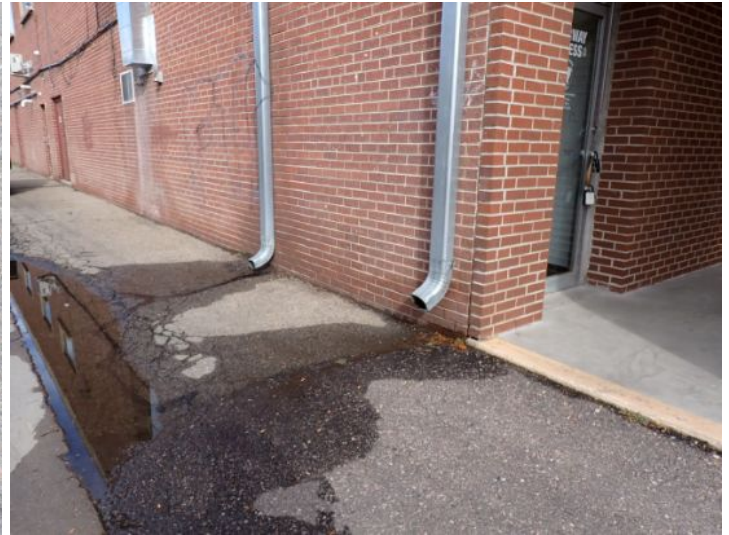
Gutters down spouts missing extensions to direct storm water away from the foundation of the structure. Recommend repairs.
