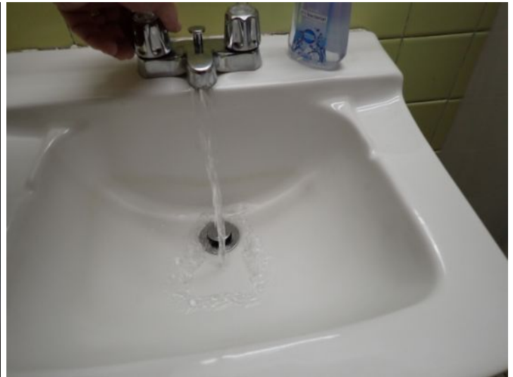
The common area restrooms in the office building and mall areas were tested and functional at the time of the inspection.
