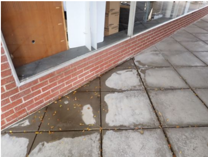
Grade falling toward structure in areas. Recommend repairs by a licensed contractor.
