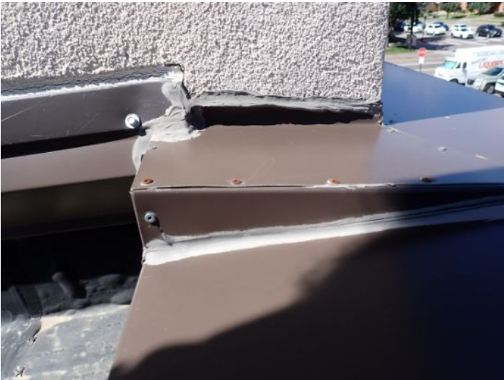
Due to flashing issues storm water was getting into one of the stucco awning support pillars and running down the inside of the system. Recommend repairs as needed by a licensed contractor.
