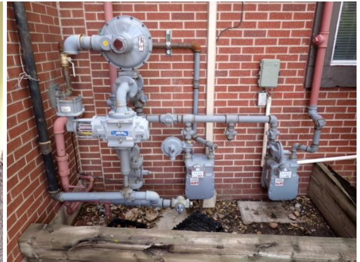
The main gas shutoff valve(s) was/were functional at the time of the inspection
