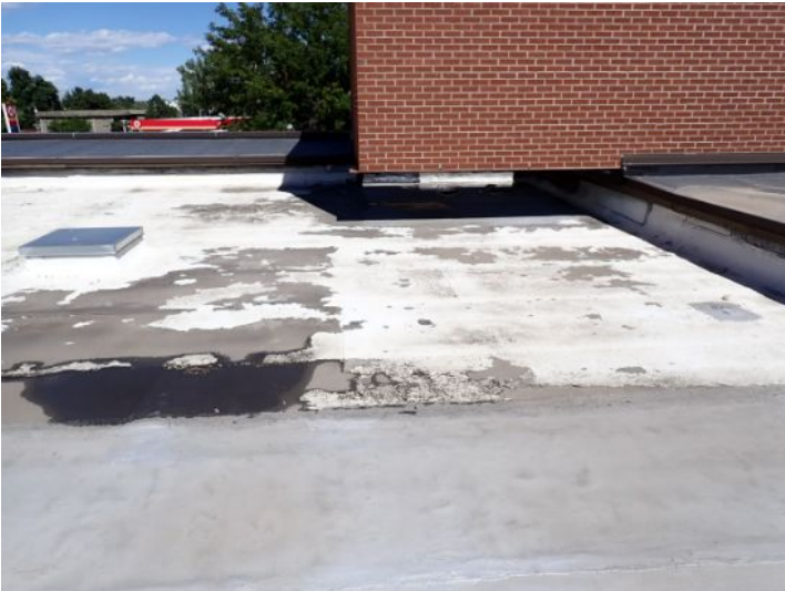
The rolled torch down roofing membrane located above the fitness center on the north end of the west wing was an extremely poor condition and has reached the end of the service for life expectancy. Recommend complete replacement by licensed roofing contractor.
