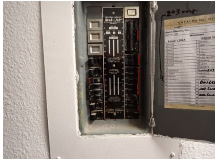
Old Federal Pacific Stab Lock breaker systems noted in some of the units at the time of the inspection. These systems have been proven to be safety/fire issues. Recommend replacement of all FPE panels and stab lock breaker systems by a licensed contractor prior to taking possession of the property.
