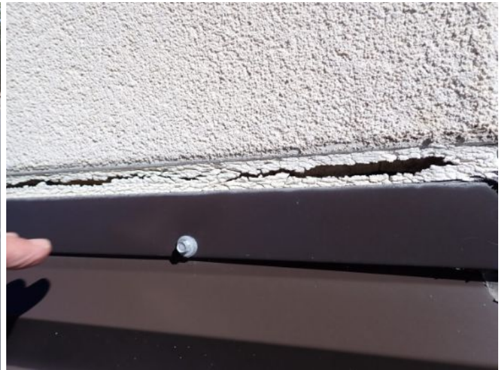
Caulking of the flashing in areas of the EPDM membrane is required in areas. Recommend repairs by licensed contractor.
