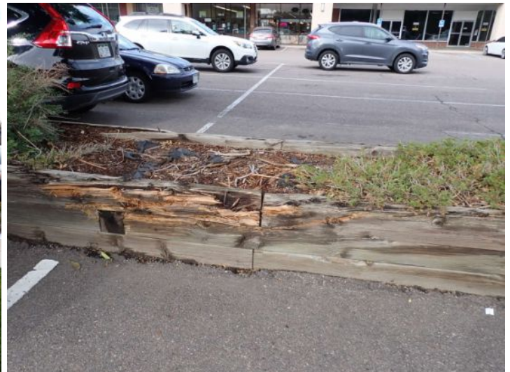
The timber retaining walls located around the planning beds in the parking lot were in poor condition at the time of the inspection. Recommend repairs by a licensed contractor.
