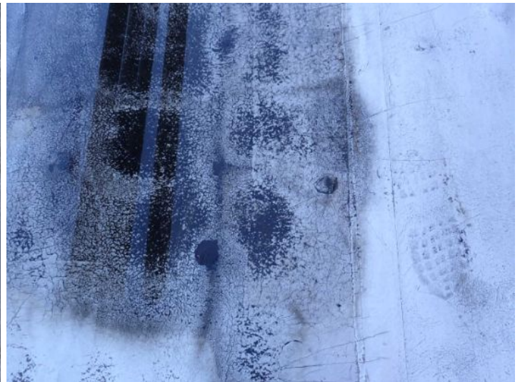
The rolled torch down roofing system located above the east end of the south wing appeared to have reached the end of its serviceable life expectancy with areas of significant ponding and cracking noted. Recommend repairs/replacement by licensed contractor.
