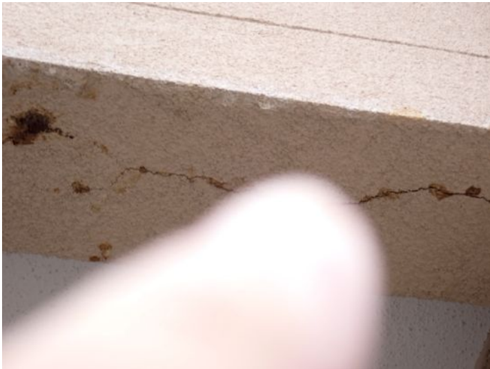
Due to flashing issues storm water was getting into one of the stucco awning support pillars and running down the inside of the system. Recommend repairs as needed by a licensed contractor.
