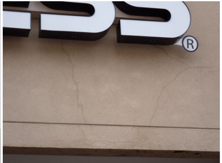
Stucco cracking noted in areas around the structure at the time of the inspection. Recommend repairs by a licensed contractor.
