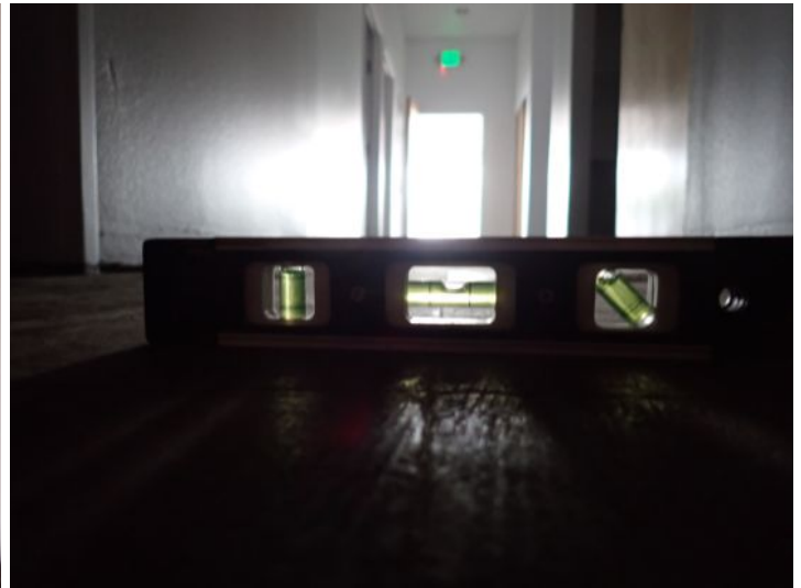
Unit 110C&D: Unit was vacant. Floor settling/deflection noted. Recommend repairs as needed by a licensed contractor.
