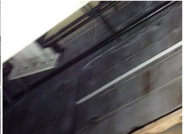
Unit 110G: Acoustical tile ceiling damage noted. Missing knockouts noted in electrical panel. Recommend repairs.
