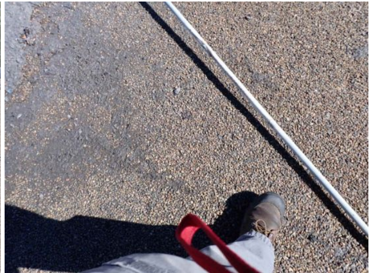
The BUR roofing system located on the east end of the south wing of the building is showing signs of excessive wear excessive ponding it was an extremely poor condition at the time of the inspection. Recommend replacement by a licensed contractor.
