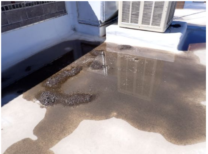
TPO roofing membrane located above the mall area of the property while appearing to be in fair condition was showing signs of excessive deferred maintenance and ponding at the time of the inspection. Recommend repairs by licensed contractor.
