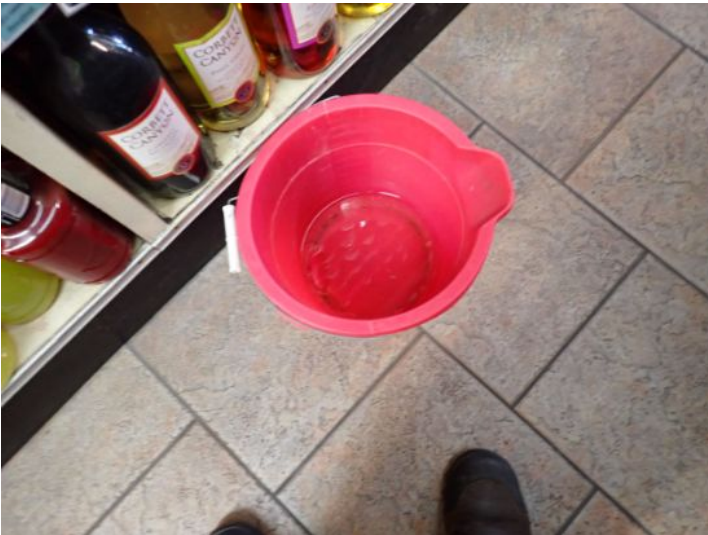
Unit 101: Active leak noted coming from roof drain. Restroom in poor condition. Recommend repairs.
