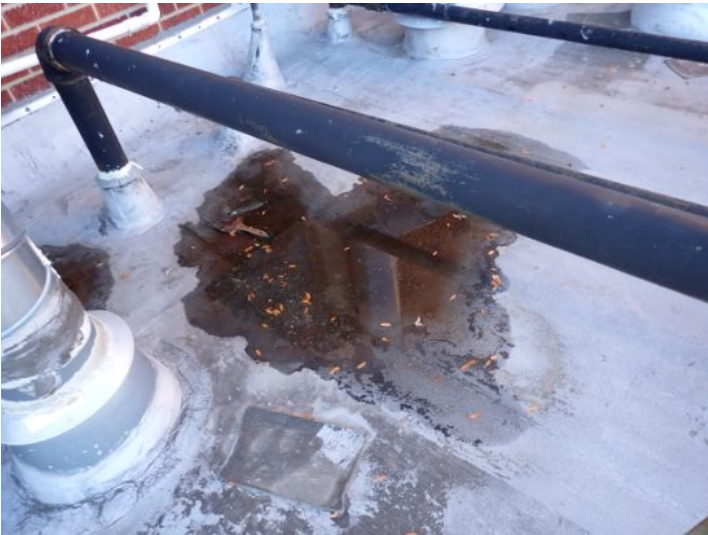
The rolled torch down roofing system located above the east end of the south wing appear did reach the end of its serviceable life expectancy with areas of significant ponding and cracking noted. Recommend repairs/replacement by licensed contractor.
