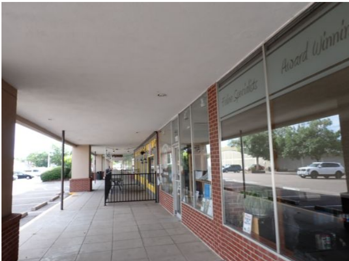
The majority of the exterior envelope of the structure appeared to be in fair condition with no significant structural movement noted at the time of the inspection.
