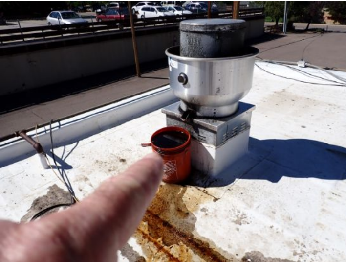
One or more kitchen roof top vent systems were showing signs of significant deferred maintenance. Recommend repairs by a licensed contractor.
