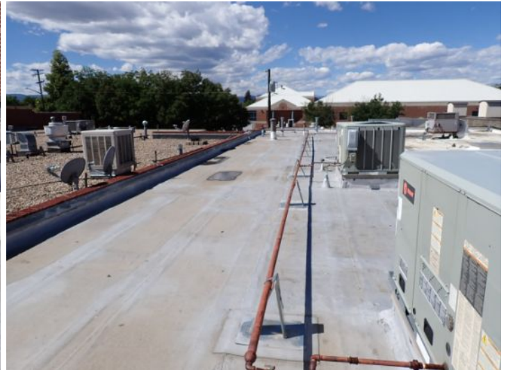
The rolled torch down roofing membrane located above the fitness center on the north end of the west wing was an extremely poor condition and has reached the end of the service for life expectancy. Recommend complete replacement by licensed roofing contractor.
