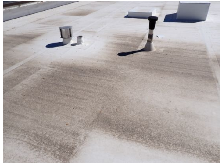
The TPO membrane located above the lower level west end of the south unit appeared to be in fair condition at time of inspection.
