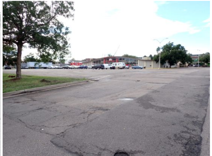
Deteriorated paving material noted in areas. Recommend repairs by a licensed contractor.
