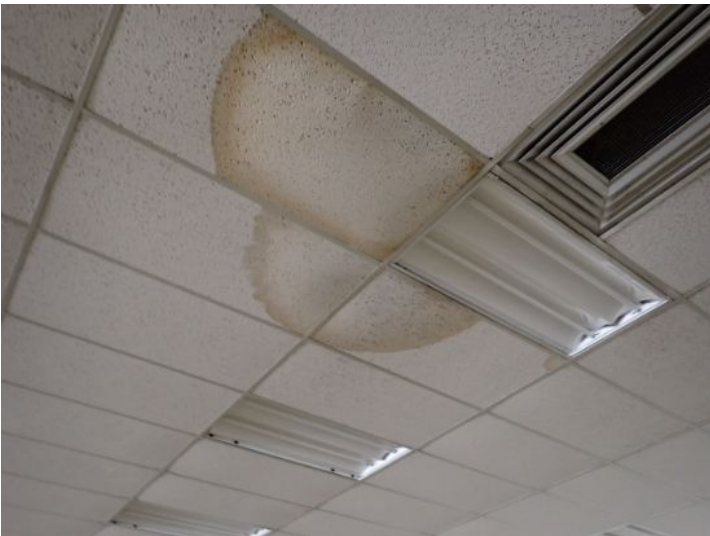
Unit 108-107: Vacant: Unit will require significant renovations prior to installing tenant. Active moisture noted in interior wall with possible microbial growth. Significant drywall damage noted in ceiling in loading dock area. Basement area in poor condition. Basement bathrooms in poor condition. Electrical not working at the time of the inspection. Moisture intrusion/damage noted in basement walls. Recommend repairs as needed by a licensed contractor.
