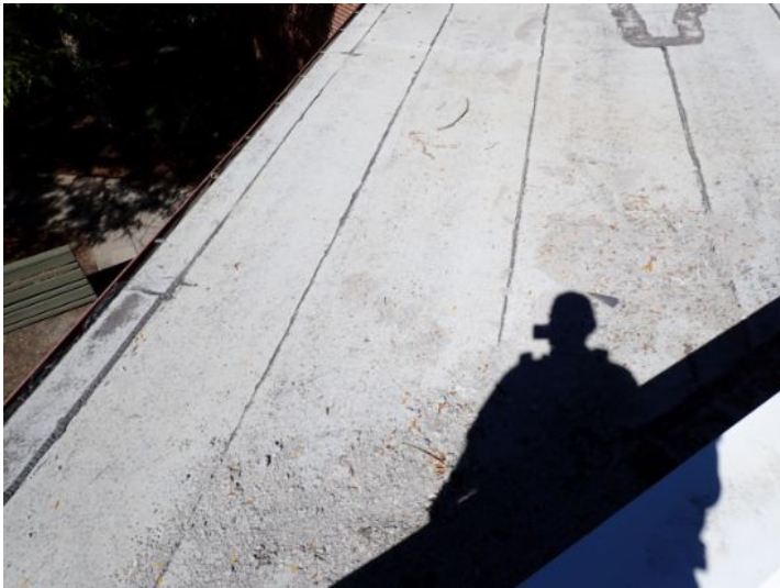
The rolled asphalt composition roof and system located above the awning between the two wings was in extremely poor condition why is it a plate replacement. Recommend repair by a licensed contractor.
