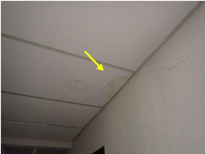
Moisture staining noted in areas of the acoustical tile ceilings throughout the building at the time of the inspection. Recommend repairs and monitoring
