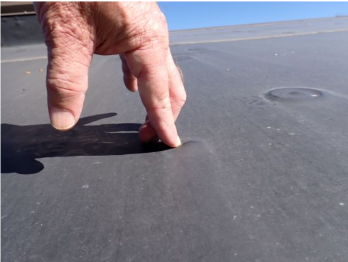
The EPDM membrane on the low slope front sections of each wing appeared be in fair condition at time of inspection. There were areas where it appeared that debris below the membrane was attempting to push through the membrane but had not penetrated at the time of the inspection. Recommend monitoring for future repairs.
