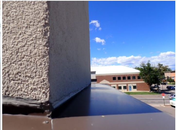
Due to flashing issues storm water was getting into one of the stucco awning support pillars and running down the inside of the system. Recommend repairs as needed by a licensed contractor.
