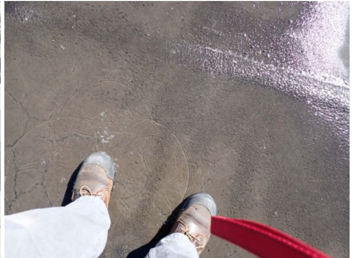
The rolled torch down roofing system above what used to be the old theater it is now currently being used as the office area appeared to be original to the structure and was showing signs of hail damage excessive ponding where and patching. Recommend replacement by licensed contractor.
