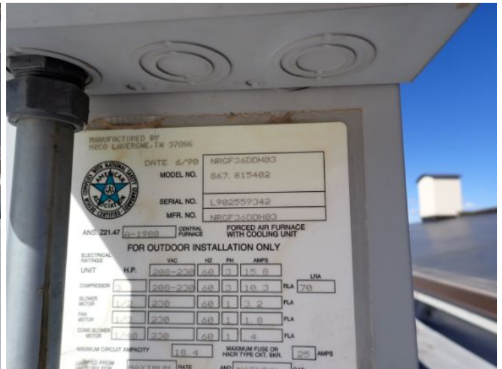
RTU 10: HRCO: M/N NRGF36DDH03 S/N L902559342. Manufacture year 1990.
