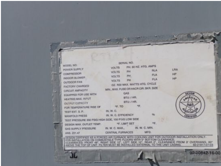
RTU 26: RUUD: M/N ? S/N ? Manufacture year ?
