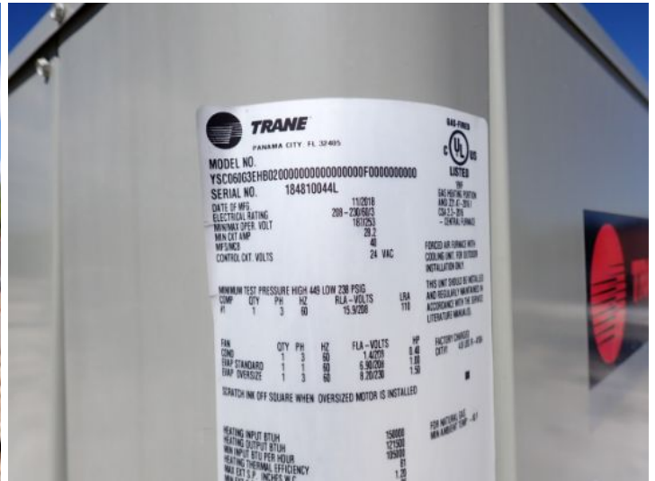
RTU 23: Trane: M/N YSC060G3EHB0200000 S/N 184810044L. Manufacture year 2018.
