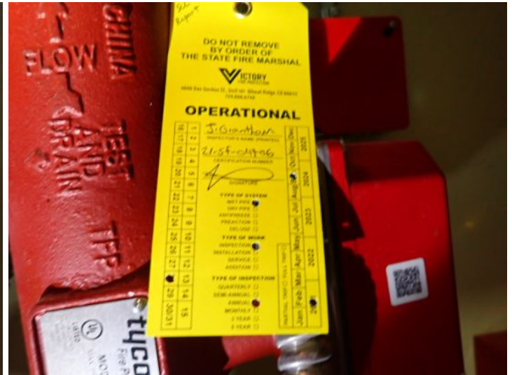
Last date of inspection/certification of the fire suppression system was 9/21.
