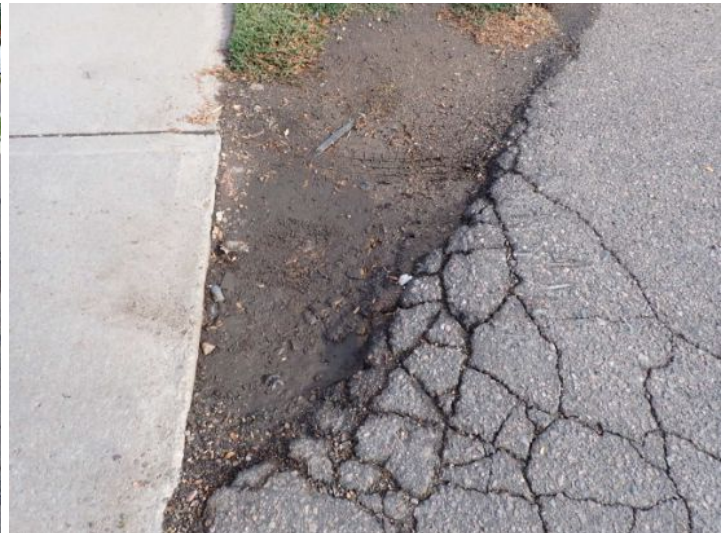
Deteriorated paving material noted in areas. Recommend repairs by a licensed contractor.
