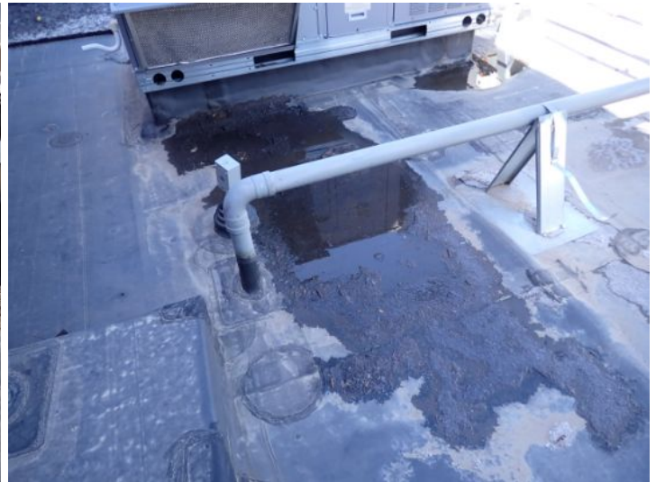
The EPDM roofing membrane located on the lower level of the south wing appeared to be in fair condition at the time of the inspection but was showing signs of excessive ponding and minor seam issues in areas. Recommend repairs as required by a licensed contractor.
