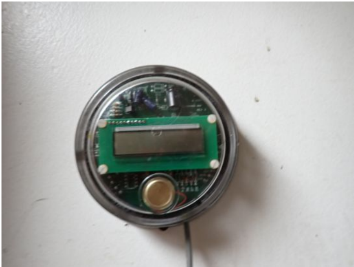
Some of the tenant units appeared to have sub meters located within them but the meters did not appear to be functional at the time of the inspection. Recommend consulting with the current owners/management company to determine what is going on with these systems as well as where the main shutoffs are all located and how water metering is performed.
