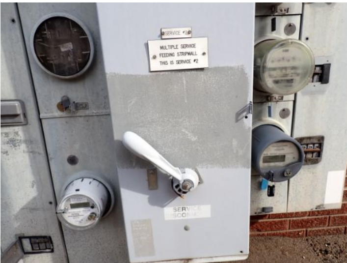
The main electrical disconnects appeared functional at the time of the inspection.
