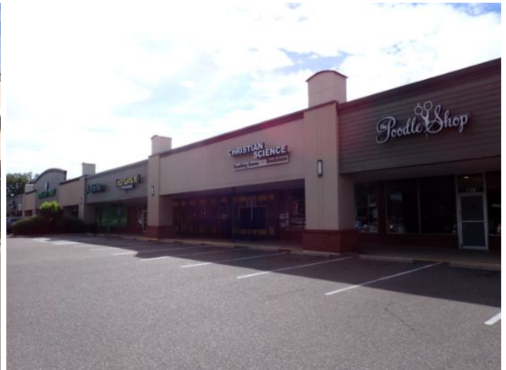
The majority of the exterior envelope of the structure appeared to be in fair condition with no significant structural movement noted at the time of the inspection.
