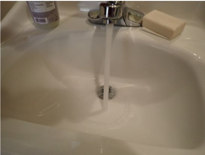
The common area restrooms in the office building and mall areas were tested and functional at the time of the inspection.
