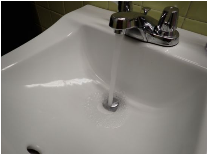
The common area restrooms in the office building and mall areas were tested and functional at the time of the inspection.
