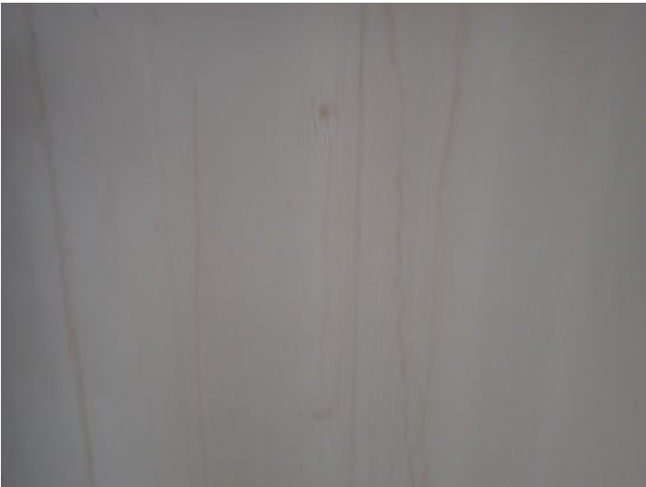
Unit 108-107: Vacant: Unit will require significant renovations prior to installing tenant. Active moisture noted in interior wall with possible microbial growth. Significant drywall damage noted in ceiling in loading dock area. Basement area in poor condition. Basement bathrooms in poor condition. Electrical not working at the time of the inspection. Moisture intrusion/damage noted in basement walls. Recommend repairs as needed by a licensed contractor.
