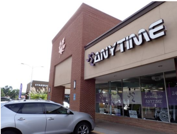
The majority of the exterior envelope of the structure appeared to be in fair condition with no significant structural movement noted at the time of the inspection.
