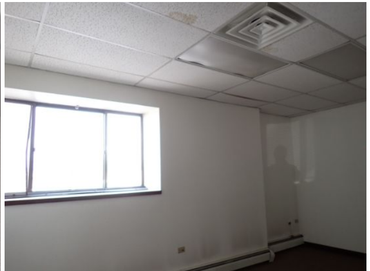
The majority of the interior offices, that were accessible at the time of the inspection, appeared to be in fair condition at the time of the inspection.
