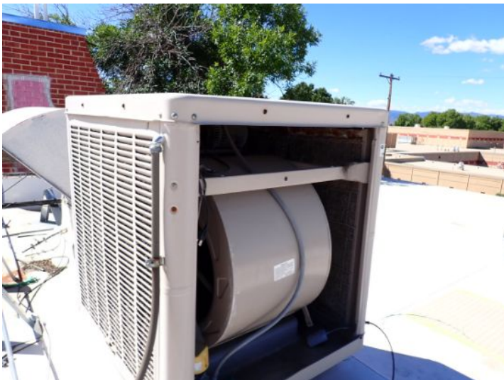
The swamp coolers located on the roofing system above the mall area were in poor condition or not functional at the time of the inspection. If the systems are still in use they require repair or replacement by licensed contractor.
