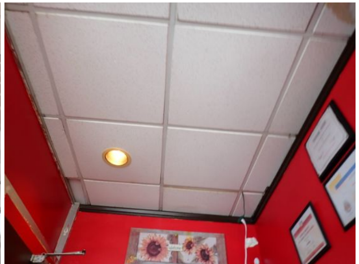
Unit 100A: No significant issues noted at the time of the inspection.
