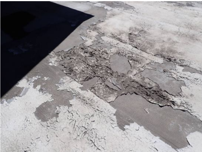
The rolled torch down roofing membrane located above the fitness center on the north end of the west wing was an extremely poor condition and has reached the end of the service for life expectancy. Recommend complete replacement by licensed roofing contractor.
