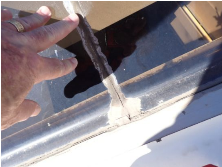
Cracked/leaking skylight system noted above the mall area. Recommend replacement by a licensed contractor.
