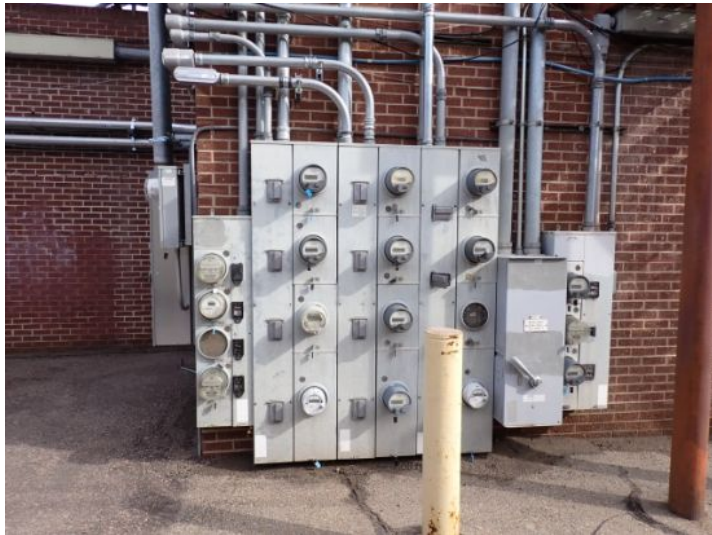
The main electrical disconnects appeared functional at the time of the inspection.
