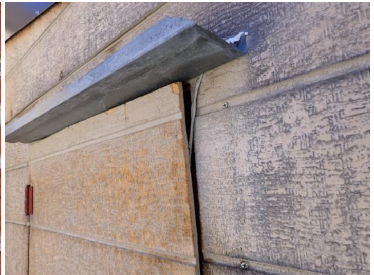
The wood siding material located above the corner awning roof on the ends of the pitched roof sections were in poor condition at the time of the inspection. Recommend repairs by a licensed contractor.
