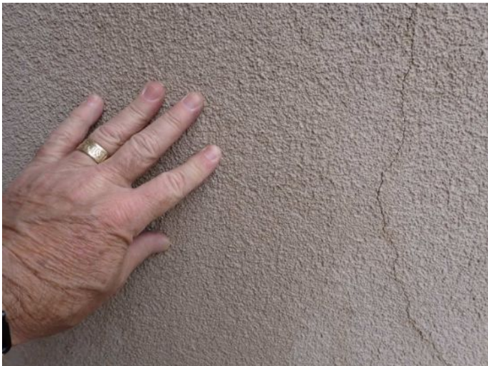
Due to flashing issues storm water was getting into one of the stucco awning support pillars and running down the inside of the system. Recommend repairs as needed by a licensed contractor.
