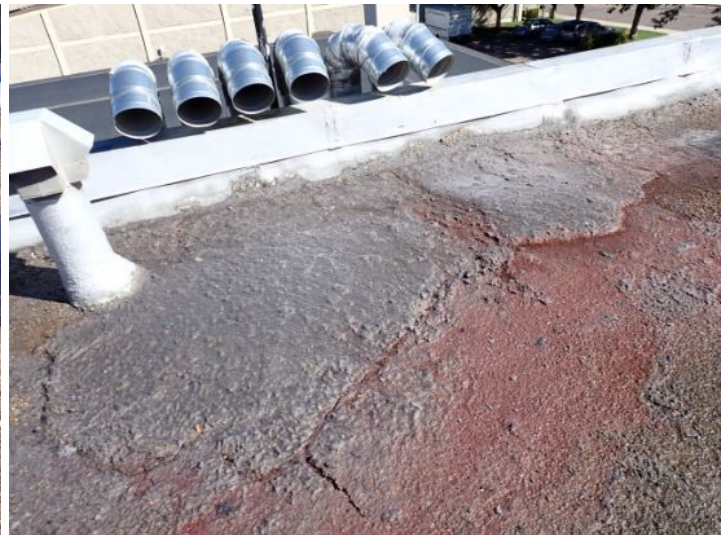
Excessive lint buildup noted on the roof tops above the laundry at the time of the inspection. This could be considered a fire hazard. Recommend cleaning by licensed contractor.
