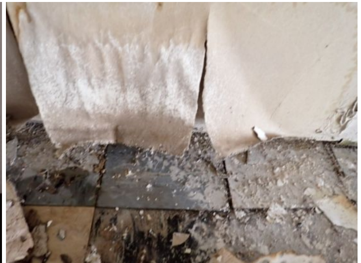
Active roof leaks noted in multiple units at the time of the inspection. Recommend repair/replacement as needed by a licensed contractor.
