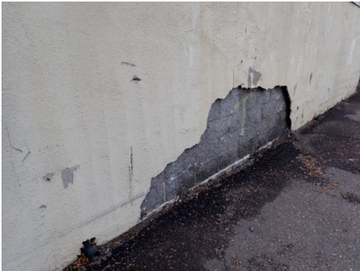
The block retaining wall for the neighboring parking garage was showing signs of significant moisture damage and deterioration in areas. Recommend monitoring to aid in possibly preventing wall failure onto your property.
