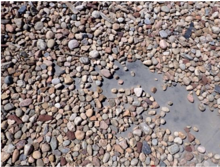
The gravel coated EPDM roofing membrane located towards the north end of the west structure was showing signs of significant ponding and deferred maintenance at the time of the inspection. Recommend repair by licensed contractor.
