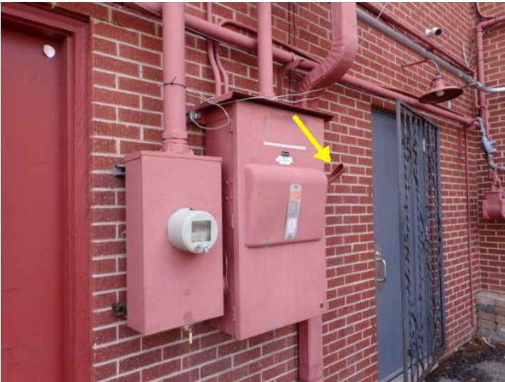
The main electrical disconnects appeared functional at the time of the inspection.
