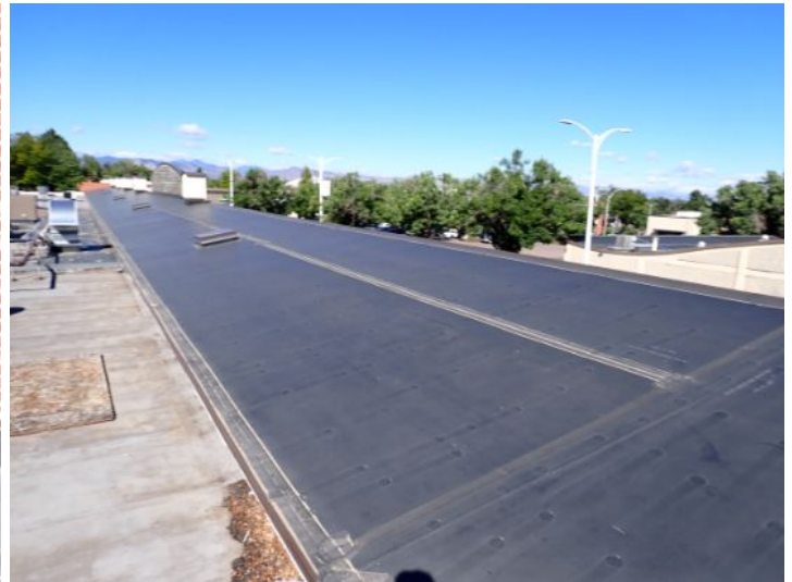
The EPDM membrane on the low slope front sections of each wing appeared be in fair condition at time of inspection. There were areas where it appeared that debris below the membrane was attempting to push through the membrane but had not penetrated at the time of the inspection. Recommend monitoring for future repairs.
