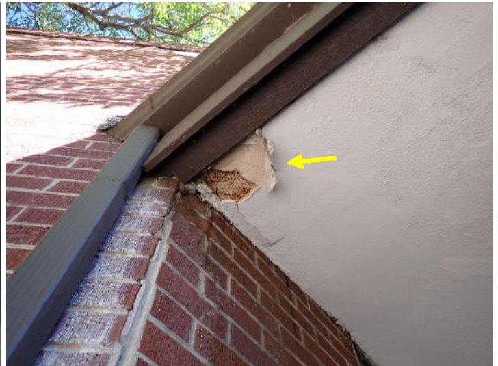
Moisture damage noted in awning ceiling. Recommend repairs by a licensed contractor.
