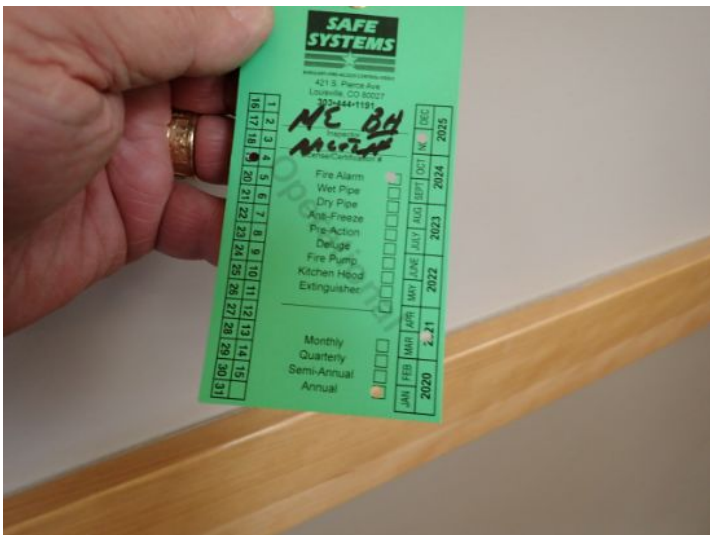
Last date of inspection/certification of the fire alarm system was 11/21.
