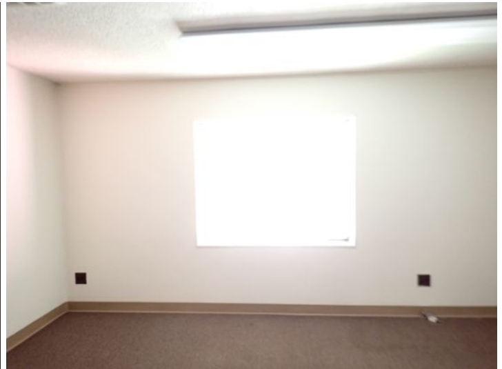
Unit 111B: Emergency egress goes through unit 111 which is locked at night. Recommend repairs by a licensed contractor prior to installing a new tenant.
