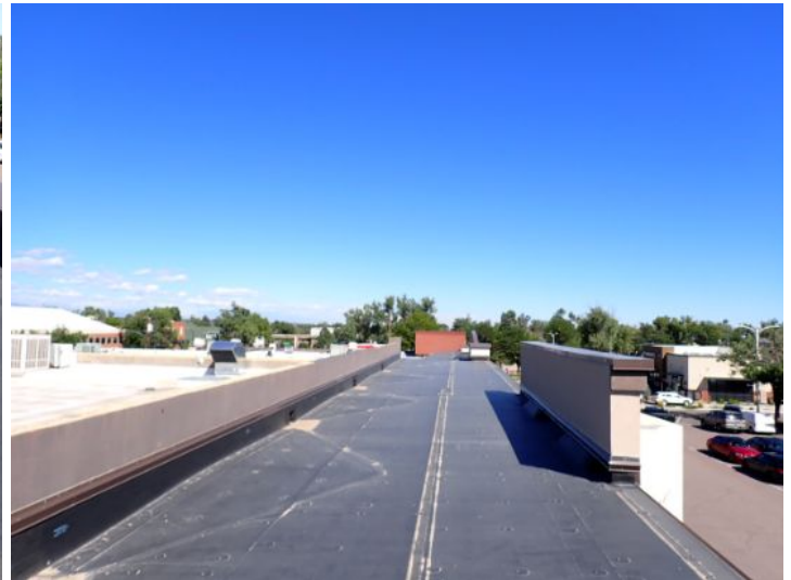
The EPDM membrane on the low slope front sections of each wing appeared to be in fair condition at time of inspection. There were areas where it appeared that debris below the membrane was attempting to push through the membrane but had not penetrated at the time of the inspection. Recommend monitoring for future repairs.
