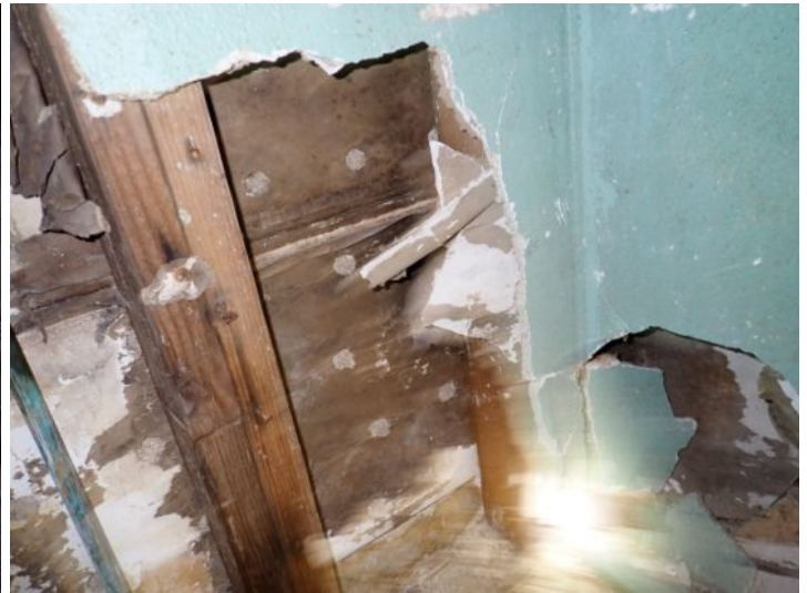
Unit 108-107: Vacant: Unit will require significant renovations prior to installing tenant. Active moisture noted in interior wall with possible microbial growth. Significant drywall damage noted in ceiling and walls in loading dock area. Basement area in poor condition. Basement bathrooms in poor condition. Electrical not working at the time of the inspection. Moisture intrusion/damage noted in basement walls. Recommend repairs as needed by a licensed contractor.
