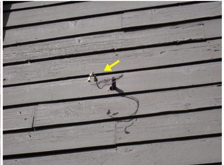
Exposed electrical wiring noted in areas around the exterior and on the roof of the structure at the time of the inspection. Recommend proper repairs by a licensed electrician.
