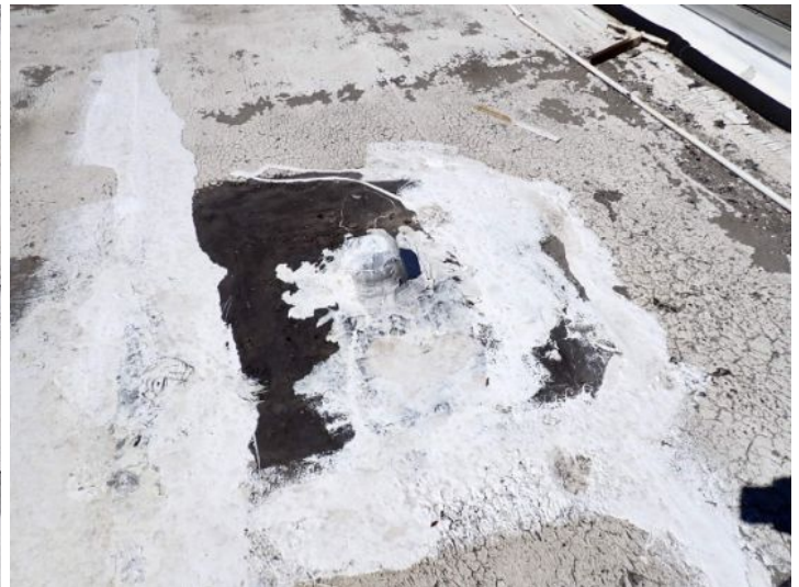
The rolled torch down roofing membrane located above the fitness center on the north end of the west wing was an extremely poor condition and has reached the end of the service for life expectancy. Recommend complete replacement by licensed roofing contractor.
