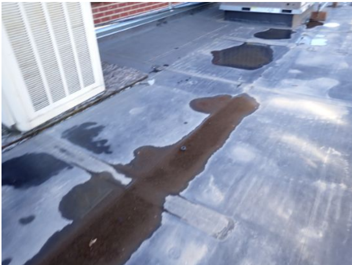
The EPDM roofing membrane located on the lower level of the south wing appeared to be in fair condition at the time of the inspection but was showing signs of excessive ponding and minor seam issues in areas. Recommend repairs as required by a licensed contractor.
