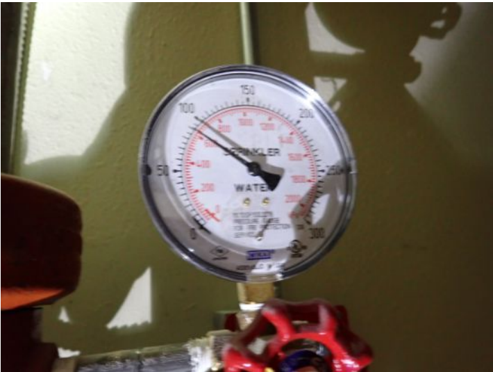
The fire suppression system was holding approximately 90 psi at the time of the inspection.
