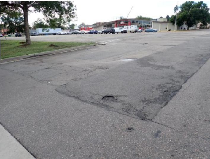
Deteriorated paving material noted in areas. Recommend repairs by a licensed contractor.
