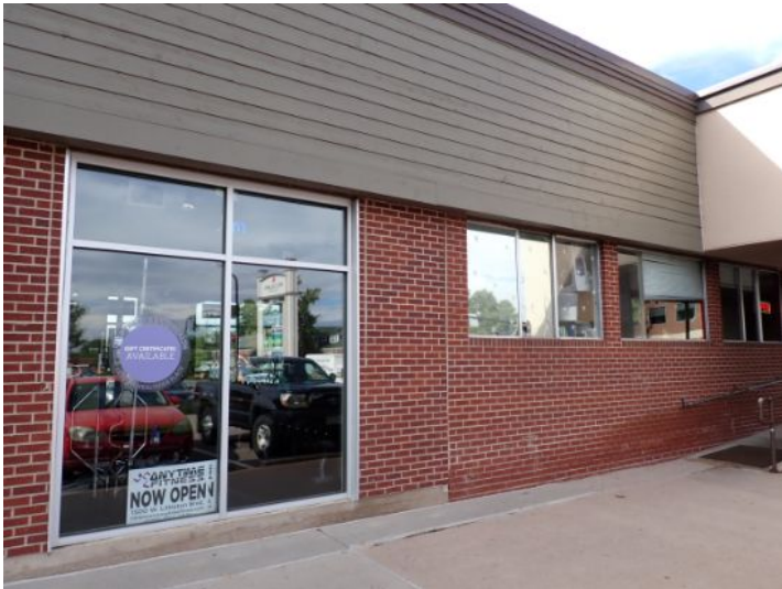
The majority of the exterior envelope of the structure appeared to be in fair condition with no significant structural movement noted at the time of the inspection.
