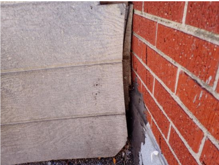
The wood siding material located above the corner awning roof on the ends of the pitched roof sections were in poor condition at the time of the inspection. Recommend repairs by a licensed contractor.
