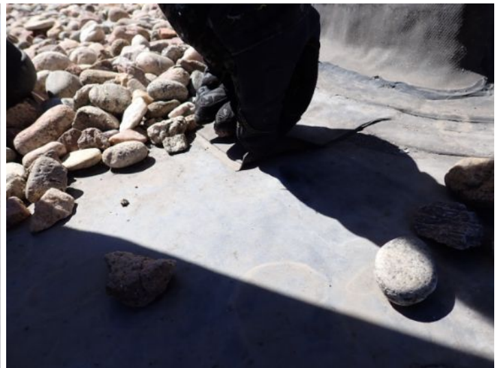
The gravel coated EPDM roofing membrane located near the north end of the west direction is showing signs of poor drainage and seem issues at the time of the inspection and appeared to have reached the end of its serviceable life expectancy. Recommend replacement by licensed roofing contractor.
