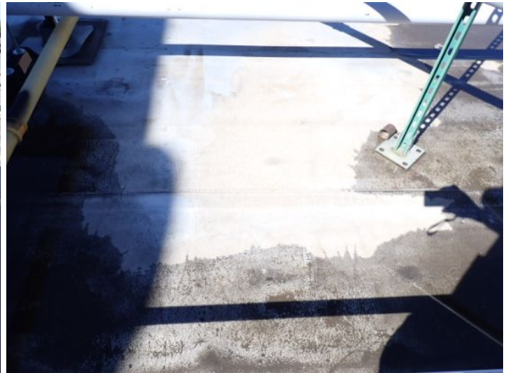
The rolled torch down roofing system located on the lower level south wing of the structure showing signs of excessive deferred maintenance, excessive ponding, possible hail damage and age. Recommend complete replacement by licensed contractor.
