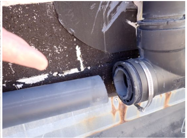
There was what appeared to be a 4 inch wet Vent piping located on the narrow roof above the center of the west wing that was not strapped properly and it becomes separated overtime. This could cause odor issues inside the building. Recommend repairs by licensed contractor.
