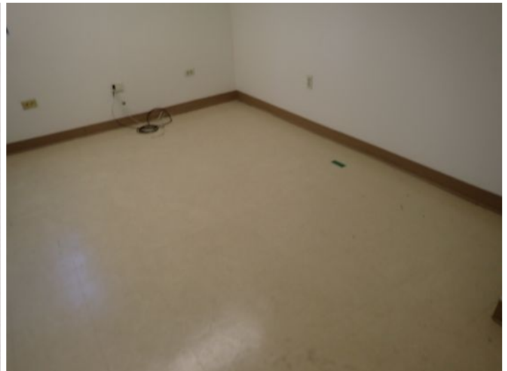
Unit 111B: Emergency egress goes through unit 111 which is locked at night. Recommend repairs by a licensed contractor prior to installing a new tenant.
