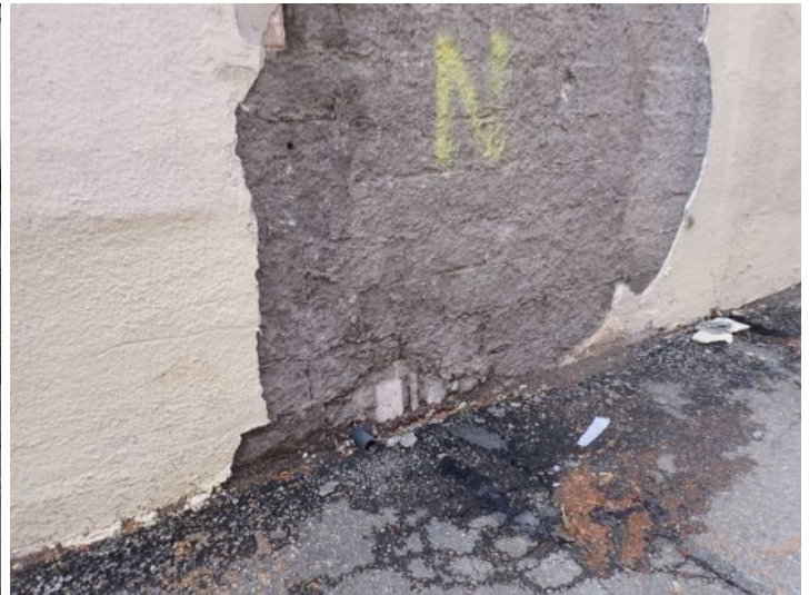
The block retaining wall for the neighboring parking garage was showing signs of significant moisture damage and deterioration in areas. Recommend monitoring to aid in possibly preventing wall failure onto your property.
