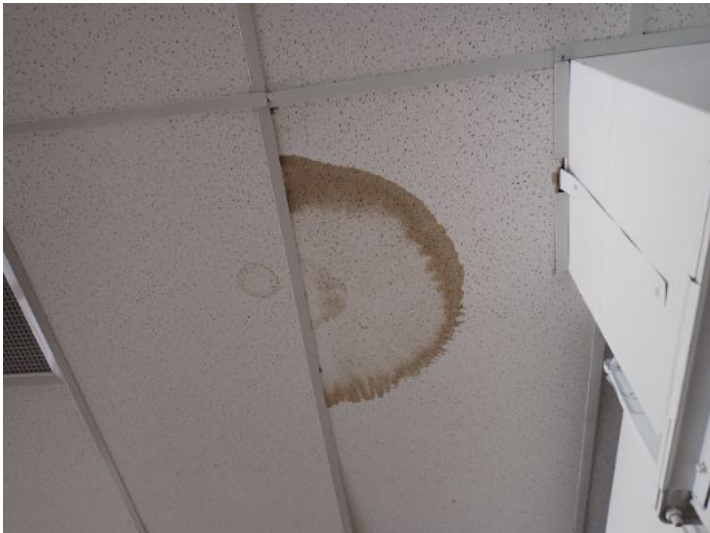
Unit 122: Moisture damage noted in ceiling tiles. Recommend repairs and monitoring.
