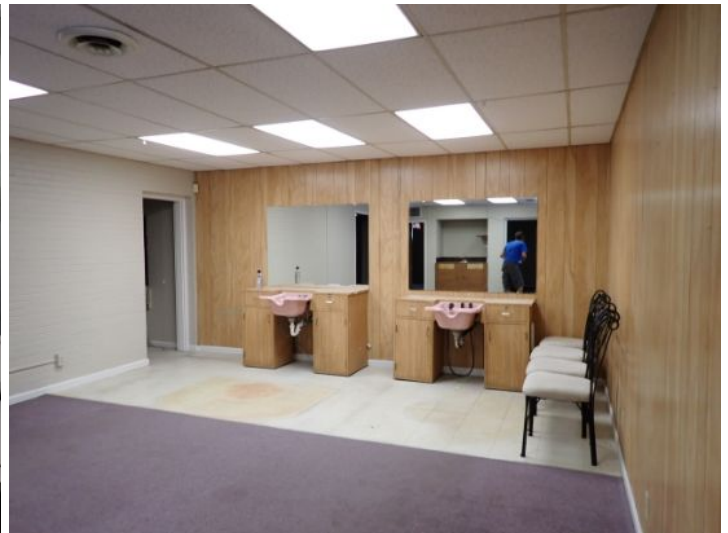
Unit 132: Unit was in poor condition and will require complete renovations prior to installing a new tenant.
