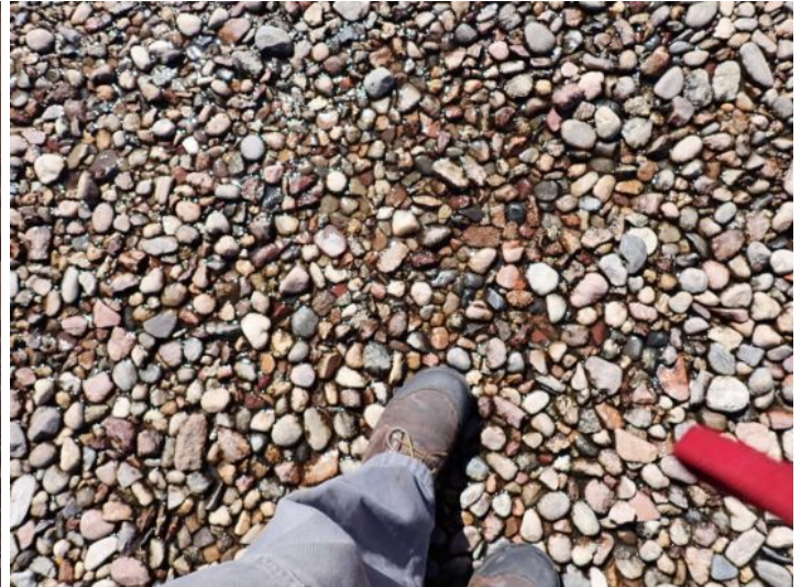
The gravel coated EPDM roofing membrane located near the north end of the west direction is showing signs of poor drainage and seem issues at the time of the inspection and appeared to have reached the end of its serviceable life expectancy. Recommend replacement by licensed roofing contractor.
