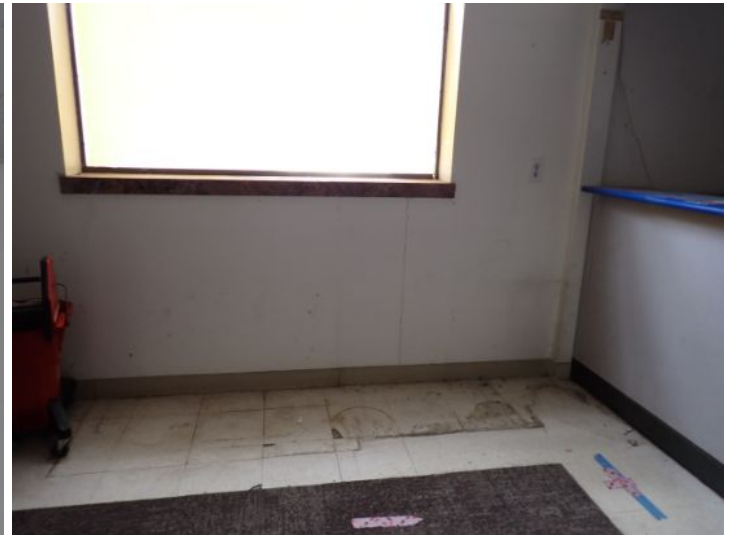
Unit 110E: Unit was vacant and will require renovations prior to placing a tenant. Recommend repairs by a licensed contractor.
