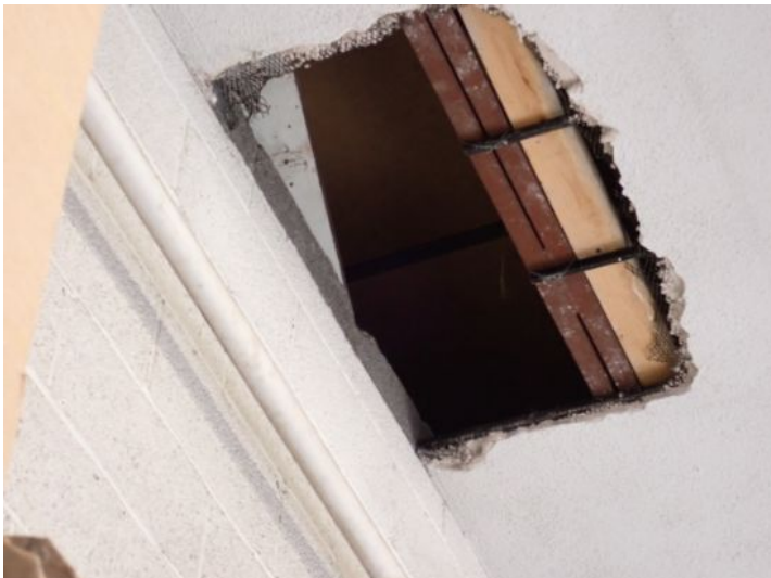
Unit 111-112: Moisture staining noted in ceiling tiles. Moisture damage noted in warehouse ceiling. Water heater not functional. Drywall ceiling damage noted. Recommend repairs.
