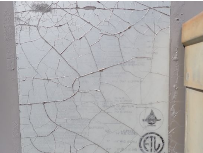
RTU 16: Goodman: M/N ? S/N ? Manufacture year ?
