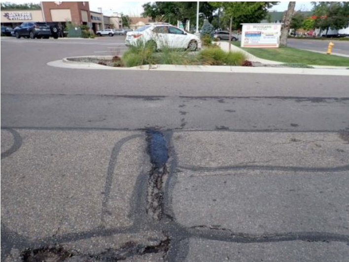
Deteriorated paving material noted in areas. Recommend repairs by a licensed contractor.
