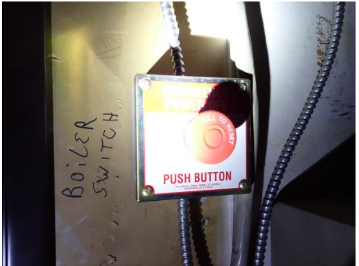
Emergency shutoff switch for the active boiler system was in place and appeared functional at the time of the inspection.
