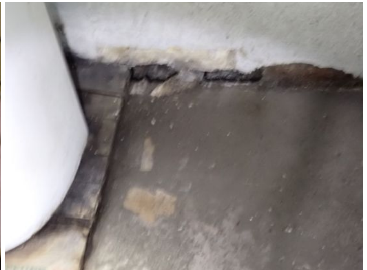
Unit 101: Active leak noted coming from roof drain. Restroom in poor condition. Recommend repairs.
