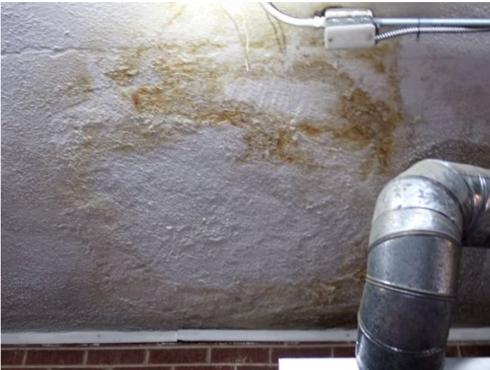
Unit 101: Active leak noted coming from roof drain. Restroom in poor condition. Recommend repairs.
