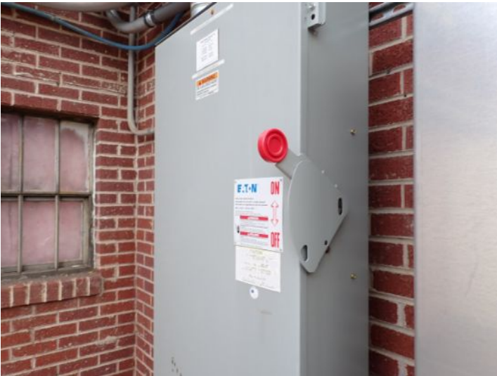
The main electrical disconnects appeared functional at the time of the inspection.
