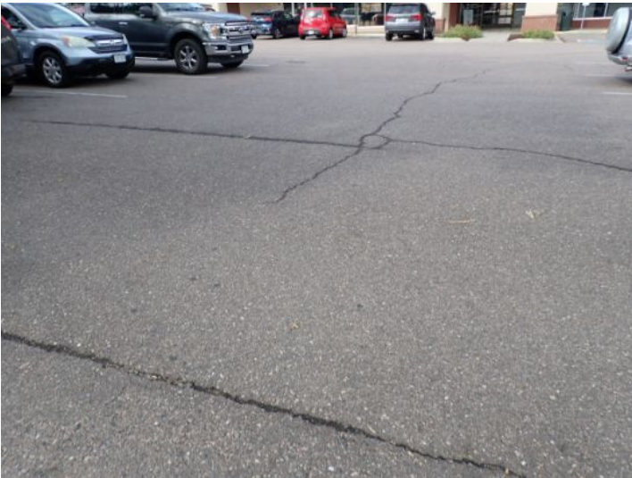
Recommend crack filling to aid in extending the life of the existing asphalt surface. Recommend repairs by a licensed contractor.
