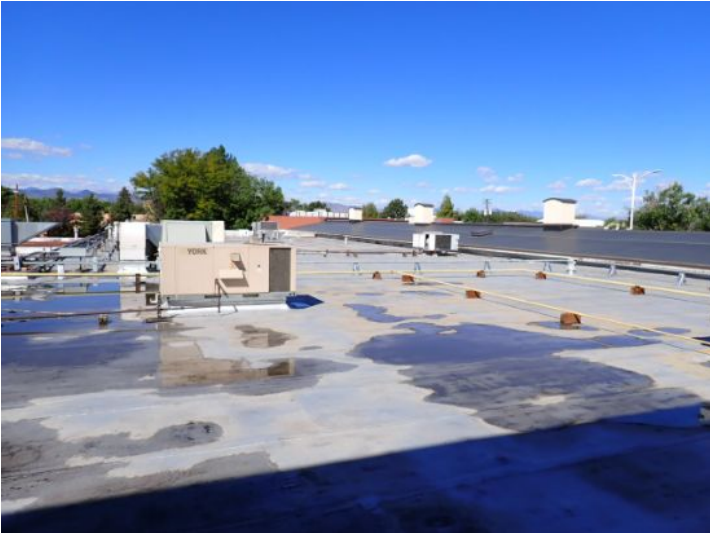
The rolled torch down roofing system located on the lower level south wing of the structure showing signs of excessive deferred maintenance, excessive ponding, possible hail damage and age. Recommend complete replacement by licensed contractor.
