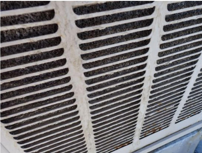
The swamp coolers located above the old theater area that is now being used as office or in fair to poor condition and require servicing and filter repairs by a licensed contractor. Recommend repairs prior to taking possession of the property.
