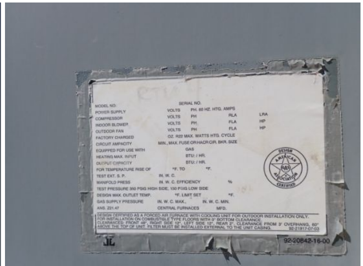
RTU 26: RUUD: M/N ? S/N ? Manufacture year ?
