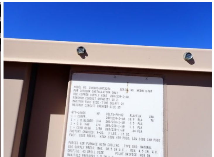
RTU 15: York: M/N D1NA036N07225A S/N NKEM116707. Manufacture year 1996.
