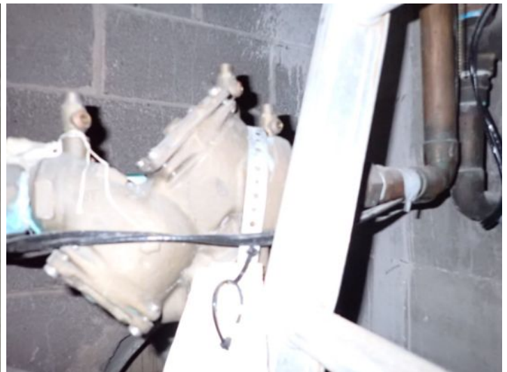
Last date of inspection/certification of the main backflow preventers appeared to be 7/22.
