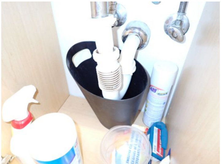
Unit 104: Sub standard plumbing noted below vanity sink. Past moisture staining noted in ceiling. Recommend repairs.
