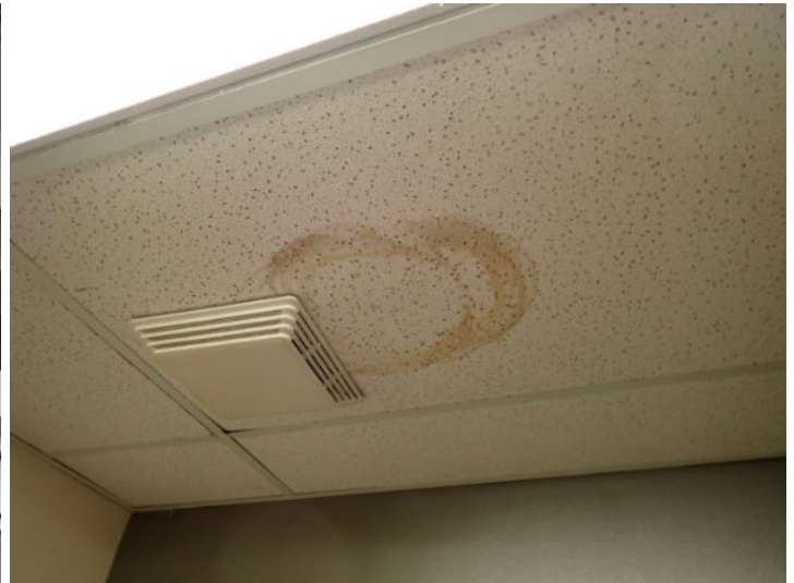
Unit 118: Moisture staining noted in ceiling. Moisture damage noted in drywall ceiling. Recommend repairs and monitoring.
