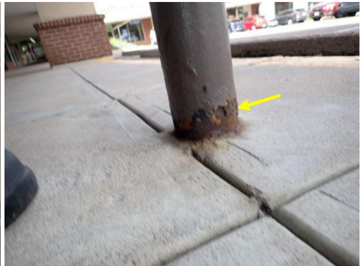
Minor rusting noted on some of the steel support posts for the front overhangs. Recommend repairs by a licensed contractor.
