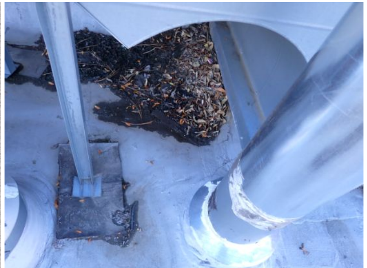
The rolled torch down roofing system located above the east end of the south wing appear did reach the end of its serviceable life expectancy with areas of significant ponding and cracking noted. Recommend repairs/replacement by licensed contractor.
