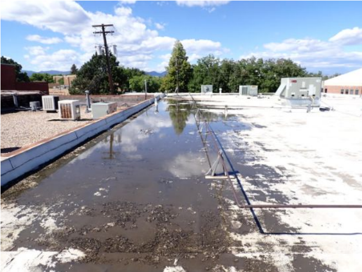
The rolled torch down roofing system above what appeared to be the old family dollar store and the vacant unit was an extremely poor condition excessive ponding feeling coding possible hail damage and excessive wear noted at the time of the inspection. Recommend complete replacement by licensed contractor.
