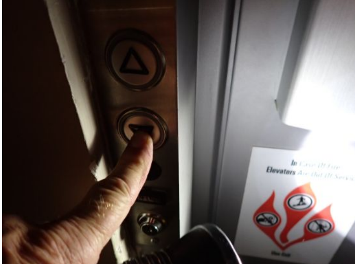
The chair lift system located in the mall area for the church was locked out and could not be tested at the time of the inspection. Based on the inspectors conversation with church personnel the system functions properly.
