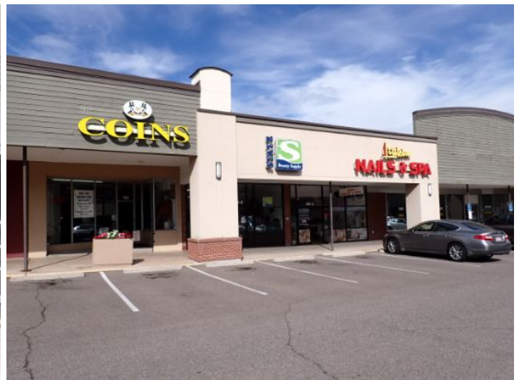
The majority of the exterior envelope of the structure appeared to be in fair condition with no significant structural movement noted at the time of the inspection.
