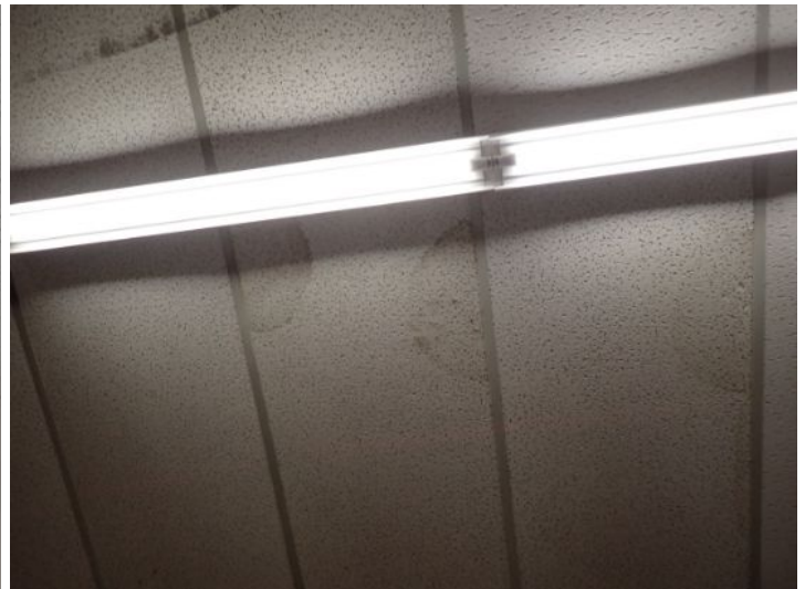
Unit 111-112: Moisture staining noted in ceiling tiles. Moisture damage noted in warehouse ceiling. Water heater not functional. Drywall ceiling damage noted. Recommend repairs.
