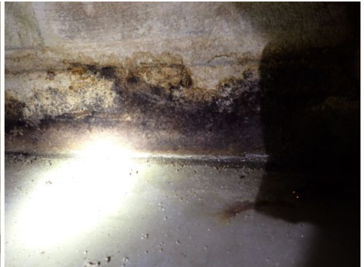
Unit 108-107: Vacant: Unit will require significant renovations prior to installing tenant. Active moisture noted in interior wall with possible microbial growth. Significant drywall damage noted in ceiling and walls in loading dock area. Basement area in poor condition. Basement bathrooms in poor condition. Electrical not working at the time of the inspection. Moisture intrusion/damage noted in basement walls. Recommend repairs as needed by a licensed contractor.
