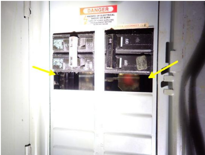
Unit 110G: Acoustical tile ceiling damage noted. Missing knockouts noted in electrical panel. Recommend repairs.
