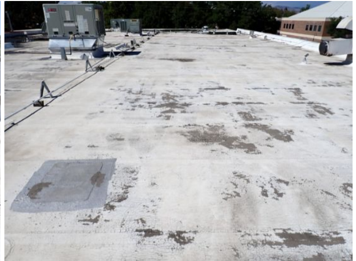
The rolled torch down roofing system above what appeared to be the old family dollar store and the vacant unit was an extremely poor condition excessive ponding feeling coding possible hail damage and excessive wear noted at the time of the inspection. Recommend complete replacement by licensed contractor.
