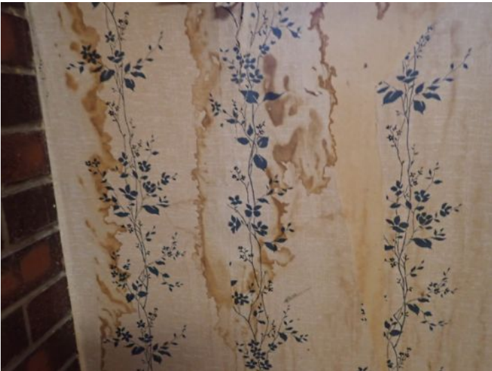
Unit 132: Unit was in poor condition and will require complete renovations prior to installing a new tenant.
