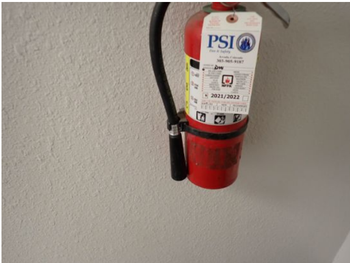
The fire suppression system was holding approximately 90 psi at the time of the inspection.
