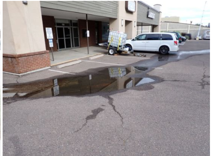
Poor drainage noted in areas. Recommend repairs by a licensed contractor.
