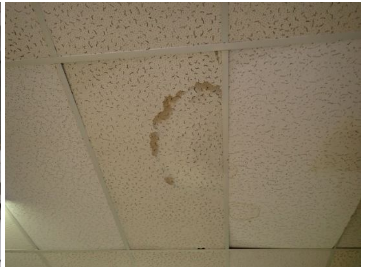
Unit 119: Moisture staining noted in ceiling tiles. Recommend repairs and monitoring
