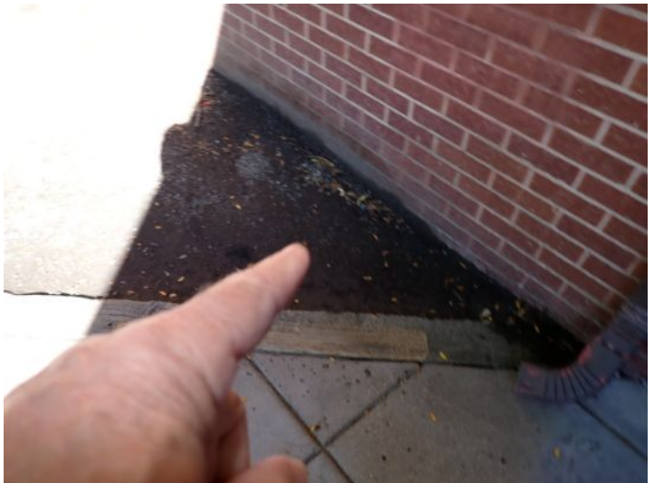
The topography of the property requires attention to assure that the grade directs ground/storm water away from the foundation of the structure.
