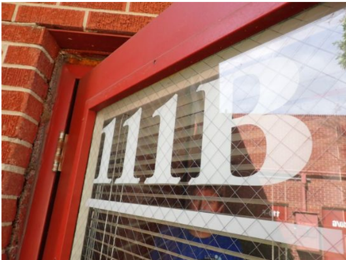
Unit 111B: Emergency egress goes through unit 111 which is locked at night. Recommend repairs by a licensed contractor prior to installing a new tenant.
