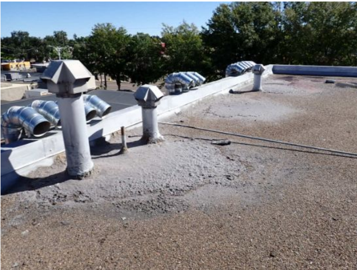
Excessive lint buildup noted on the roof tops above the laundry at the time of the inspection. This could be considered a fire hazard. Recommend cleaning by licensed contractor.
