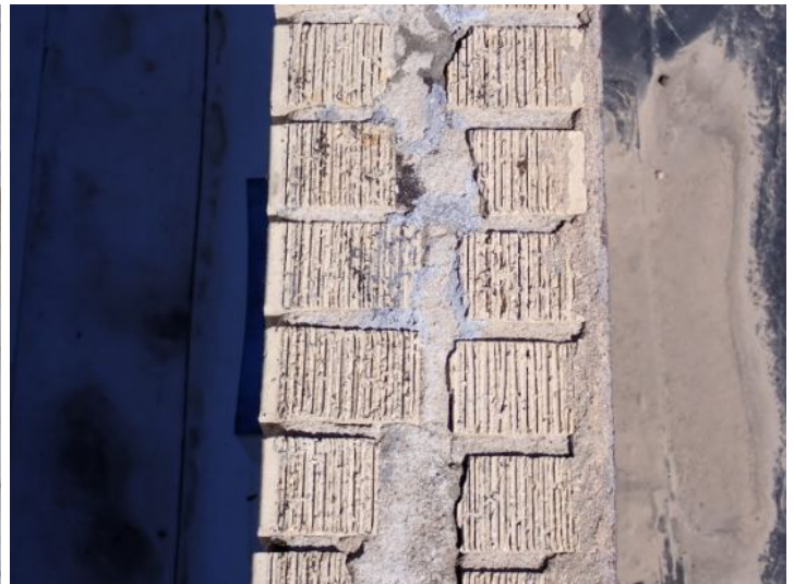
Recommend capping of all brick/block parapet walls with metal capping material. Recommend repairs by a licensed contractor.
