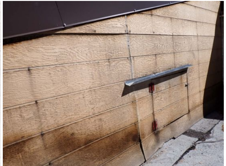
The wood siding material located above the corner awning roof on the ends of the pitched roof sections were in poor condition at the time of the inspection. Recommend repairs by a licensed contractor.
