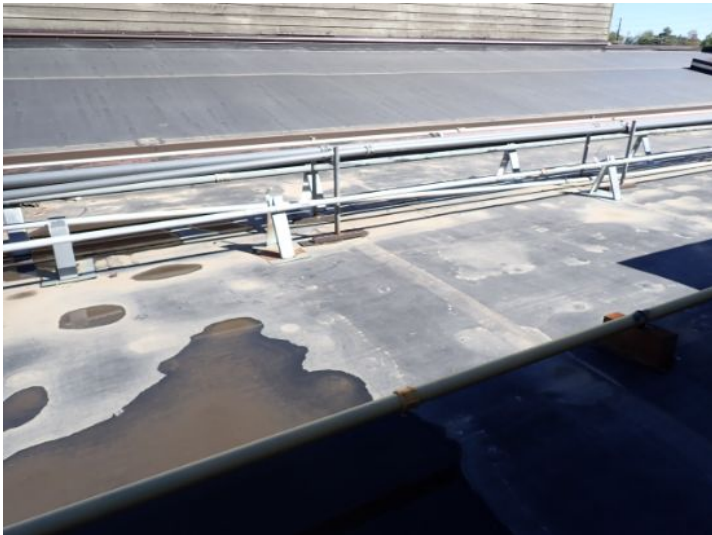
The EPDM roofing membrane located on the lower level of the south wing appeared to be in fair condition at the time of the inspection but was showing signs of excessive ponding and minor seam issues in areas. Recommend repairs as required by a licensed contractor.
