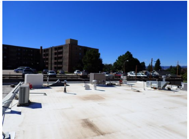
The TPO membrane located above the lower level west end of the south unit appeared to be in fair condition at time of inspection.
