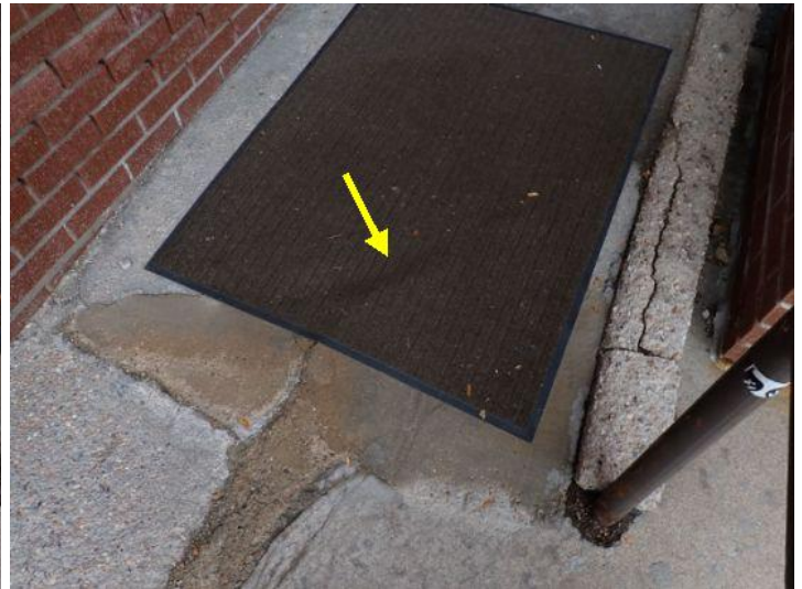
Damage/heaving noted on the flatwork at the ADA ramp for unit 100 (restaurant) at the time of the inspection. Recommend repairs by a licensed contractor.
