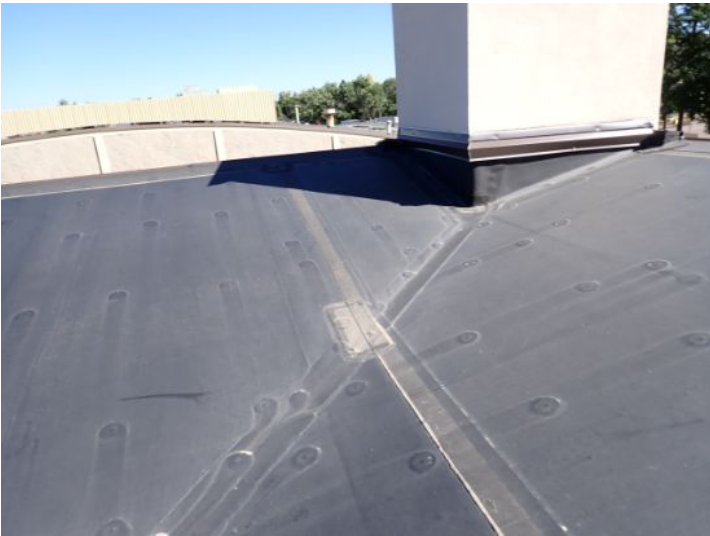
The EPDM membrane on the low slope front sections of each wing appeared be in fair condition at time of inspection. There were areas where it appeared that debris below the membrane was attempting to push through the membrane but had not penetrated at the time of the inspection. Recommend monitoring for future repairs.
