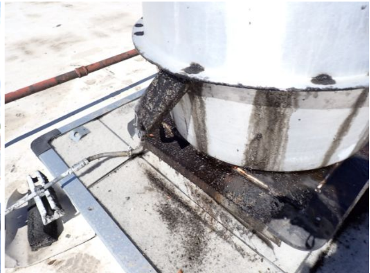
One or more kitchen roof top vent systems were showing signs of significant deferred maintenance. Recommend repairs by a licensed contractor.
