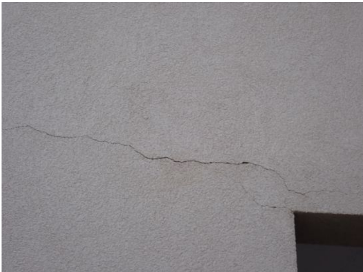
Stucco cracking noted in areas around the structure at the time of the inspection. Recommend repairs by a licensed contractor.
