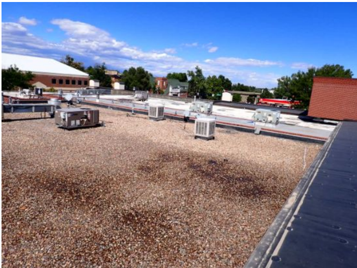
The gravel coated EPDM roofing membrane located towards the north end of the west structure was showing signs of significant ponding and deferred maintenance at the time of the inspection. Recommend repair by licensed contractor.
