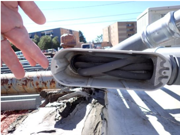
Missing cover plate noted on roof top pull box. Recommend repairs by a licensed contractor.
