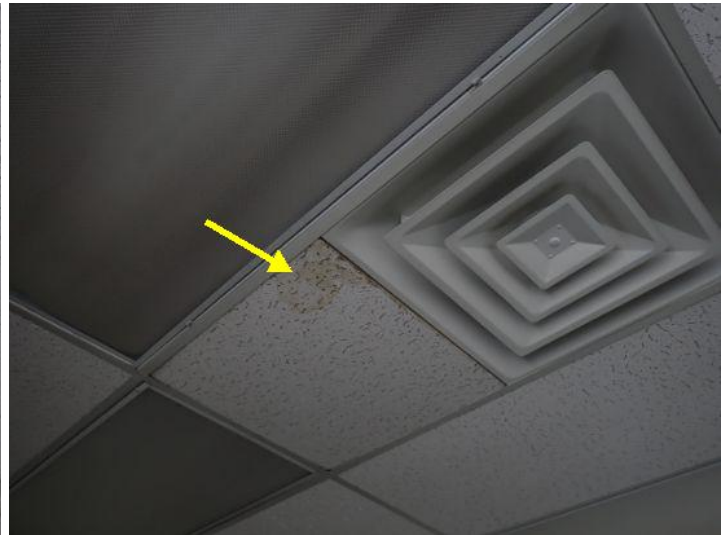
Moisture staining noted in areas of the acoustical tile ceilings throughout the building at the time of the inspection. Recommend repairs and monitoring
