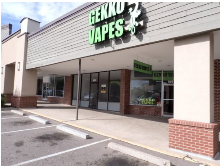
The majority of the exterior envelope of the structure appeared to be in fair condition with no significant structural movement noted at the time of the inspection.
