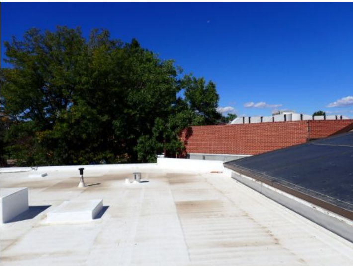
The TPO membrane located above the lower level west end of the south unit appeared to be in fair condition at time of inspection.
