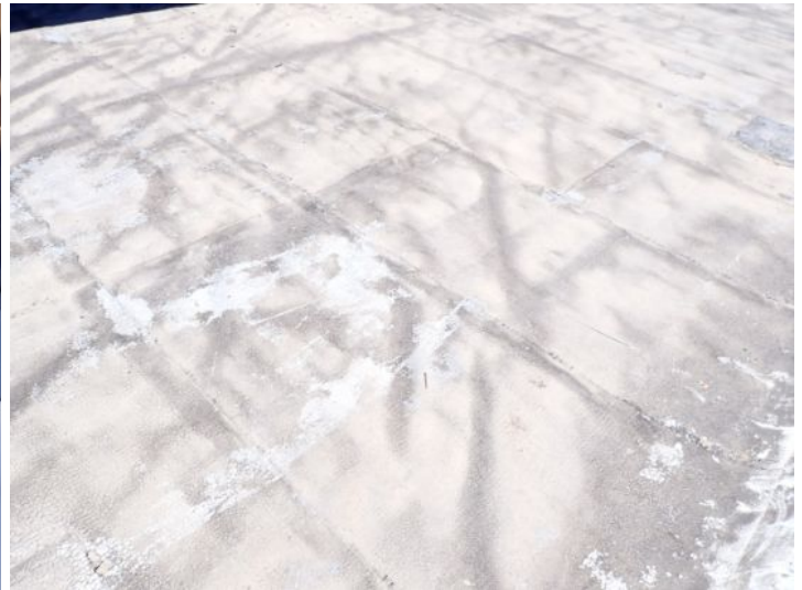
The narrow or small rolled torch down roofing system located approximately the center of the West Wing was an extremely poor condition of time inspection and requires completely recommend a licensed roofing contractor
