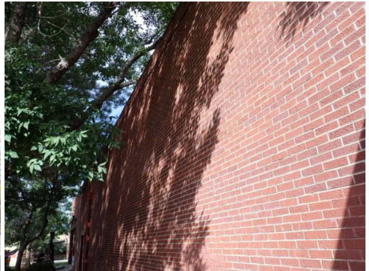
The majority of the exterior envelope of the structure appeared to be in fair condition with no significant structural movement noted at the time of the inspection.
