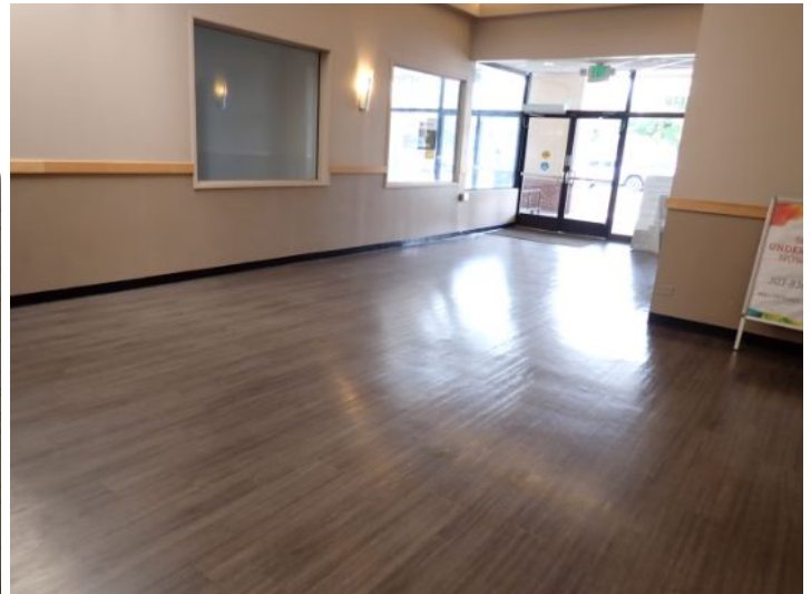
The majority of the interior common areas of the structure appeared to be in fair condition at the time of the inspection.
