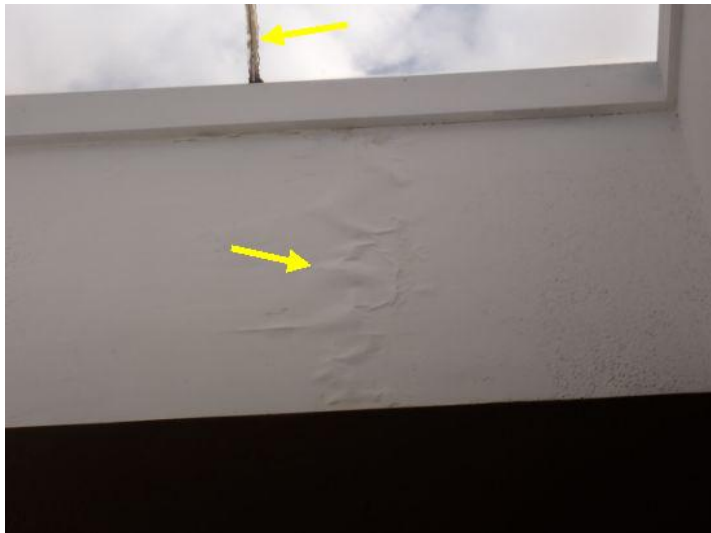
Cracked/leaking skylight system noted above the mall area. Recommend replacement by a licensed contractor.
