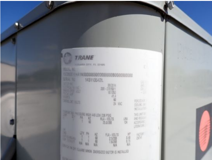
RTU 31: Trane: M/N YSC060E1EHA1N00000 S/N 143113542L. Manufacture year 2014.
