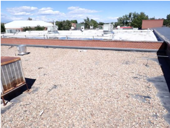
The gravel coated EPDM roofing membrane located towards the north end of the west structure was showing signs of significant ponding and deferred maintenance at the time of the inspection. Recommend repair by licensed contractor.
