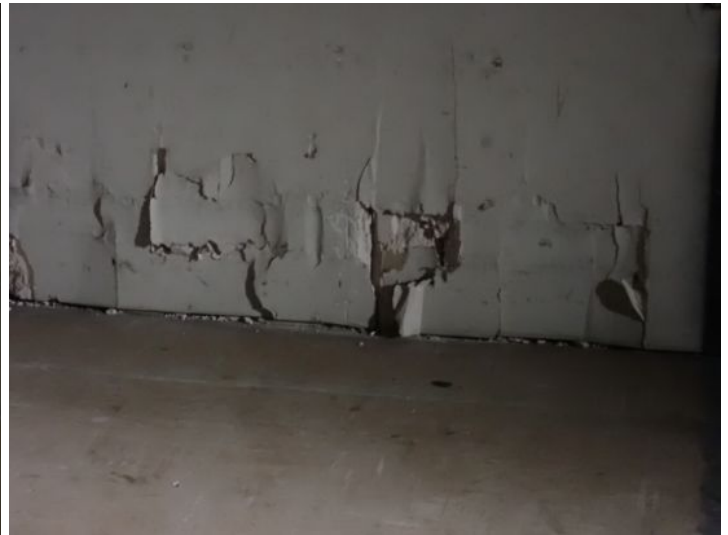
Unit 108-107: Vacant: Unit will require significant renovations prior to installing tenant. Active moisture noted in interior wall with possible microbial growth. Significant drywall damage noted in ceiling and walls in loading dock area. Basement area in poor condition. Basement bathrooms in poor condition. Electrical not working at the time of the inspection. Moisture intrusion/damage noted in basement walls. Recommend repairs as needed by a licensed contractor.
