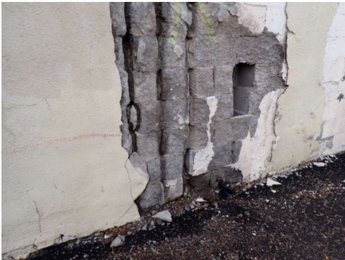
The block retaining wall for the neighboring parking garage was showing signs of significant moisture damage and deterioration in areas. Recommend monitoring to aid in possibly preventing wall failure onto your property.
