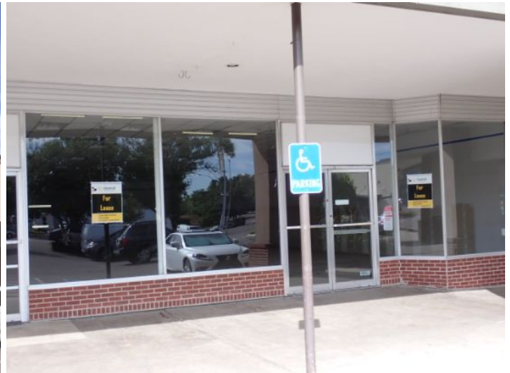
Missing safety stamps noted on some of the required safety glass panels. This is typical of structures of this age. Today's standards require that any glass located within 18" of grade level next to a walkway, in an operable door, with a leaking edge within 24" of an operable door or with a total of 9 sq. ft. or larger be glazed with safety glass and be labeled as such. Recommend repairs as needed by a certified glazing contractor.
