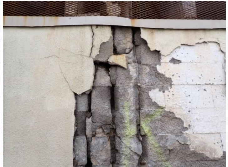
The block retaining wall for the neighboring parking garage was showing signs of significant moisture damage and deterioration in areas. Recommend monitoring to aid in possibly preventing wall failure onto your property.
