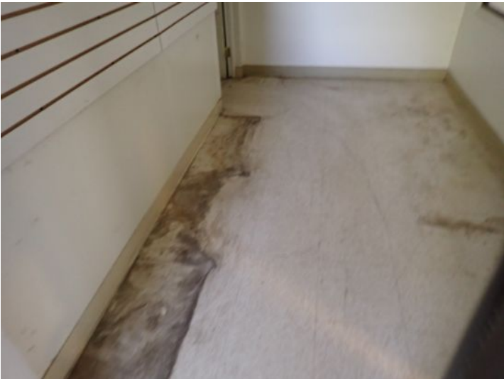
Unit 110E: Unit was vacant and will require renovations prior to placing a tenant. Recommend repairs by a licensed contractor.
