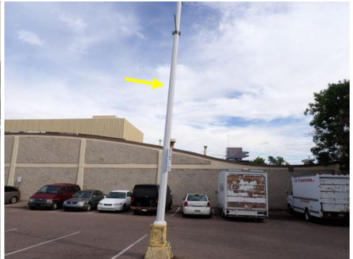
Leaning light post noted on the east side of the parking lot at the time of the inspection. Recommend repairs by a licensed contractor.
