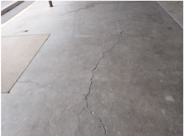
Minor cracking. Recommend monitoring for future repairs.
