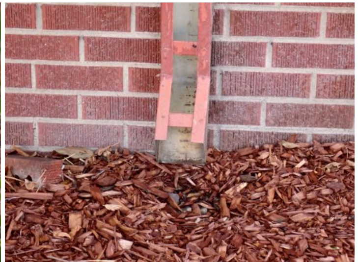
Gutters down spouts missing extensions to direct storm water away from the foundation of the structure. Recommend repairs.
