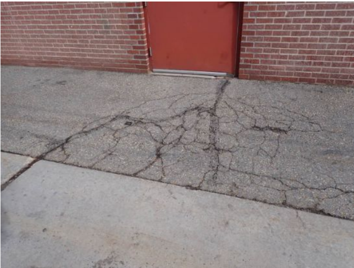
The asphalt running along the rear south side of the structure was in poor condition at the time of the inspection. Recommend resurfacing by a licensed contractor.
