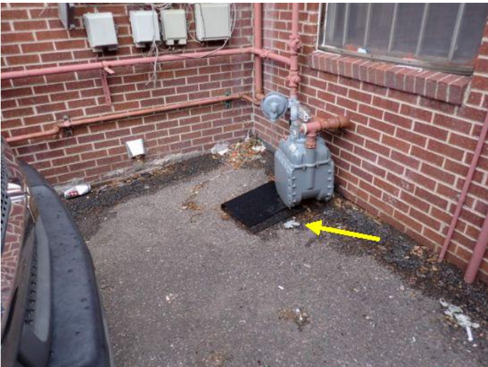
Missing protective bollard noted at one of the gas meters on the west side of the structure at the time of the inspection. Recommend repairs by a licensed contractor.
