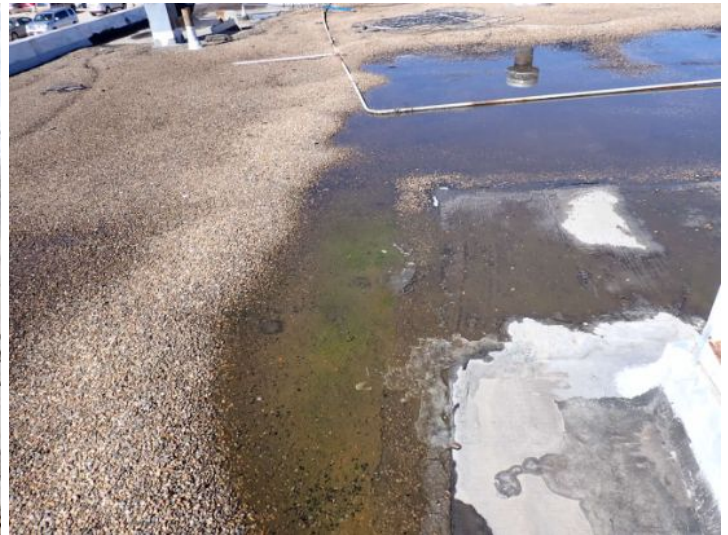
The BUR roofing system located on the east end of the south wing of the building is showing signs of excessive wear excessive ponding it was an extremely poor condition at the time of the inspection. Recommend replacement by a licensed contractor.
