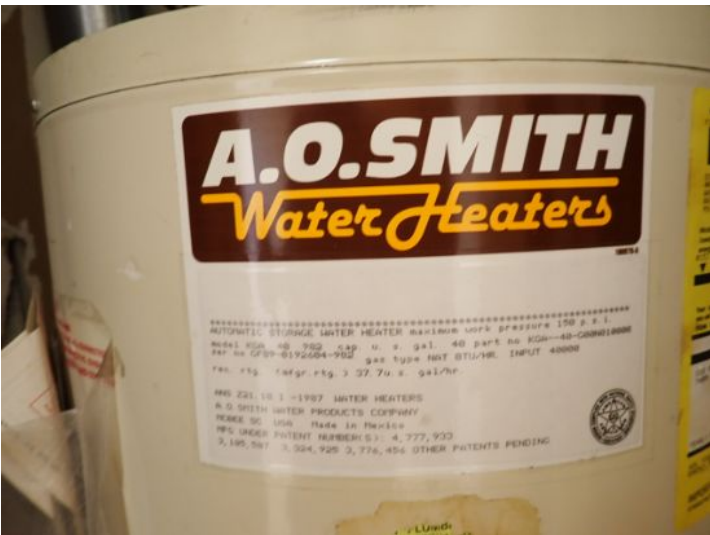
The nominal serviceable life expectancy of a gas fired water heater is 10 years. Based on the inspectors findings there were multiple units noted throughout the property that have surpassed their serviceable life expectancy. Recommend replacement or budgeting for replacement by a licensed contractor.
