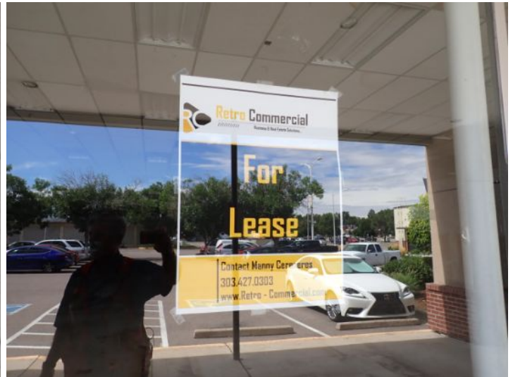
Unit 108-107: Vacant: Unit will require significant renovations prior to installing tenant. Active moisture noted in interior wall with possible microbial growth. Significant drywall damage noted in ceiling in loading dock area. Basement area in poor condition. Basement bathrooms in poor condition. Electrical not working at the time of the inspection. Moisture intrusion/damage noted in basement walls. Recommend repairs as needed by a licensed contractor.
