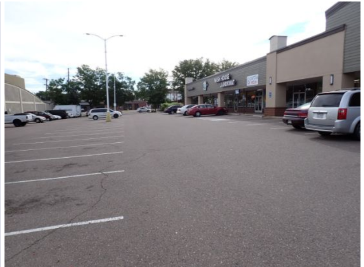
The majority of the parking lot surface was in fair condition at the time of the inspection.
