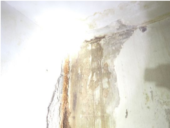
Unit 108-107: Vacant: Unit will require significant renovations prior to installing tenant. Active moisture noted in interior wall with possible microbial growth. Significant drywall damage noted in ceiling and walls in loading dock area. Basement area in poor condition. Basement bathrooms in poor condition. Electrical not working at the time of the inspection. Moisture intrusion/damage noted in basement walls. Recommend repairs as needed by a licensed contractor.
