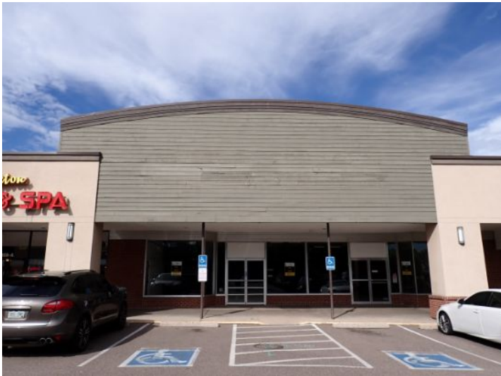
The majority of the exterior envelope of the structure appeared to be in fair condition with no significant structural movement noted at the time of the inspection.
