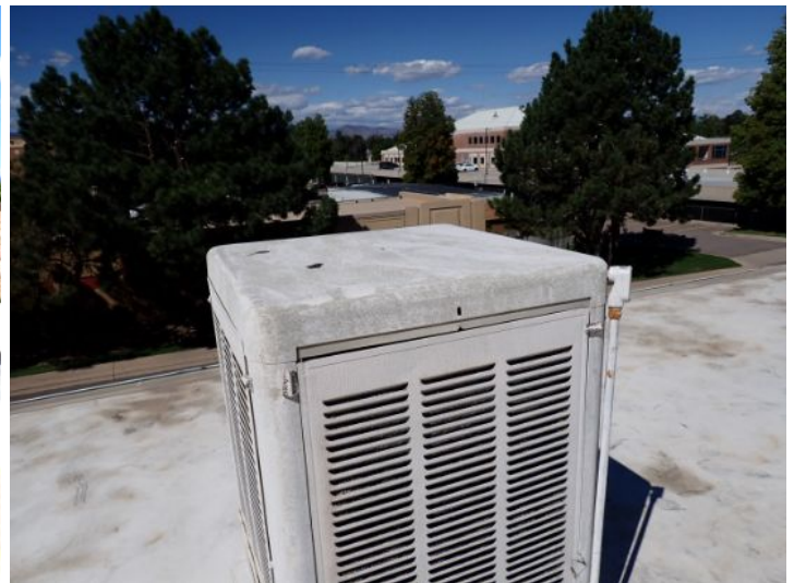
The swamp coolers located on the roofing system above the mall area were in poor condition or not functional at the time of the inspection. If the systems are still in use they require repair or replacement by licensed contractor.
