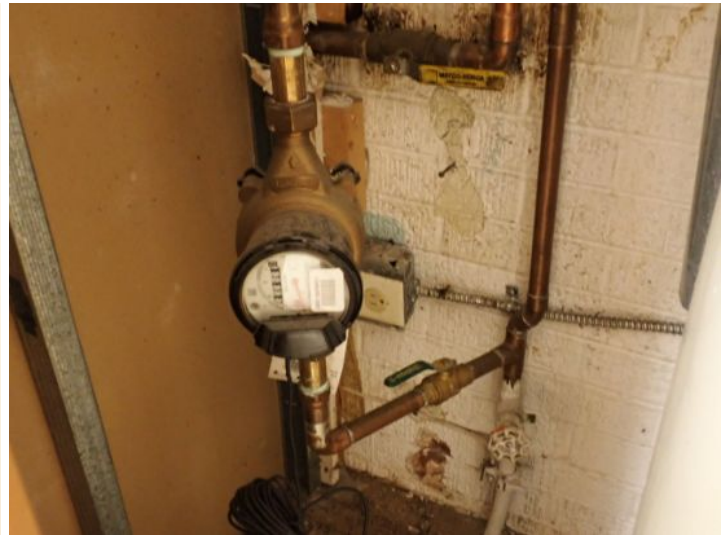
Some of the tenant units appeared to have sub meters located within them but the meters did not appear to be functional at the time of the inspection. Recommend consulting with the current owners/management company to determine what is going on with these systems as well as where the main shutoffs are all located and how water metering is performed.
