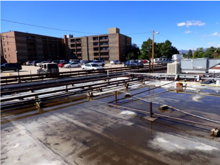
The rolled torch down roofing system located on the lower level south wing of the structure showing signs of excessive deferred maintenance, excessive ponding, possible hail damage and age. Recommend complete replacement by licensed contractor.
