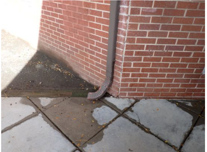
The topography of the property requires attention to assure that the grade directs ground/storm water away from the foundation of the structure.
