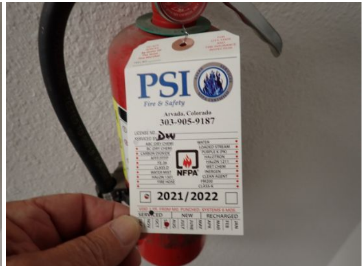
Last date of inspection/certification for the fire extinguishers was 9/21.
