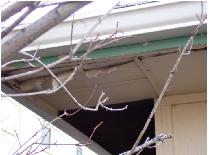
Moisture damaged soffit/eave material noted in areas around both of the structures at the time of the inspection. This was most likely caused by ice damming which was caused by inadequate attic insulation and ventilation. Recommend repairs as needed by a licensed contractor.
