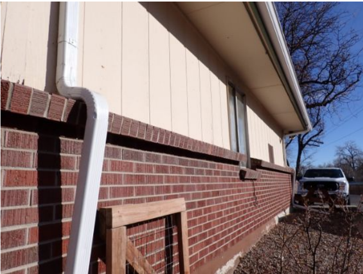
The majority of the exterior envelopes of the structures appeared to be in fair condition at the time of the inspection.
