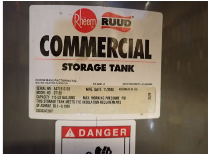
West Bldg. Holding Tank: Rheem/RUUD: M/N ST120 S/N A471810193. Manufacture year 2018.
