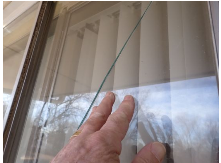
Unit 13: Cracked window glass. Broken window glass in rear of unit. Tub/shower surround requires caulk/grout repairs. Tub finish in poor condition. Closet door damage noted. Vinyl flooring damage noted. Recommend repairs.
