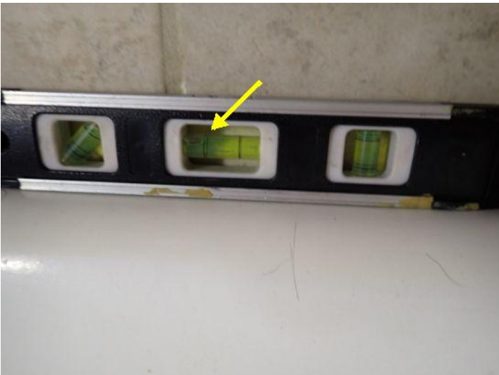
Unit 1: Significant floor deflection noted. Missing bedroom door. Significant wall/ceiling junction cracking noted. Carpet damage. Significant floor settling noted. Recommend repairs.
