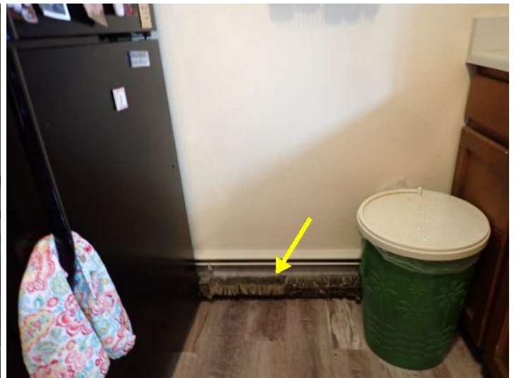
Unit 20: Damaged radiator system noted. Significant flooring deflection noted. Tub finish in poor condition. Significant wall movement noted. Recommend repairs.
