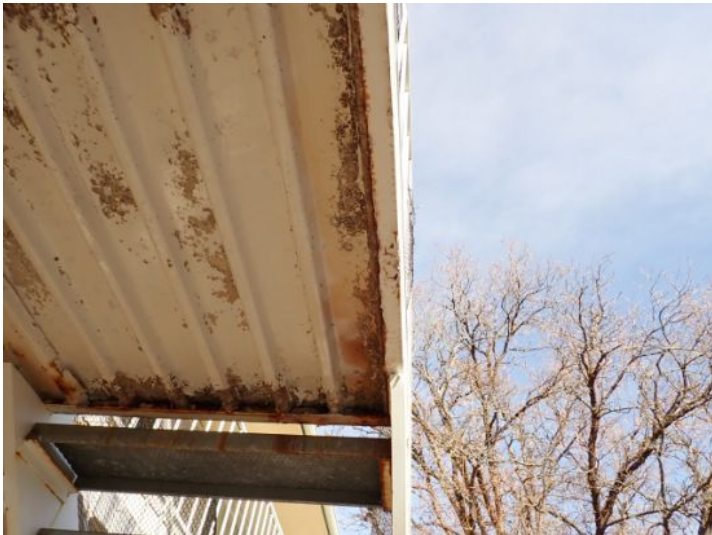
Pan rusting and deterioration noted below the upper level walkways and landings at the time of the inspection. Recommend repairs by a licensed contractor prior to taking possession of the property.
