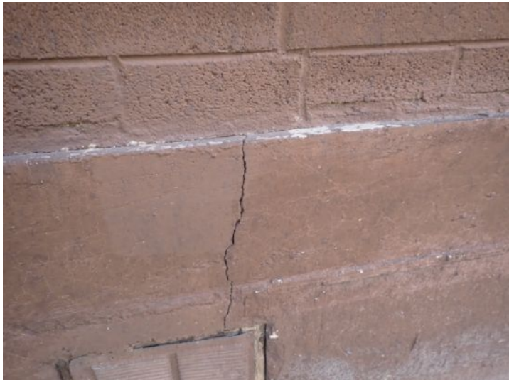
Minor foundation wall cracking noted in areas. Recommend monitoring for future repairs.
