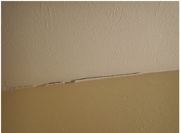
Unit 24: Carpet in poor condition. Ceiling/wall junction cracking. Vinyl floor damage. Wall damage noted below kitchen sink. Recommend repairs.
