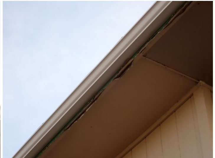
Moisture damaged fascia noted in areas. Recommend repairs by a licensed contractor.
