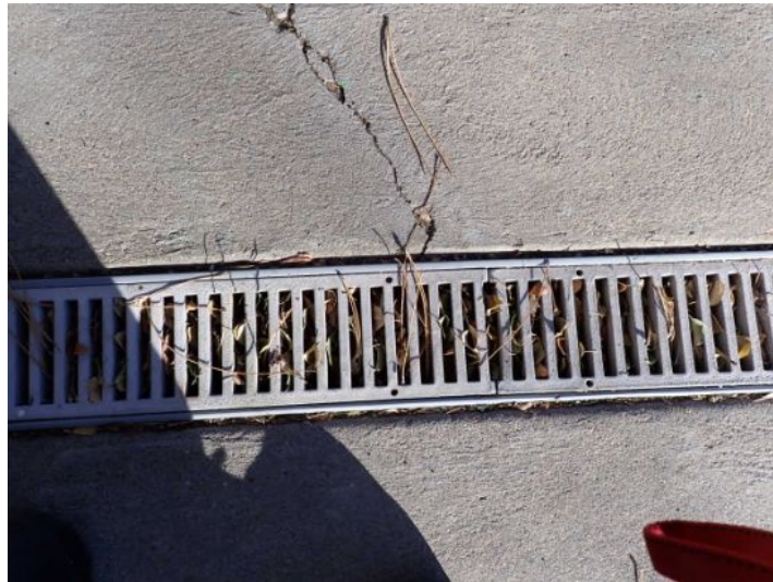
Drainage systems blocked by debris in areas. Recommend repairs.
