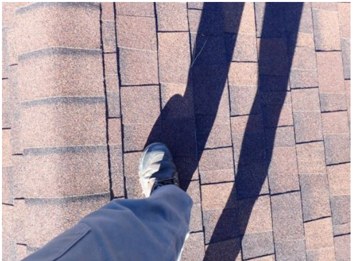
Spongy/weak decking noted under foot on both roofing systems at the time of the inspection. Recommend monitoring for future repairs.
