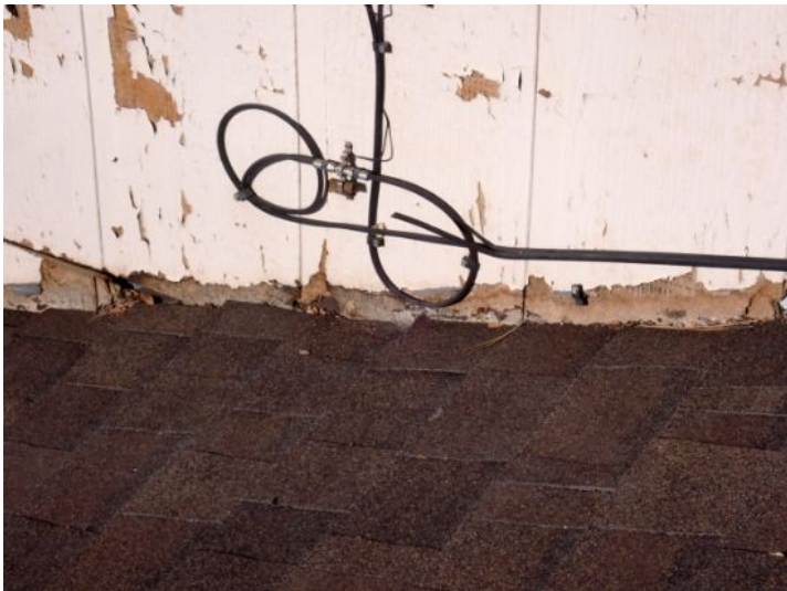
Wood rot/deterioration noted on the wood/composition siding in areas on both structures at the time of the inspection. Recommend repairs by a licensed contractor.
