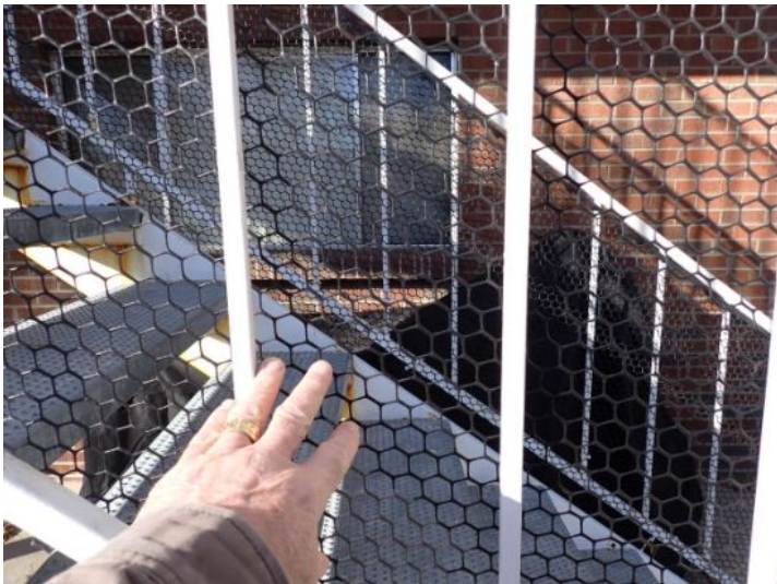
Balustrade openings too wide on the stairs and upper level railing systems at the time of the inspection. Opening should not exceed 4". Recommend repairs by a licensed contractor.
