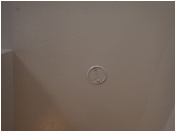
One or more smoke alarms or carbon monoxide detectors missing at the time of the inspection. Recommend repairs by a licensed contractor,
