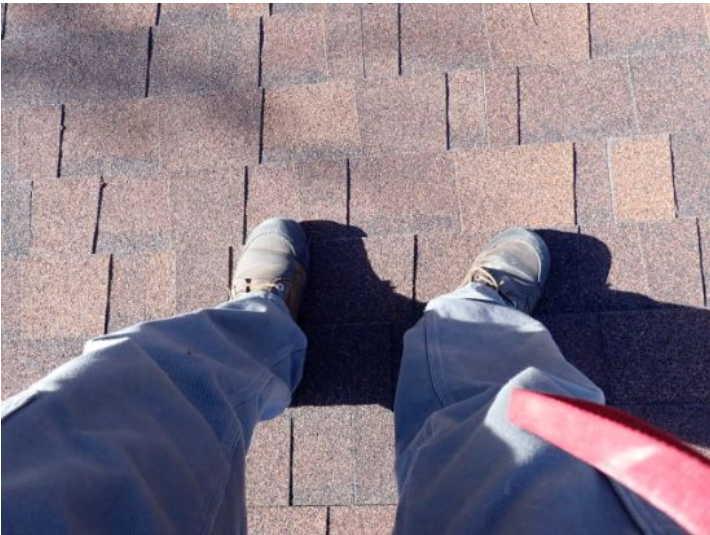
Spongy/weak decking noted under foot on both roofing systems at the time of the inspection. Recommend monitoring for future repairs.
