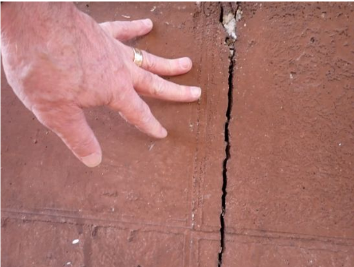
Significant foundation wall cracking noted on both structures at the time of the inspection. Recommend repairs by a licensed contractor.
