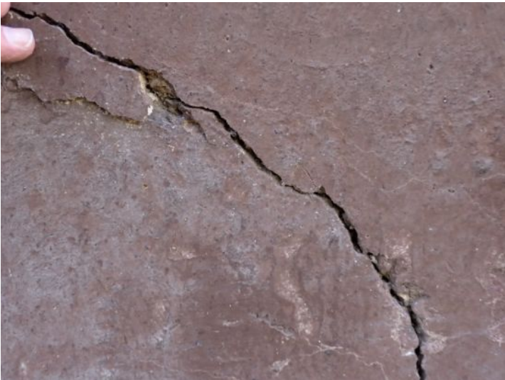
Significant foundation wall cracking noted on both structures at the time of the inspection. Recommend repairs by a licensed contractor.
