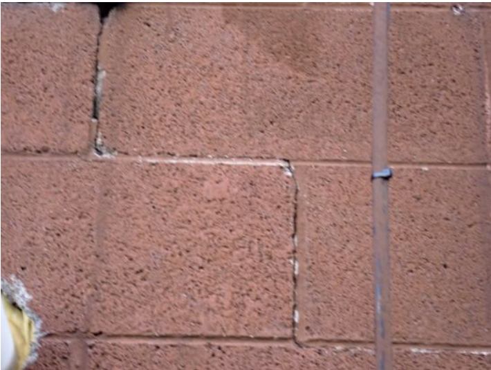
Cracked mortar noted in areas. Recommend tuck pointing repairs by a licensed contractor.
