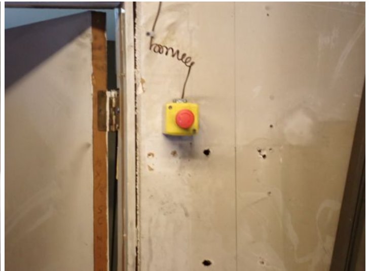
The emergency shutdown switches for the boiler systems were in place and appeared functional at the time of the inspection.
