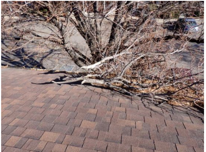
Tree touching roof on the upper west side structure. Recommend removal and roof evaluation in this area prior to taking possession of the property.
