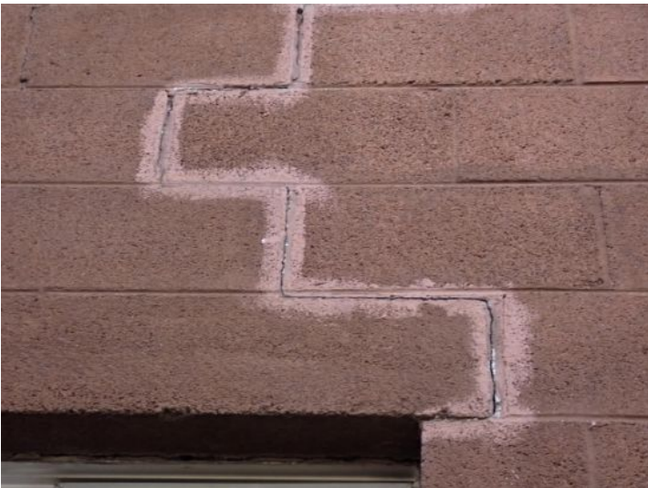
Cracked mortar noted in areas. Recommend tuck pointing repairs by a licensed contractor.
