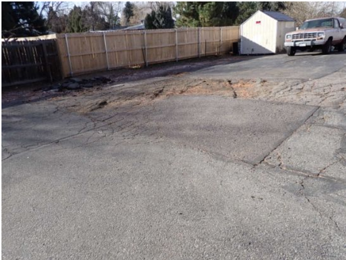
Significant deterioration noted in areas of the parking lots surface. Recommend repairs by a licensed contractor.
