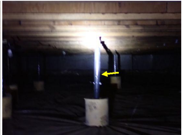
Leaning support posts noted in areas below the structures at the time of the inspection. Recommend repairs by a licensed contractor.
