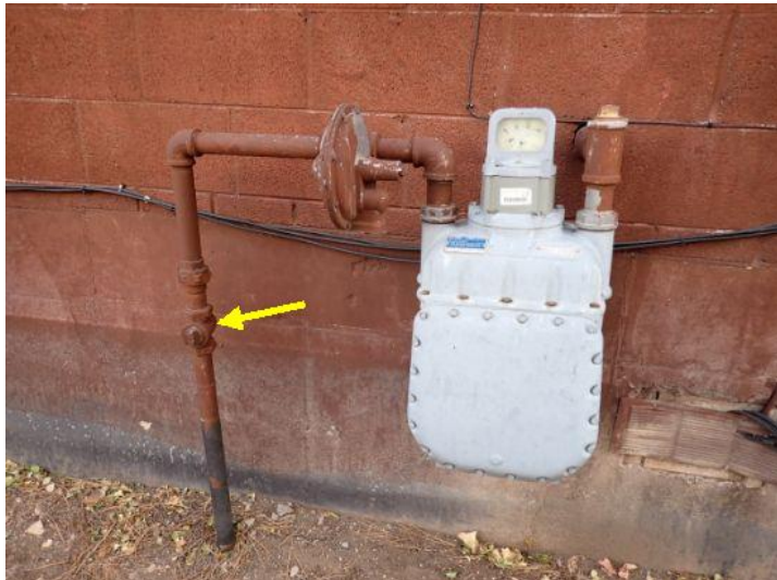
The main gas shutoff valve(s) was/were functional at the time of the inspection
