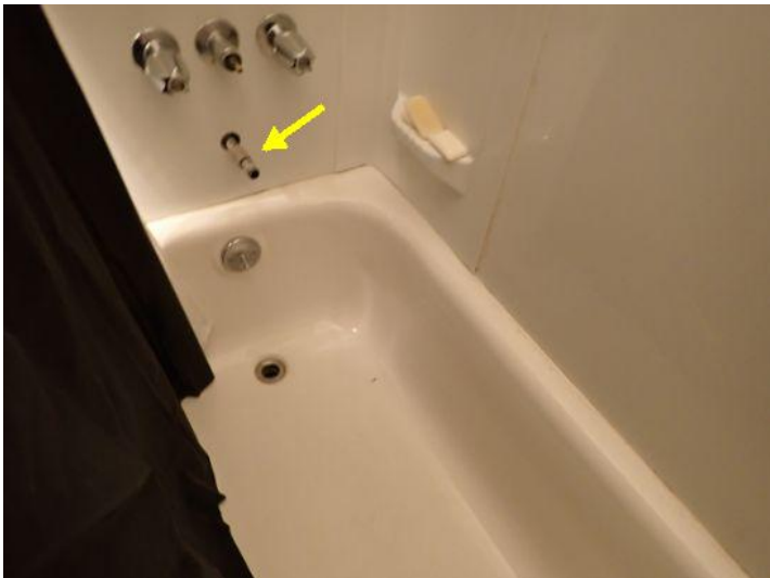
Unit 21: Missing cover plate noted on electrical panel. Wall damage noted in bathroom. Flooring damage noted. Tub spigot missing. Recommend repairs.
