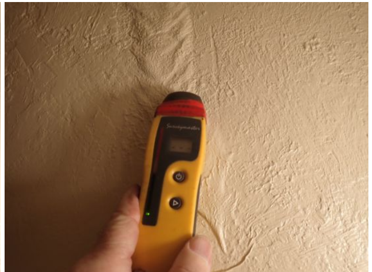
Unit 4: Kitchen counter and wall separation noted. Vanity sink rusting. Past moisture damage noted in bathroom wall but no moisture present at the time of the inspection. Recommend repairs.
