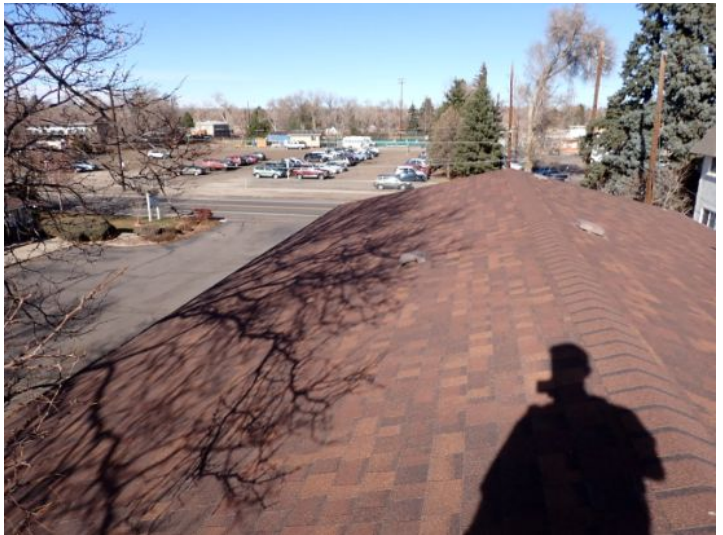
The majority of the roofing systems appeared to be in fair condition at the time of the inspection.
