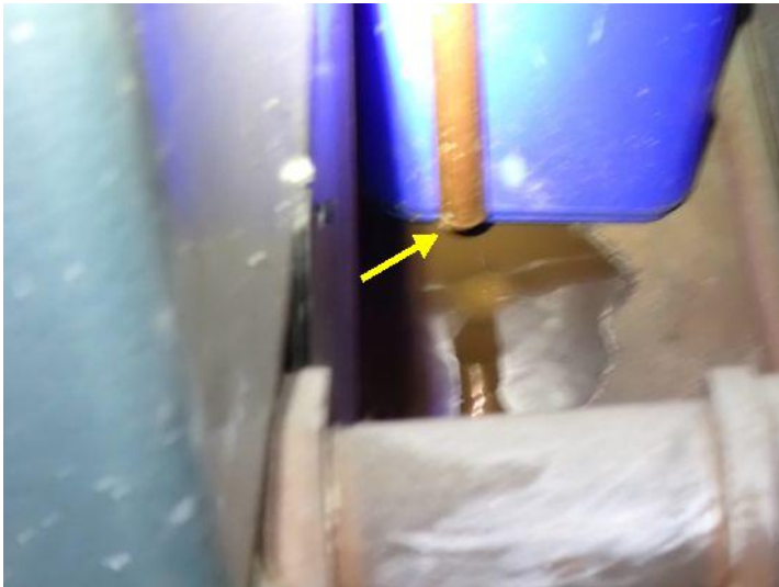
East Bldg. Boiler: The TPRV for the boiler was leaking at the time of the inspection. Recommend repairs by a licensed contractor.
