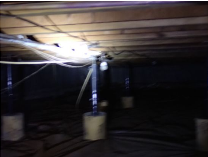
Due to the amount of structural movement, flooring deflection as well as improper/inadequate past repairs we recommend that both of the structures be evaluated by a licensed structural contractor prior to taking possession of the property.
