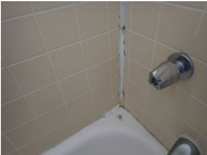
Unit 10: Flooring damage. Tub/shower surround requires caulk/grout repairs. Tub finish in poor condition. Broken bathroom window glass. Recommend repairs.
