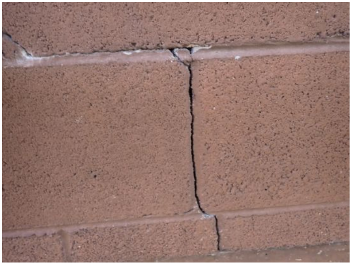
Cracked mortar noted in areas. Recommend tuck pointing repairs by a licensed contractor.
