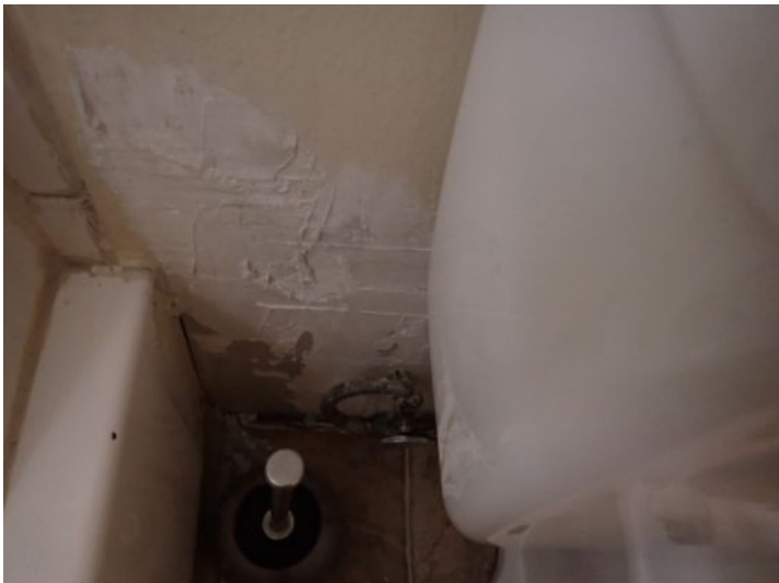
Unit 22: Carpeting in poor condition. Vinyl flooring damage noted. Missing dead cover on electrical panel. Wall damage noted in bathroom. Cracked mirror on closet door. Recommend repairs.
