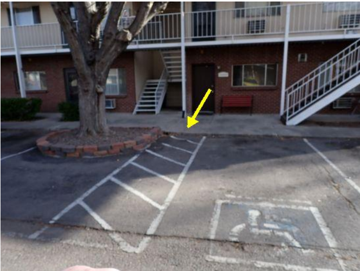
No ADA ramp system installed at the ADA parking area on the east side structure at the time of the inspection.
