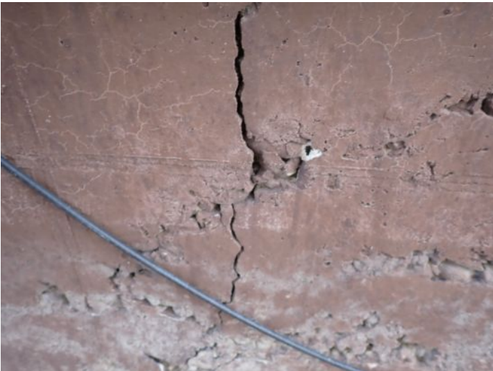
Significant foundation wall cracking noted on both structures at the time of the inspection. Recommend repairs by a licensed contractor.
