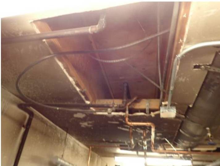
Damaged ceilings noted in boiler rooms at the time of the inspection. Fire Hazard. Recommend repairs by a licensed contractor.
