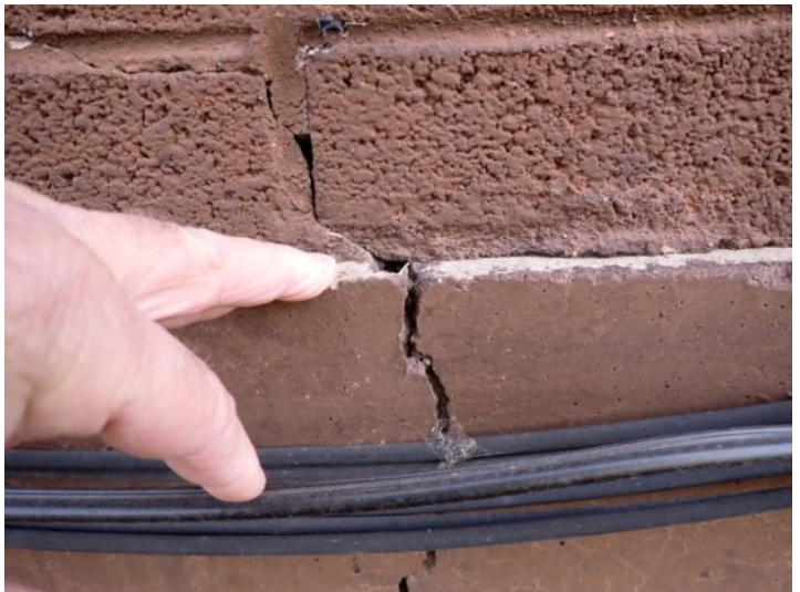
Significant foundation wall cracking noted on both structures at the time of the inspection. Recommend repairs by a licensed contractor.
