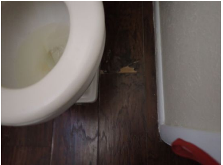
Unit 10: Flooring damage. Tub/shower surround requires caulk/grout repairs. Tub finish in poor condition. Broken bathroom window glass. Recommend repairs.
