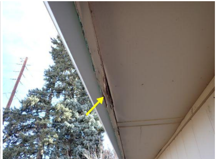
Moisture damaged fascia noted in areas. Recommend repairs by a licensed contractor.
