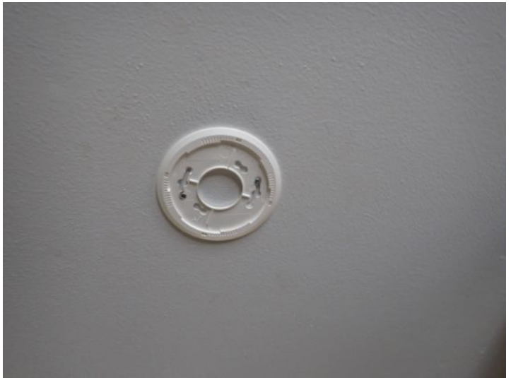
One or more smoke alarms or carbon monoxide detectors missing at the time of the inspection. Recommend repairs by a licensed contractor,
