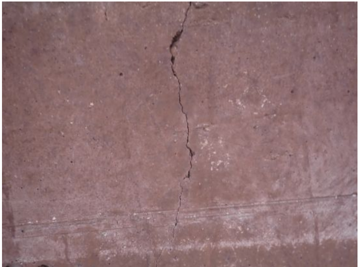
Minor foundation wall cracking noted in areas. Recommend monitoring for future repairs.
