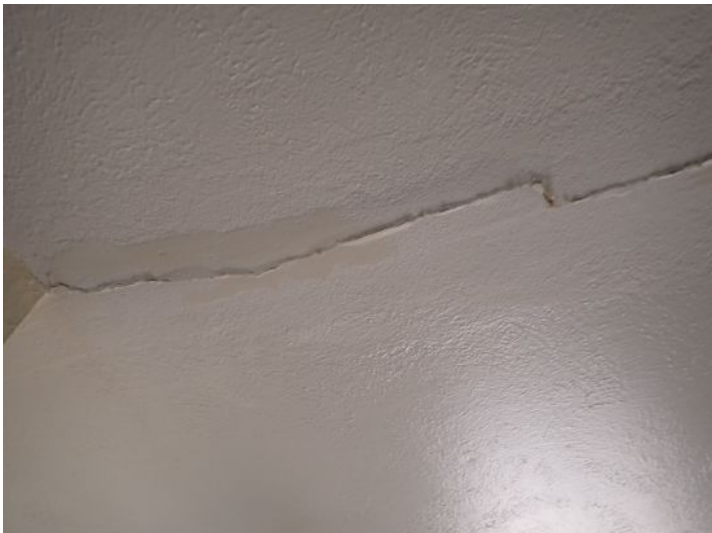
Unit 9: Ceiling cracking. Sub standard plumbing noted below kitchen sink. Carpet in poor condition. Tub finish in poor condition. Recommend repairs.
