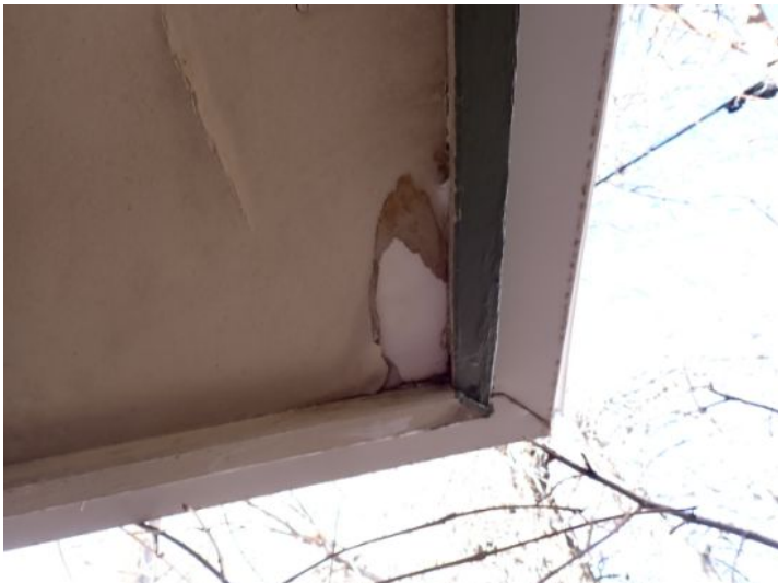
Moisture damaged soffit/eave material noted in areas around both of the structures at the time of the inspection. This was most likely caused by ice damming which was caused by inadequate attic insulation and ventilation. Recommend repairs as needed by a licensed contractor.
