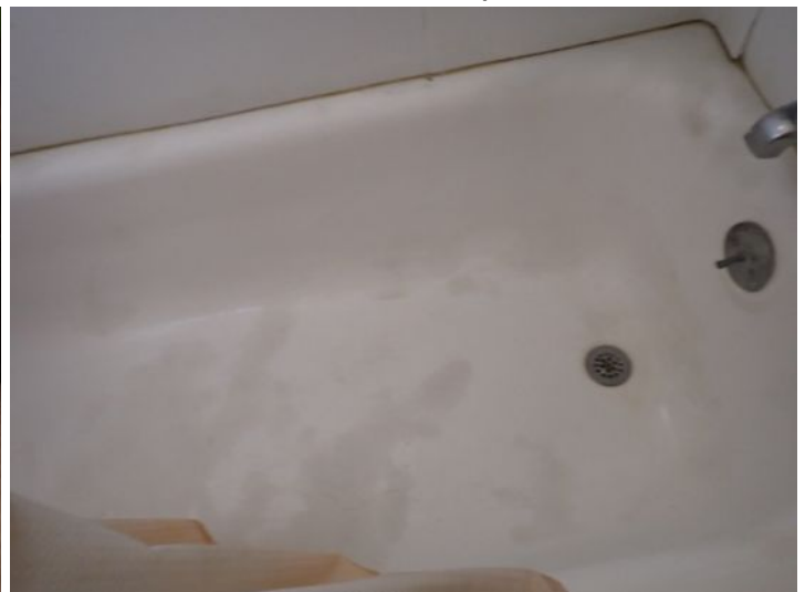
Unit 20: Damaged radiator system noted. Significant flooring deflection noted. Tub finish in poor condition. Significant wall movement noted. Recommend repairs.
