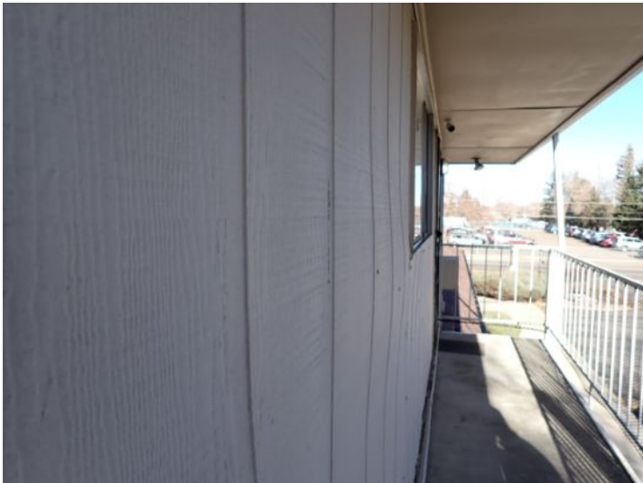
Warped siding material noted on upper level east side of west building. Recommend repairs by a licensed contractor.
