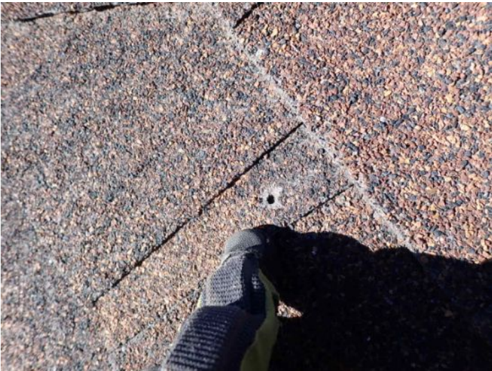
Minor shingle damaged noted in areas at the time of the inspection. Recommend monitoring for future repairs.
