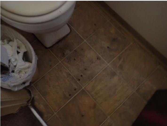
Unit 12: Carpet in poor condition. Vinyl flooring damage. Moisture damage noted below bedroom window. Recommend repairs.
