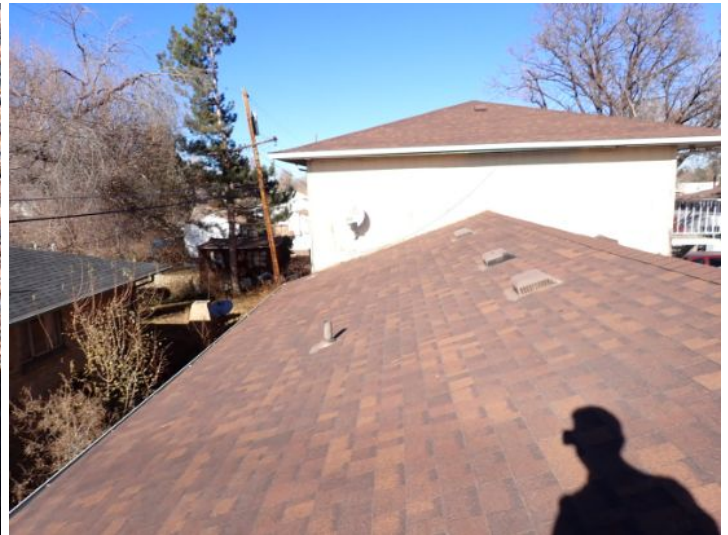
The majority of the roofing systems appeared to be in fair condition at the time of the inspection.
