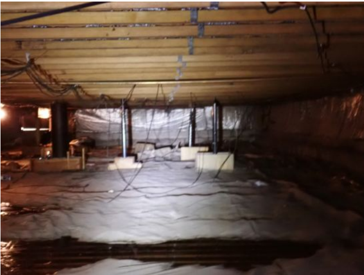
Due to the amount of structural movement, flooring deflection as well as improper/inadequate past repairs we recommend that both of the structures be evaluated by a licensed structural contractor prior to taking possession of the property.
