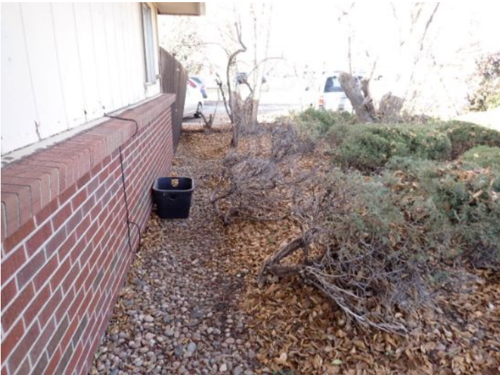
The landscaping requires attention.
