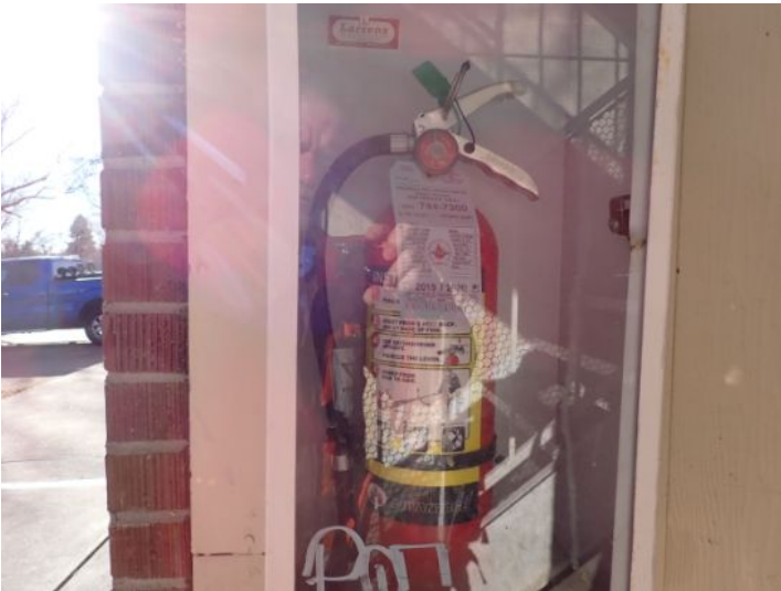
There were fire extinguishers located within the common areas of the structure
