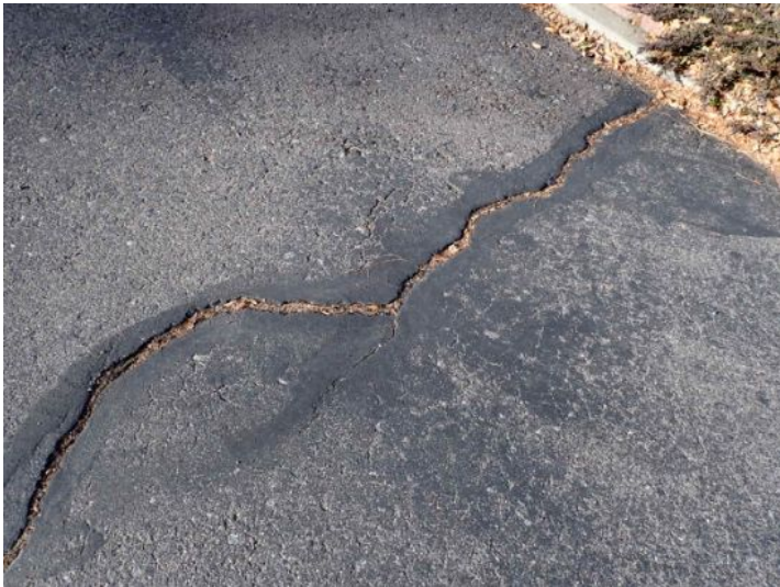
Recommend crack filling to aid in extending the life of the existing asphalt surface. Recommend repairs by a licensed contractor.
