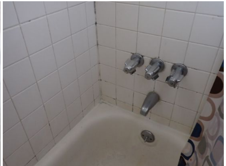
Unit 13: Cracked window glass. Broken window glass in rear of unit. Tub/shower surround requires caulk/grout repairs. Tub finish in poor condition. Closet door damage noted. Vinyl flooring damage noted. Recommend repairs.
