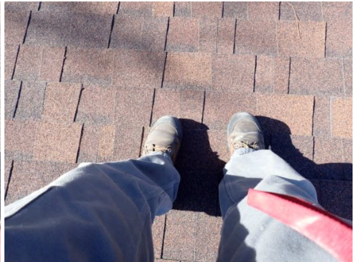
Spongy/weak decking noted under foot on both roofing systems at the time of the inspection. Recommend monitoring for future repairs.
