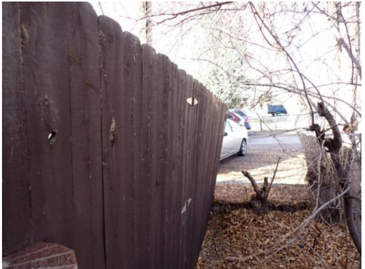
Fencing damage noted around the property at the time of the inspection. Recommend repairs by a licensed contractor.
