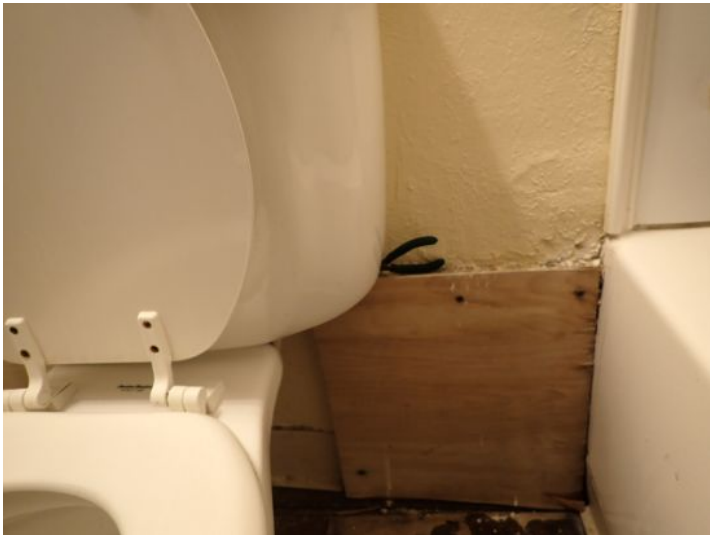
Unit 21: Missing cover plate noted on electrical panel. Wall damage noted in bathroom. Flooring damage noted. Tub spigot missing. Recommend repairs.
