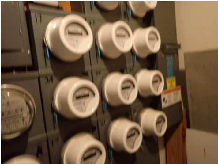
The tenant units were individually metered for electricity at the time of the inspection.
