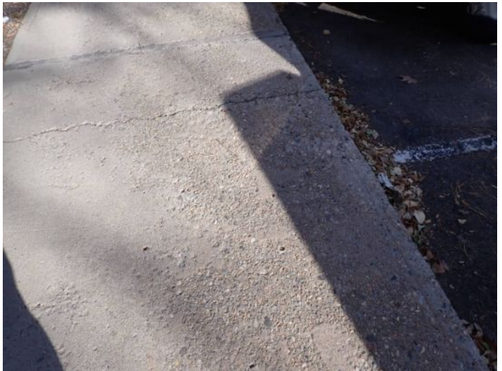
Significant spalling noted in areas of the flatwork at the time of the inspection. Recommend repairs by a licensed contractor.
