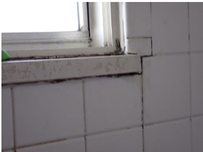
Unit 13: Cracked window glass. Broken window glass in rear of unit. Tub/shower surround requires caulk/grout repairs. Tub finish in poor condition. Closet door damage noted. Vinyl flooring damage noted. Recommend repairs.
