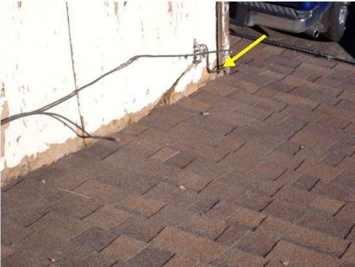
Missing kickout flashing noted in areas on the lower level roofing systems. Recommend repairs by a licensed contractor.
