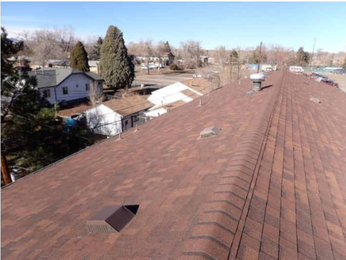
The majority of the roofing systems appeared to be in fair condition at the time of the inspection.
