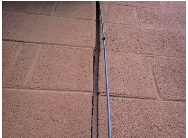
Expansion joint sealant repairs required in areas. Recommend repairs by a licensed contractor.
