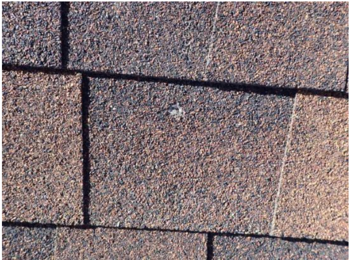
Minor shingle damaged noted in areas at the time of the inspection. Recommend monitoring for future repairs.
