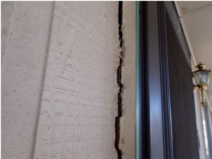
Unit 11: Front door trim damaged. Significant flooring deflection. Flooring damage noted. Recommend repairs.
