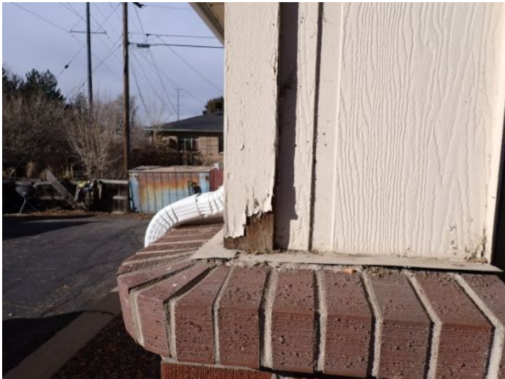
Peeling paint noted on the wood/composition siding material on both structures. Recommend repairs by a licensed contractor.
