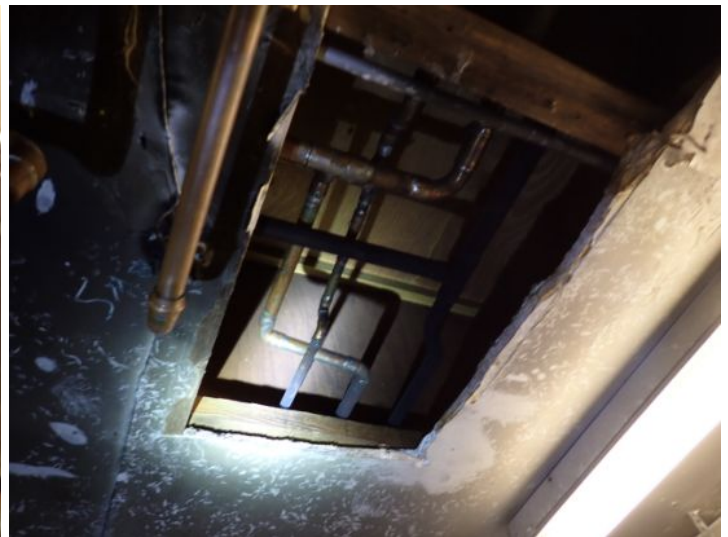
Damaged ceilings noted in boiler rooms at the time of the inspection. Fire Hazard. Recommend repairs by a licensed contractor.
