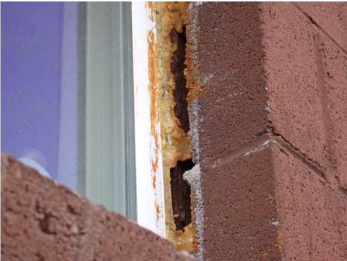
Recommend assuring that any area where 2 separate substrates meet should be properly caulked/sealed. Recommend repairs by a licensed contractor.
