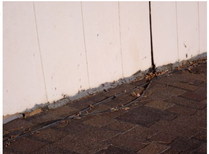
Siding material touching the roofing material in areas at the time of the inspection. Recommend repairs by a licensed contractor.
