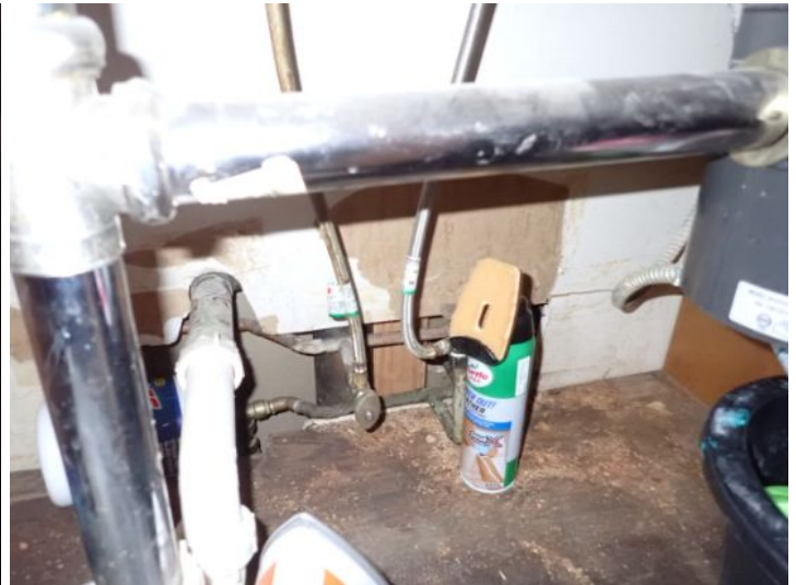
Unit 24: Carpet in poor condition. Ceiling/wall junction cracking. Vinyl floor damage. Wall damage noted below kitchen sink. Recommend repairs.
