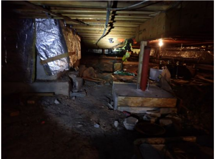
Due to the amount of structural movement, flooring deflection as well as improper/inadequate past repairs we recommend that both of the structures be evaluated by a licensed structural contractor prior to taking possession of the property.
