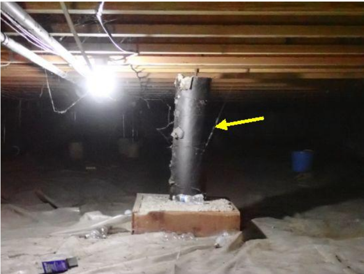
Leaning support posts noted in areas below the structures at the time of the inspection. Recommend repairs by a licensed contractor.
