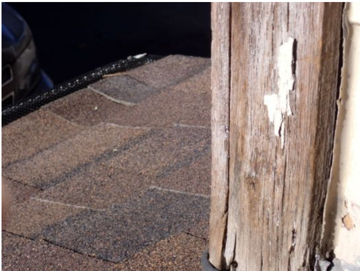
Missing/rotted/deteriorated wood trim noted in areas at the time of the inspection. Recommend repairs by a licensed contractor.
