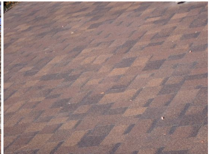
The majority of the roofing systems appeared to be in fair condition at the time of the inspection.
