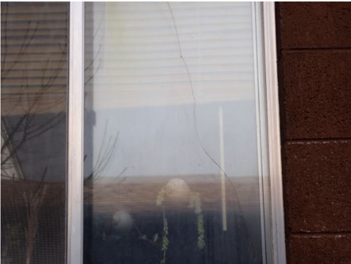
Cracked/broken window glass noted in areas. Recommend repairs by a licensed contractor.
