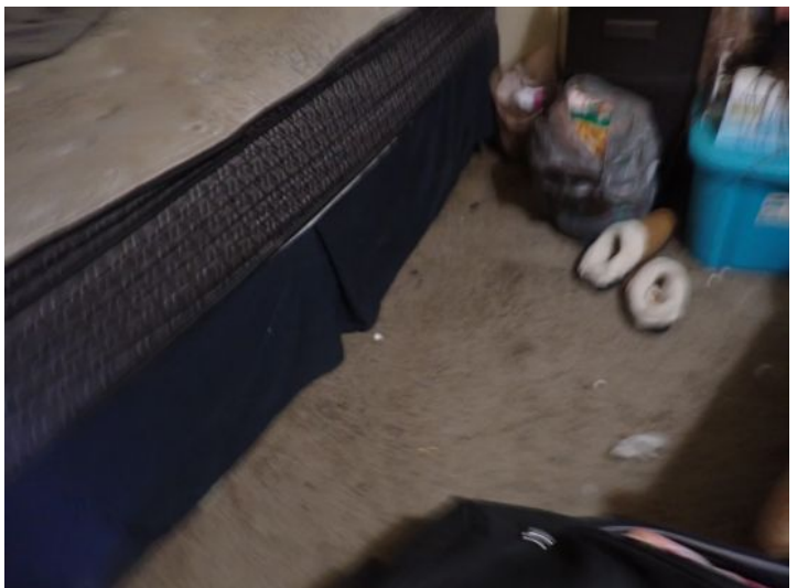
Unit 8: Carpet in poor condition. Recommend repairs.
