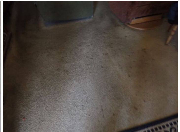
Unit 23: Carpet damage noted. Tub in poor condition. Recommend repairs.
