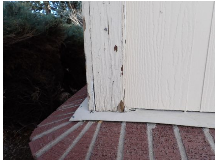
Peeling paint noted on the wood/composition siding material on both structures. Recommend repairs by a licensed contractor.
