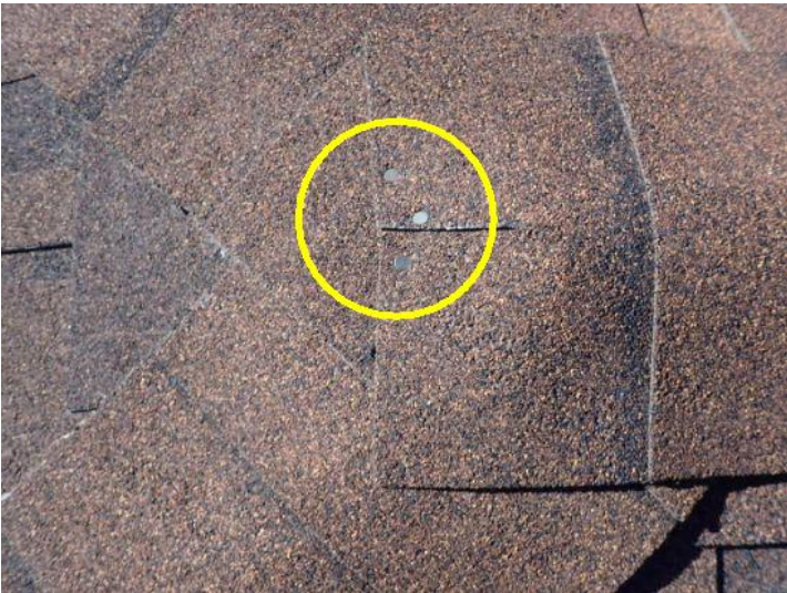
Missing sealant on exposed ridge row nails noted on the west side structures roof at the time of the inspection. Recommend repairs by a licensed contractor.
