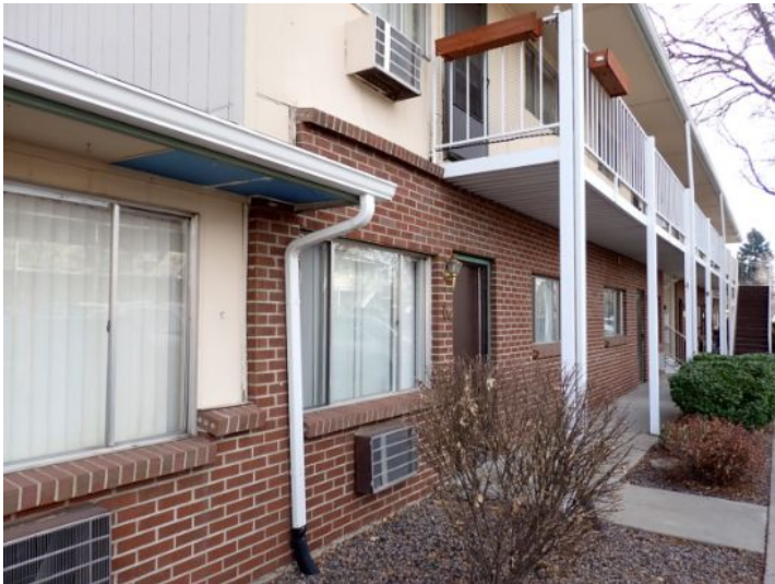
The majority of the exterior envelopes of the structures appeared to be in fair condition at the time of the inspection.
