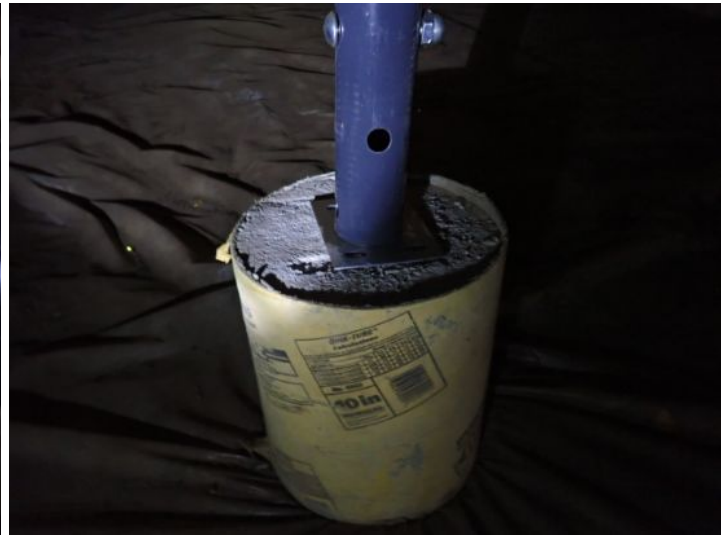
Due to the amount of structural movement, flooring deflection as well as improper/inadequate past repairs we recommend that both of the structures be evaluated by a licensed structural contractor prior to taking possession of the property.
