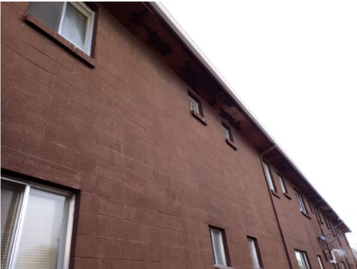
The majority of the exterior envelopes of the structures appeared to be in fair condition at the time of the inspection.
