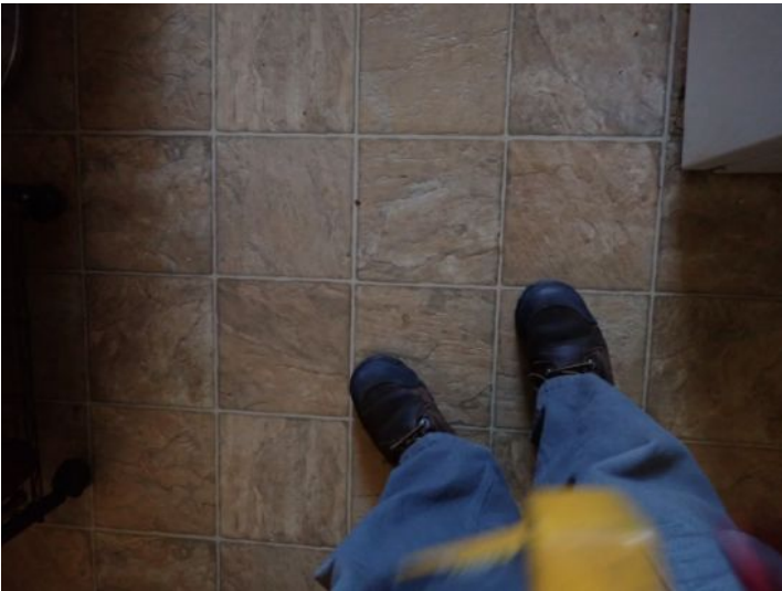
Unit 1: Significant floor deflection noted. Missing bedroom door. Significant wall/ceiling junction cracking noted. Carpet damage. Significant floor settling noted. Recommend repairs.
