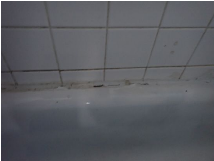
Unit 18: Carpet damage noted. Tub/shower surround requires caulk/grout repairs. Significant flooring deflection noted. Recommend repairs.
