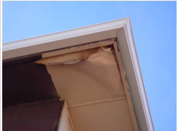
Moisture damaged soffit/eave material noted in areas around both of the structures at the time of the inspection. This was most likely caused by ice damming which was caused by inadequate attic insulation and ventilation. Recommend repairs as needed by a licensed contractor.
