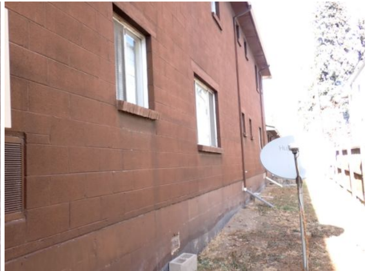
The majority of the exterior envelopes of the structures appeared to be in fair condition at the time of the inspection.
