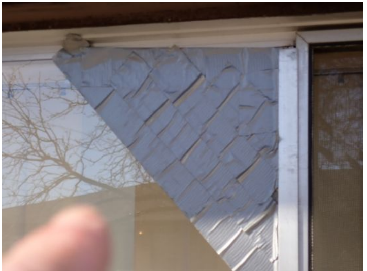
Cracked/broken window glass noted in areas. Recommend repairs by a licensed contractor.
