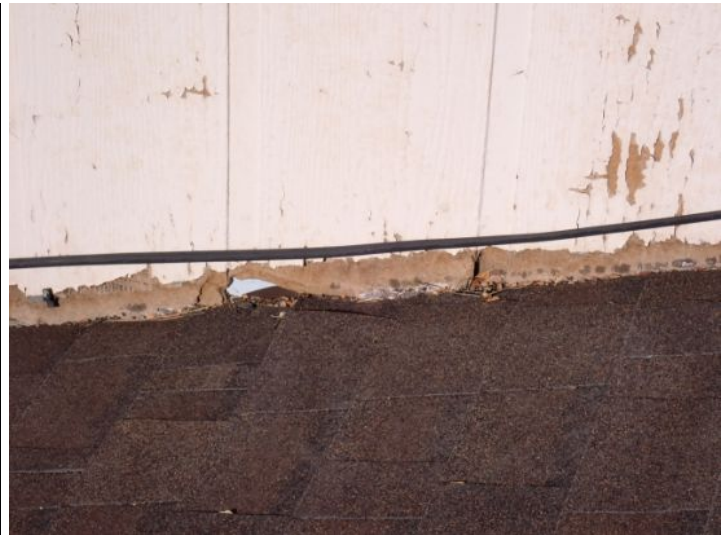
Siding material touching the roofing material in areas at the time of the inspection. Recommend repairs by a licensed contractor.
