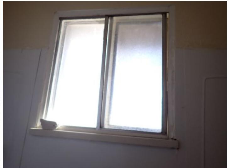
Missing safety stamps noted on the bathroom windows at the time of the inspection. While not required at the time of construction today's standards require any window located within 3 feet of a tub/shower surround be glazed with safety glass. Recommend repairs as needed by a licensed contractor.
