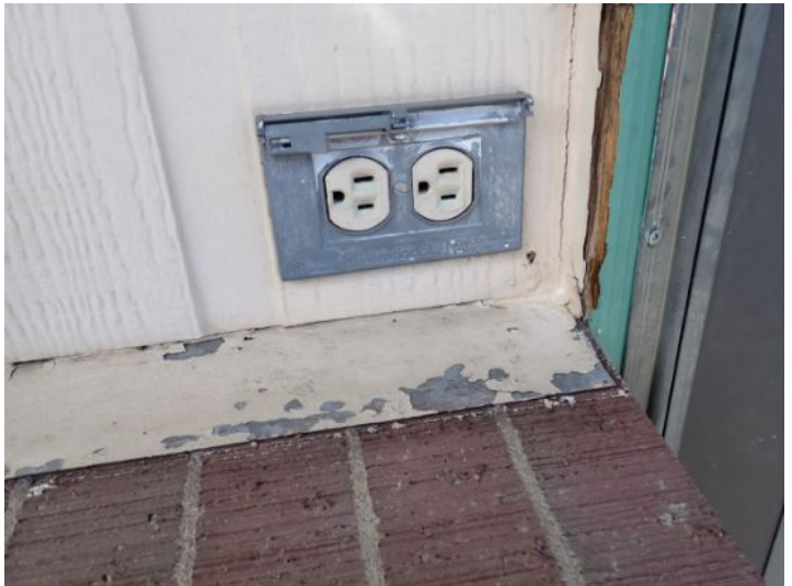
Exterior outlet missing weather cover. Recommend repairs.
