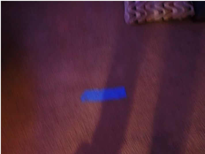
Unit 18: Carpet damage noted. Tub/shower surround requires caulk/grout repairs. Significant flooring deflection noted. Recommend repairs.
