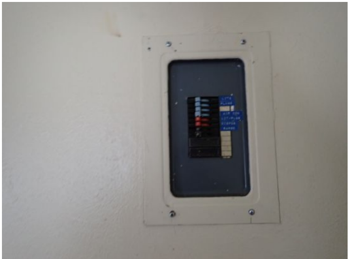
Unit 21: Missing cover plate noted on electrical panel. Wall damage noted in bathroom. Flooring damage noted. Tub spigot missing. Recommend repairs.
