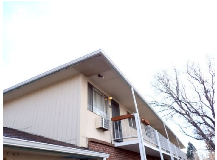
The majority of the exterior envelopes of the structures appeared to be in fair condition at the time of the inspection.
