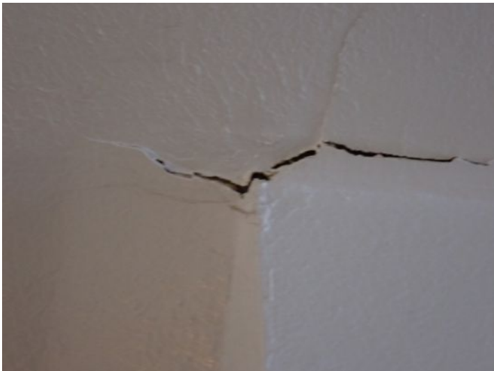
Unit 2: Tub/shower surround requires caulk/grout repairs. Significant ceiling cracking noted. Significant wall movement noted. Recommend repairs.
