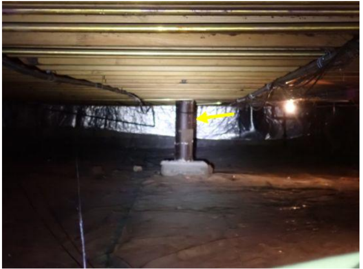
Leaning support posts noted in areas below the structures at the time of the inspection. Recommend repairs by a licensed contractor.
