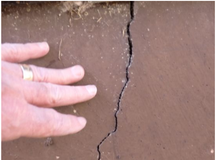
Significant foundation wall cracking noted on both structures at the time of the inspection. Recommend repairs by a licensed contractor.
