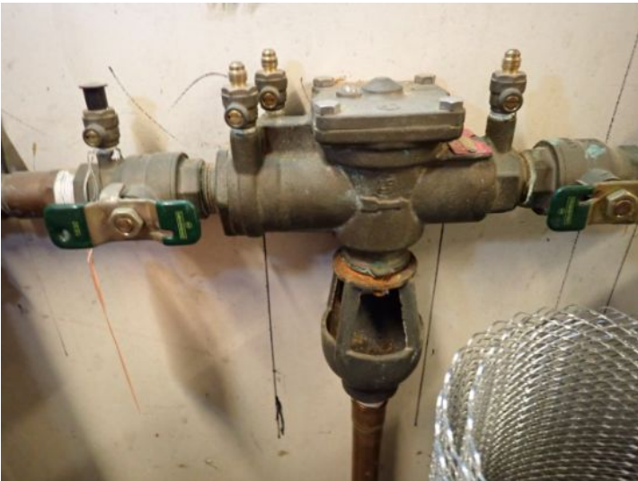
A backflow preventer was installed on the potable water supply lines for both structures at the time of the inspection.
