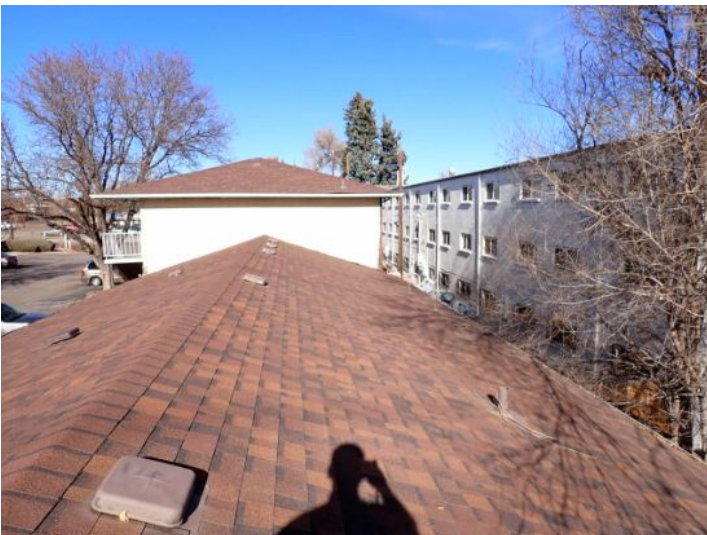
The majority of the roofing systems appeared to be in fair condition at the time of the inspection.
