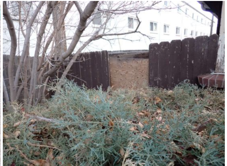
Fencing damage noted around the property at the time of the inspection. Recommend repairs by a licensed contractor.
