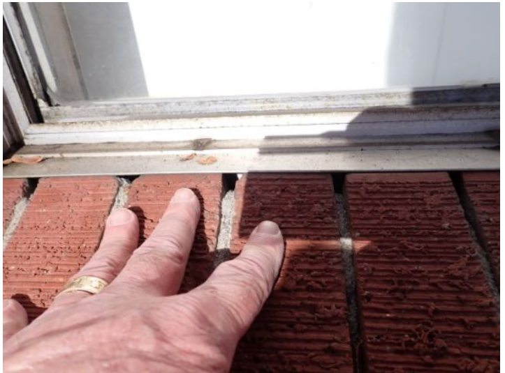
Tuck pointing required in areas. Recommend repairs by a licensed contractor.
