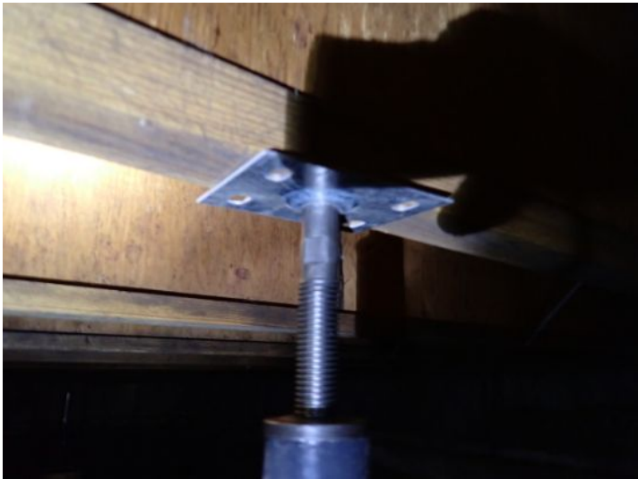
Due to the amount of structural movement, flooring deflection as well as improper/inadequate past repairs we recommend that both of the structures be evaluated by a licensed structural contractor prior to taking possession of the property.
