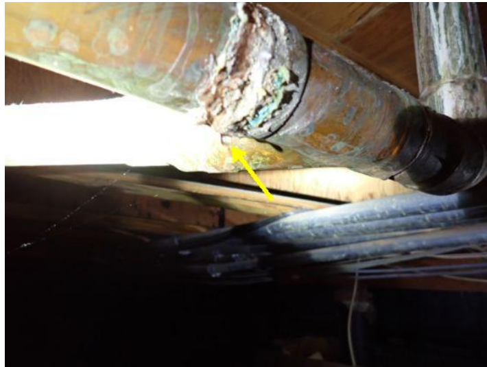
Minor leak noted on boiler piping in west side crawl space. Recommend repairs by a licensed contractor.
