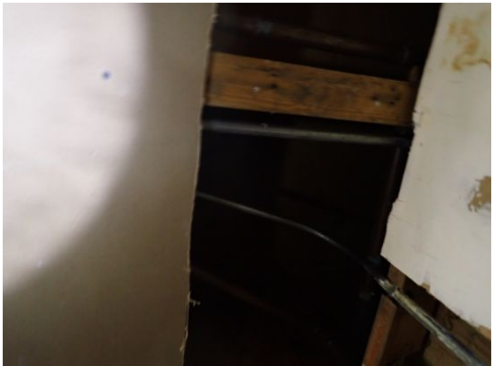
Damaged ceilings noted in boiler rooms at the time of the inspection. Fire Hazard. Recommend repairs by a licensed contractor.
