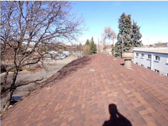
The majority of the roofing systems appeared to be in fair condition at the time of the inspection.
