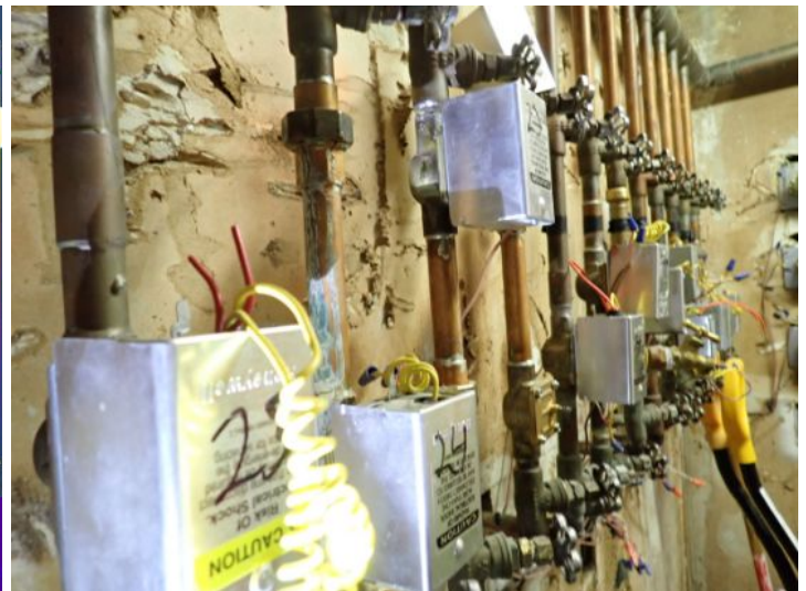
One or more zone valves did not appear to be functioning properly at the time of the inspection. Recommend repairs as needed by a licensed contractor.
