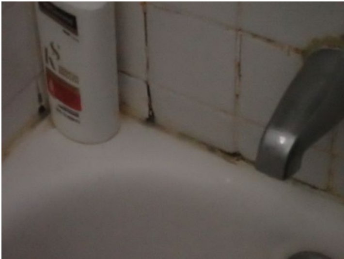
Unit 2: Tub/shower surround requires caulk/grout repairs. Significant ceiling cracking noted. Significant wall movement noted. Recommend repairs.
