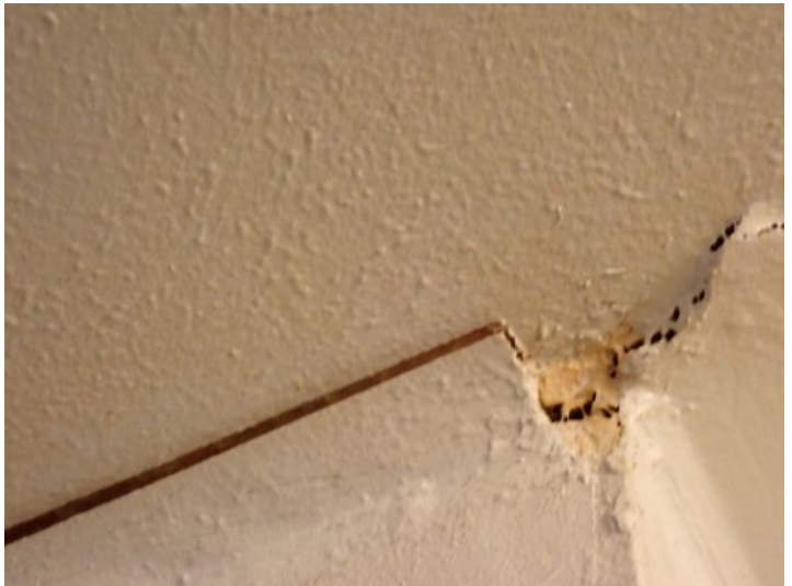
Unit 19: Significant wall movement and ceiling cracking noted. Recommend repairs.
