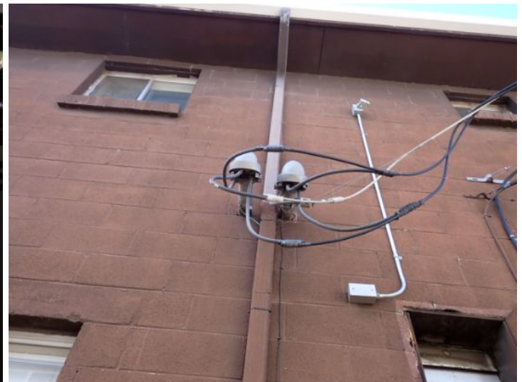
The main electrical system was a 1 phase 3 wire system
