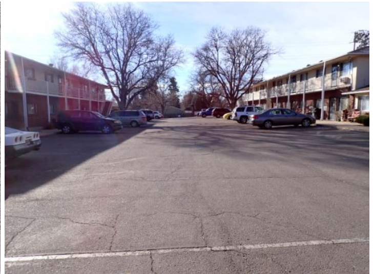
The parking lot surface was in fair condition at the time of the inspection.
