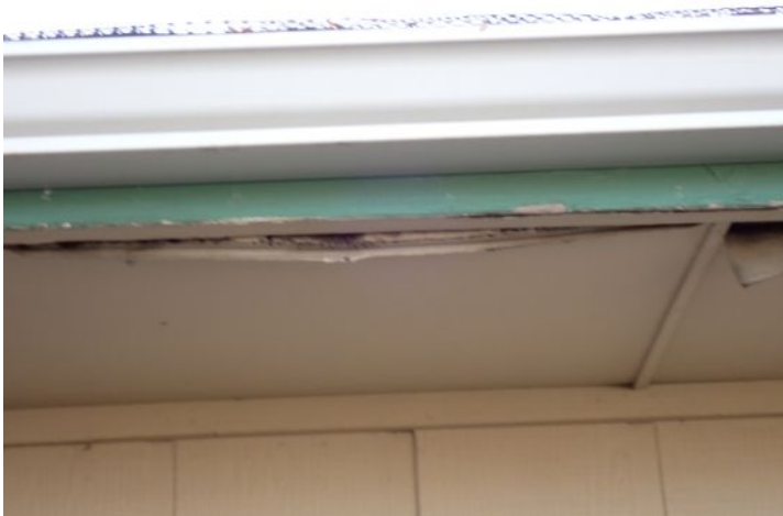
Moisture damaged soffit/eave material noted in areas around both of the structures at the time of the inspection. This was most likely caused by ice damming which was caused by inadequate attic insulation and ventilation. Recommend repairs as needed by a licensed contractor.
