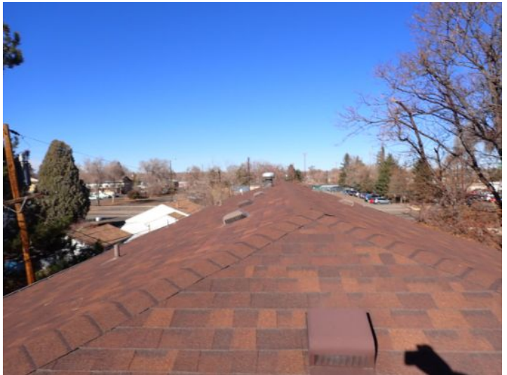
The majority of the roofing systems appeared to be in fair condition at the time of the inspection.
