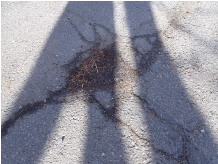
Significant deterioration noted in areas of the parking lots surface. Recommend repairs by a licensed contractor.
