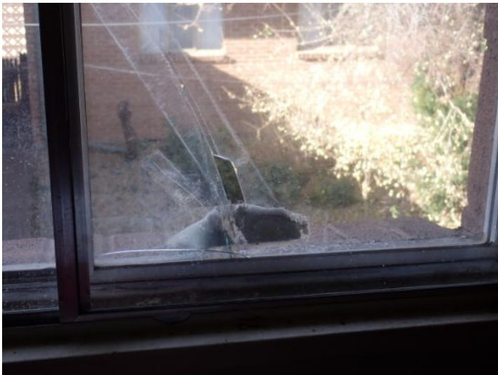
Unit 13: Cracked window glass. Broken window glass in rear of unit. Tub/shower surround requires caulk/grout repairs. Tub finish in poor condition. Closet door damage noted. Vinyl flooring damage noted. Recommend repairs.
