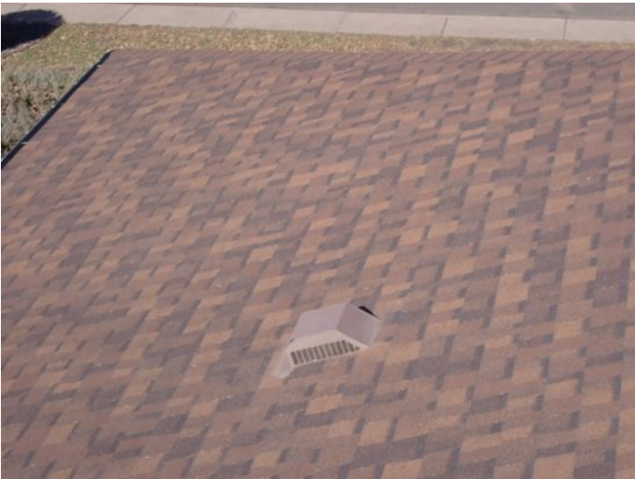
The majority of the roofing systems appeared to be in fair condition at the time of the inspection.
