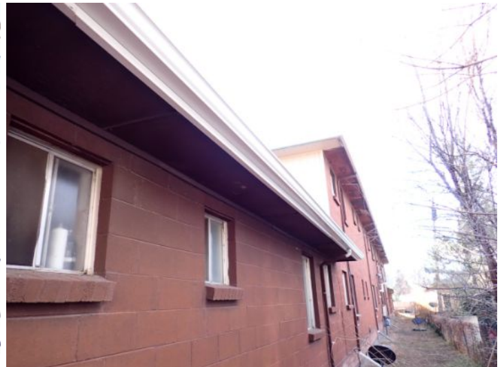
The majority of the exterior envelopes of the structures appeared to be in fair condition at the time of the inspection.
