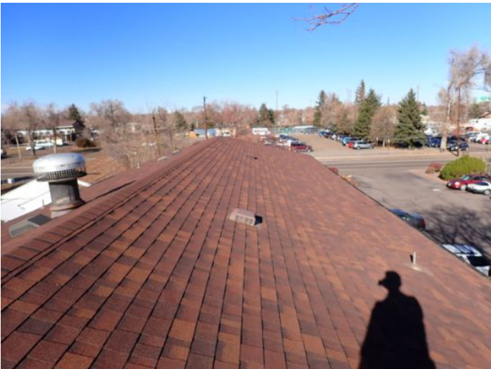
The majority of the roofing systems appeared to be in fair condition at the time of the inspection.
