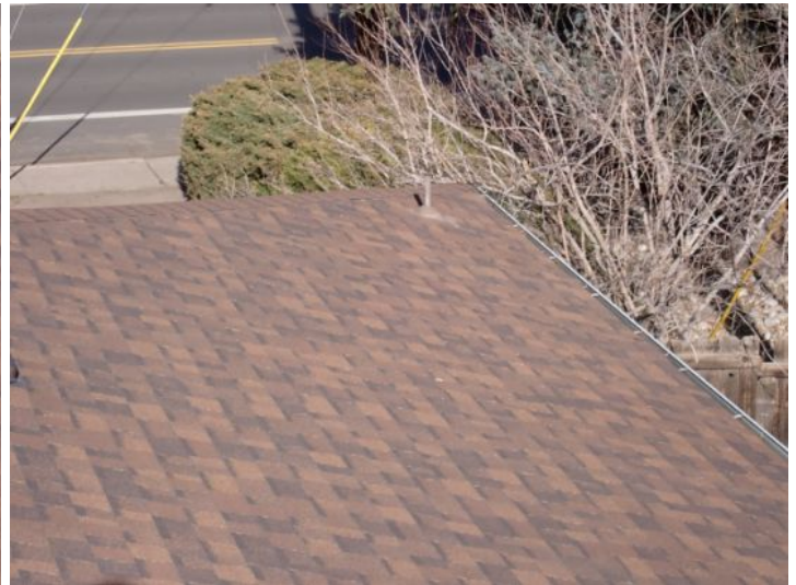
The majority of the roofing systems appeared to be in fair condition at the time of the inspection.
