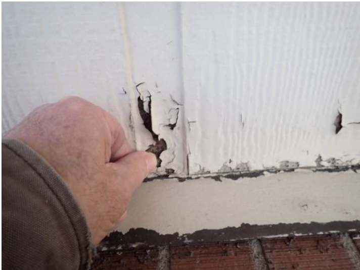
Wood rot/deterioration noted on the wood/composition siding in areas on both structures at the time of the inspection. Recommend repairs by a licensed contractor.
