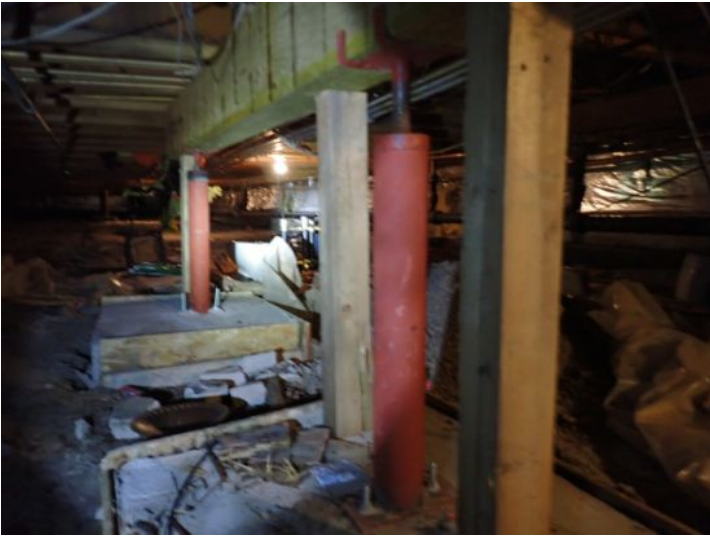
Due to the amount of structural movement, flooring deflection as well as improper/inadequate past repairs we recommend that both of the structures be evaluated by a licensed structural contractor prior to taking possession of the property.
