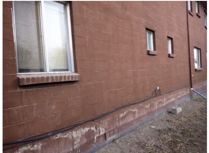
The majority of the exterior envelopes of the structures appeared to be in fair condition at the time of the inspection.
