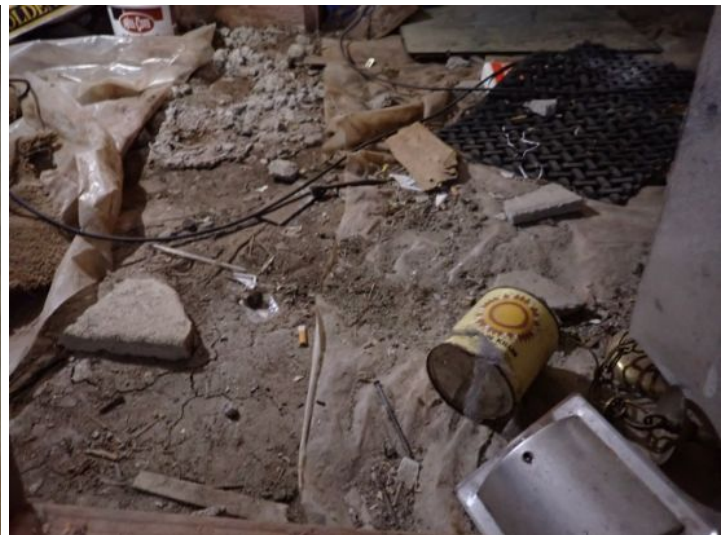
No vapor barrier noted in crawl spaces at the time of the inspection. Recommend repairs by a licensed contractor.
