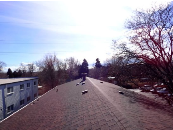
The majority of the roofing systems appeared to be in fair condition at the time of the inspection.
