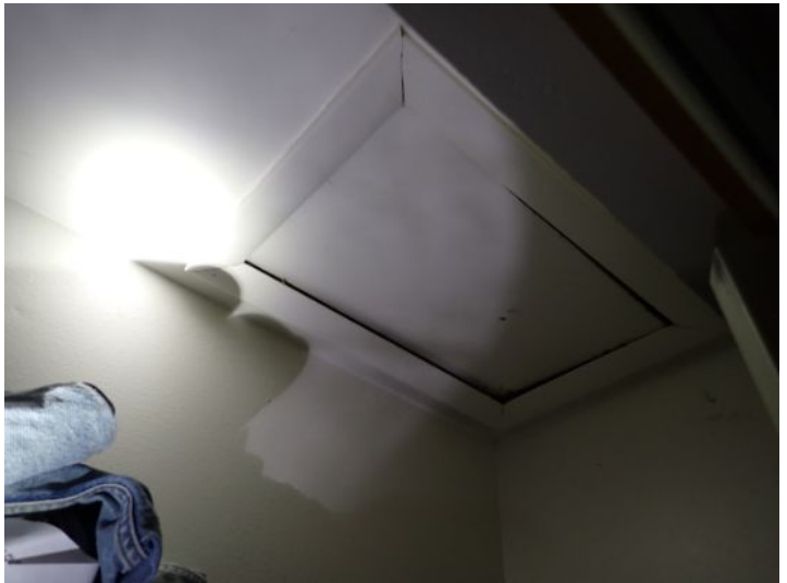
Some attic areas were not able to be viewed due to either the hatch systems being sealed shut or the inspector not being able to open the hatches for some reason.
