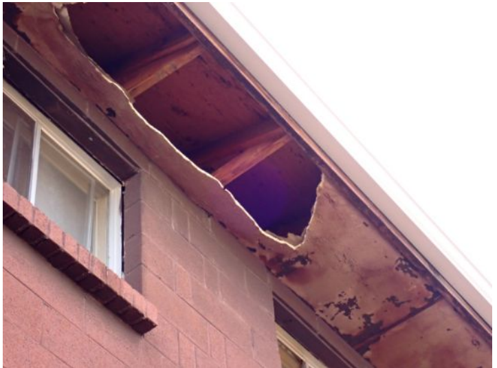
Moisture damaged soffit/eave material noted in areas around both of the structures at the time of the inspection. This was most likely caused by ice damming which was caused by inadequate attic insulation and ventilation. Recommend repairs as needed by a licensed contractor.
