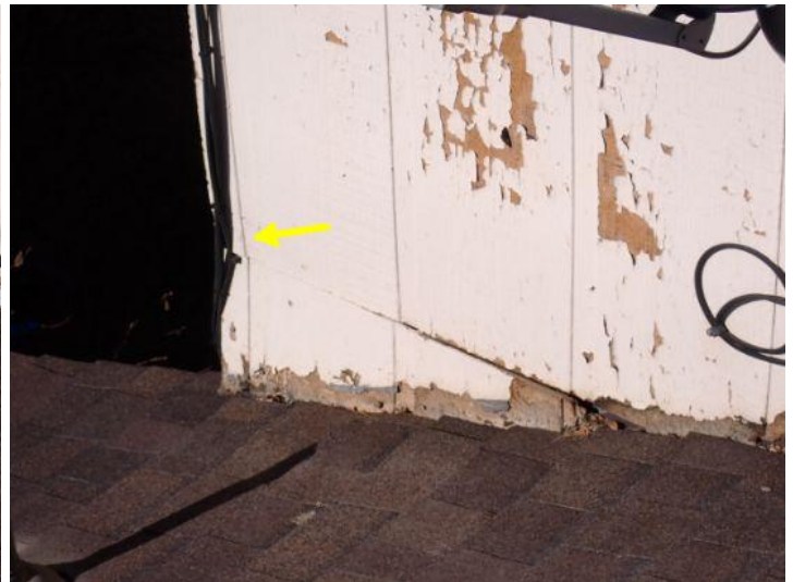
Missing/rotted/deteriorated wood trim noted in areas at the time of the inspection. Recommend repairs by a licensed contractor.
