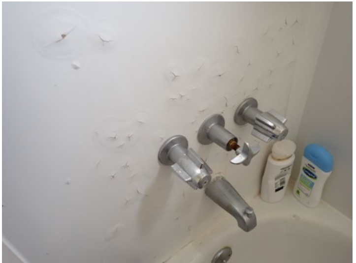
Unit 17: Tub/shower surround damage noted. Tub faucet damage. Recommend repairs.
