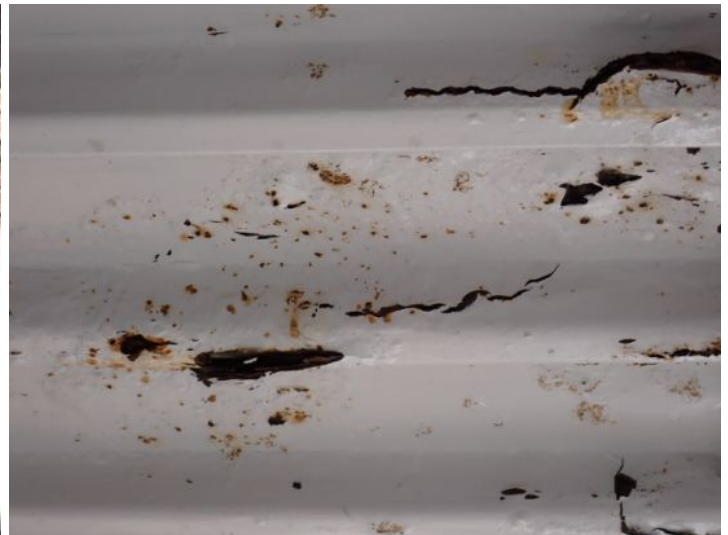
Pan rusting and deterioration noted below the upper level walkways and landings at the time of the inspection. Recommend repairs by a licensed contractor prior to taking possession of the property.
