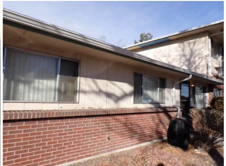
The majority of the exterior envelopes of the structures appeared to be in fair condition at the time of the inspection.
