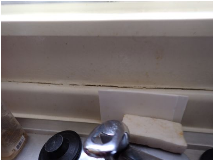
Unit 4: Kitchen counter and wall separation noted. Vanity sink rusting. Past moisture damage noted in bathroom wall but no moisture present at the time of the inspection. Recommend repairs.
