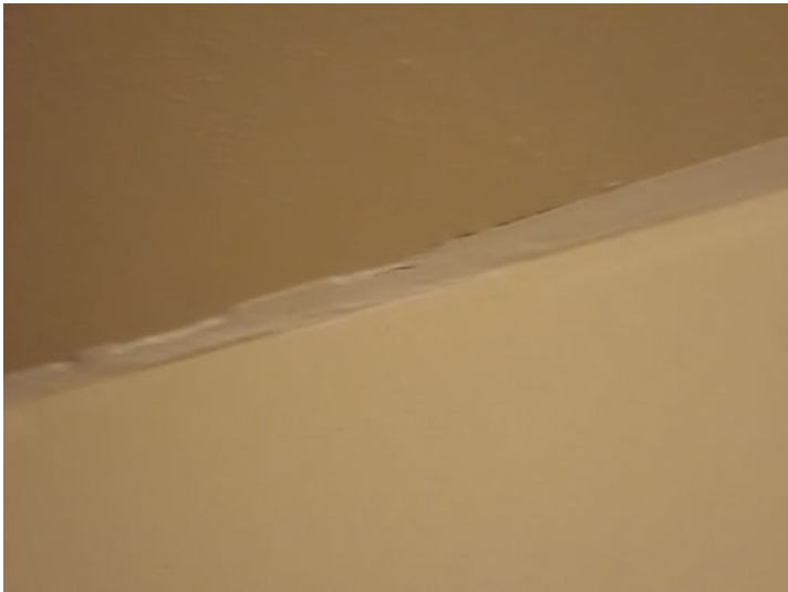
Unit 20: Damaged radiator system noted. Significant flooring deflection noted. Tub finish in poor condition. Significant wall movement noted. Recommend repairs.
