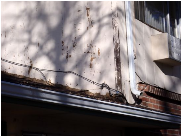
Peeling paint noted on the wood/composition siding material on both structures. Recommend repairs by a licensed contractor.
