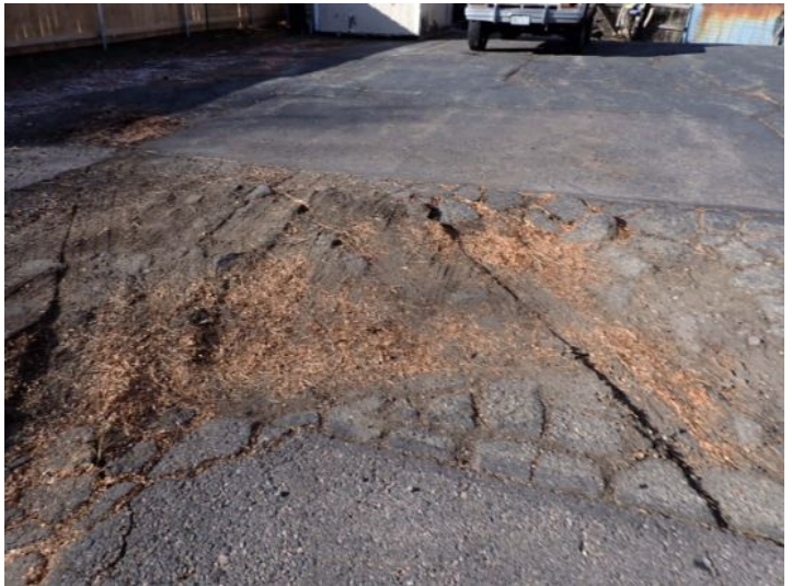
Significant deterioration noted in areas of the parking lots surface. Recommend repairs by a licensed contractor.
