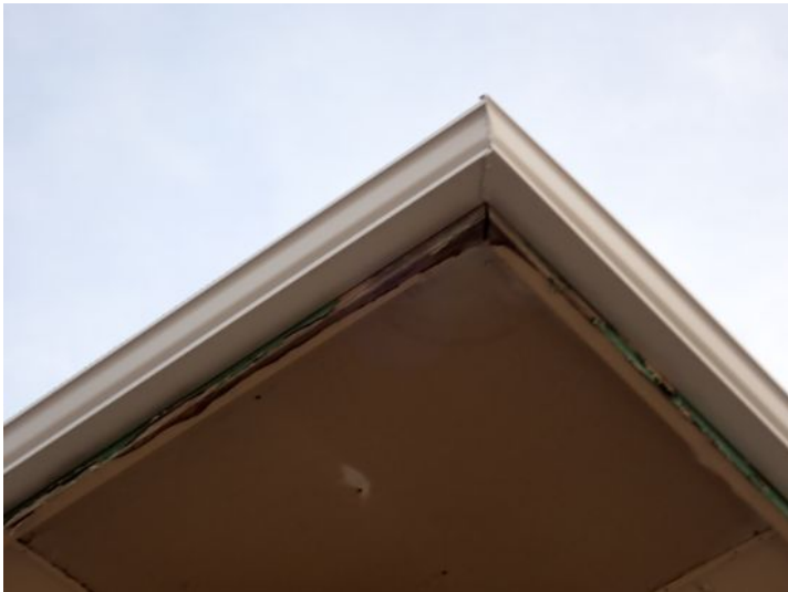
Moisture damaged fascia noted in areas. Recommend repairs by a licensed contractor.
