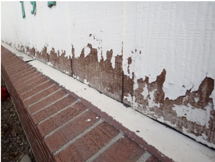
Peeling paint noted on the wood/composition siding material on both structures. Recommend repairs by a licensed contractor.
