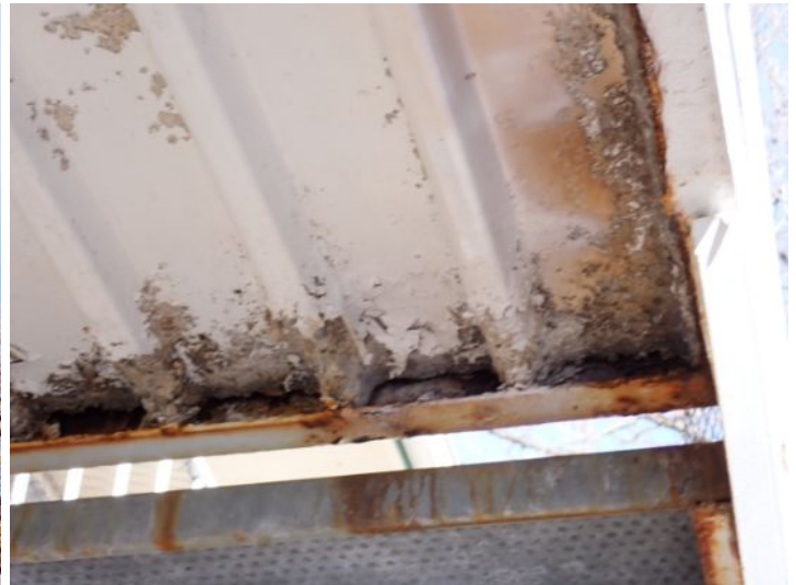
Pan rusting and deterioration noted below the upper level walkways and landings at the time of the inspection. Recommend repairs by a licensed contractor prior to taking possession of the property.
