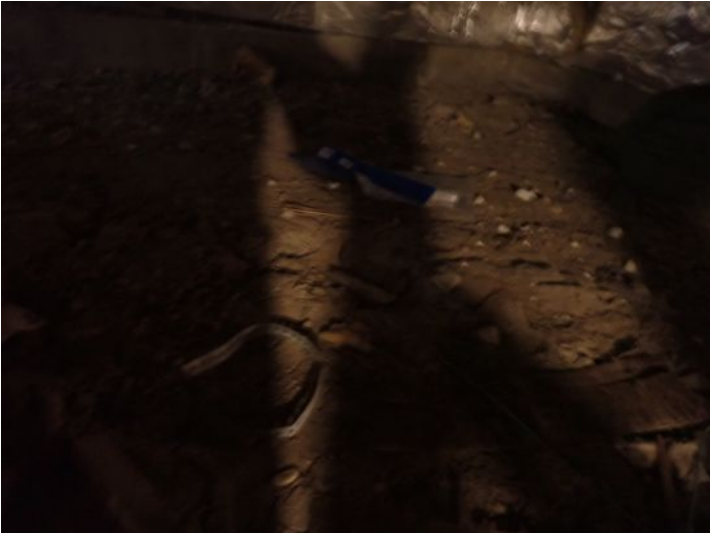
No vapor barrier noted in crawl spaces at the time of the inspection. Recommend repairs by a licensed contractor.
