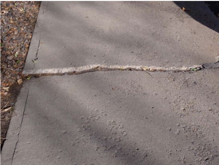
Significant cracking noted at the time of the inspection. Recommend repairs.
