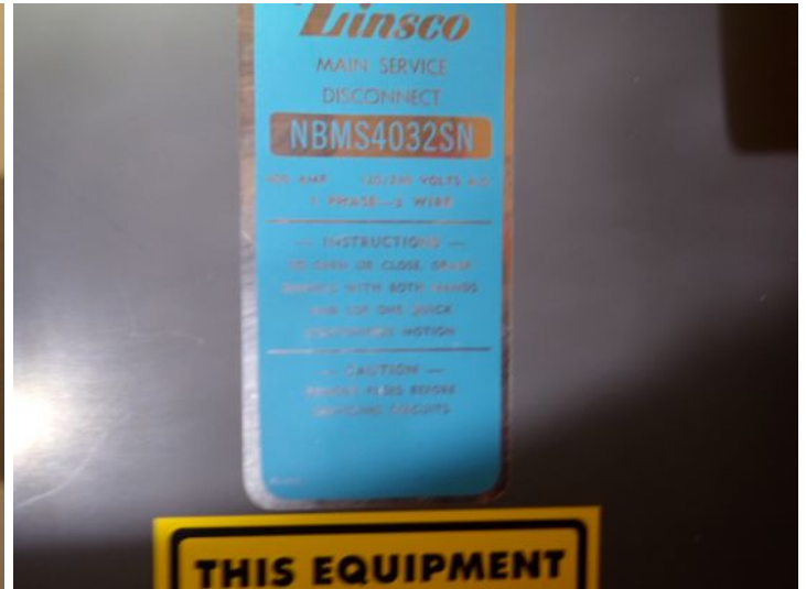
The main electrical disconnects appeared functional at the time of the inspection.
