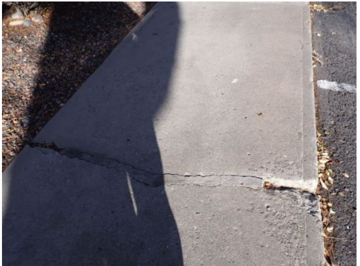
Trip hazards noted. Recommend repairs.
