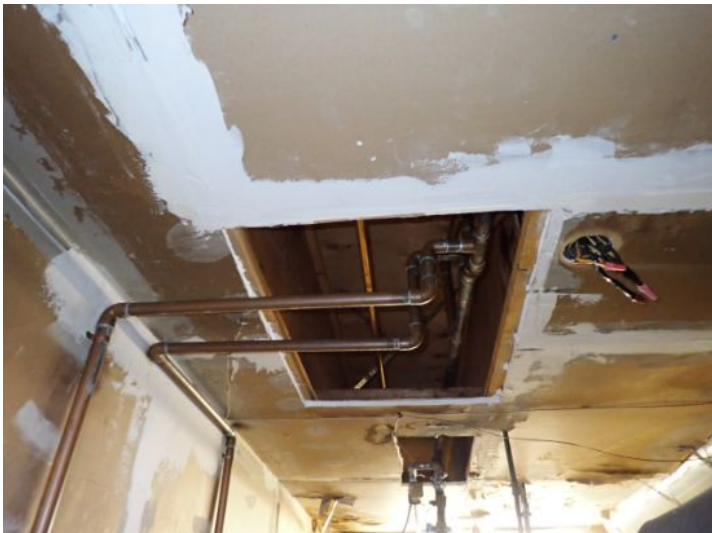
Damaged ceilings noted in boiler rooms at the time of the inspection. Fire Hazard. Recommend repairs by a licensed contractor.
