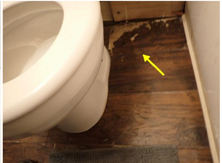
Unit 21: Missing cover plate noted on electrical panel. Wall damage noted in bathroom. Flooring damage noted. Tub spigot missing. Recommend repairs.
