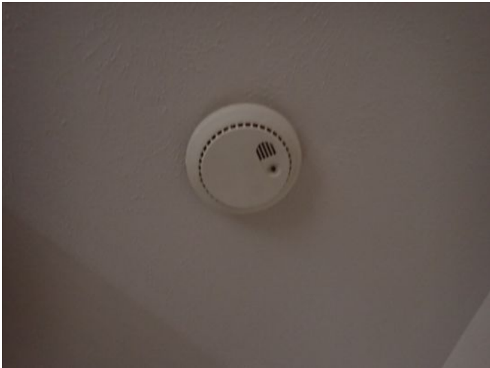
Recommend replacement of any/all smoke alarms and carbon monoxide detectors 10 years of age or older.
