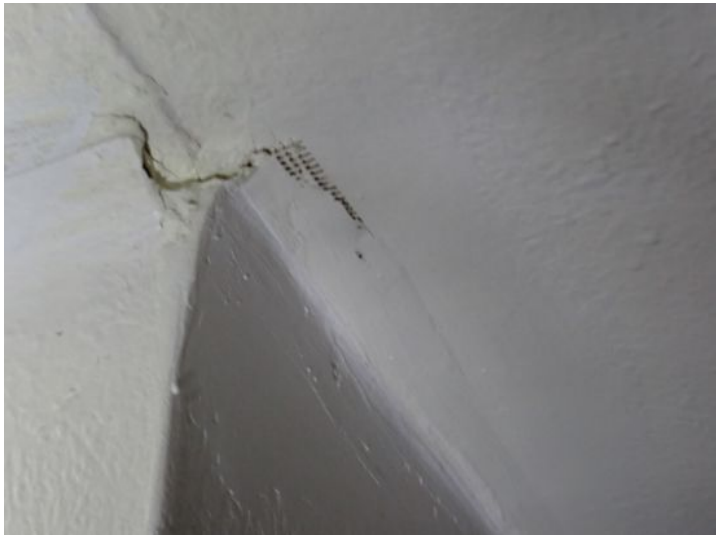
Unit 1: Significant floor deflection noted. Missing bedroom door. Significant wall/ceiling junction cracking noted. Carpet damage. Significant floor settling noted. Recommend repairs.
