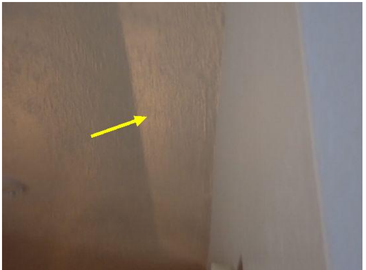
Unit 2: Tub/shower surround requires caulk/grout repairs. Significant ceiling cracking noted. Significant wall movement noted. Recommend repairs.
