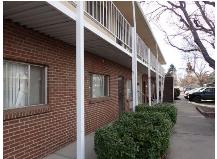
The majority of the exterior envelopes of the structures appeared to be in fair condition at the time of the inspection.
