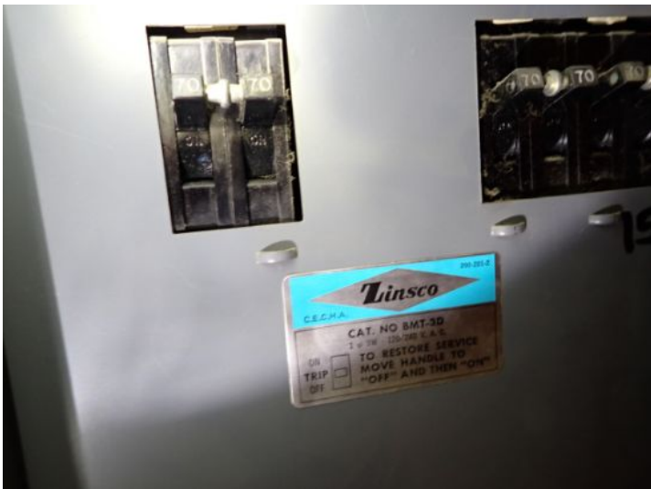
The tenant units appeared to have 70 amp main disconnect breakers located in the main electrical rooms.
