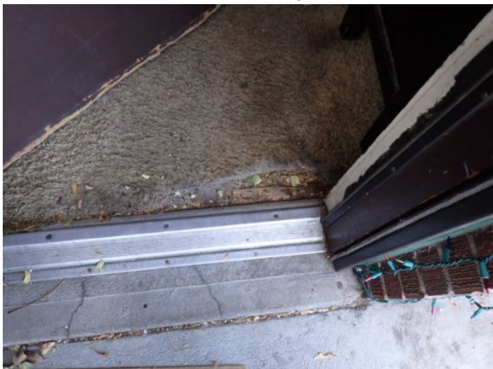
Unit 3: Carpet damage. Separation noted between kitchen counter and wall. Kitchen cabinet failure noted. Vinyl flooring damage. Tub/shower surround requires caulk/grout repairs. Bedroom closet door damage noted. Recommend repairs.
