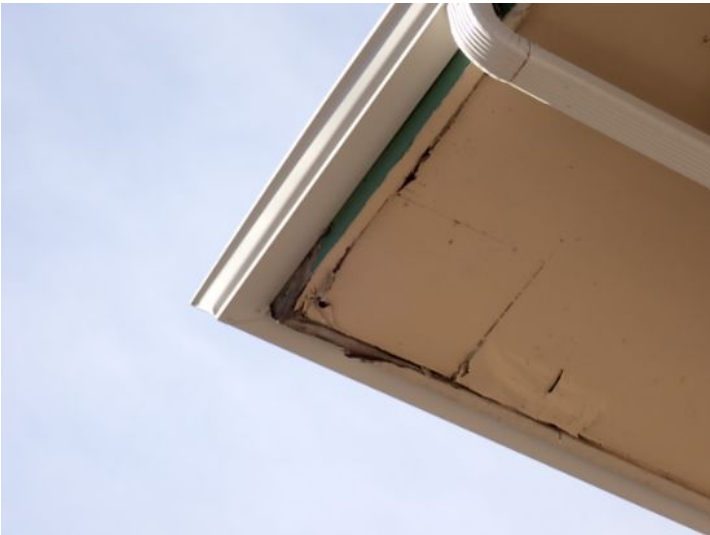
Moisture damaged soffit/eave material noted in areas around both of the structures at the time of the inspection. This was most likely caused by ice damming which was caused by inadequate attic insulation and ventilation. Recommend repairs as needed by a licensed contractor.
