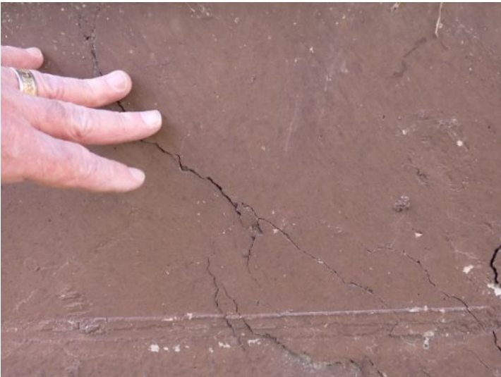
Minor foundation wall cracking noted in areas. Recommend monitoring for future repairs.
