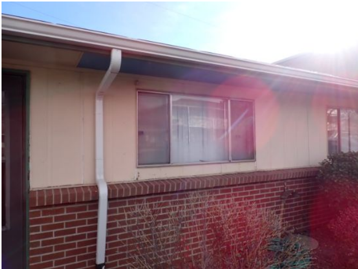
The majority of the exterior envelopes of the structures appeared to be in fair condition at the time of the inspection.
