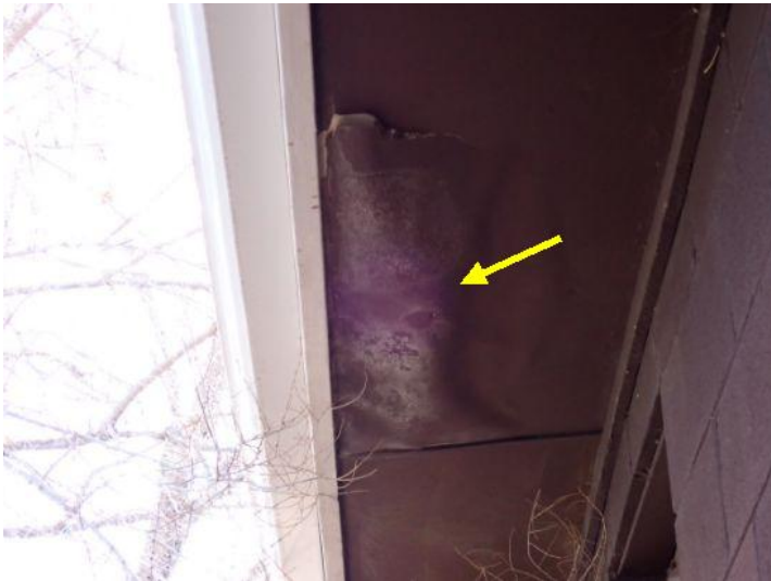
Moisture damaged soffit/eave material noted in areas around both of the structures at the time of the inspection. This was most likely caused by ice damming which was caused by inadequate attic insulation and ventilation. Recommend repairs as needed by a licensed contractor.
