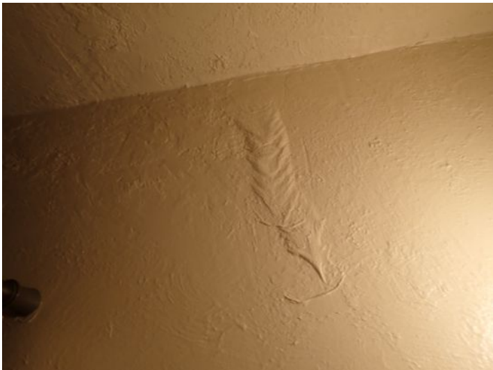
Unit 4: Kitchen counter and wall separation noted. Vanity sink rusting. Past moisture damage noted in bathroom wall but no moisture present at the time of the inspection. Recommend repairs.
