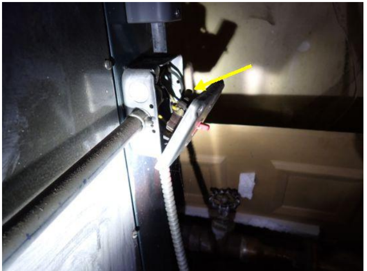
Exposed electrical wiring noted in areas. Recommend repairs by a licensed electrician.
