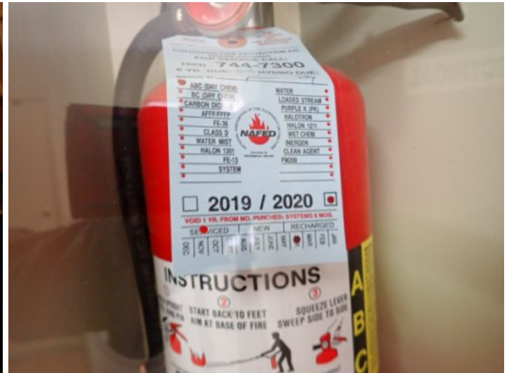
Last date of inspection/certification for the fire extinguishers was 4/20. These systems are required to be inspected/certified annually. Recommend repairs by a licensed contractor.
