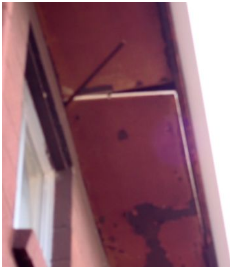
Moisture damaged soffit/eave material noted in areas around both of the structures at the time of the inspection. This was most likely caused by ice damming which was caused by inadequate attic insulation and ventilation. Recommend repairs as needed by a licensed contractor.
