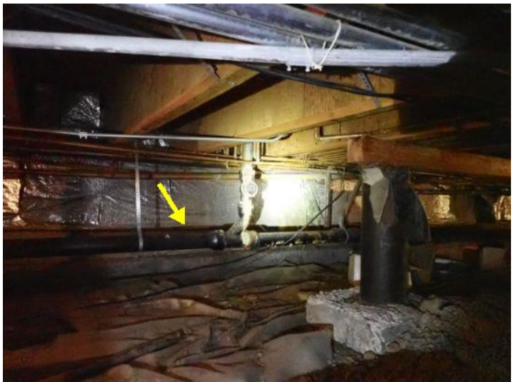
Improper slope noted in the sewer line below the east side structure at the time of the inspection. Recommend repairs as needed by a licensed contractor.
