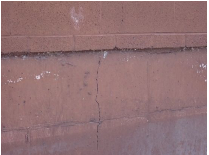
Minor foundation wall cracking noted in areas. Recommend monitoring for future repairs.
