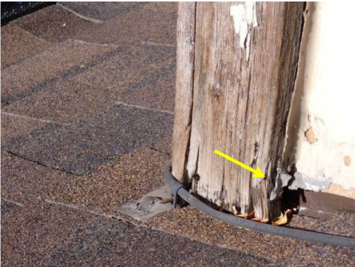
Missing kickout flashing noted in areas on the lower level roofing systems. Recommend repairs by a licensed contractor.
