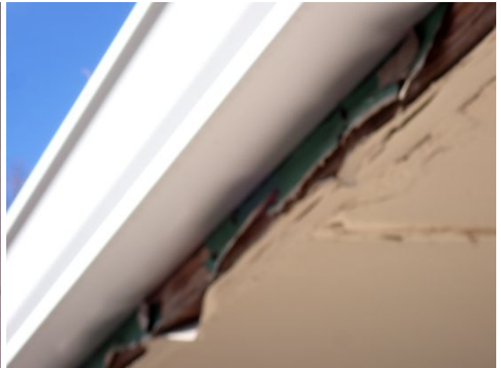
Moisture damaged fascia noted in areas. Recommend repairs by a licensed contractor.
