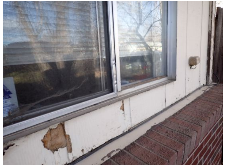
Peeling paint noted on the wood/composition siding material on both structures. Recommend repairs by a licensed contractor.
