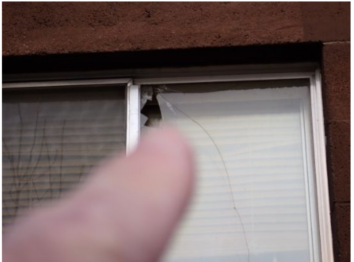
Cracked/broken window glass noted in areas. Recommend repairs by a licensed contractor.
