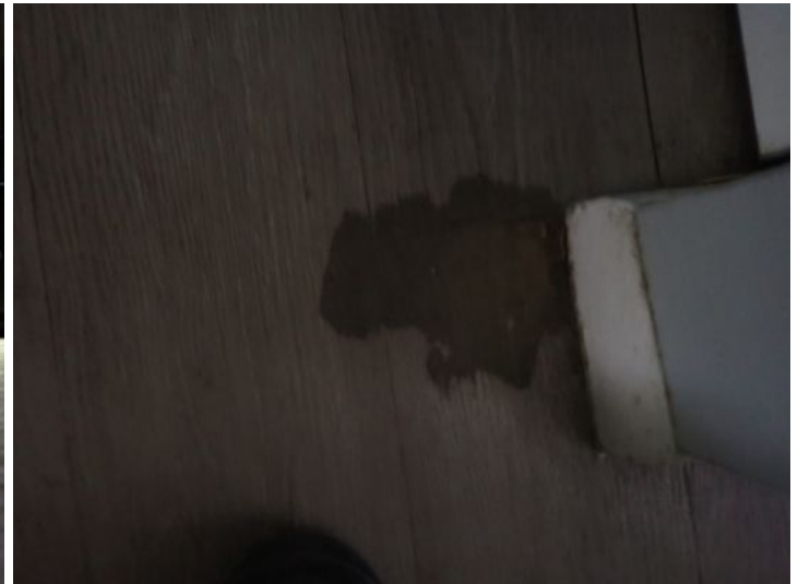
Unit 11: Front door trim damaged. Significant flooring deflection. Flooring damage noted. Recommend repairs.
