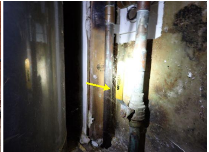
The main water shut off valves were functional at the time of the inspection.
