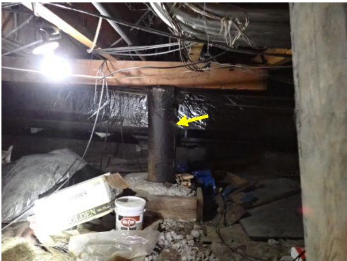
Leaning support posts noted in areas below the structures at the time of the inspection. Recommend repairs by a licensed contractor.
